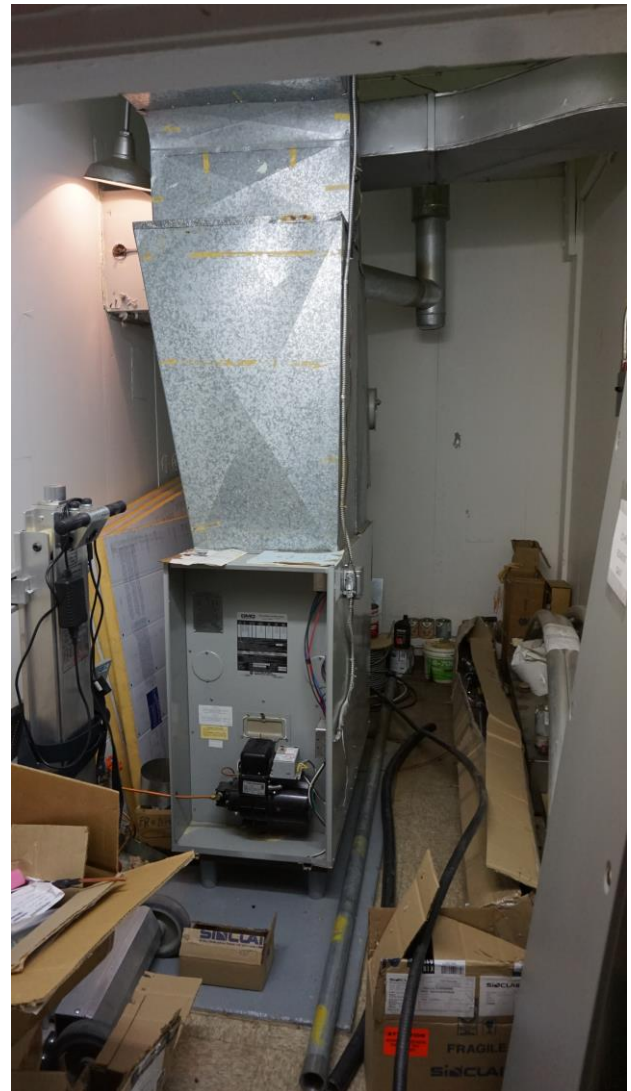
Figure 11: HVAC room Note, furnace has been removed.
