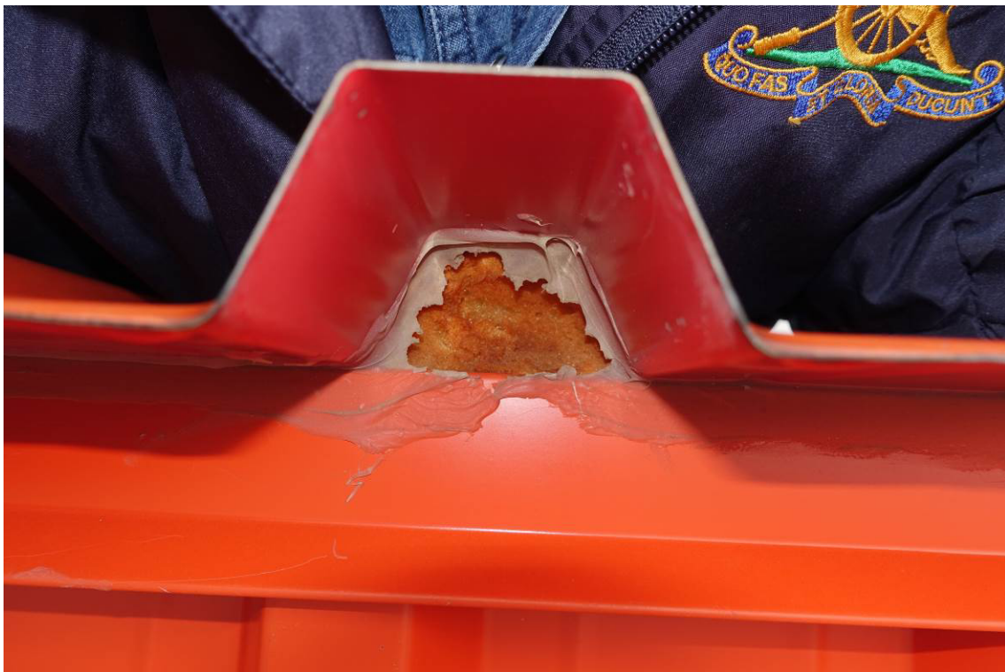
Photograph 4. View of deteriorating sealant and insulation in flute opening of roof.
