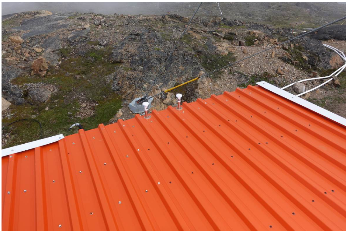
Photograph 2. View of the northeast corner of metal batten roof with flashing removed.
