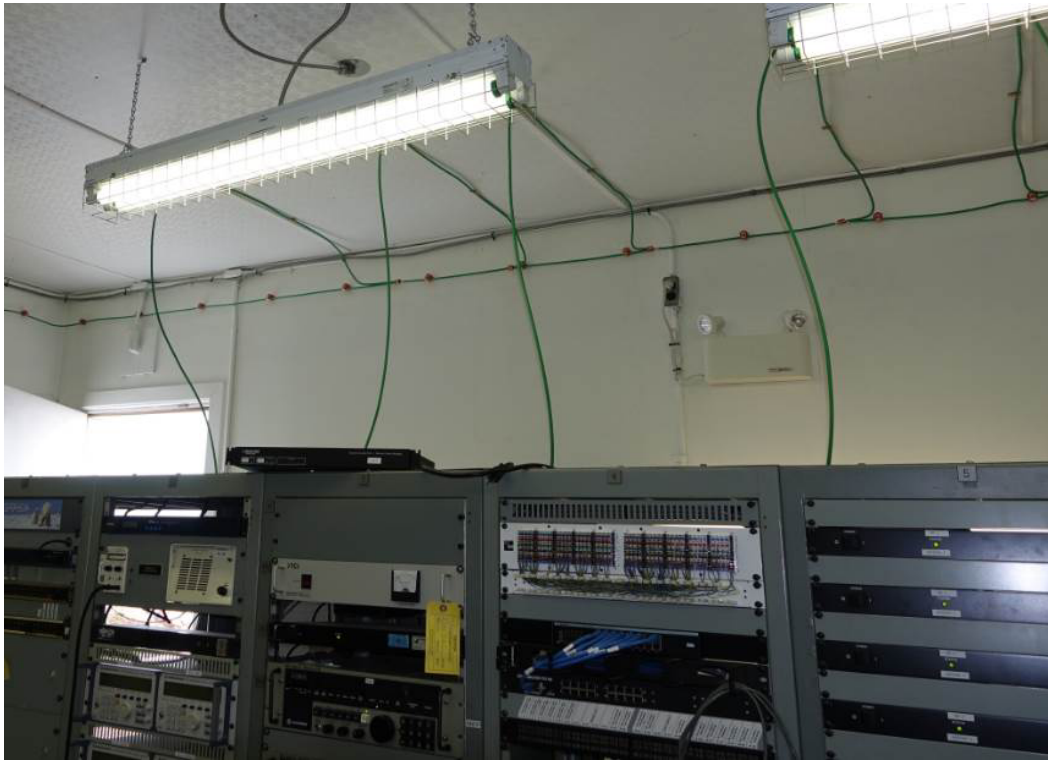
Photograph 11. View of the generator room showing emergency lighting and fluorescent light tubes with potentially PCB containing ballasts.
