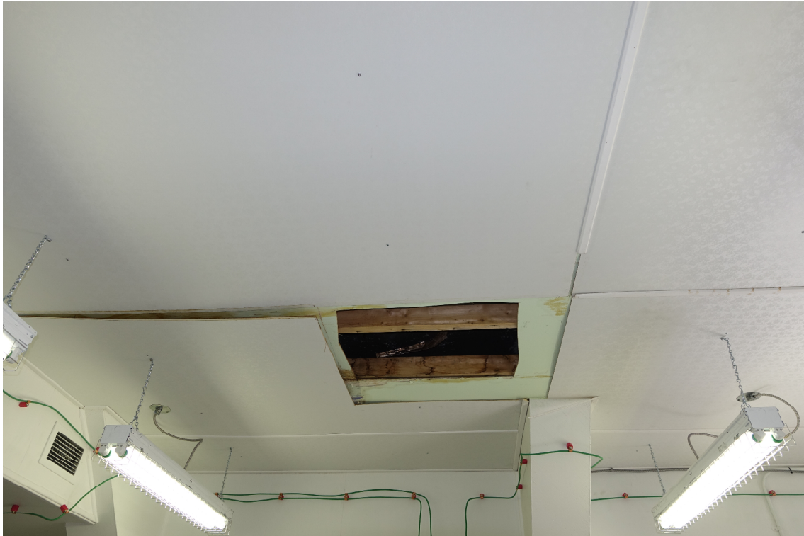
Photograph 3. View of test cut opening in the ceiling of the Radio room.
