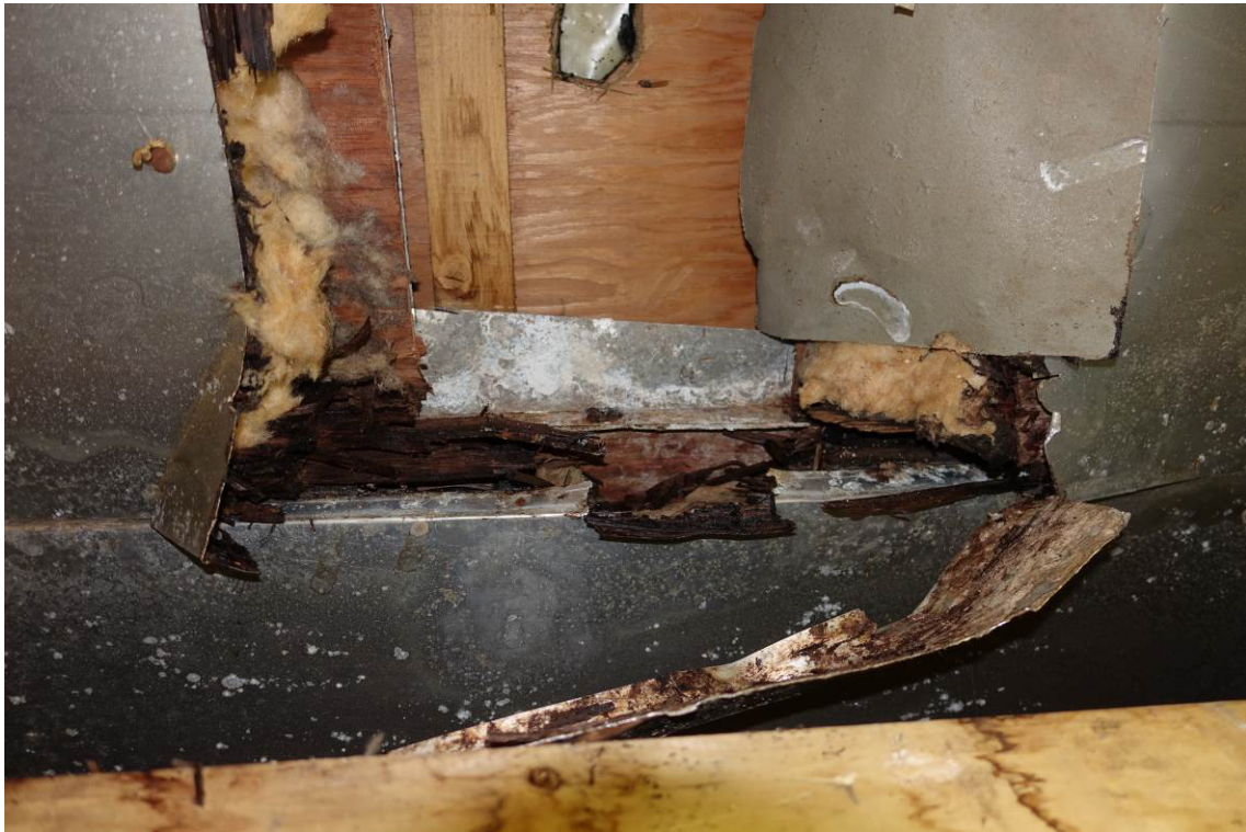
Photograph 9. View of rotted wood and mould-contamination in the attic space.
