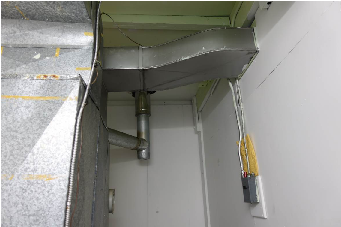
Photograph 10. Asbestos-containing cement board walls in the furnace room.
