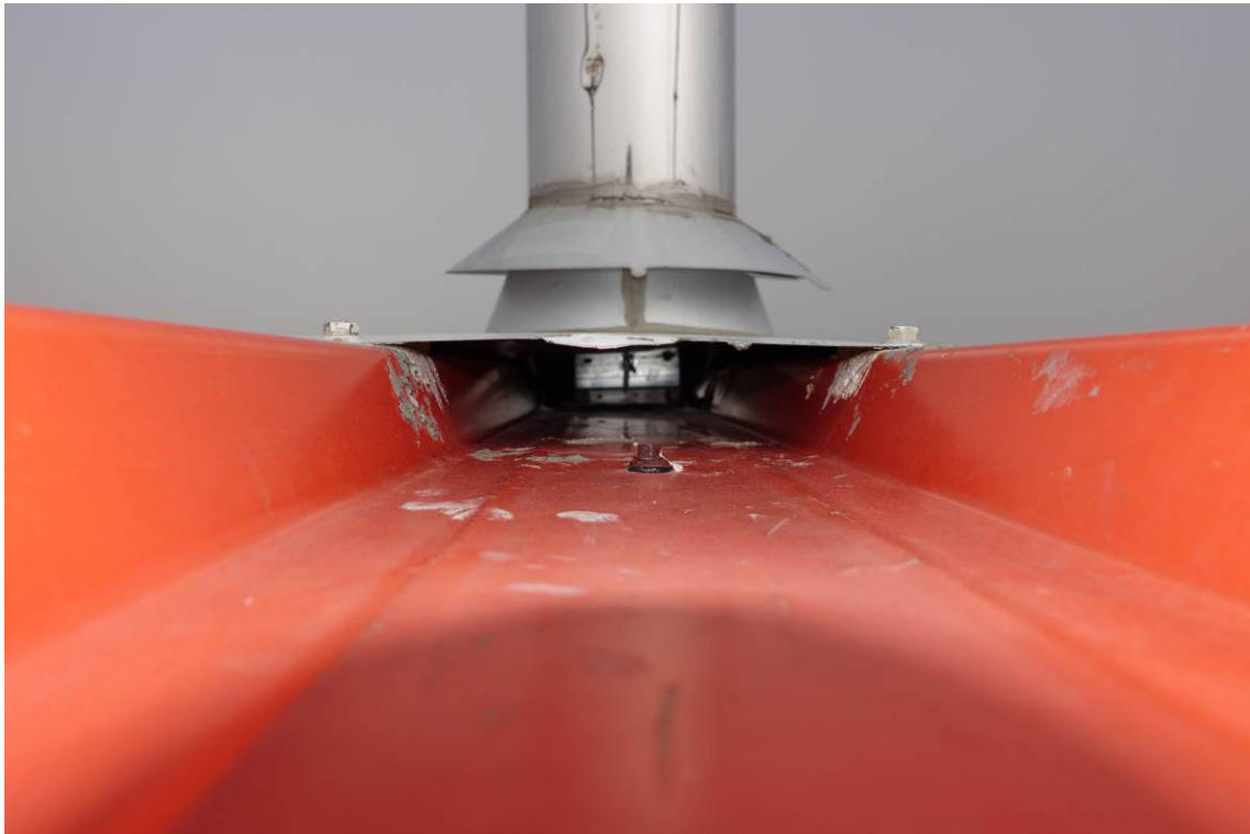
Photograph 5. View of the base of flue vent showing underlying cavity.
