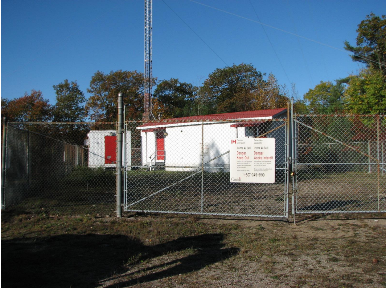
Figure 5: Operational radio equipment building [Right]. Old Generator Building [Left] (To be demolished at start of project)
