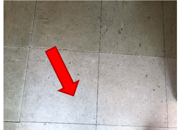
Pink 12" x 12" vinyl tile (S-007AC) contain chrysotile asbestos.
