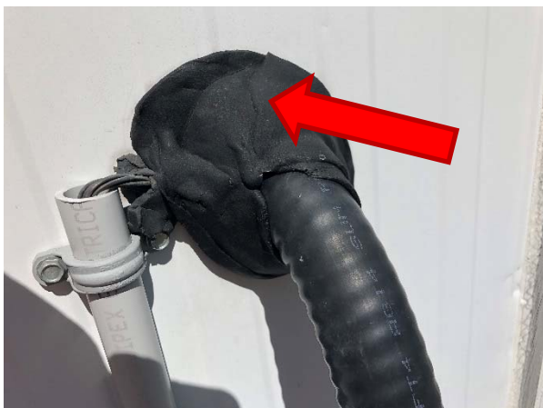
Black putty around wiring on the exterior of the trailer unit building (S-008A-C) does not contain asbestos.
