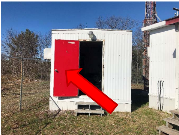
Red paint on the exterior doors (LP-01) contains 2.37% lead.
