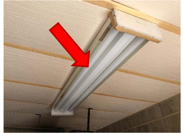
Fluorescent light tubes present throughout the Site contain mercury gas.
