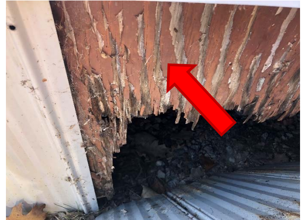
Brown paint on exterior trailer skirting beneath steel cladding (LP-04) contains 0.14% lead.
