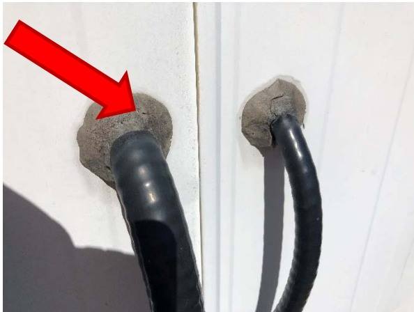
Grey caulking around wiring on the exterior of the trailer unit building (PCB-03) does not contain PCBs.
