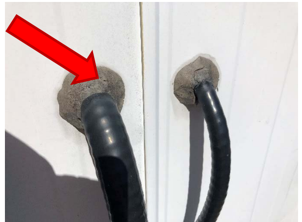
Grey caulking around wiring on the exterior of the trailer unit building (S-003A-C) does not contain asbestos.
