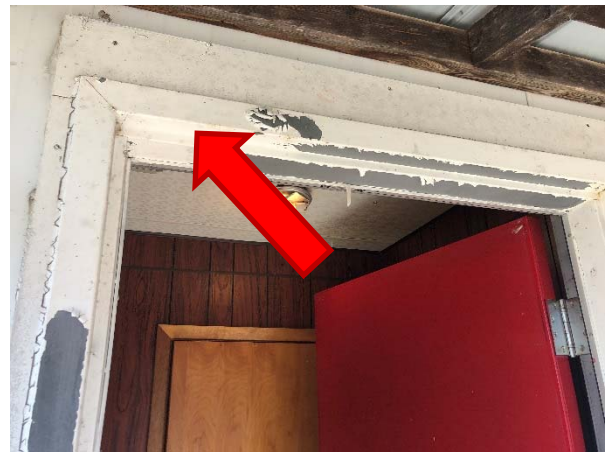
White paint on door trim on the exterior doors (LP-02) contains lead.
