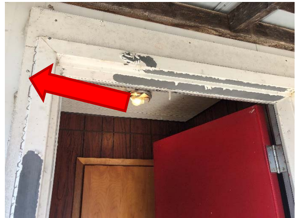
White caulking around doors on the exterior of the trailer unit building (PCB-02) does not contain PCBs.
