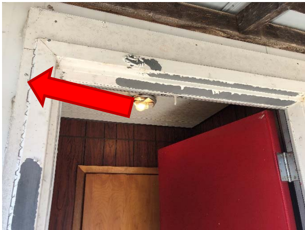
White caulking around doors on the exterior of the trailer unit building (S-002A-C) does not contain asbestos.
