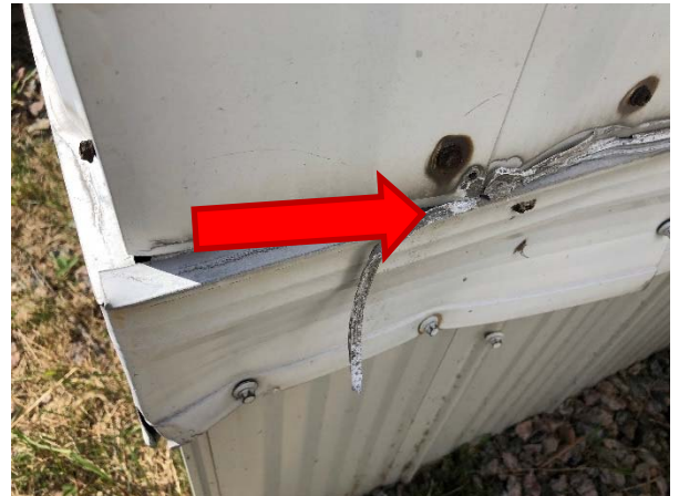
Silicone caulking around the base of steel exterior panels on the shed building. Known to not contain asbestos.
