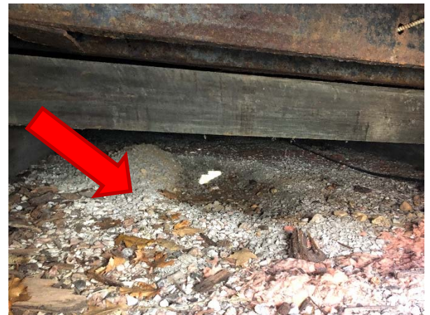
Gravel used for timber foundation contains silica.
