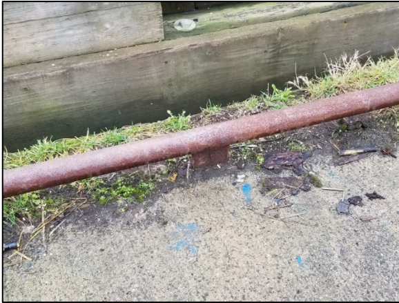
Image 7. Steel pipe bull rail welded to steel deck plates set into concrete deck.
