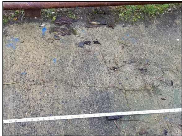
Image 10. Typical cracking observed on the surface of the concrete deck.
