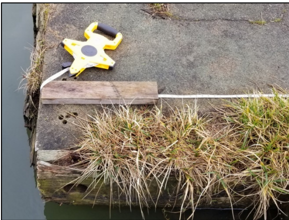
Image 9. Heavy fungal damage in fascia.
