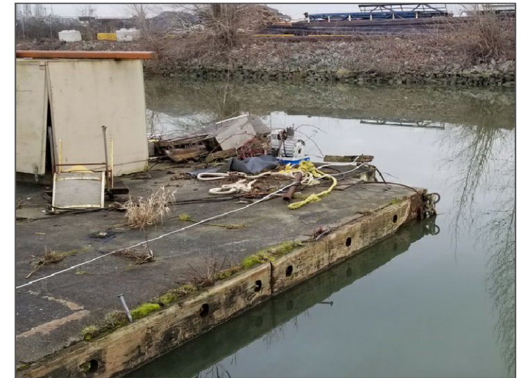
Photo 8. Looking at bow port corner along bow fascia. Note debris collected on float.
