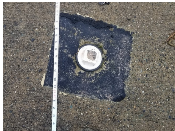
Image 6. Deck bung with removable plastic cap and internal sleeve set into concrete deck.
