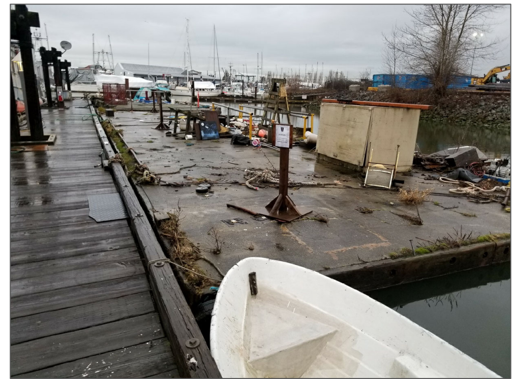
Photo 1. Looking from the bow towards the stern of the concrete float. Note debris collected on float.
