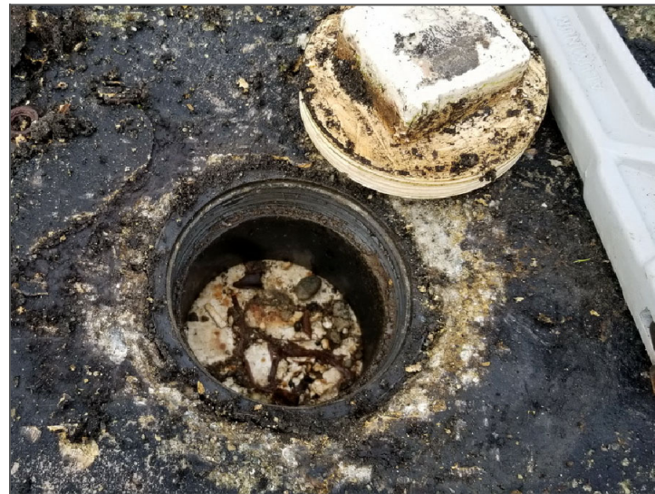
Photo 6. Plastic bung opened to reveal internal Styrofoam used to fill the internal hull of the float.
