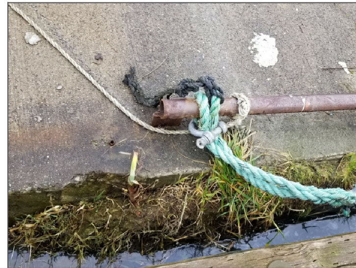
Photo 7. Broken steel pipe bull rail. Note bull rail welded to steel flat bar stand-offs protruding from concrete deck.
