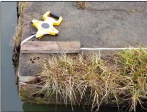
Image 9. Heavy fungal damage in fascia.
