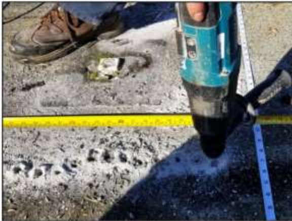
Image 3. Test holes drilled to determine location of bulkhead walls below the concrete deck.
