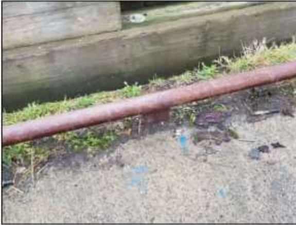
Image 7. Steel pipe bull rail welded to steel deck plates set into concrete deck.
