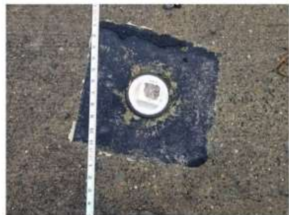
Image 6. Deck bung with removeable plastic cap and internal sleeve set into concrete deck.
