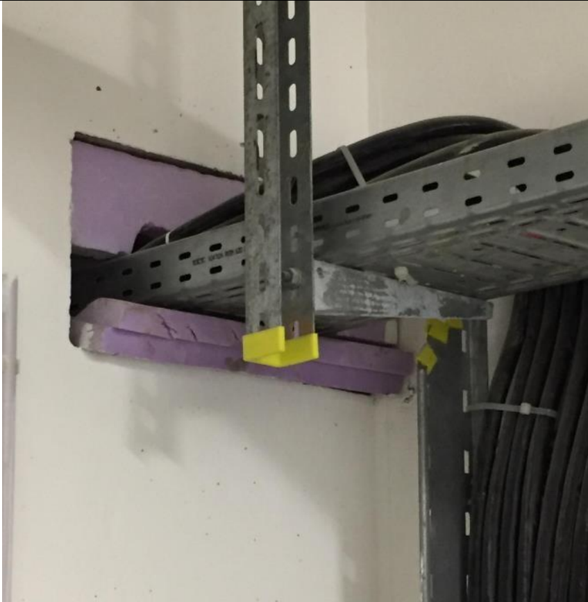
Fire stopping attempted with fire rated plasterboard, however no fire seal achieved.
