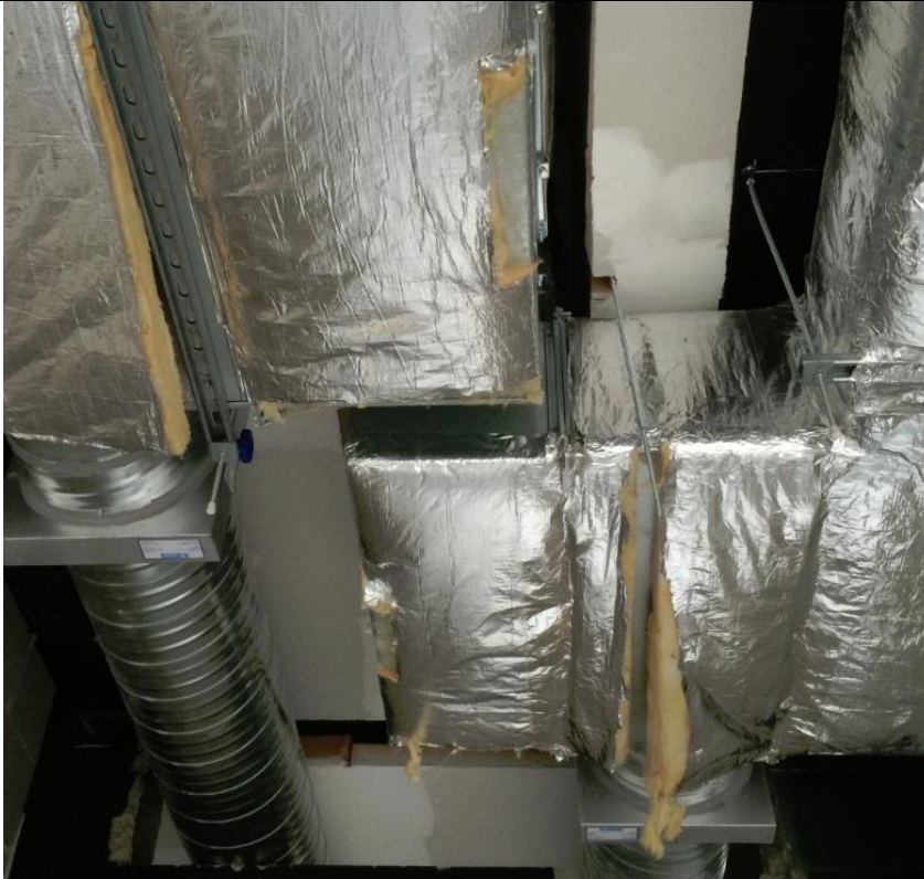
Inadequate insulation installation.
