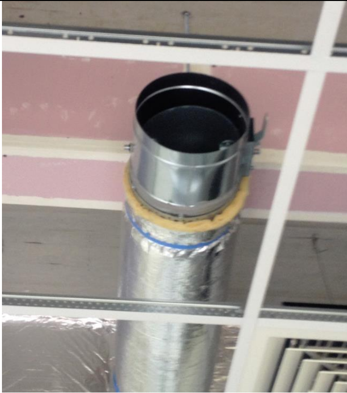
Ductwork open-ended during the construction period.
