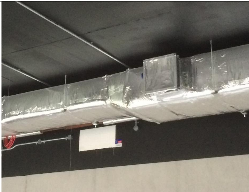
Insulation to have complete coverage and be vapour sealed. Thermal bridge between the ductwork support and the duct must also be separated – insulation must be installed between the duct and support.
