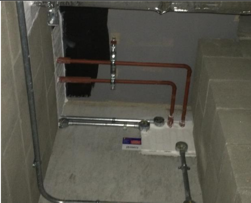
Fire stopping completely sealing up opening, and pipework sleeves installed to protect pipework.
