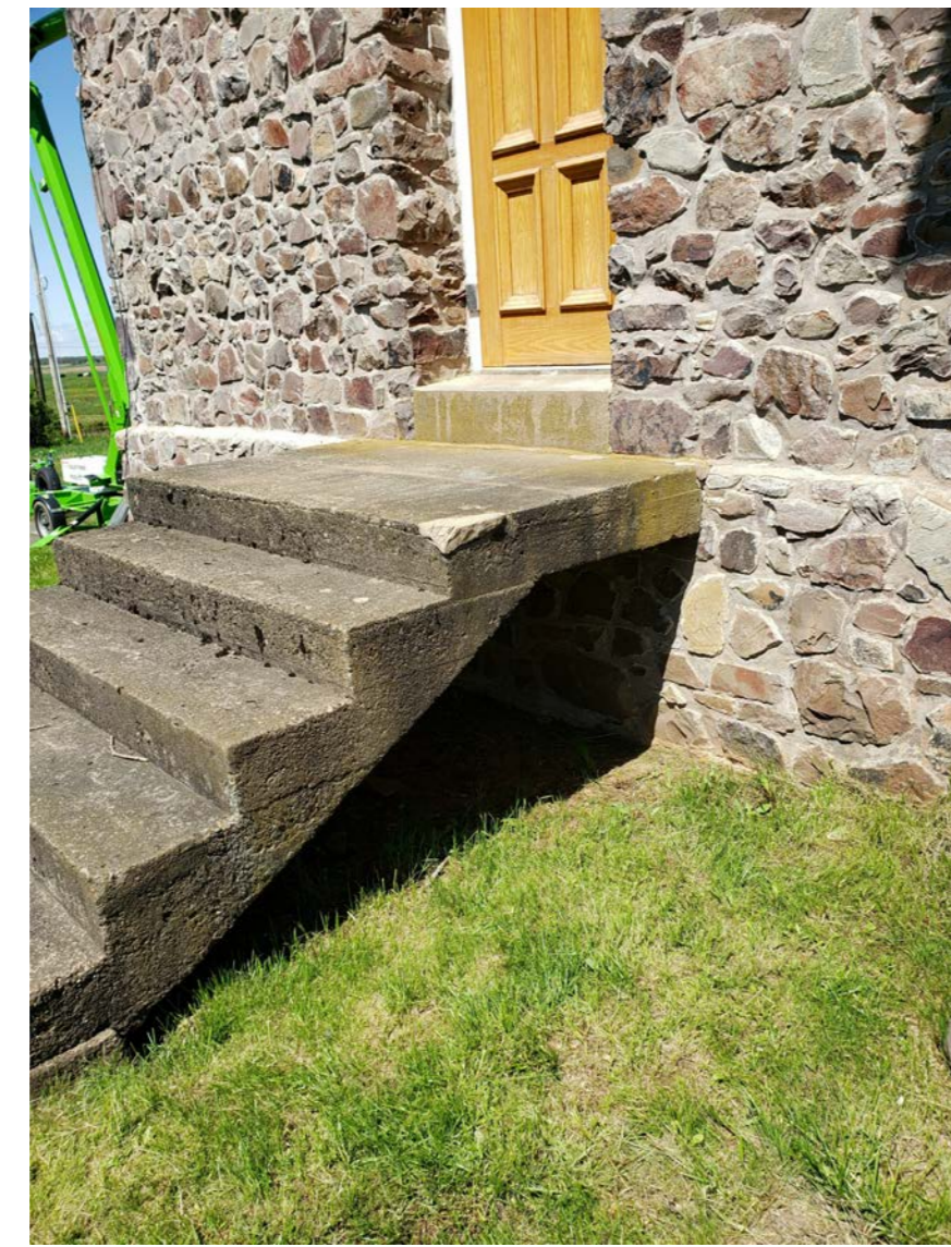
W2 PREVIOUS CONCRETE REPAIR AND ORGANIC GROWTH ON CONCRETE STAIR AND SILL
