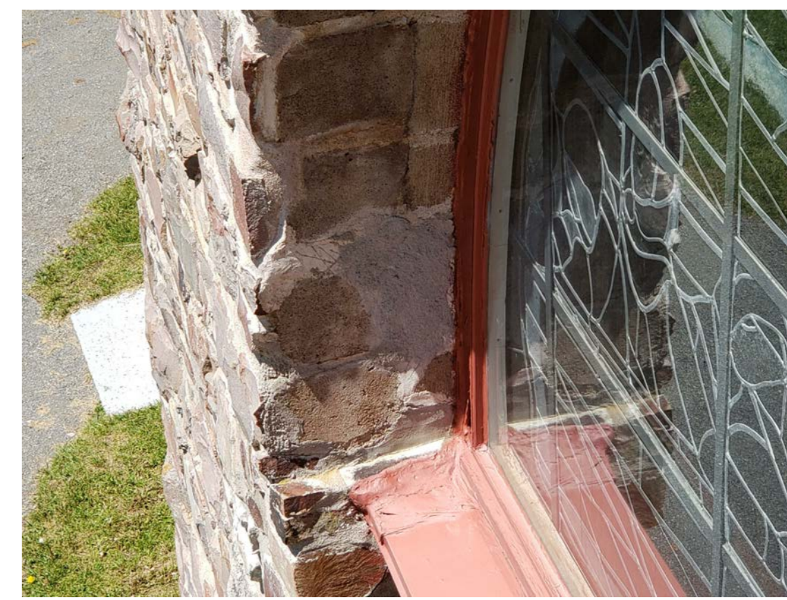
S6 PREVIOUS PATCH REPAIR OF CONCRETE BLOCK ARCH
