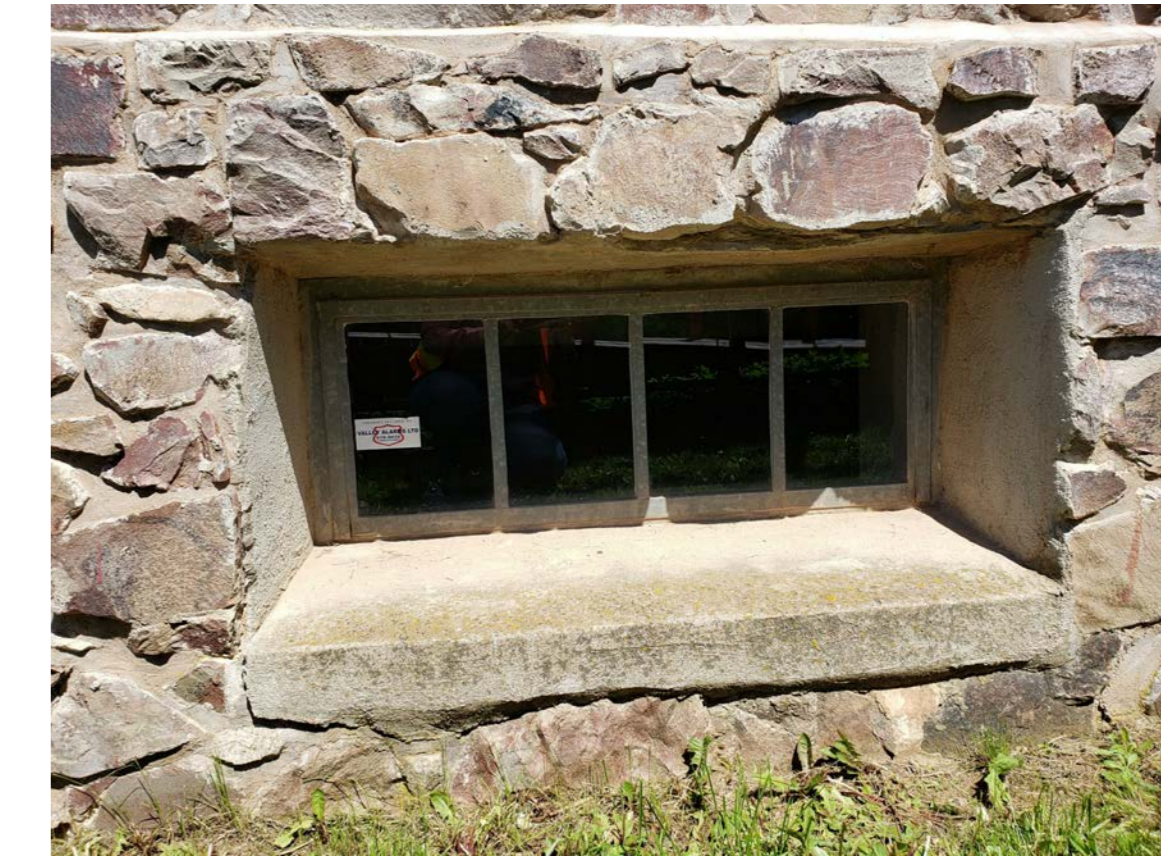
W6 MORTAR DAMAGE AT HEAD OF ROUGH OPENING, ORGANIC GROWTH ON CONCRETE SILL, ALUMINUM FRAME WINDOW STAINED
