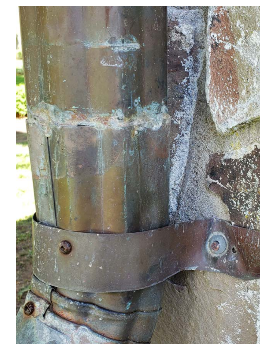
N4 CORRODED COPPER RAINWATER LEADER, CORRODED MISCELLANEOUS FASTENERS
