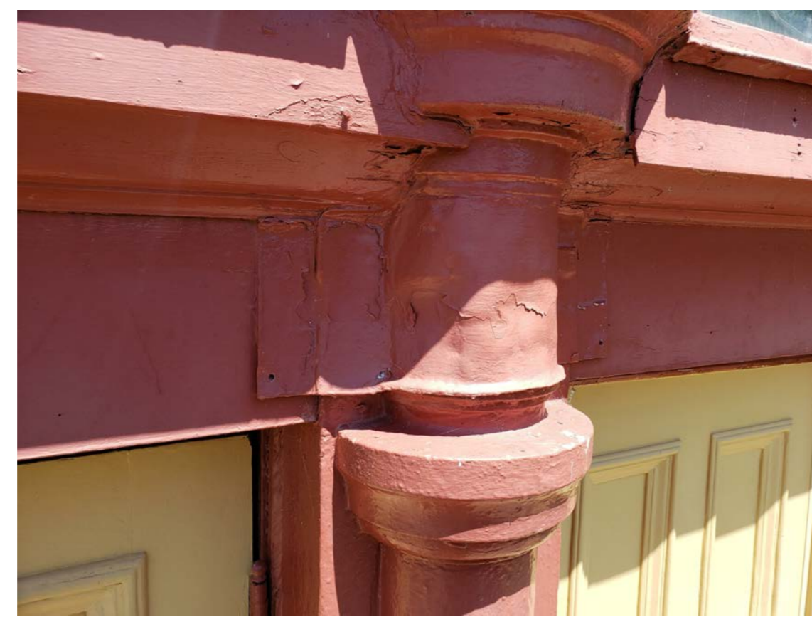
S14 PEELING PAINT, AND MISSING FASTENERS ON LEAD FLASHING AT PILASTER
