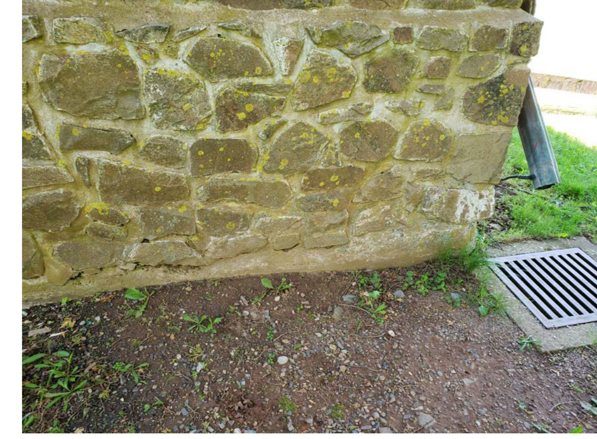
E8 CRACKED MORTAR, EFFLORESCENCE, OPEN JOINTS AND ORGANIC GROWTH AT NORTHEAST CORNER OF CHANCEL
