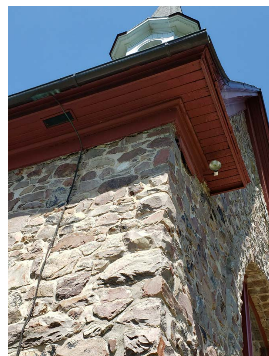
W15 CRACKING AND OPEN JOINTS AT CORNER, CRACKED MORTAR AT JOINT BELOW PROFILED FRIEZE
