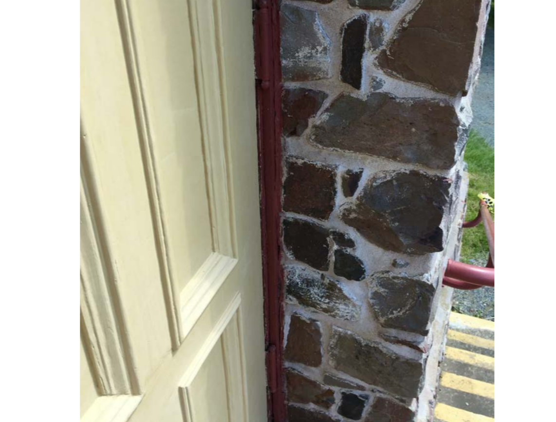
S21 PANEL TO SOUTHWEST OF DOOR HAS CRACKED MORTAR AND EFFLORESCENCE IN JAMB
