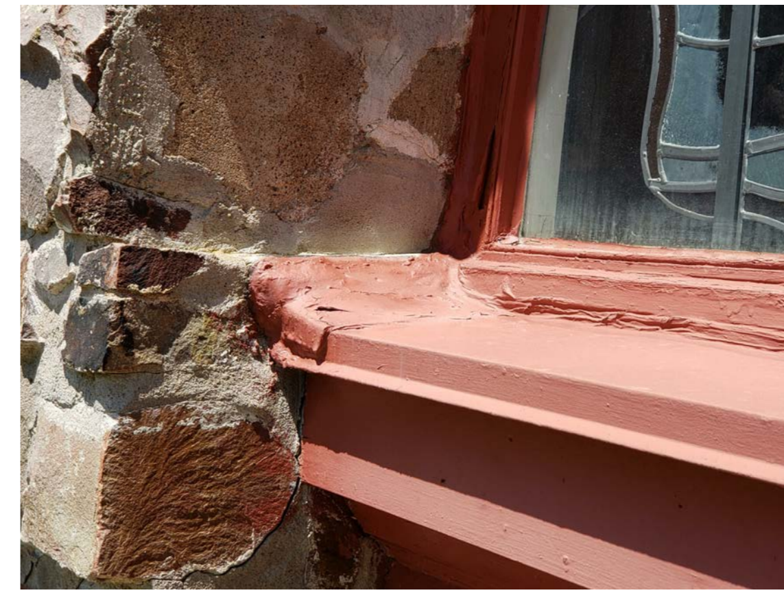
S11 PEELING PAINT, ROTTEN AND WEATHERED WOOD ON WINDOW FRAME, FAILED CAULKING
