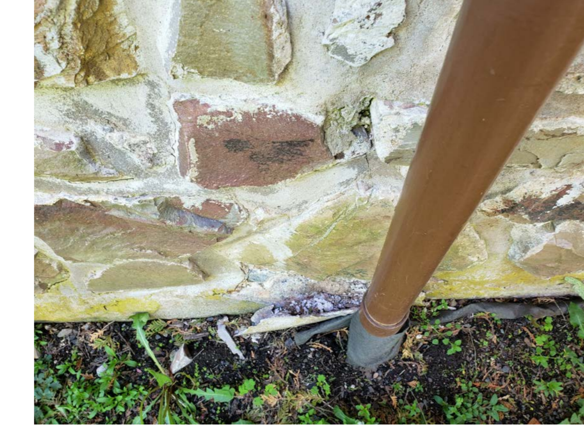
E9 CRACKED MORTAR, EFFLORESCENCE, AND OPEN JOINTS BEHIND OIL TANK VENT PIPE
