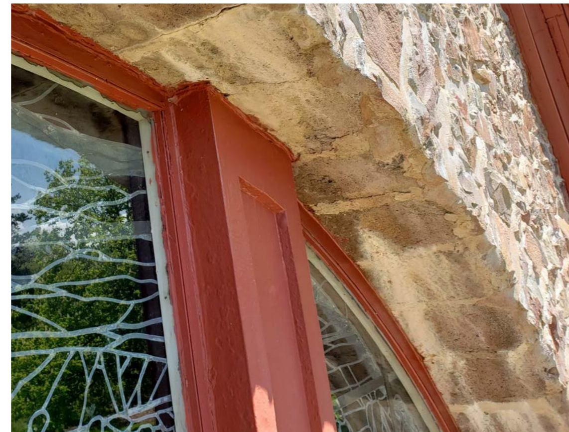
S9 DETERIORATION OF CONCRETE BLOCK ARCH INCLUDING EFFLORESCENCE, WEATHERING AND OPEN JOINTS
