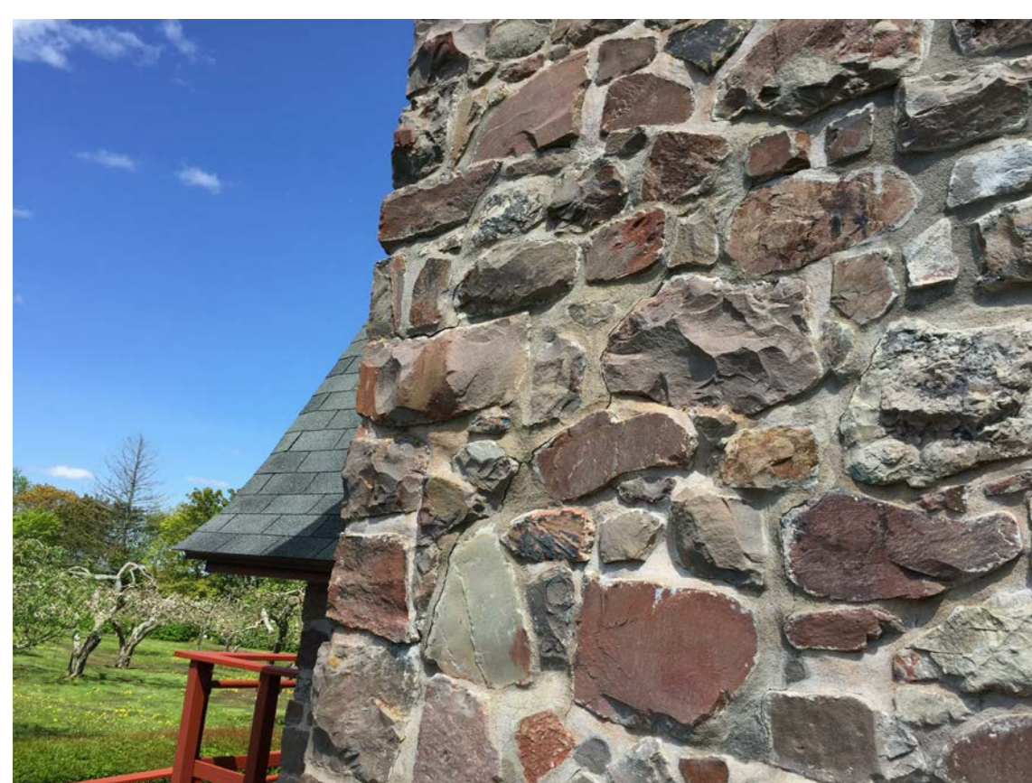
S19 PANEL TO SOUTHWEST OF DOOR HAS CRACKED MORTAR, OPEN JOINTS AND PREVIOUS MORTAR REPAIRS
