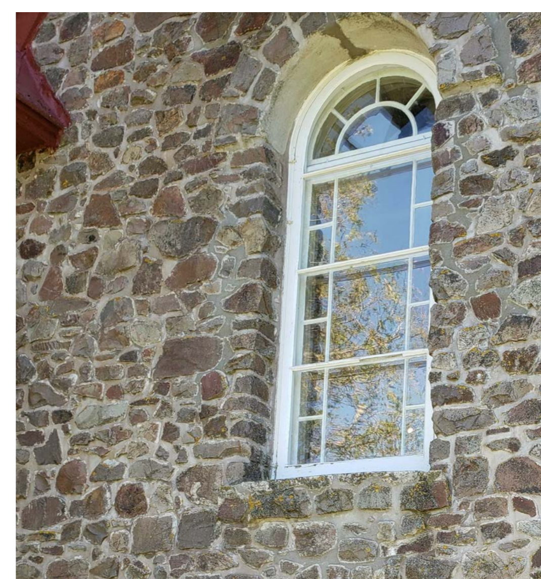
N8 PREVIOUS MORTAR REPAIRS AROUND WINDOW, CRACK AND PREVIOUS REPAIR AT HEAD OF ROUGH OPENING
