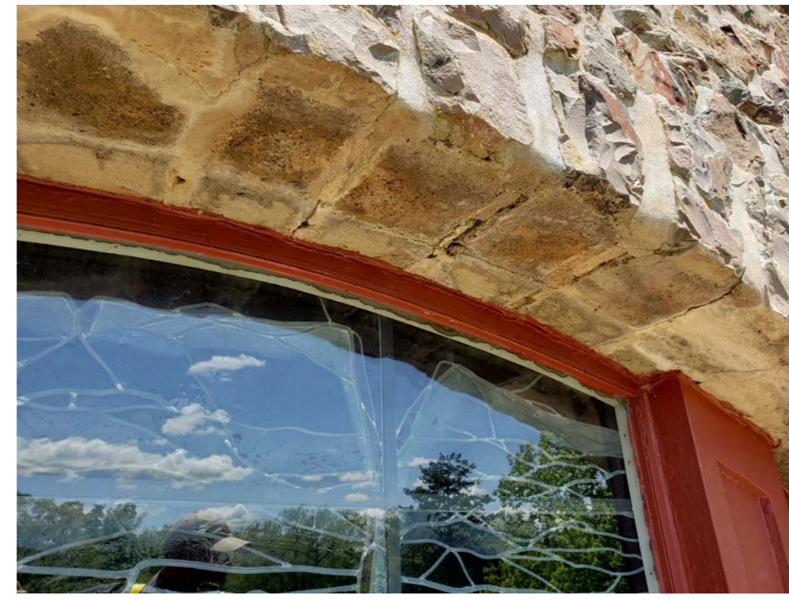
S8 DETERIORATION OF CONCRETE BLOCK ARCH INCLUDING EFFLORESCENCE, WEATHERING AND OPEN JOINTS
