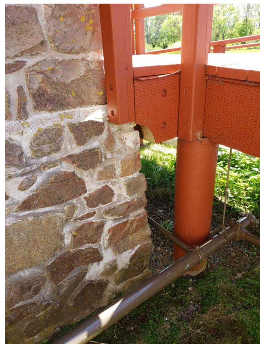
W7 CRACKED MORTAR, OPEN JOINTS, ORGANIC GROWTH AND PREVIOUS MORTAR REPAIRS AT CORNER OF SOUTHWEST PORCH
