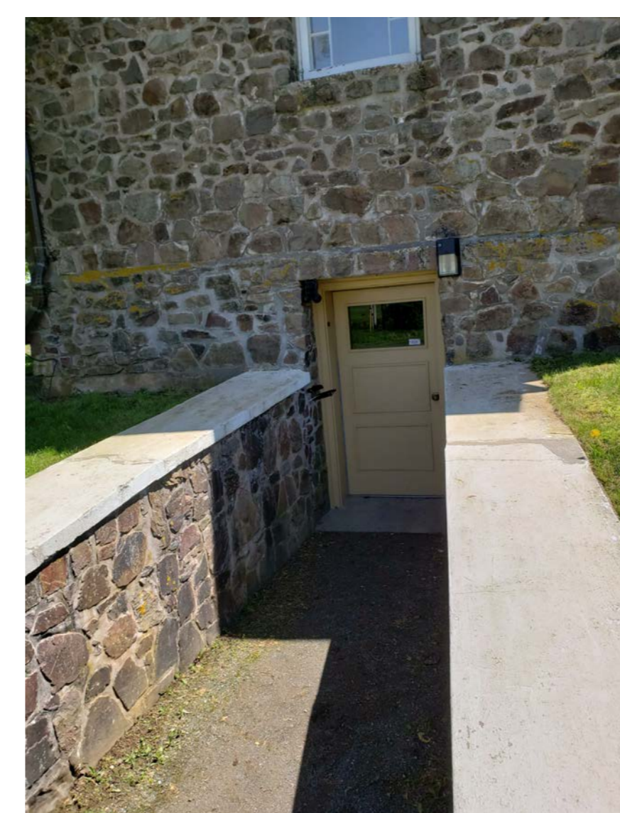
N9 NORTH CHANCEL BASEMENT ENTRANCE, SATURATED BRICK AND MORTAR BELOW END OF WINDOWSILL, ORGANIC GROWTH ON PLINTH
