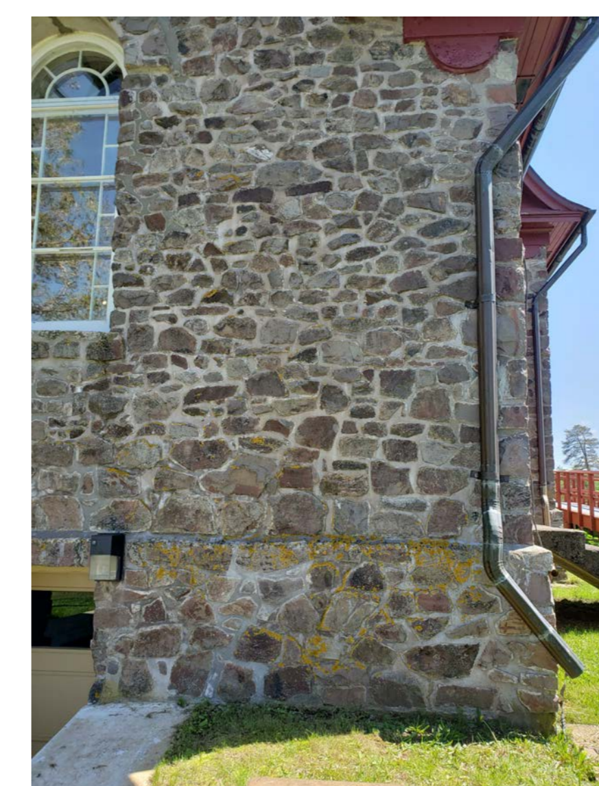
N10 CRACKING AND OPEN JOINTS AT CORNER, ORGANIC GROWTH ON PLINTH
