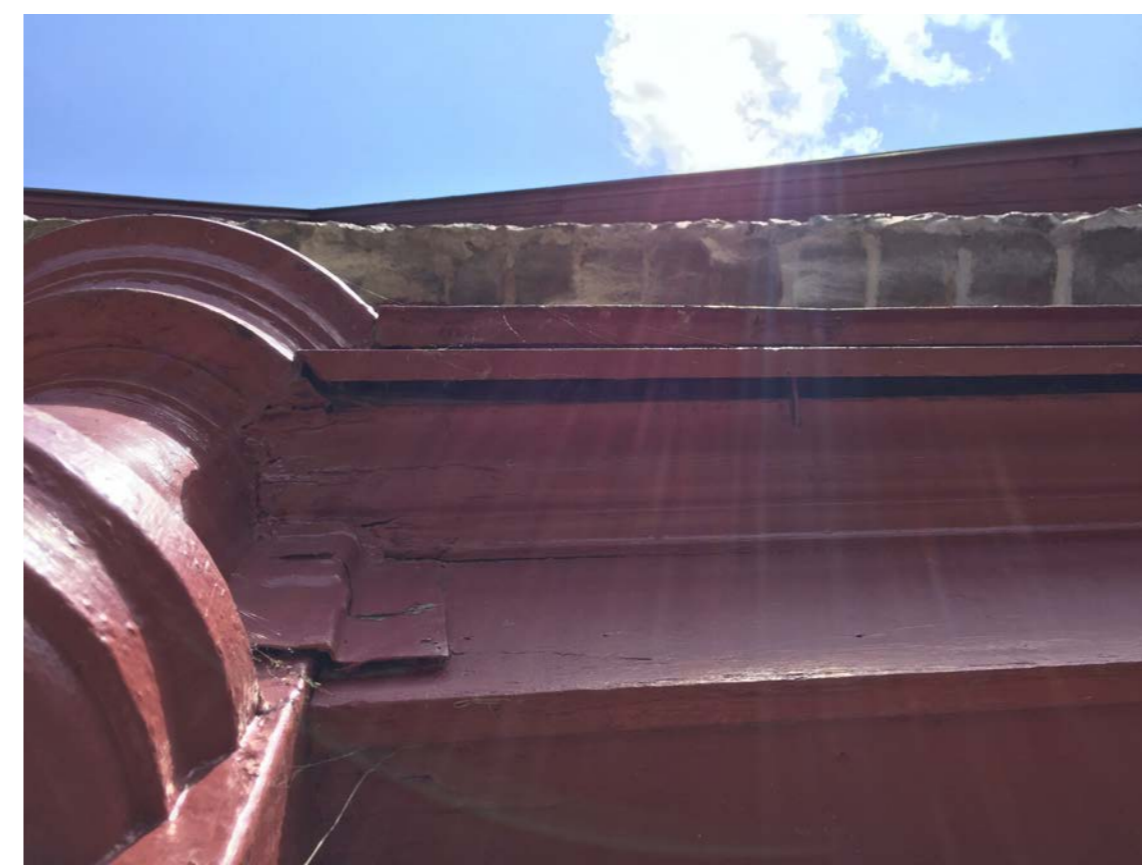
S16 WOOD AND FLASHING DETACHMENT
