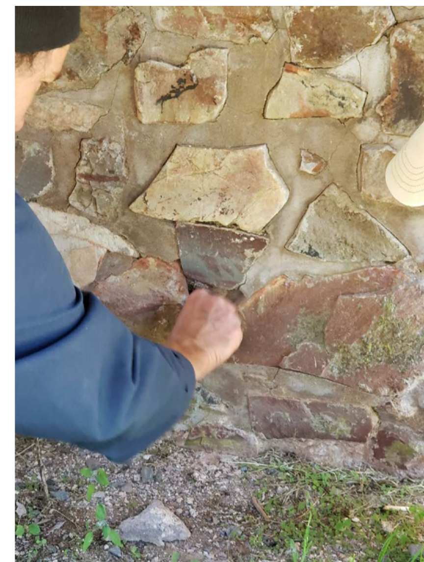
W10 LOSS OF BINDER FROM MORTAR AND MISSING STONE LANDING AT SOUTHWEST PORCH
