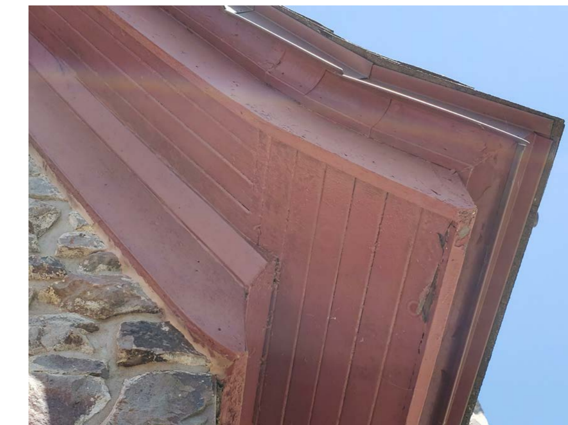
W13 PEELING PAINT, ROTTEN AND WEATHERED WOOD ON SOUTHWEST PORCH SOFFIT AND FASCIA
