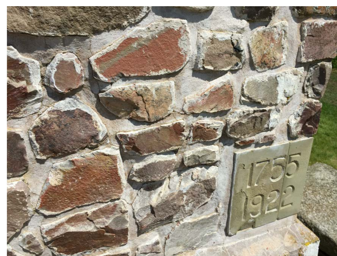
S22 PANEL TO SOUTHWEST OF DOOR HAS CRACKED MORTAR, OPEN JOINTS AND PREVIOUS MORTAR REPAIRS
