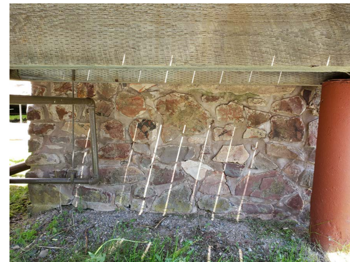
W9 CRACKED MORTAR, OPEN JOINTS, ORGANIC GROWTH AND PREVIOUS MORTAR REPAIRS BELOW LANDING AT SOUTHWEST PORCH
