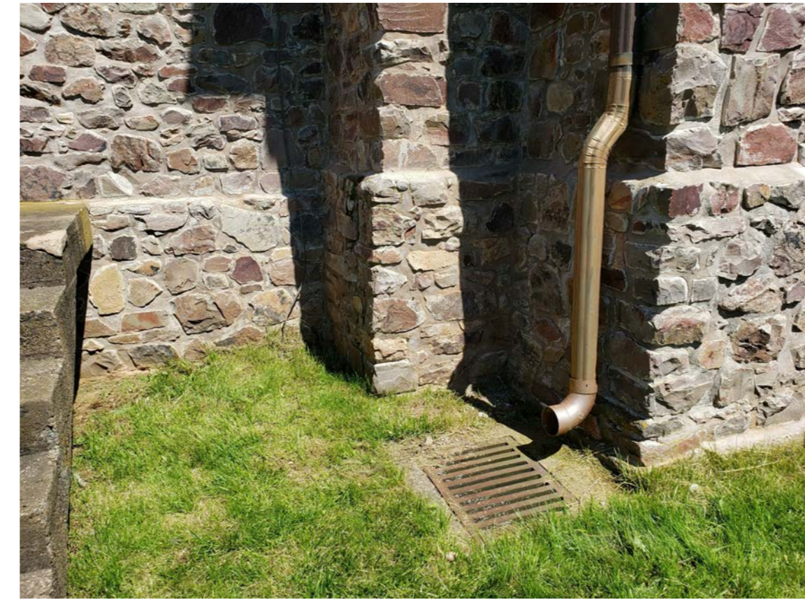
W3 CRACKED MORTAR AND OPEN JOINTS AT CORNERS, VARIOUS MATERIALS AND COLOURS ON DOWNSPOUT
