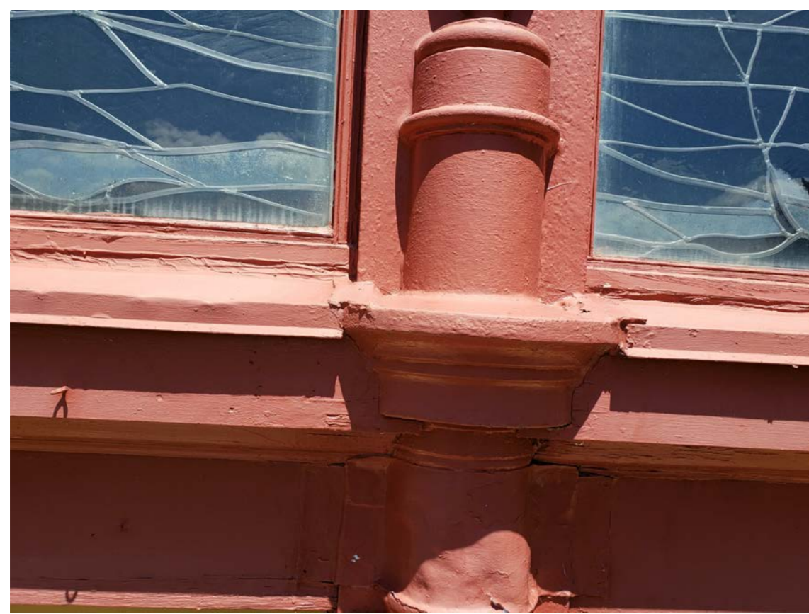
S13 PEELING PAINT, ROTTEN AND WEATHERED WOOD ADJACENT CAST IRON PILASTER
