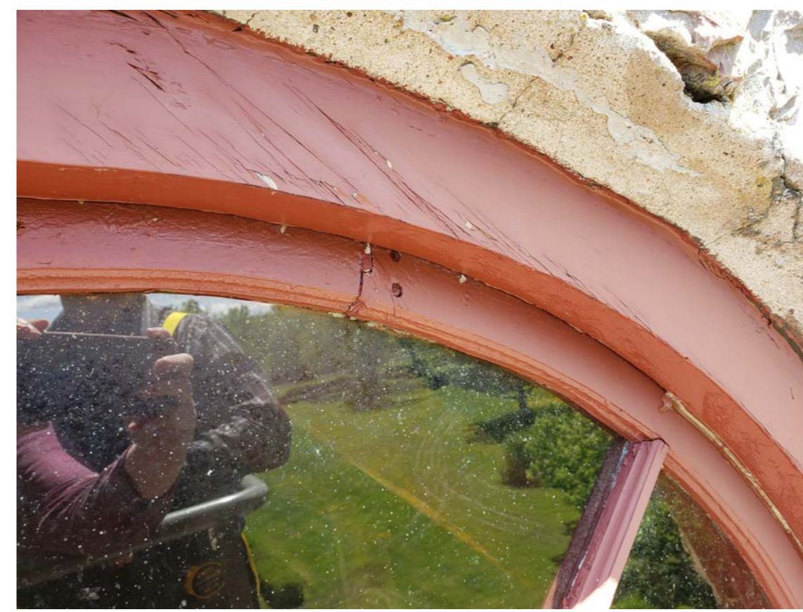
S4 PEELING PAINT, ROTTEN AND WEATHERED ON LUNETTE WINDOW FRAME
