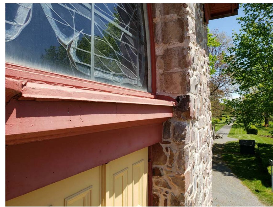
S15 PEELING PAINT, ROTTEN AND WEATHERED WOOD, PEELING PAINT ON CAP FLASHING
