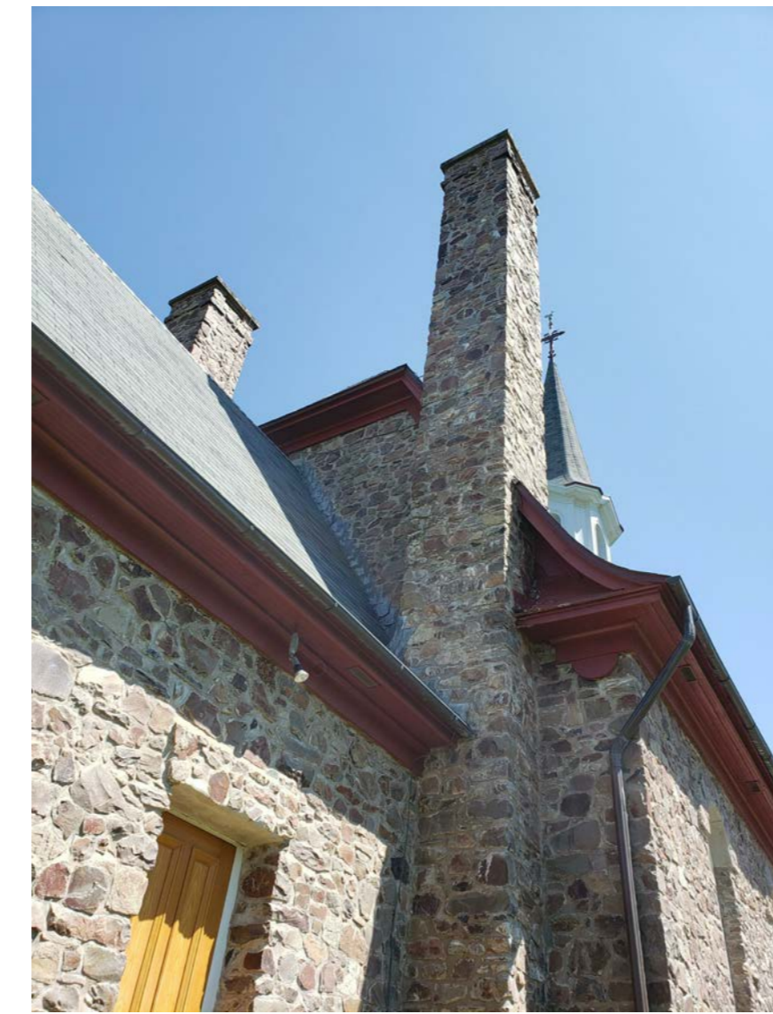
W4 EFFLORESCENCE ON BACKSIDE OF CHIMNEY, SATURATES MORTAR AND STONE AT END OF GUTTER, WATER DAMAGE AND ORGANIC GROWTH BELOW, PEELING PAINT ON FAKE RETURN FLASHING, GAP BEHIND WOOD MEDALLION
