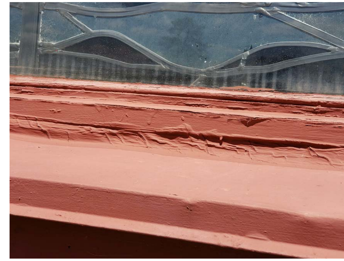
S12 PEELING PAINT, ROTTEN AND WEATHERED WOOD ON WINDOW FRAME, FAILED CAULKING
