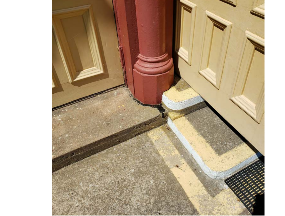
S17 PEELING PAINT, ROTTEN AND WEATHERED WOOD ON DOOR FRAMES
