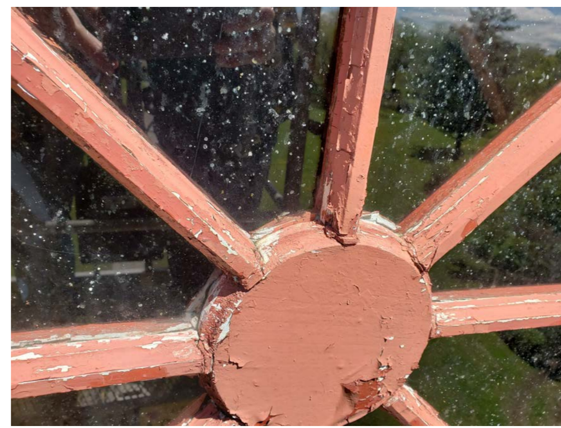
S3 PEELING PAINT, ROTTEN AND WEATHERED WOOD ON LUNETTE WINDOW SASH
