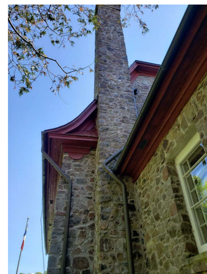
N1 EFFLORESCENCE ON BACKSIDE OF CHIMNEY, PEELING PAINT ON RAKE RETURN FLASHING
