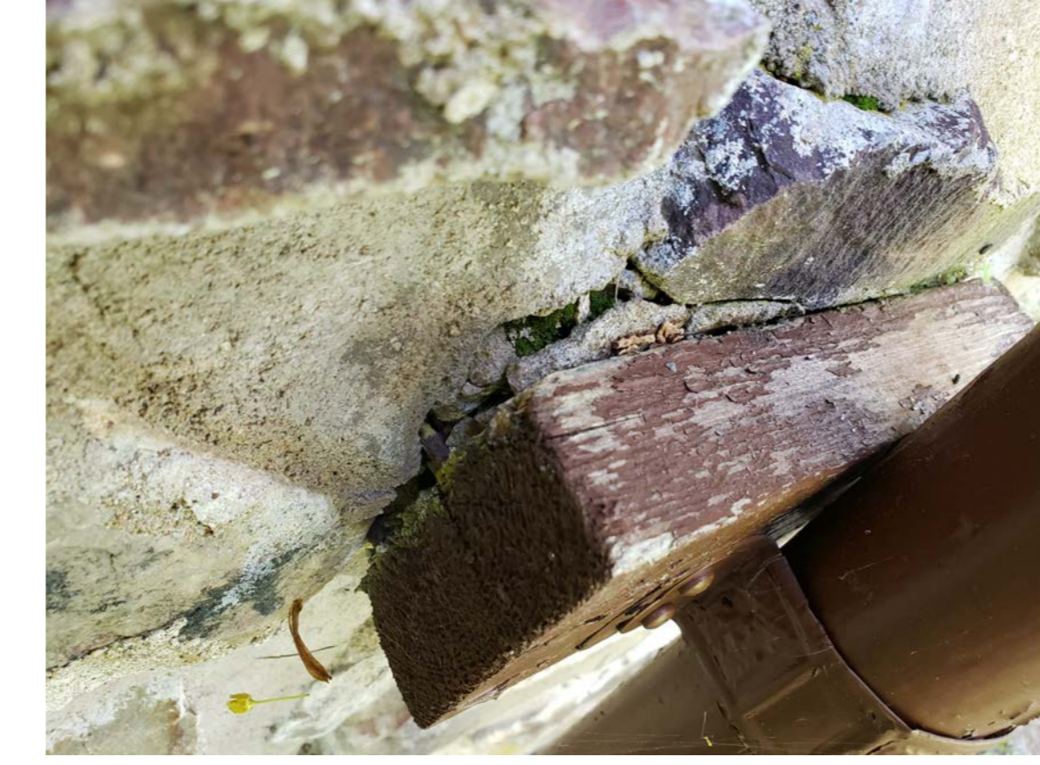
E10 CRACKED MORTAR, EFFLORESCENCE, OPEN JOINTS AND ROTTEN WOOD BLOCKING BEHIND OIL TANK VENT PIPE
