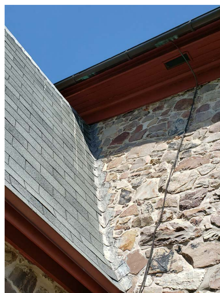
W14 STAINING ON ROOF SHINGLES, LEAKING COPPER GUTTER
