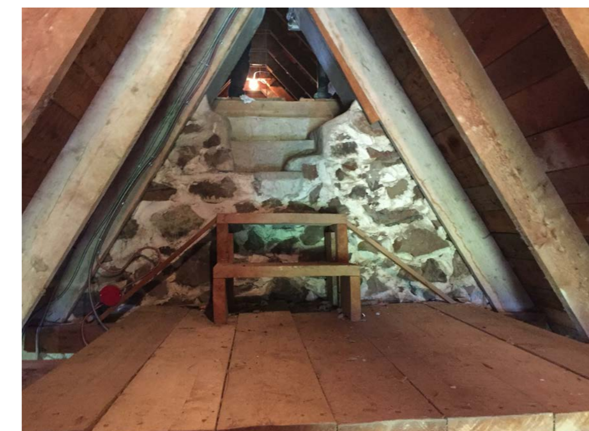
I2 INTERIOR PORTION OF NORTH NAVE WALL BELOW CHANCEL ROOF AND ACCESS TO ATTIC ABOVE NAVE
