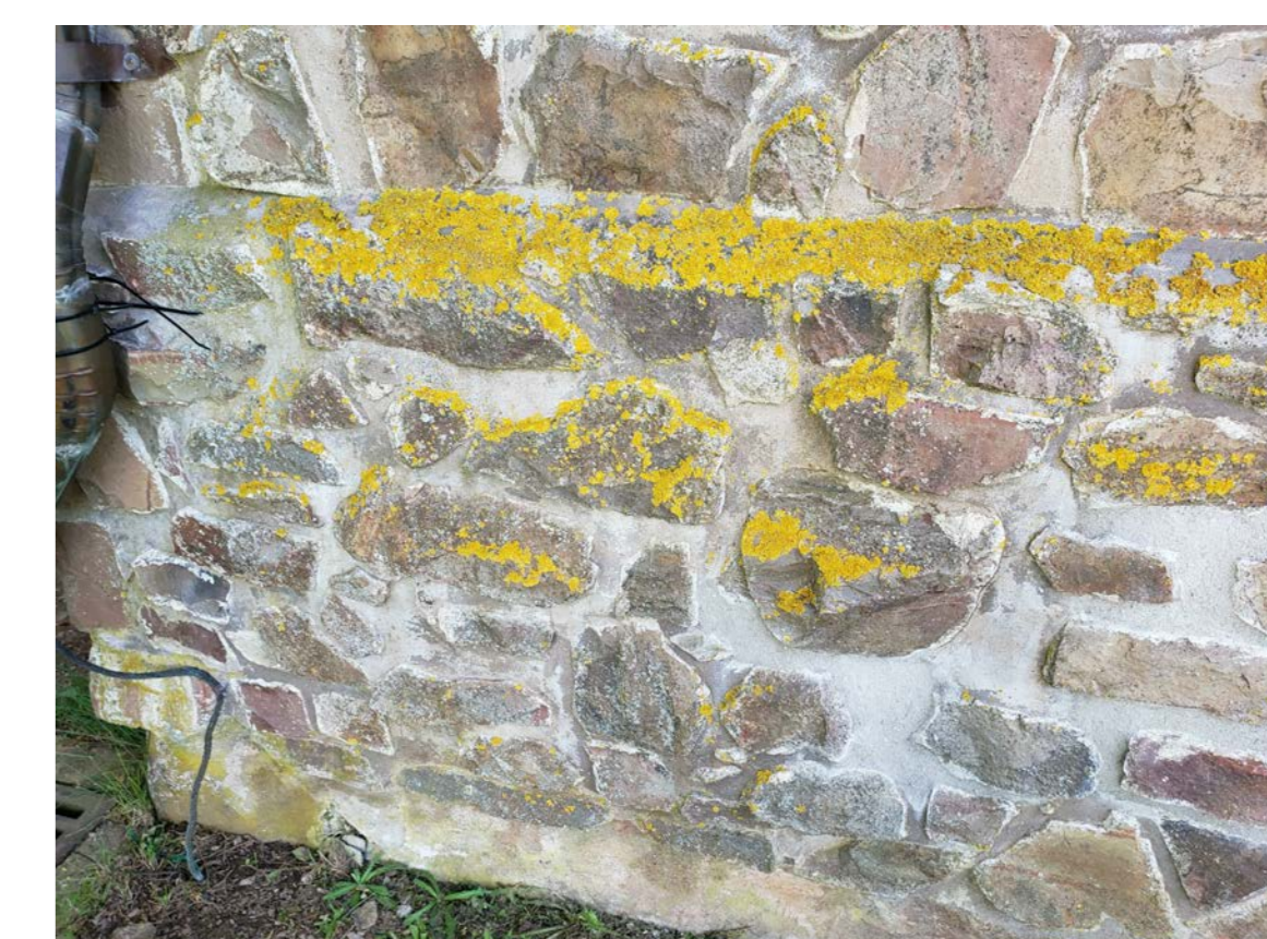
N11 ORGANIC GROWTH ON PLINTH, PREVIOUS MORTAR REPAIR, CRACKED MORTAR AND MISSING STONE AT BASE OF PLINTH
