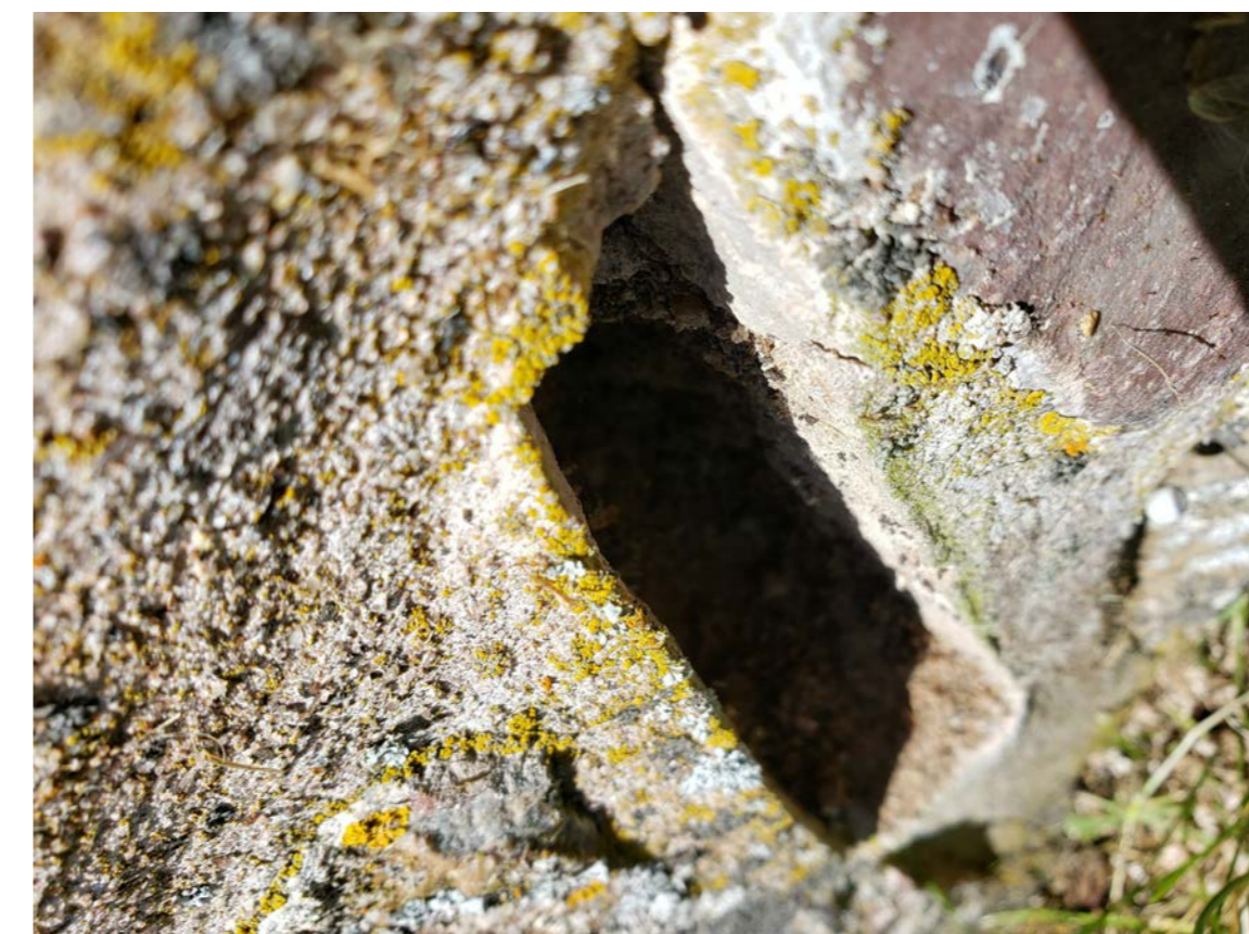
W11 SAND (LOSS OF BINDER) FROM MORTAR JOINT BELOW LANDING AT SOUTHWEST PORCH
