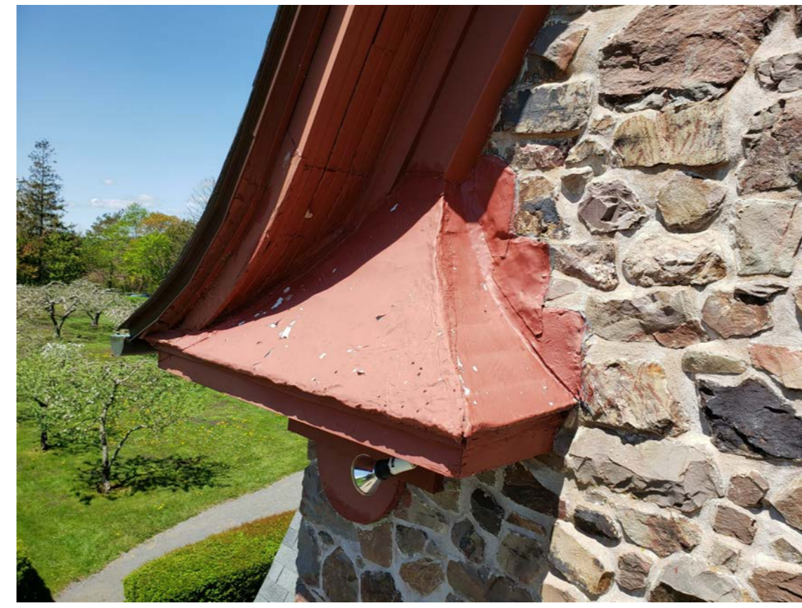
S10 PEELING PAINT ON RAKE RETURN, ROTTED WOOD SOFFIT
