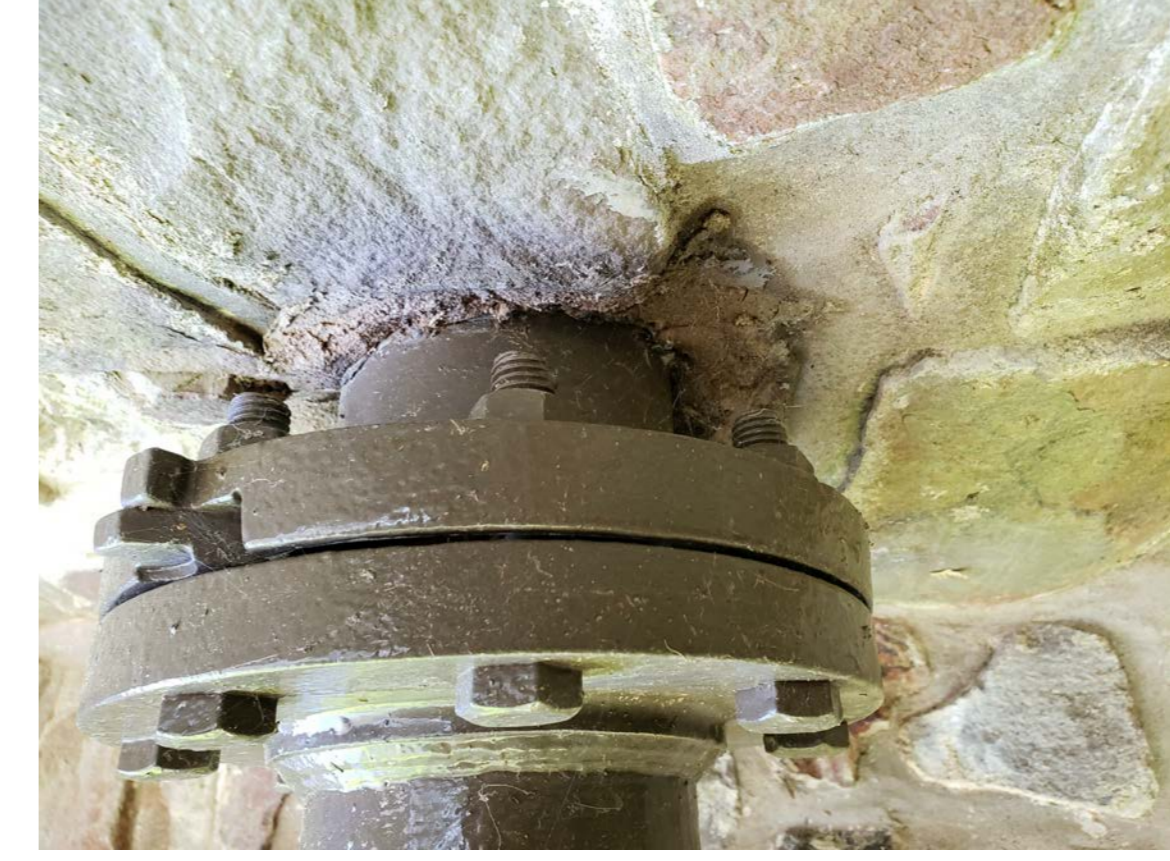
E11 POOR MORTAR REPAIR AT THROUGH WALL PENETRATION
