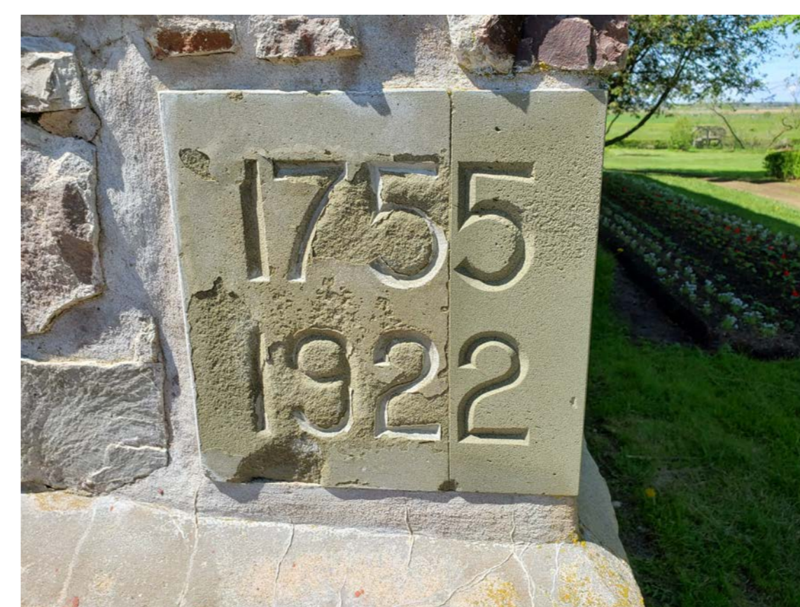
S23 SANDSTONE CORNER STONE IS CHIPPED AND EXFOLIATING
