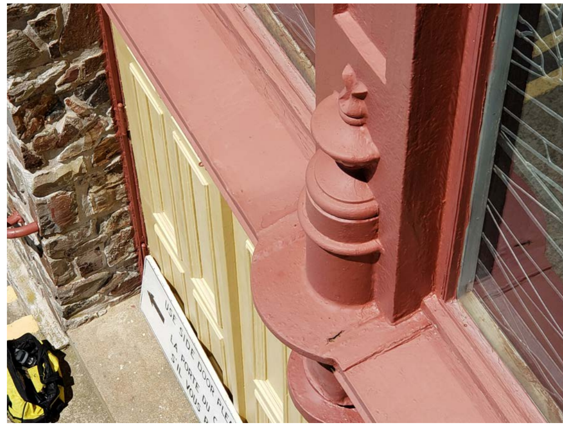
S7 MINOR DAMAGE TO LEDGE OF CAST IRON PILASTER
