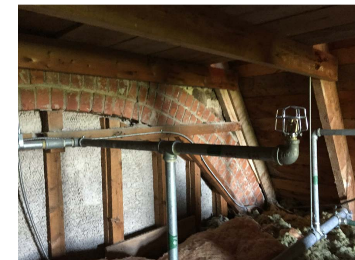
I6 INTERIOR FACE OF SOUTH NAVE WALL, BRICK ARCH WITH LATCH AND PLASTER INFILL
