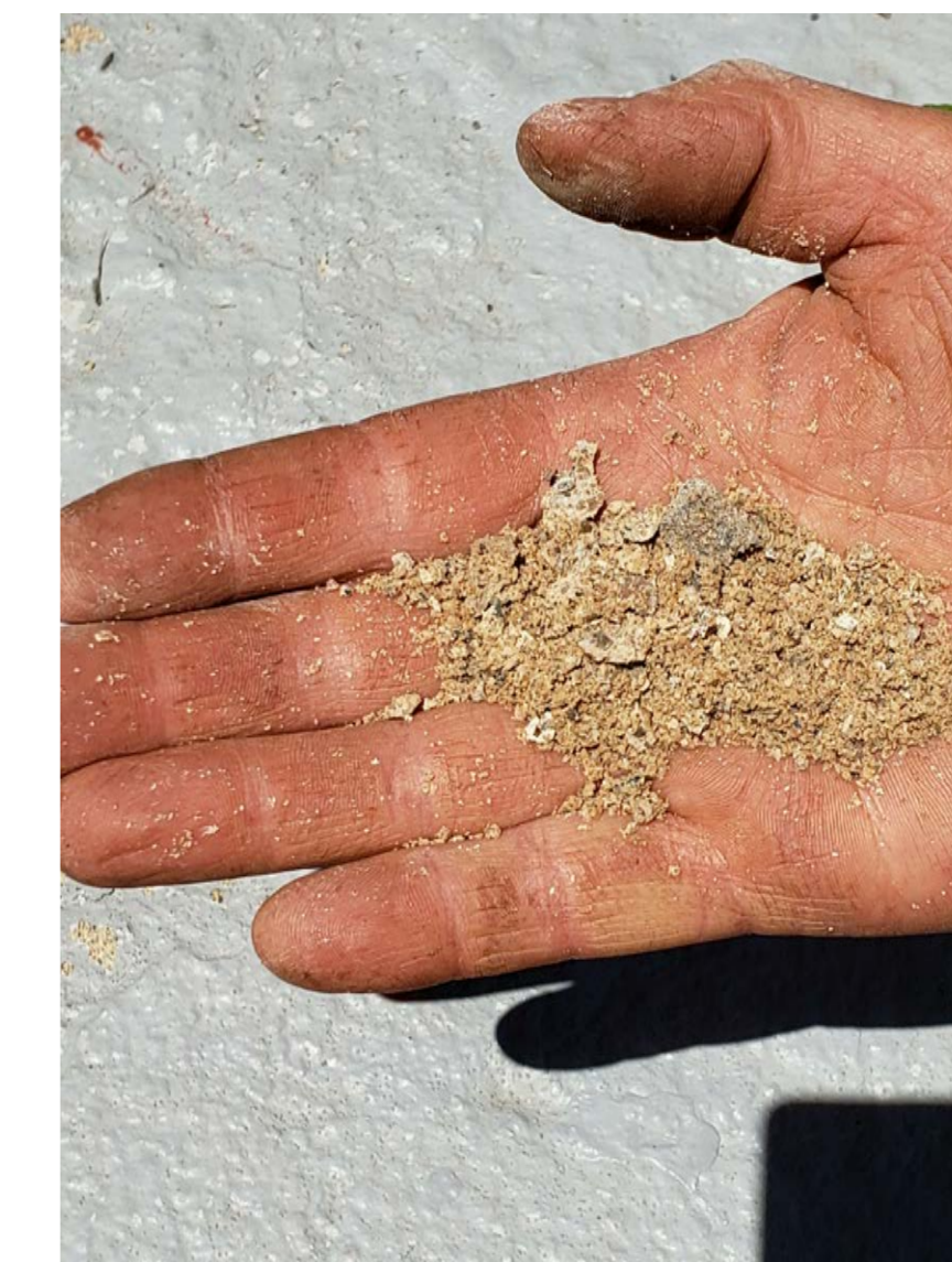
W12 SAND (LOSS OF BINDER) FROM MORTAR JOINT BELOW LANDING AT SOUTHWEST PORCH
