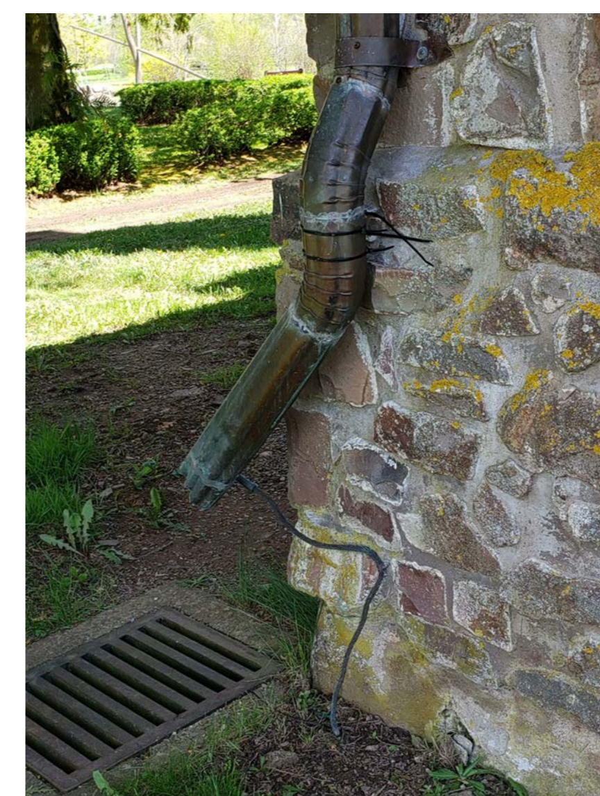
N3 DAMAGED AND CORRODED COPPER RAINWATER LEADER, MAKESHIFT REPAIR WITH ZIP TIES
