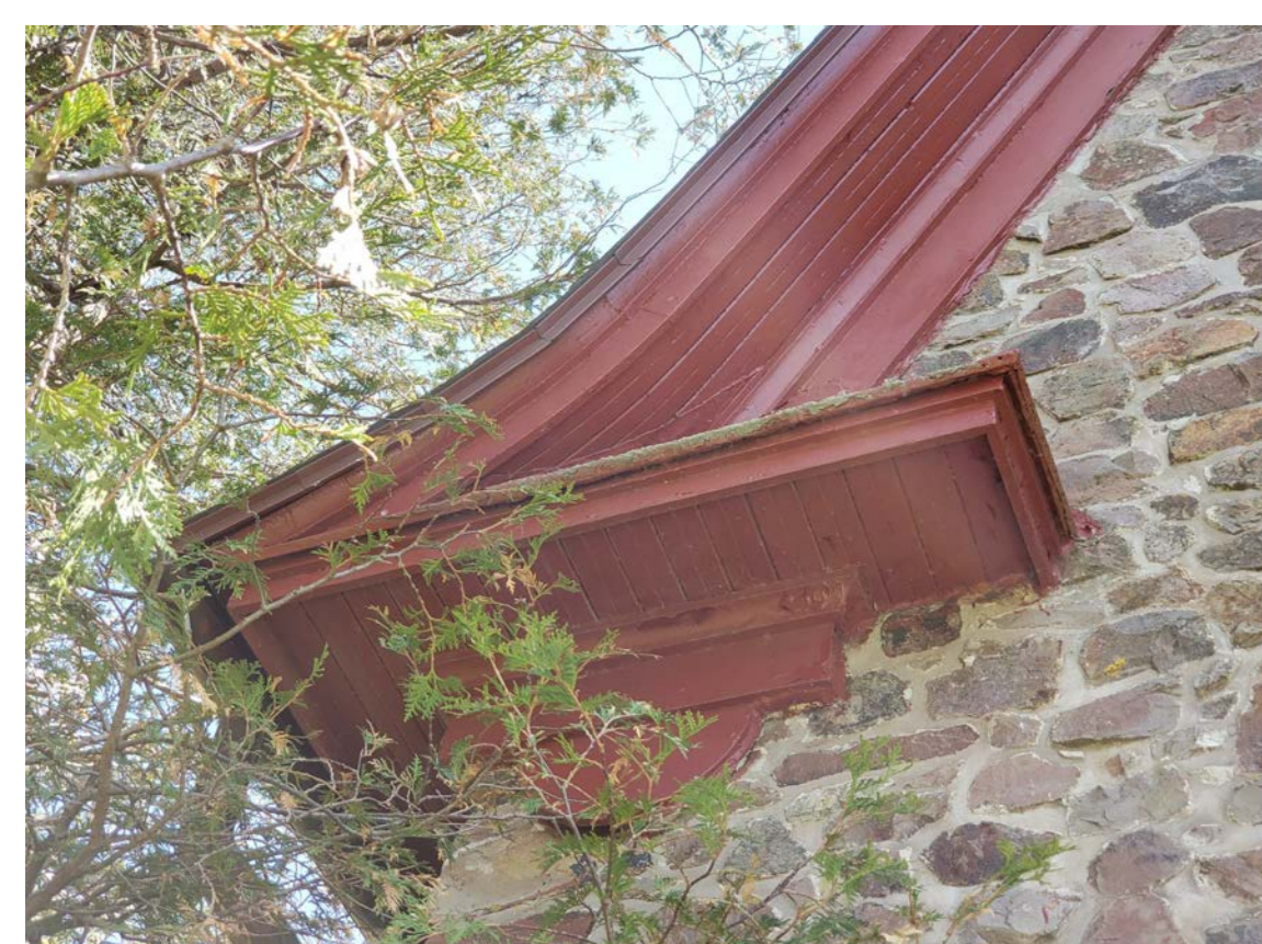
N6 GAP BEHIND WOOD MEDALLION, ORGANIC GROWTH ON ROTTEN WOOD
