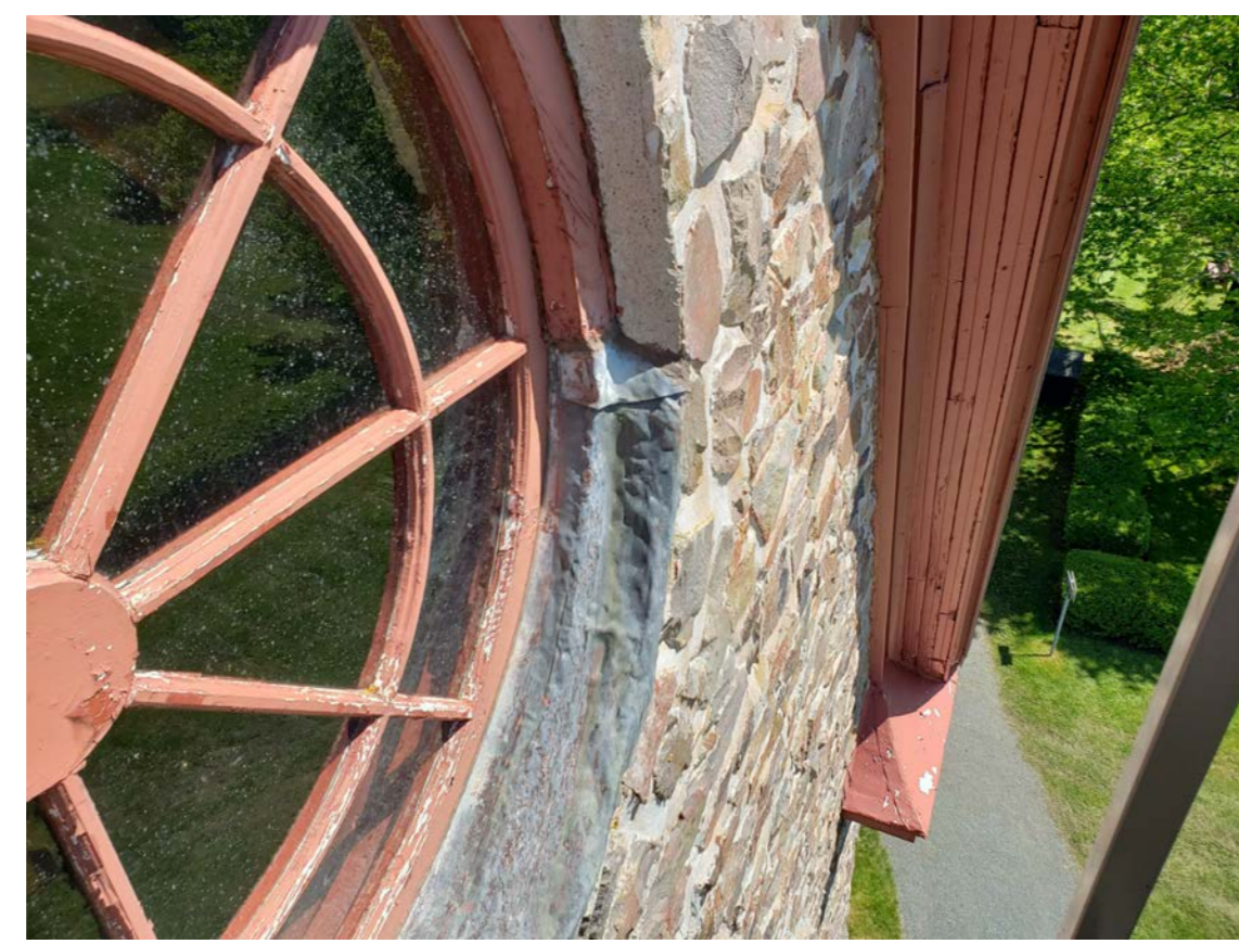
S2 PEELING PAINT, ROTTEN AND WEATHERED WOOD ON LUNETTE WINDOW, SOFFIT AND RAKE RETURN. LUNETTE WINDOW INSTALLED BACKWARDS
