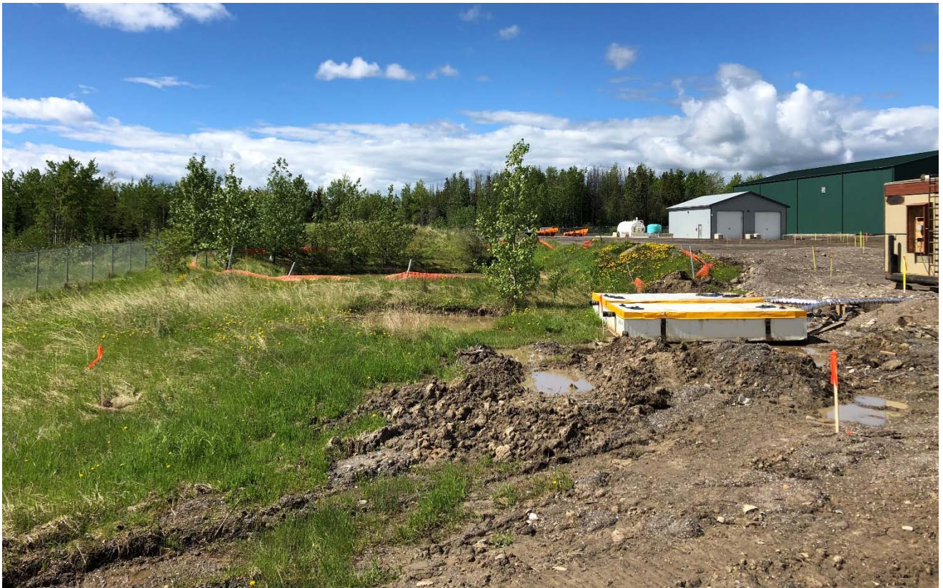
Photograph 5: View of eastern corner of the site, east of the trailers, looking southwest (June 2020).
