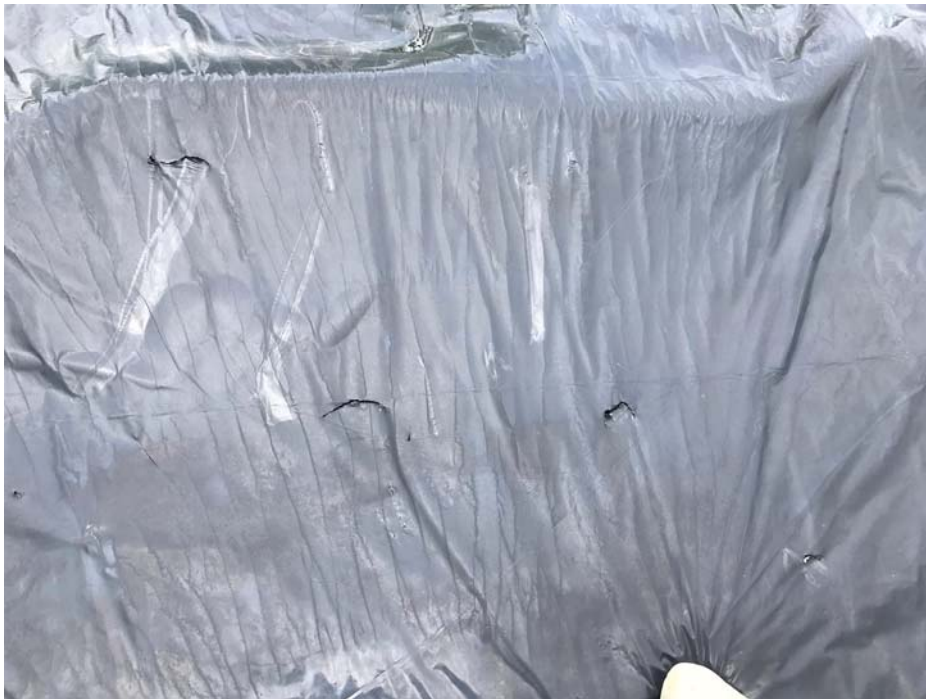
Photo: Example of liner damage
