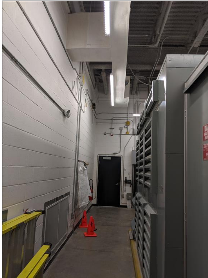
Picture 1 - Electric Room Access
