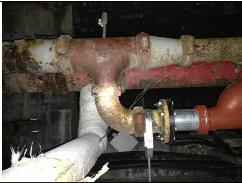
Fixed wharf water and fire line piping
