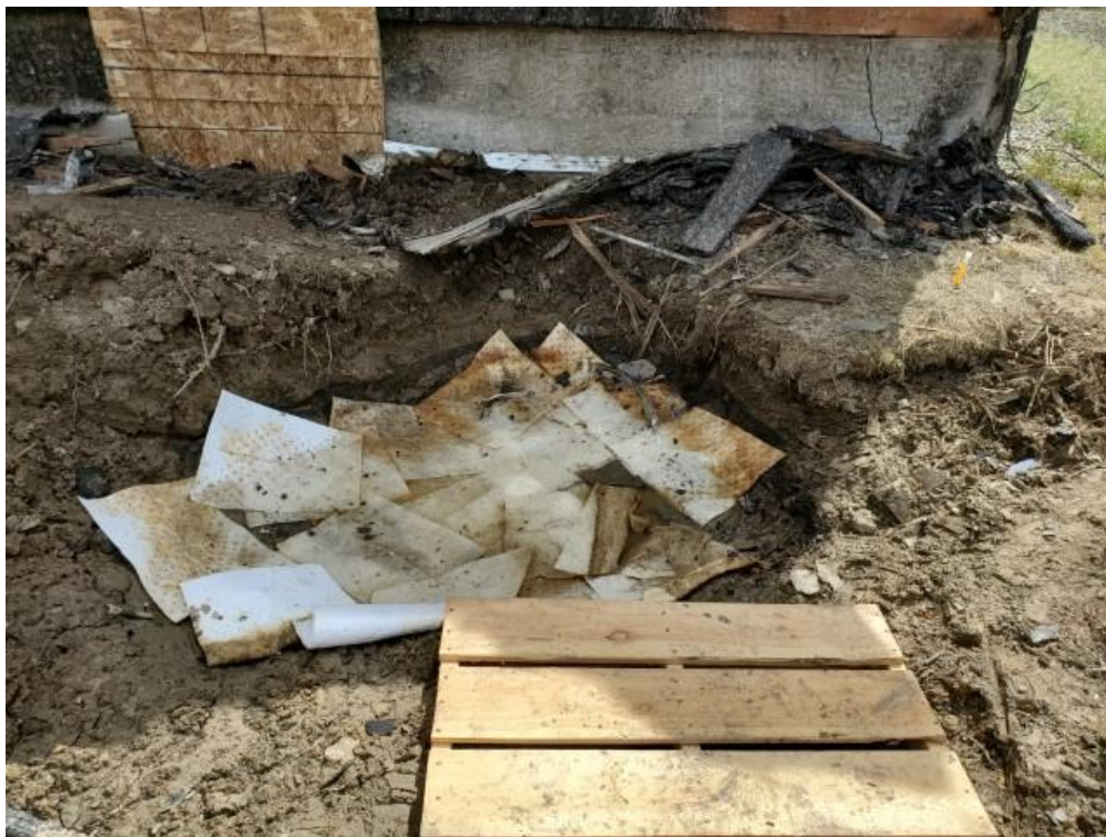
Photo 2: A view of the main impact area prior to being filled in/levelled. Note the crack in the foundation on the right edge of the building. The basement window of the home is boarded up at the top left of the photograph.
