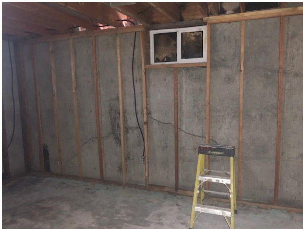
Photo 9: A view of the basement wall/foundation, looking north. The boarded-up basement window visible in Photo 2 is visible. Cracking of the foundation is evident.
