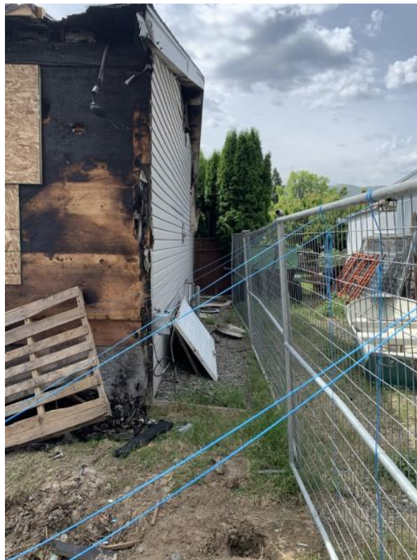
Photo 5: A view of the west side of the home at 2425 Glenview Avenue, looking south; the severed hydro-electric and telecommunications connections are visible at the top right corner of the home; the Fortis BC gas meter is present on the west side of the home, midway along the wall. The fence shown in the photograph, and associated anchor ropes, will be removed prior to remediation.
