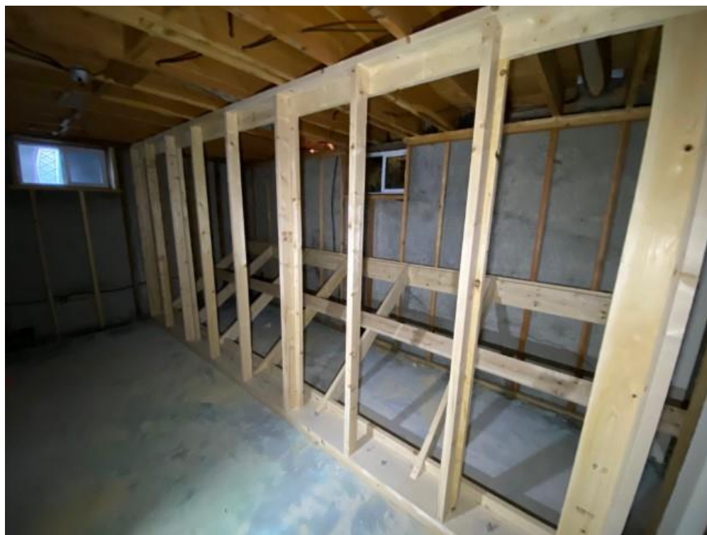
Photo 10: A view of the basement with temporary bracing and a support wall installed.
