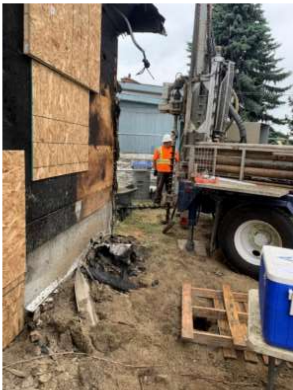
Photo 6: Auger drill rig onsite at location MW20-02 on 11 June 2020 for soil sampling and monitoring well installation.
