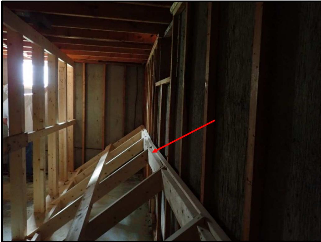
Photo 8: View Along North Concrete Basement Wall In Storage Room Showing Convex Inward Deflection of Wall And Also Temporary Stud Wall Support.
