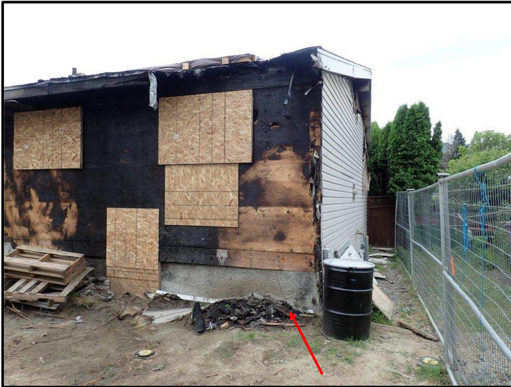
Photo 3: Damage At North West Corner Of Residence Including Damage To Eaves/Soffit, Superficial Fire Damage To North Face Of Timber Stud Wall And Crack In Concrete Basement Wall Due To Exterior Soil Pressure.
