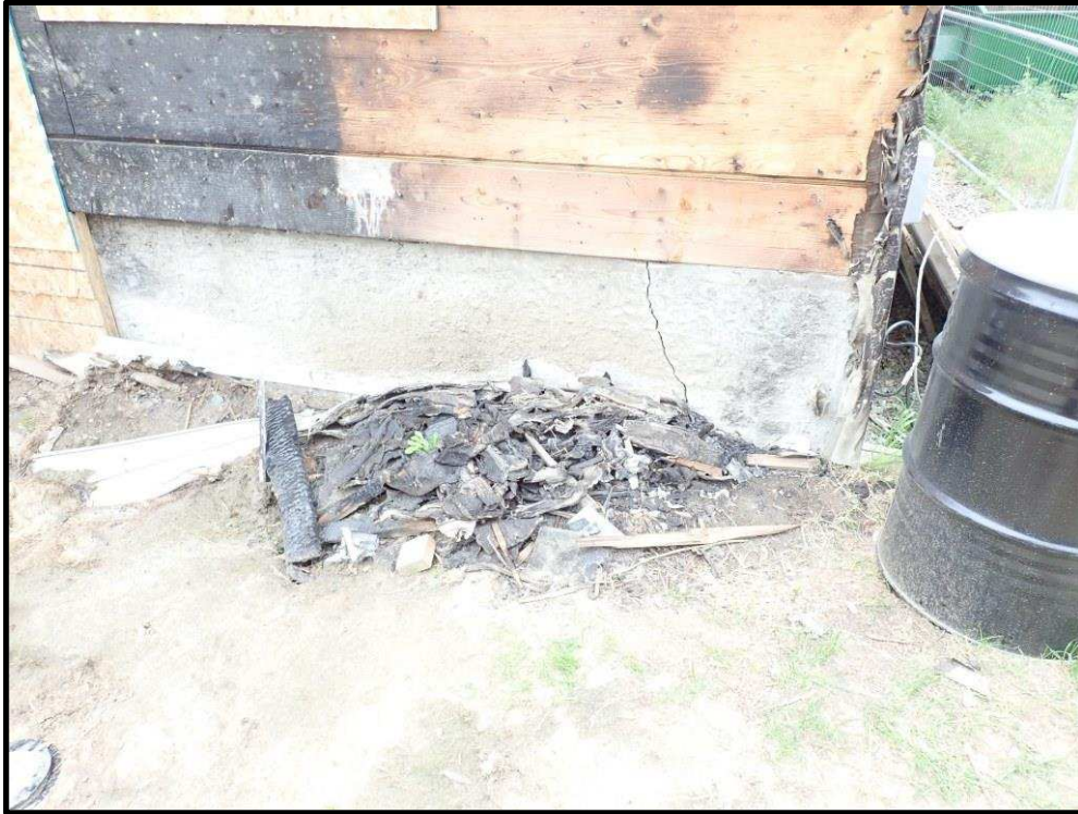
Photo 5: Close Up Of Crack In Concrete Basement Wall At North West Corner Due To Exterior Soil Pressure
