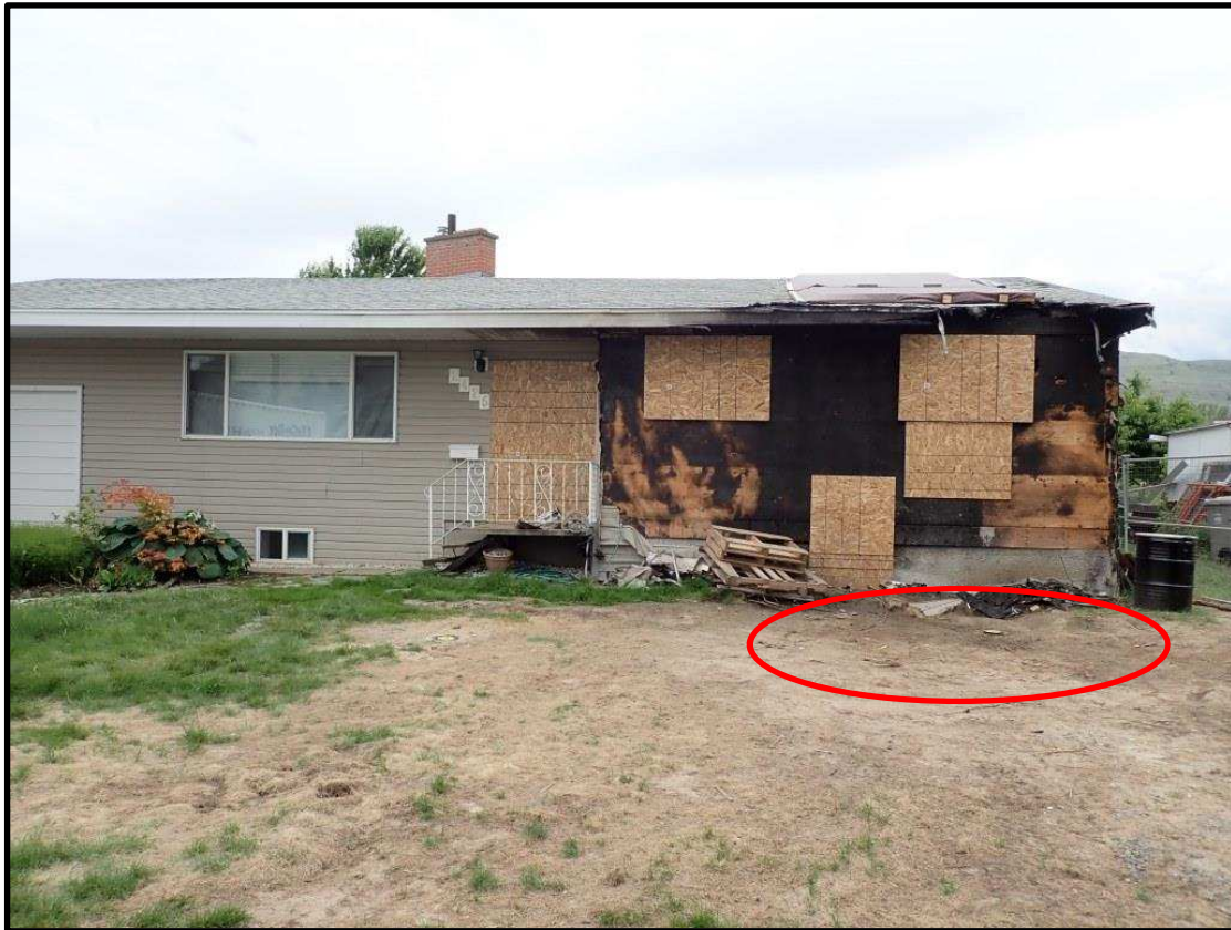
Photo 1: Front View Of 2425 Glenview Ave. From The North Side. Note Approximate Area Of Aircraft Impact And Anticipated Excavation For Remediation/Removal Of Contaminated Soils.
