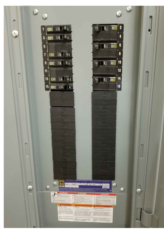
PICTURE OF EXISTING PANEL #UD IN ROOM D-104
