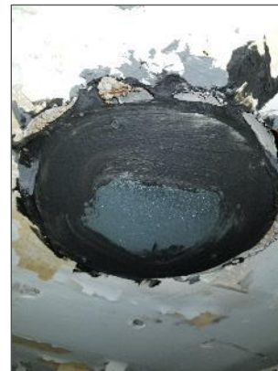
View of non-asbestos, dark grey mastic present around a ceiling vent in Room 235.
