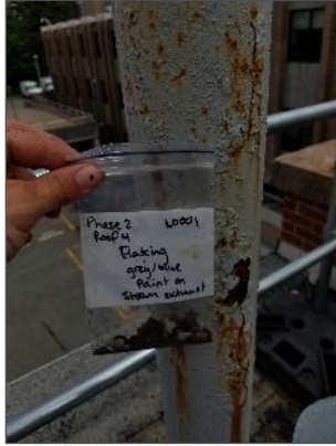
View of low level, lead-containing, grey/blue paint on the steam exhaust pipe.
