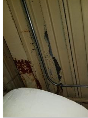
View of lead-containing, cream paint on the steel deck in the Penthouse.
