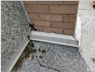
View of asbestos-containing, white caulking present on Phase 1 – Roof 4.
