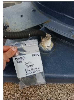
View of non-PCB, dark grey caulking on duct wiring.
