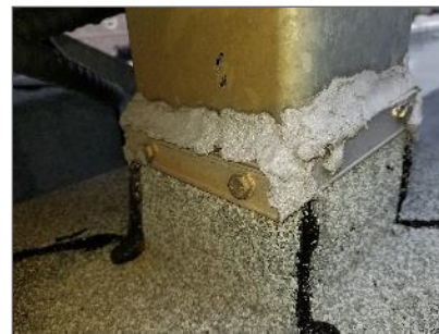
View of non-asbestos, grey caulking present around a roof/vent connection on Phase 1 - Roof 3.
