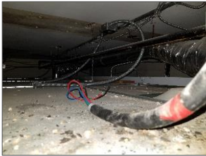
View of plaster debris present in the North West Corner Offices above the acoustic ceiling tile.
