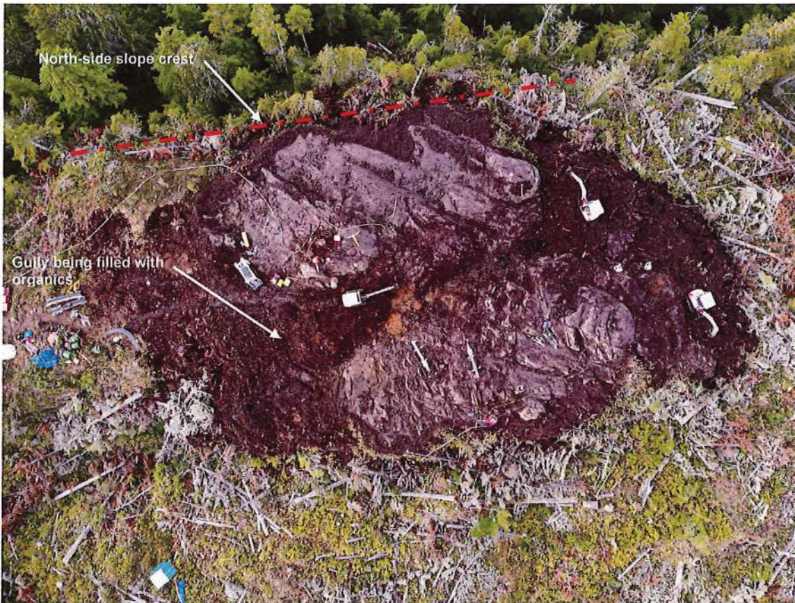
Photo 1 – Provided photo of site during clearing. General outline of bedrock surface can be seen, as well as crest of steep north-side slope. Stripped organics are being pushed into gully to southwest of cleared bedrock.
