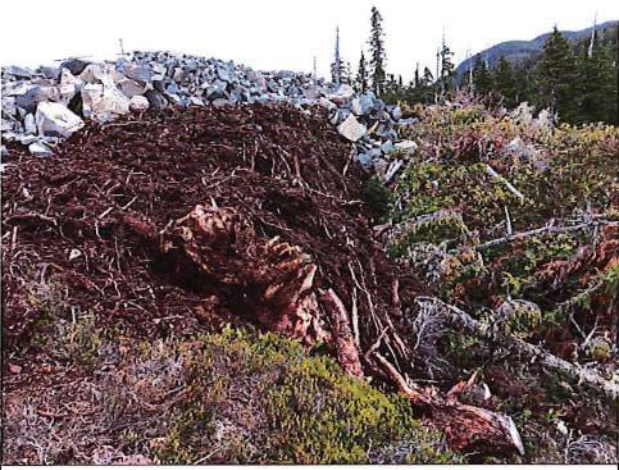
Photo 6 – Gully at southwest corner of site filled with organics and capped with blast rock.
