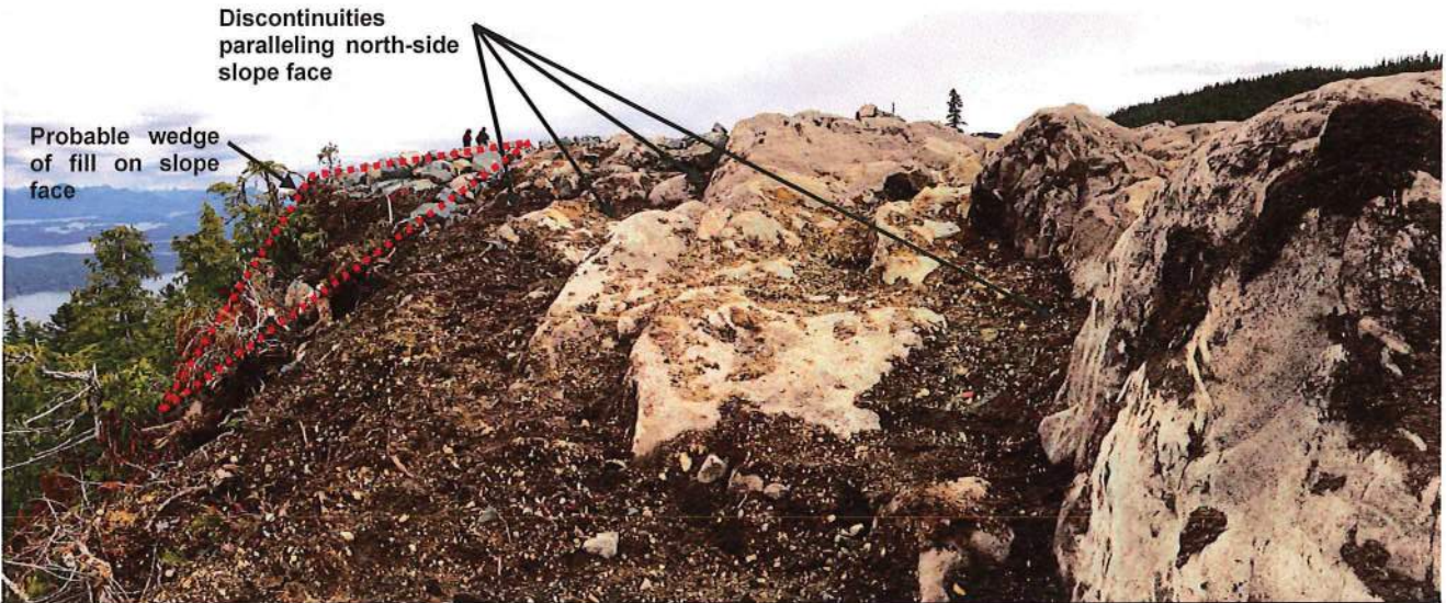
Photo 5 – Looking eastwards along northern side of site. Persistent bedrock discontinuities that generally parallel northern slope face are visible, as well as probable wedge of fill on north side slope crest.
