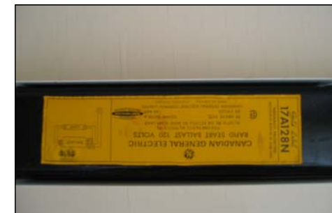
Photo 7: Fluorescent Light Ballast Suspected to Contain PCBs
