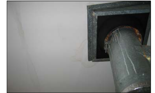
Photo 9: Water Stains at Chimney
