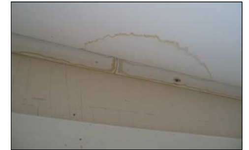
Photo 8: Water Stains on the Ceiling
