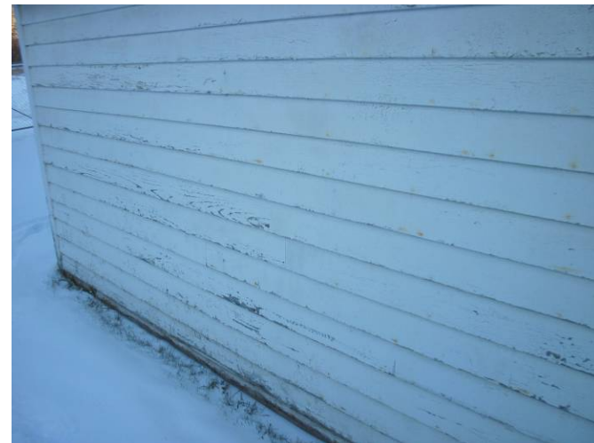
AR-004 – Deteriorated paint finish at exterior wall.
