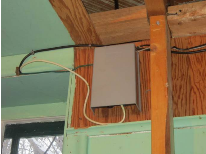
EL-023 – Internal telephone wiring in basement.
