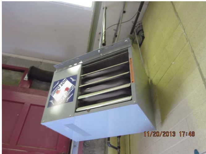
ME-005 – Gas fired unit heater.
