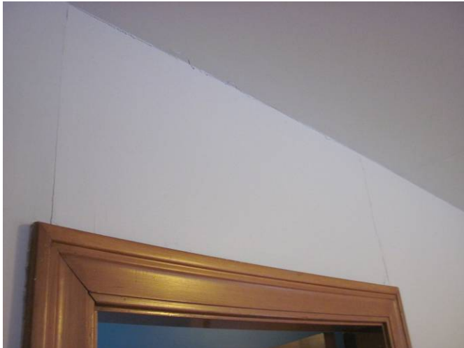
AR-009 – Cracked gypsum board at wall.
