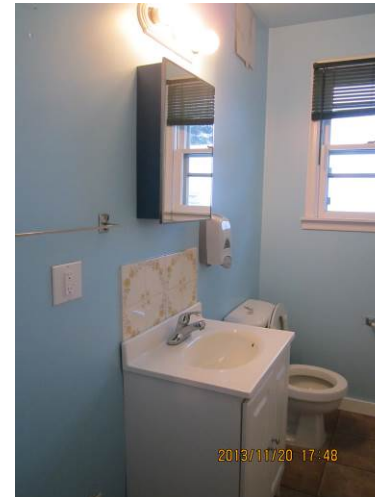
EL-014 – Interior lighting in washroom with GFCI that must be replaced.
