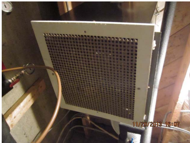
ME-027 – Exhaust fan in basement.
