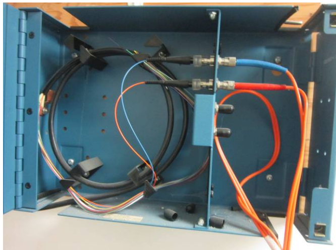
EL-031 – Fibre optic and data equipment for site.
