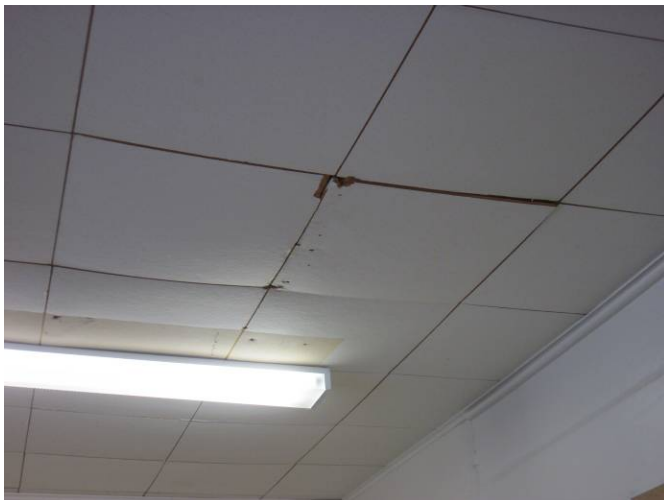
AR-015 – Loose and damaged fibreboard ceiling.
