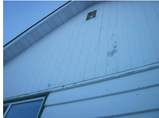
AR-006 – Deteriorated paint finish at gable.
