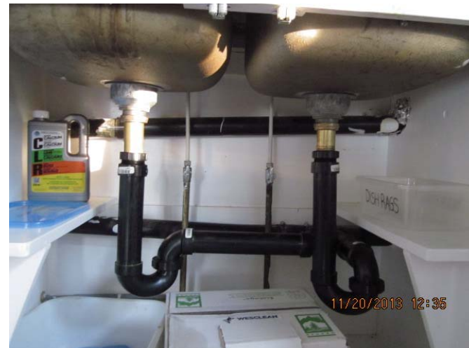
ME-012 – Piping and drainage.
