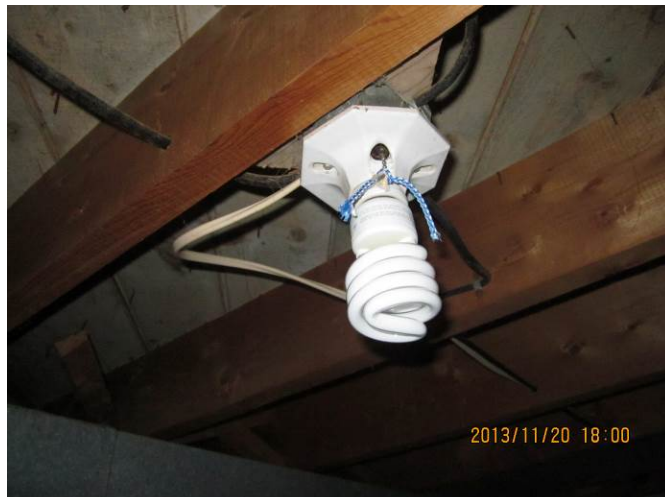
EL-015 – Compact fluorescent lamp used in other fixture in basement. Note the various wiring.
