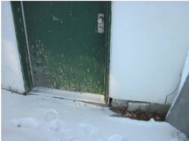
AR-007 – Deteriorated paint finish at door.
