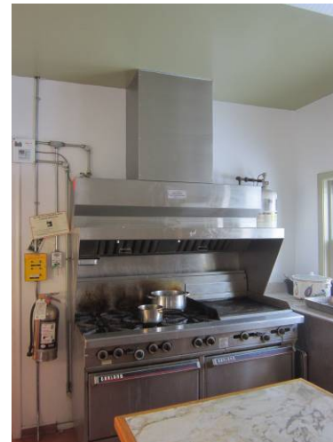
EL-016 – View of kitchen stove with junction box above.
