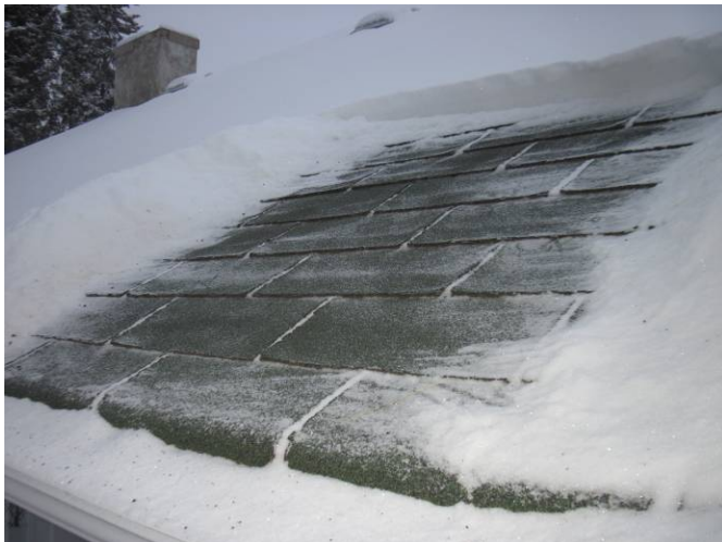
AR-007 – Initial deterioration of asphalt shingles.
