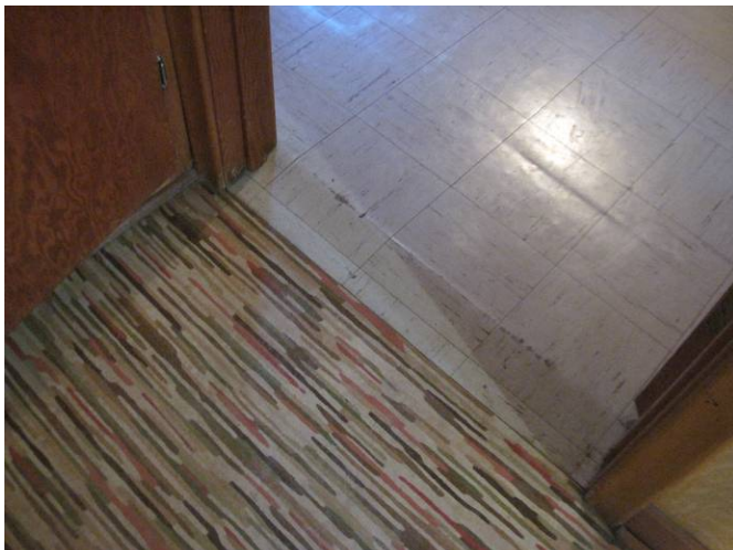
AR-007 – Suspect ACM flooring at basement bedroom/corridor.
