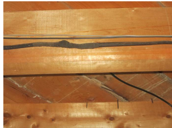
EL-008 – View of electrical splice made without junction box.
