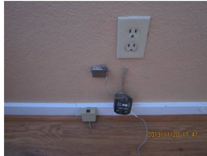
EL-022 – One of the telephone outlets in building
