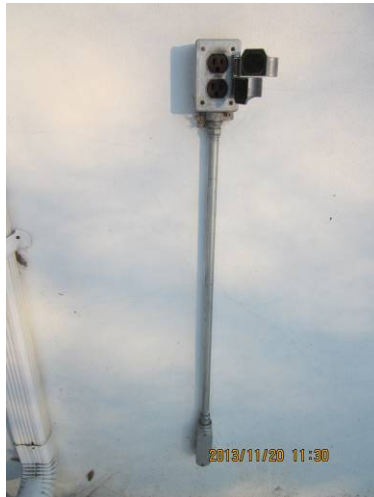
EL-013 – Exterior receptacle to be replaced with GFCI and rainproof cover.
