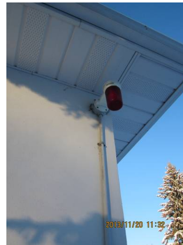
EL-024 – Indicator light for sewage system.
