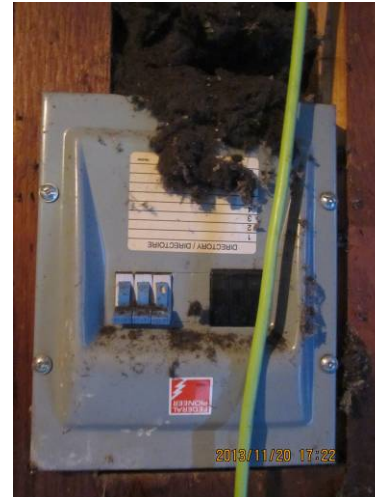
EL-002 – Branch circuit panel recessed in around combustible material.
