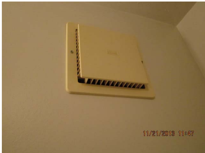
ME-011 – Wall mounted exhaust fan.
