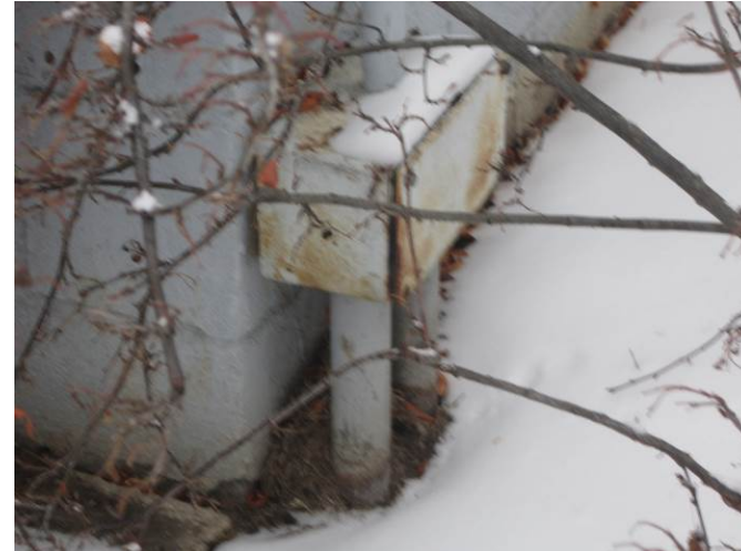
EL-002 – Incoming service junction box showing signs of deterioration, with opening in side allowing water penetration.
