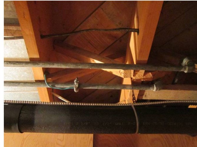
EL-006 – Poor and ineffective electrical grounding of installation. Point of termination needs to be cleaned and conductor secured.
