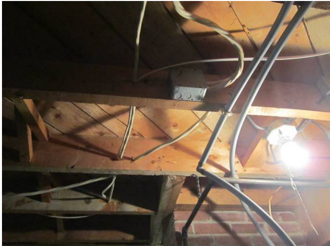
EL-005 – New and old wiring with cable clips required as per code.
