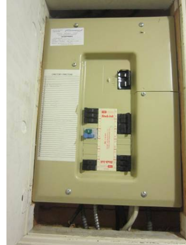
EL-004 – Incomplete panel directory and some of the wiring materials used.
