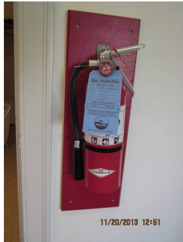
ME-025 – Fire extinguisher.
