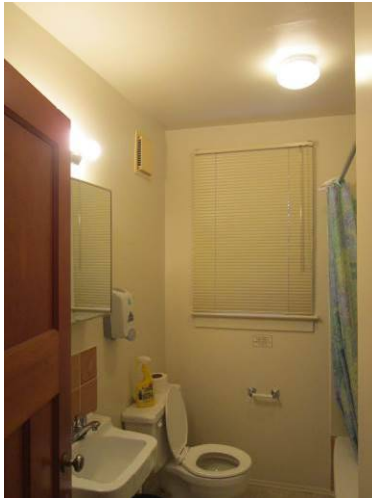
EL-017 – Interior lighting in washroom.
