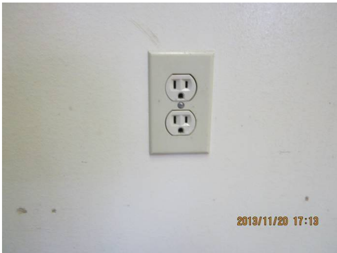
EL-007 – Flush mounted receptacle mounted in one half of the building.
