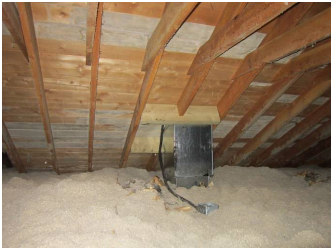
EL-015 – Open junction box above kitchen stove with missing cover plate.
