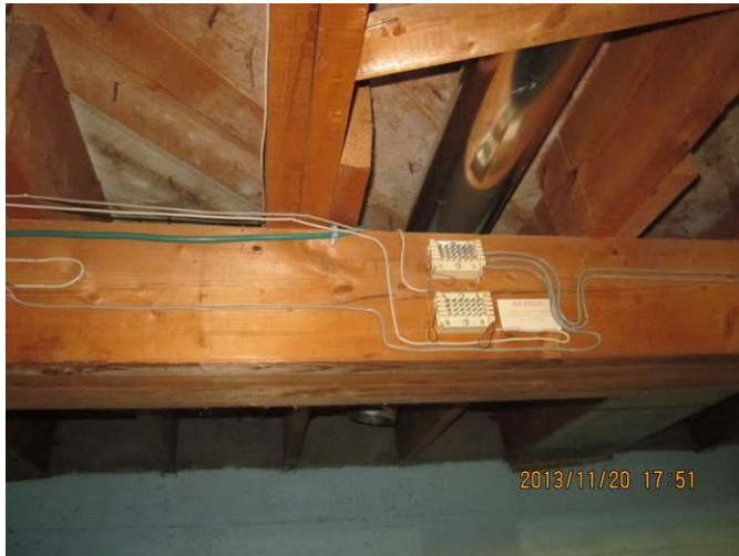
EL-021 – Internal telephone wiring in basement.
