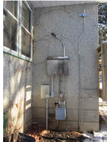
EL-002 – Incoming services to an exterior disconnect and branch circuit panel, all of which needs to be removed and installation rewired and placed indoors.
