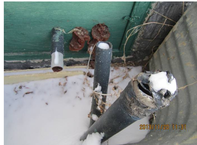
EL-012 – Abandoned conduits to be removed, cut off and holes fire stopped.
