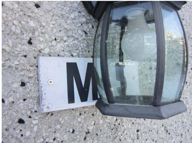
EL-025 – Exterior carriage lighting at the front and rear entrance of building.
