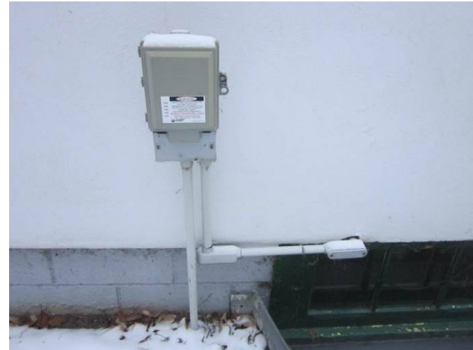
EL-022 – Telephone junction box provided by AGT.
