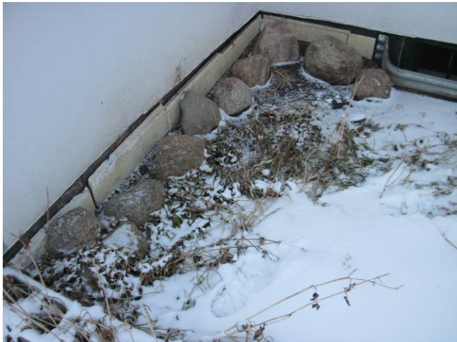
AR-003 – Exposed and deteriorating insulation at foundation perimeter.
