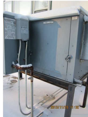
EL-014 – Exterior exhaust fan with local disconnect to be labelled.
