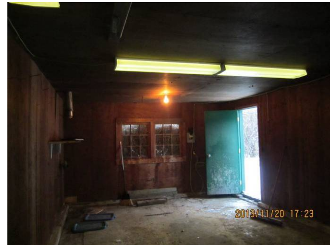
EL-008 – View of interior lighting in garage.
