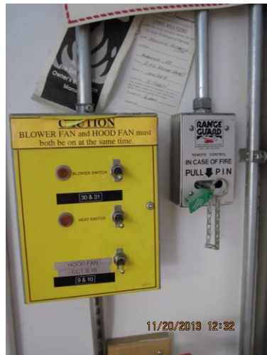
ME-019 – Exhaust fan and make-up air control switches.
