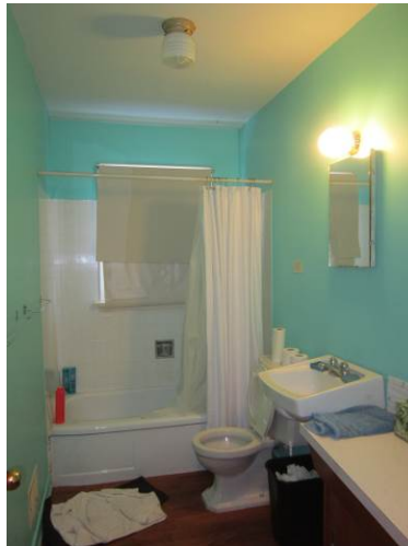
EL-021 – Interior lighting of bathroom.
