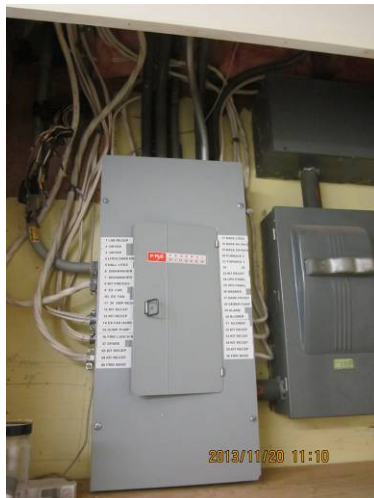
EL-003 – Frontal view of branch circuit panel showing panel disconnect.
