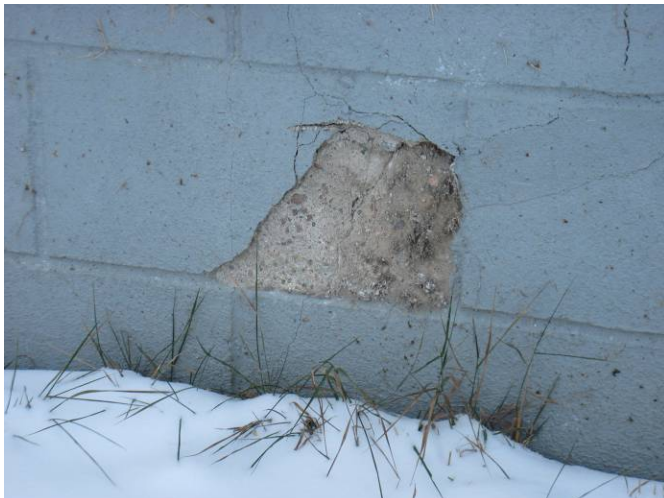
AR-003 – Area of deteriorated concrete at foundation wall exterior surface.
