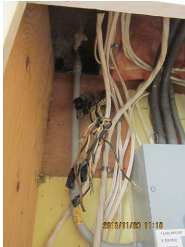
EL-005 – Condition of some of the wiring left hanging by the panel.
