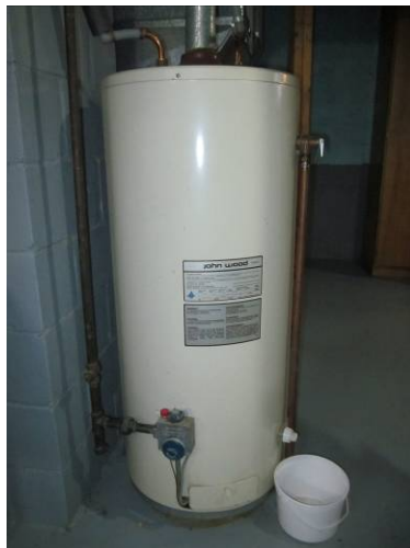
ME-019 – Gas fired hot water tank.
