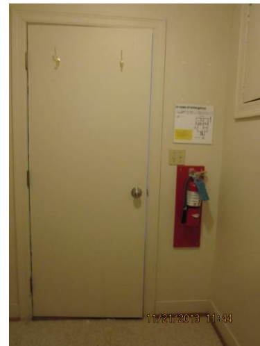
ME-020 – Fire extinguisher.
