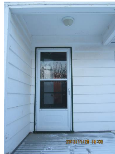
EL-024 – Exterior lighting at front of building.
