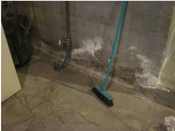
AR-003 – Efflorescence at foundation wall and cracked concrete floor.
