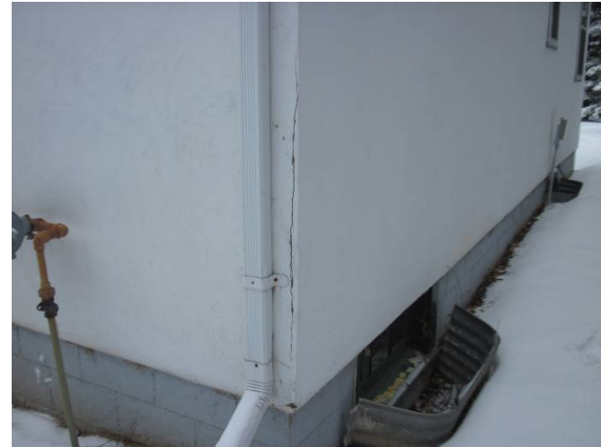
AR-006 – Deteriorated stucco finish.
