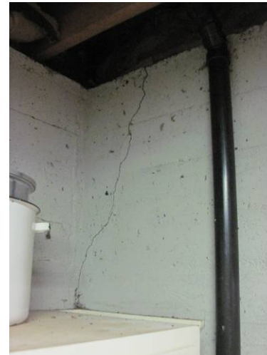
AR-004 – Crack in foundation wall below main entrance.
