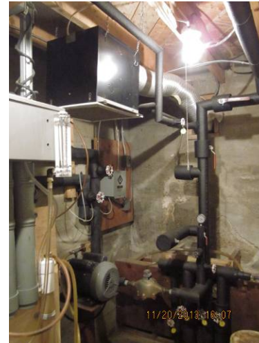
ME-022 – Water distribution.
