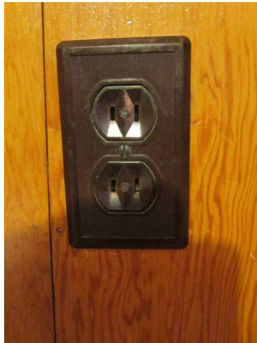
EL-013 – An old two wire duplex receptacle without ground terminal still in use.
