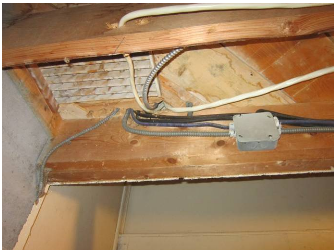
EL-007 – Cable drilled too close to bottom of beam requires mechanical protection or re-routing.
