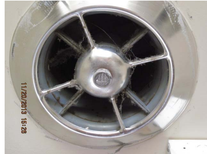
ME-026 – Kitchen exhaust fan.
