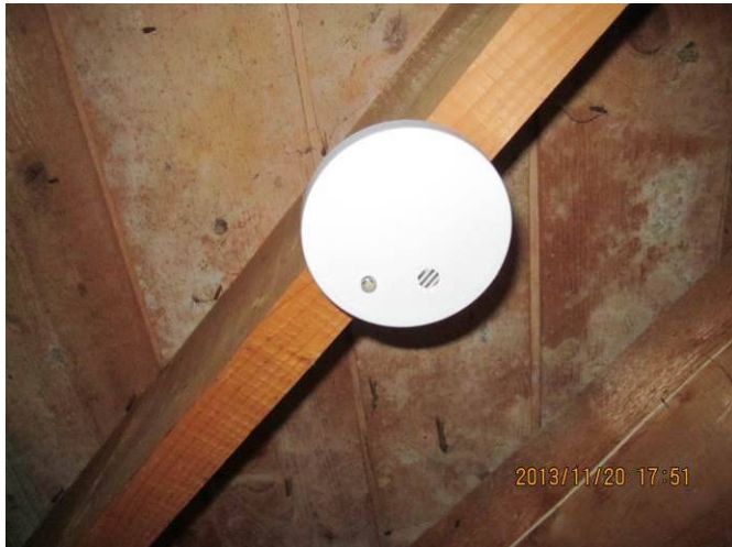
EL-017 – Smoke alarm to be interconnected.
