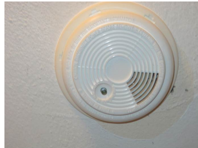
EL-024 – View of non-working 120 volt smoke alarm, all of which are to be interconnected.
