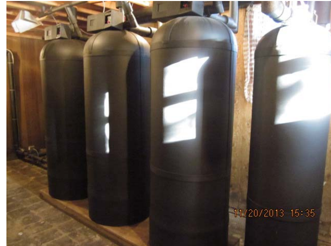
ME-018 – Water treatment system.
