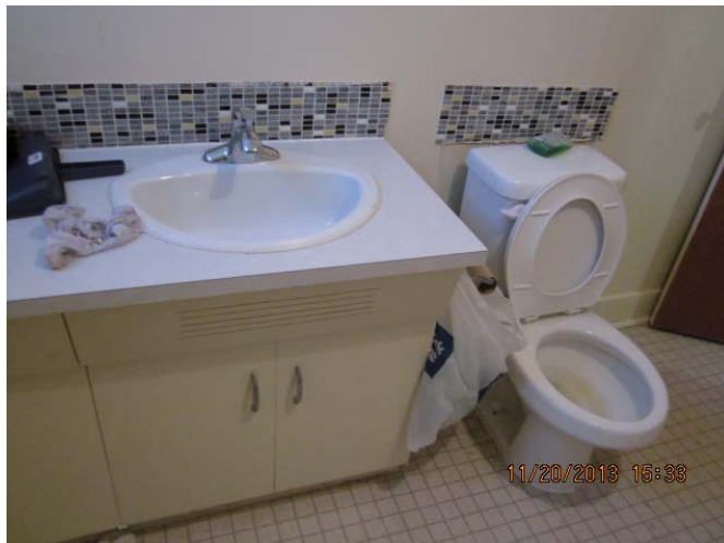
ME-015 – Plumbing fixtures.
