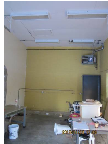
EL-012 – Interior lighting and door leading to the exterior.
