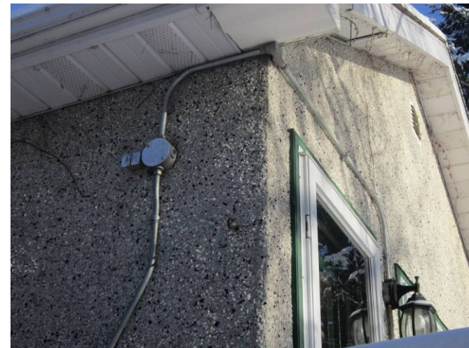
EL-028 – View of photocell that controls exterior lighting
