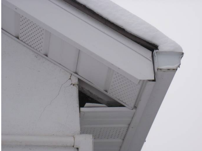
AR-007 – Missing metal soffit piece providing opening to attic space.
