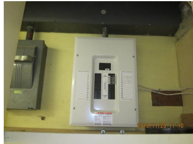
EL-004 – View of a more recent branch circuit panel.
