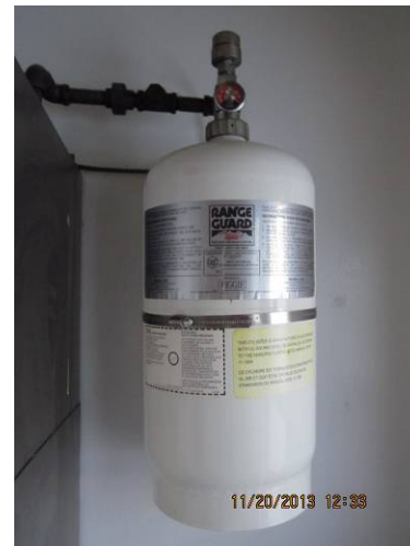
ME-020 – Fire extinguisher cylinder.
