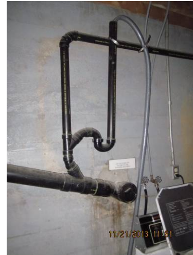
ME-014 – Sanitary piping.
