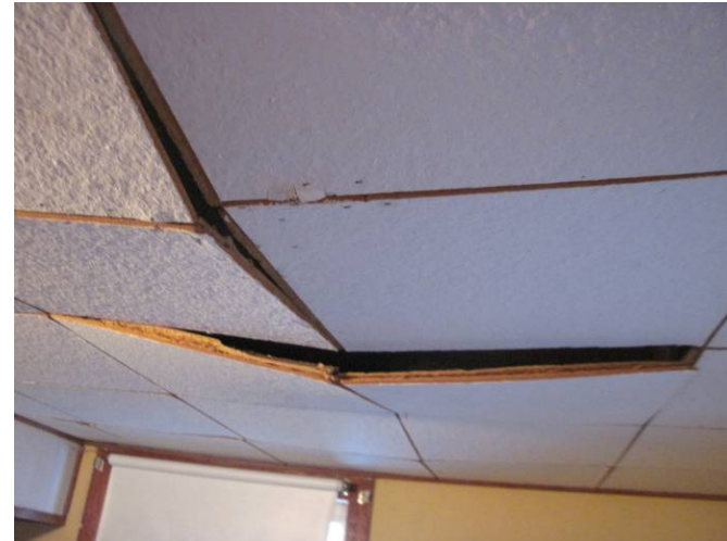
AR-010 – Ceiling falling down in basement bedroom.
