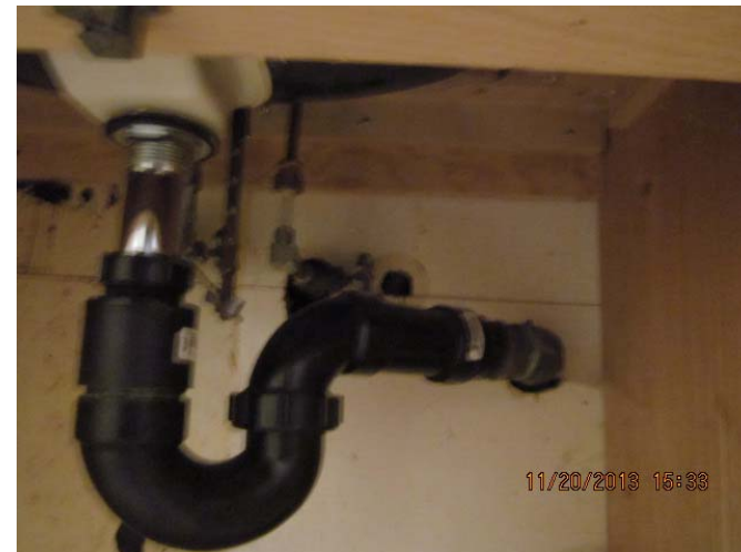
ME-016 – Piping and drainage.
