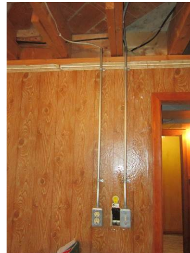
EL-012 – Surface mounted outlets wired with non-metallic sheathed cables in conduit, lacking mechanical protection in ceiling.
