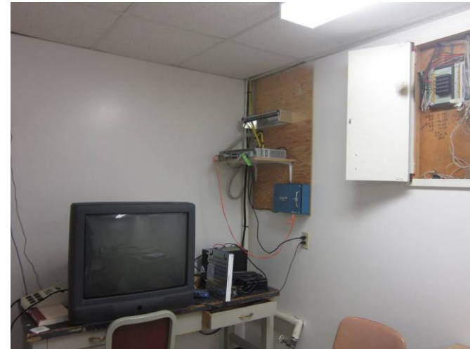
EL-030 – View of data equipment for site and location of telephone junction box.
