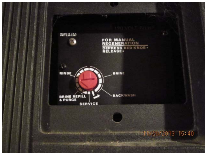
ME-019 – Water treatment control.
