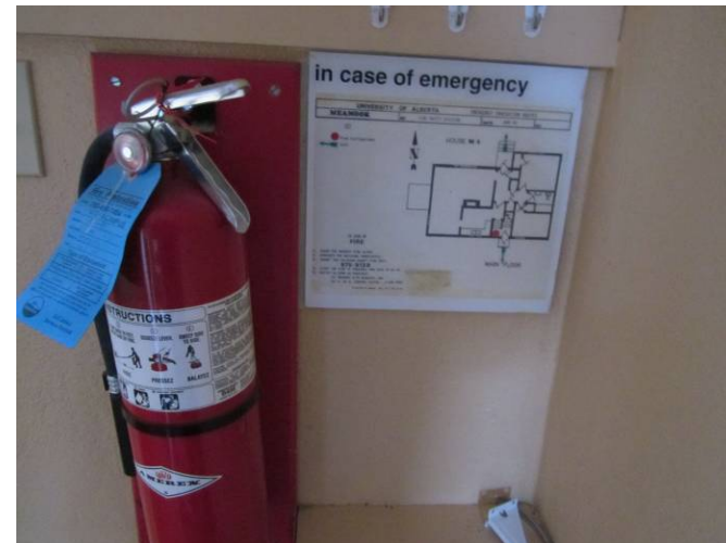
ME-020 – Fire extinguisher.
