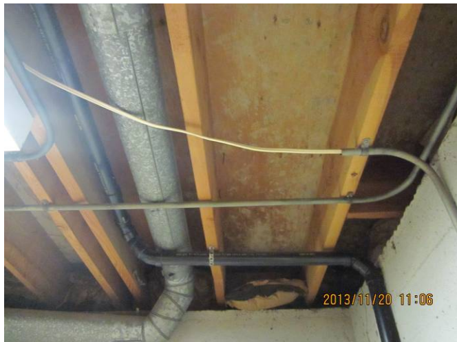
EL-007 – Cable run in conduit without insuliner or mechanical protection, and cable resting on heating duct.
