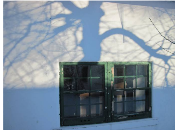
AR-010 – Deteriorated paint finish at window.
