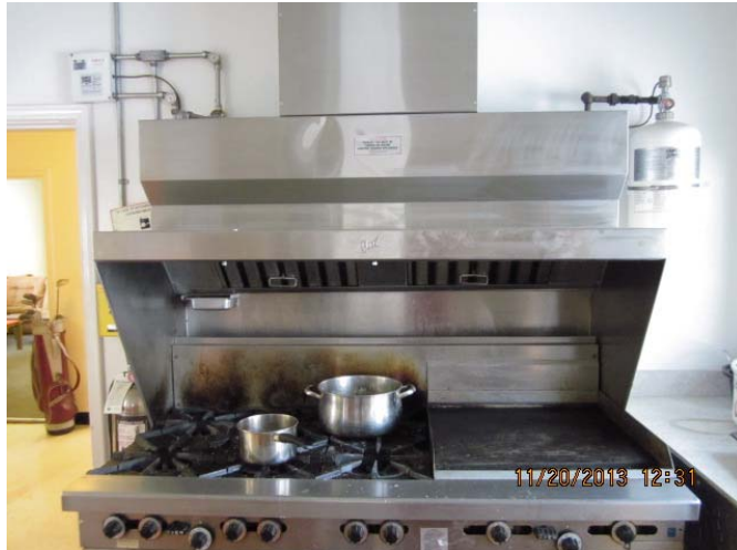
ME-017 – Commercial stove and range hood.
