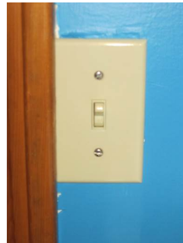
EL-012 – Wall mounted toggle switch used in the building.
