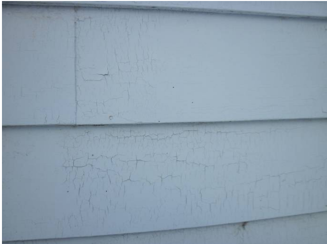
AR-005 - Deteriorated paint finish at exterior wall.
