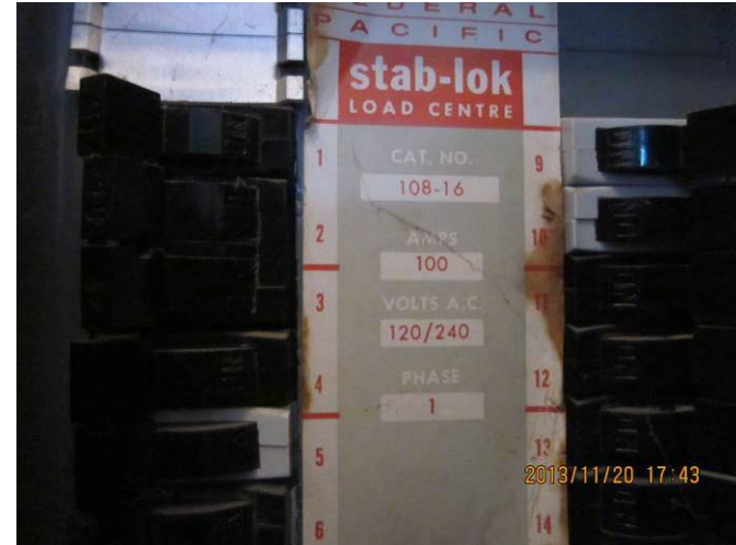
EL-006 – Frontal view of branch circuit panel showing old and new circuit breakers.
