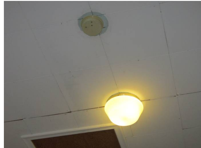
EL-026 – A different style of smoke alarm all to be replaced and interconnected when installing new units.
