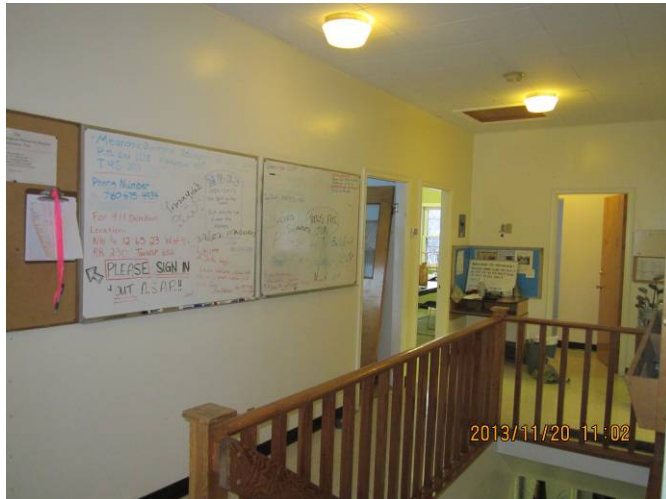
EL-021 – Decorative dome style light fixtures using incandescent and compact fluorescent lamps.
