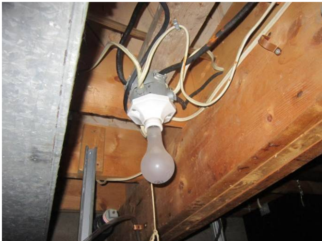
EL-007 – View of an undersized outlet box with various types of wiring and a pendant fixture with an oversized incandescent lamp.
