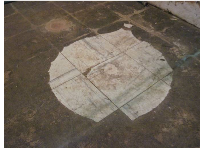
AR-006 – Deteriorated flooring in basement service area.
