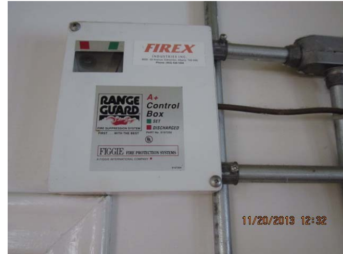
ME-018 – Range guard control box.
