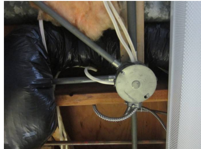
EL-006 – View of an undersized junction in ceiling.
