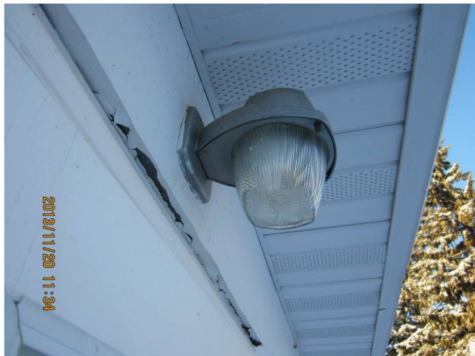
EL-023 – Exterior high intensity discharge (HID) fixture.
