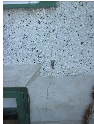
AR-004 – Crack and minor deterioration of stucco finish.
