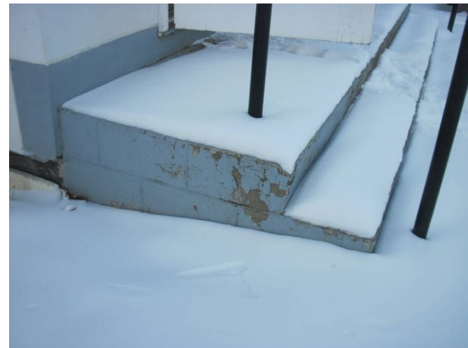
AR-008 – Deteriorated paint finish at concrete entrance landing/steps.
