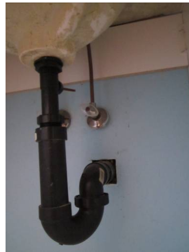
ME-012 – Piping and drainage.
