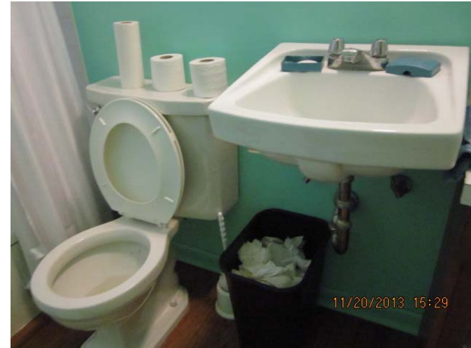
ME-010 – Plumbing fixtures.
