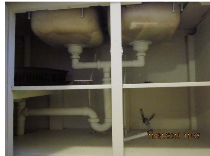
ME-008 – Plumbing and drainage.
