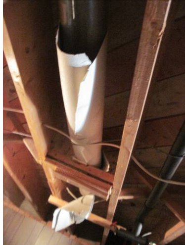
AR-011 – Basement view of suspect ACM duct-wrap paper.
