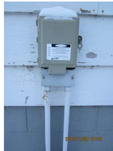
EL-020 – Telephone junction box provided by AGT.
