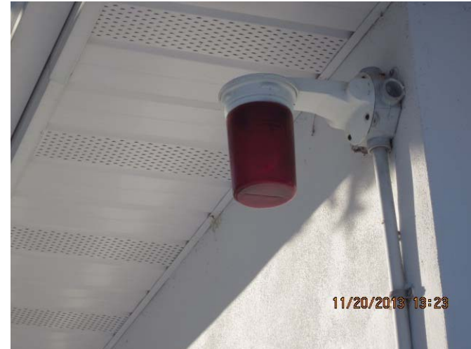
ME-026 – Strobe light - septic tank monitor.
