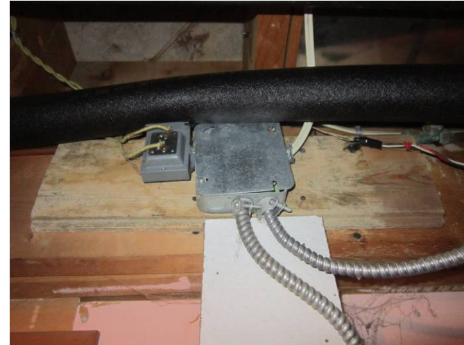
EL-010 – Metallic sheathed cables with low voltage wiring and junction box that could not be properly closed; cable supports needed.
