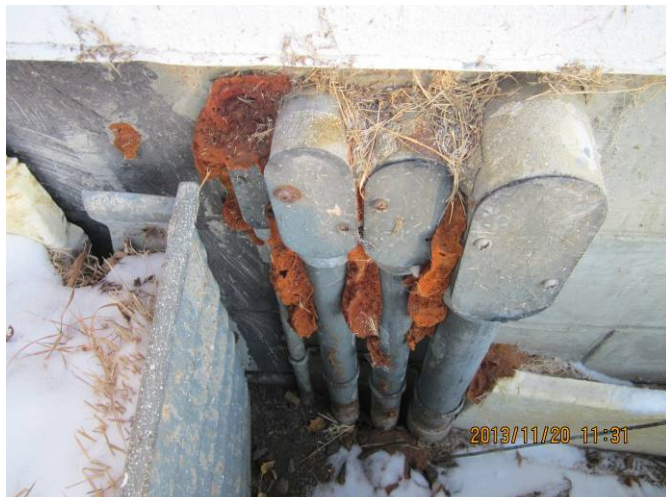
EL-011 – Conduits penetrating wall presently sealed with mono foam is deteriorating, a certified fire retardant material must be used.
