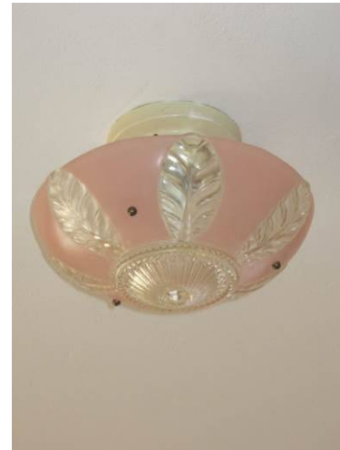
EL-018 – Interior decorative light fixture utilizing incandescent lamp.
