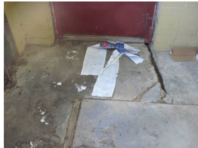
AR-004 – Cracked/shifted foundation at southwest corner.
