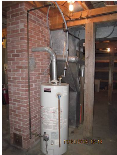
ME-017 – Hot water heater.
