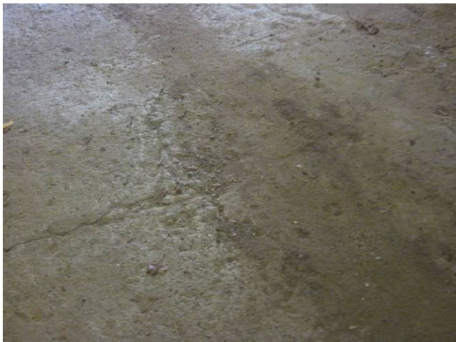
AR-003 – Cracked/pitted concrete floor surface.
