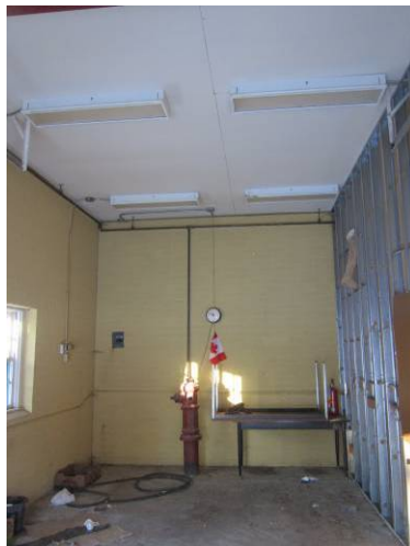
EL-011 – Interior lighting.
