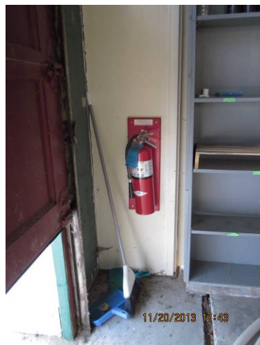
ME-007 – Portable fire extinguisher.
