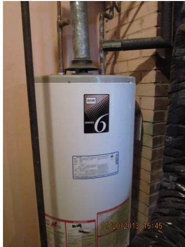
ME-025 – Hot water tank.
