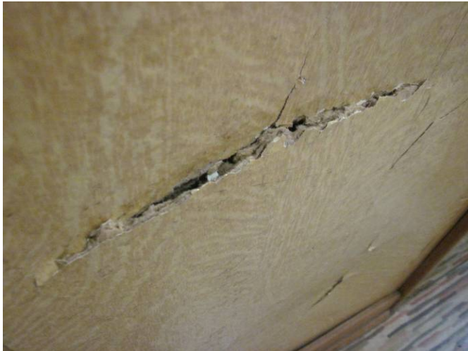
AR-009 – Damaged basement wall in basement corridor.
