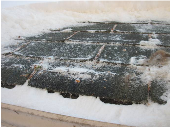
AR-009 – Deteriorating asphalt shingles.
