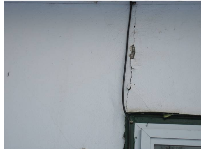
AR-006 – Cracked/broken stucco finish.
