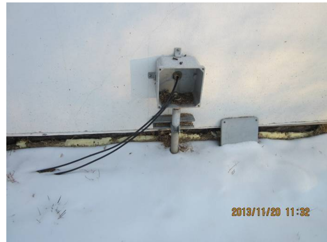
EL-028 – Cables to be installed properly and junction box closed.
