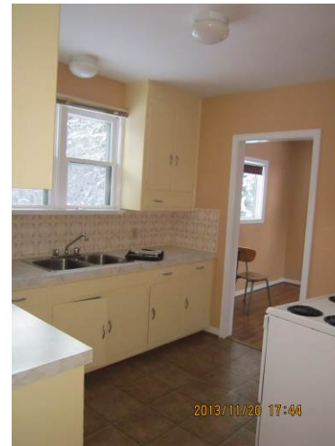
EL-012 – Interior lighting in kitchen.
