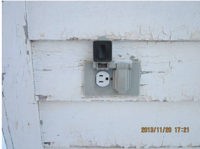
EL-005 – Exterior receptacle to be replaced with GFCI.
