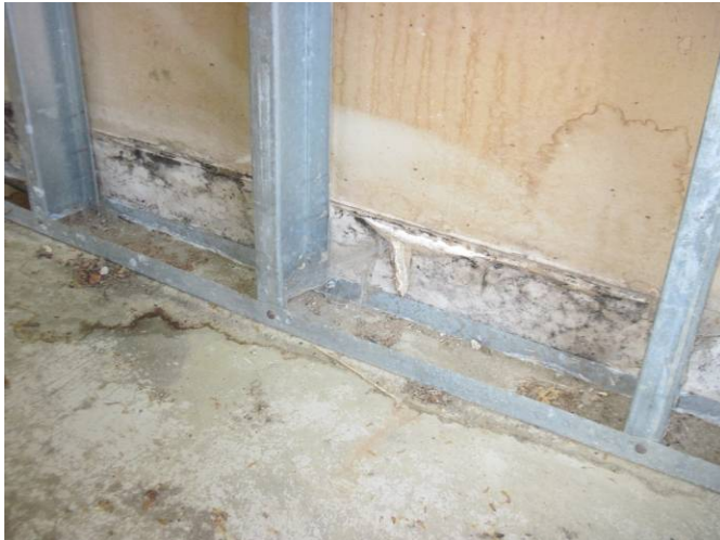
AR-009 – Suspect mould along bottom of interior partition.
