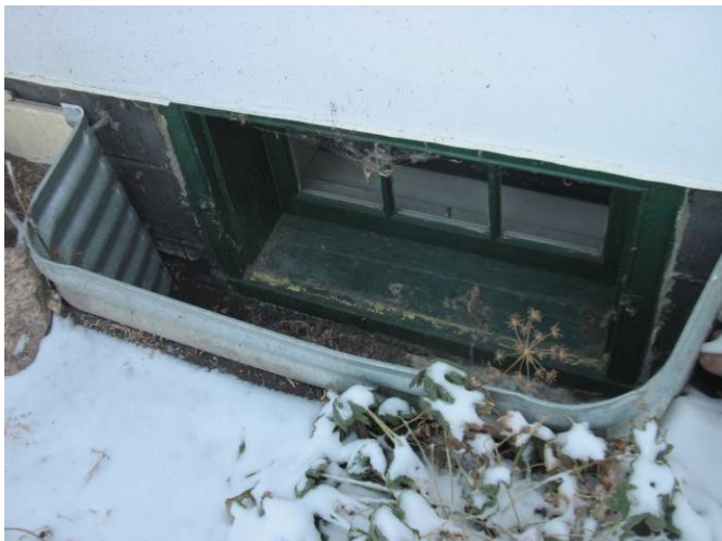
AR-007 – Deteriorated paint finish at wood window, and uninsulated portion of foundation wall.
