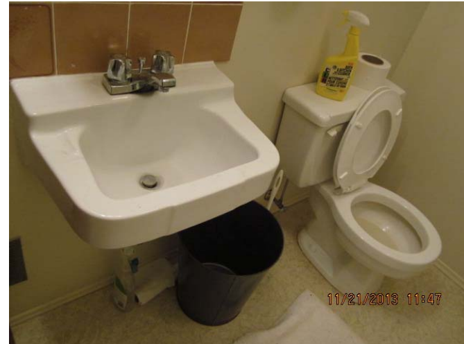
ME-010 – Sink and toilet.
