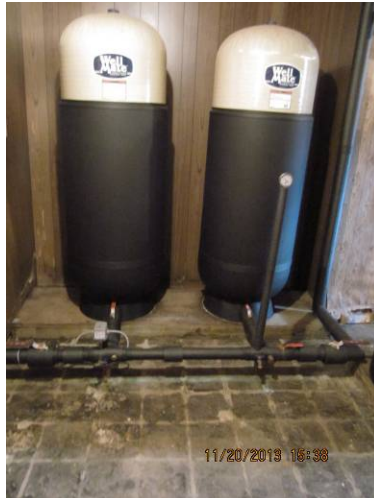
ME-017 – Water treatment system.
