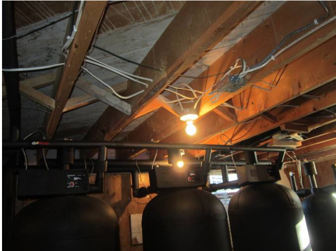
EL-009 – Open junction box without cover plate and a pendant light fixture utilizing incandescent lamp.
