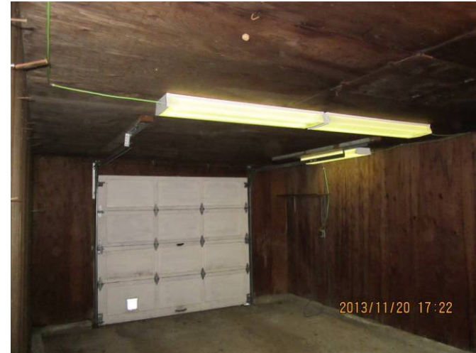
EL-006 – View of extension cord used to wire through light fixtures running across ceiling.
