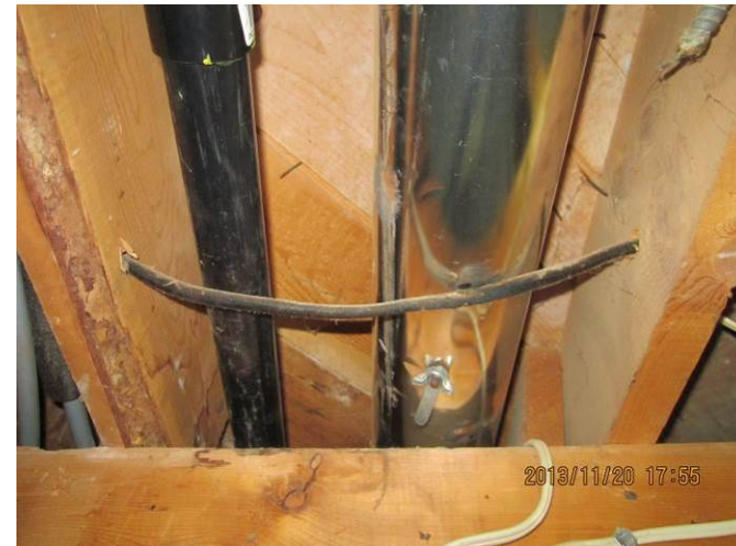
EL-008 – Section of electrical wiring pressing against the heating duct to be protected and various types of wiring shown.
