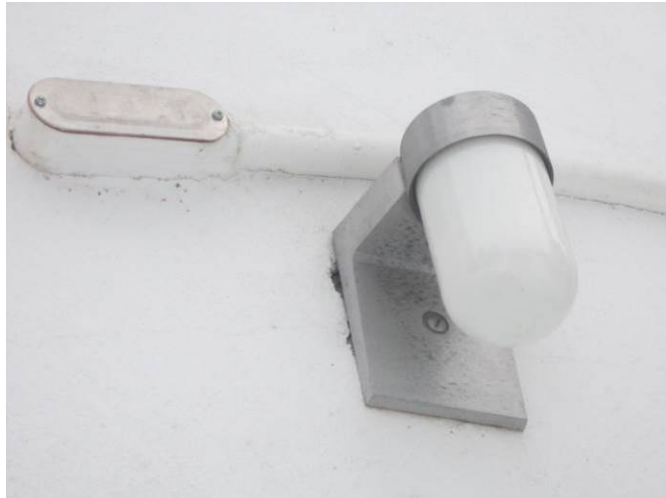
EL-013 – Exterior lighting at rear of building.
