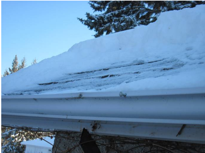
AR-005 – Initial deterioration of asphalt shingles.
