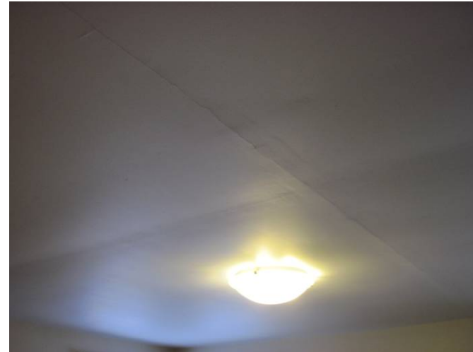
AR-010 – Cracked gypsum board at ceiling.
