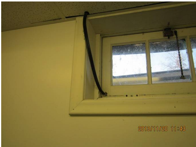
EL-027 – Cable to be re-routed removed from window casing.
