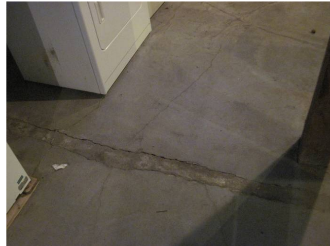
AR-004 – Area of unstable concrete floor.
