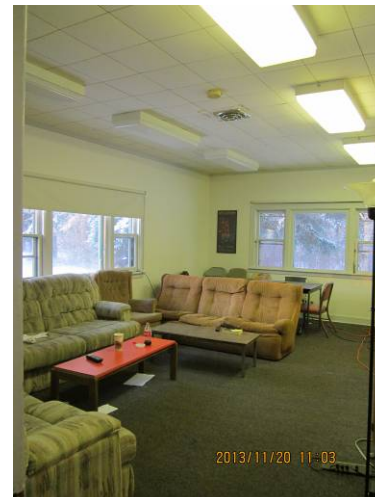
EL-020 – Three-lamp ceiling wrap-around fluorescent fixtures.
