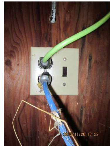
EL-004 – Receptacle used to feed light fixtures with old non-metallic sheathed cable running above switch.
