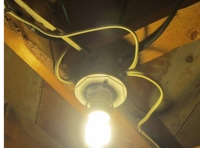
EL-020 – View of junction box that is undersized for the number of cables allowed.
