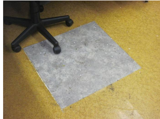
AR-014 – Patched floor finish in office.
