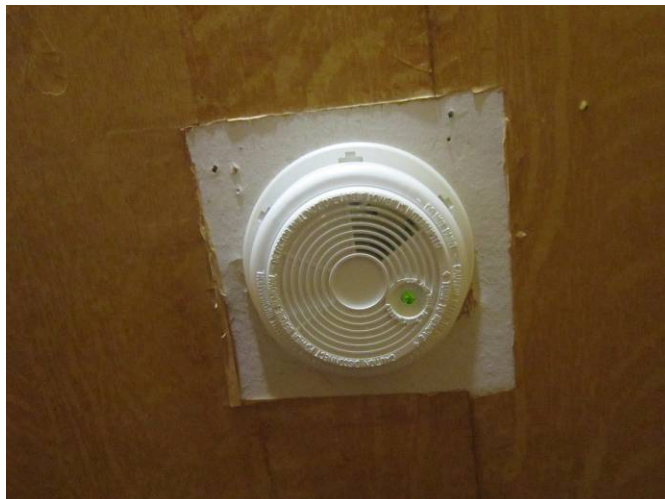
EL-023 – View of 120 volt working smoke alarm.
