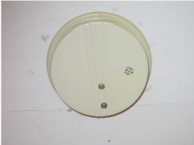
EL-021 – Smoke alarm on main floor only.
