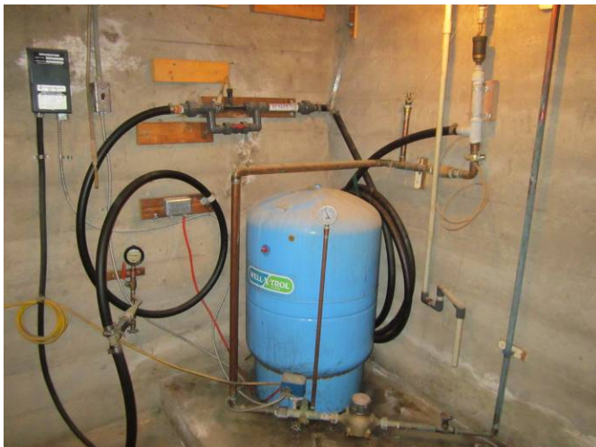
ME-015 – Water supply system.
