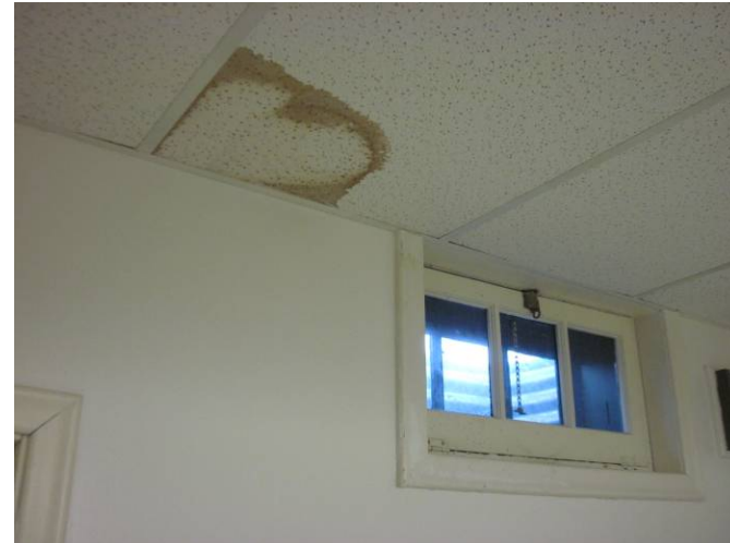
AR-010 – Water stained/damaged tile at basement ceiling below main entrance.
