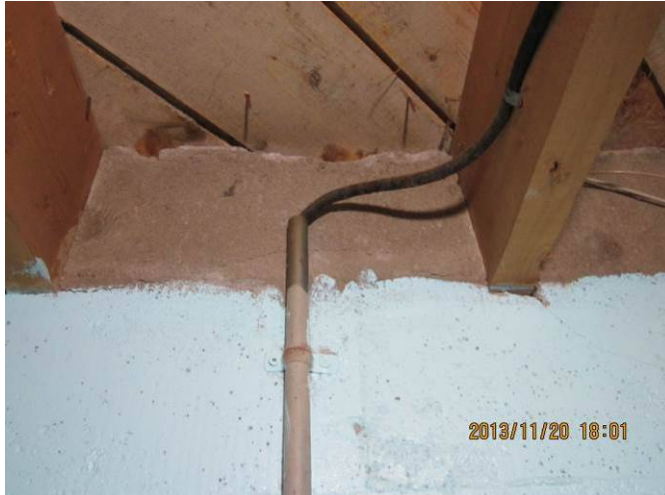
EL-009 – Protective bushing required to prevent damage to non-metallic sheathed cables.
