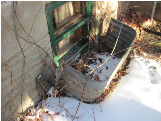
AR-003 – Basement bedroom window and well, shifted and not code compliant.
