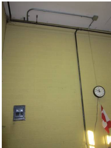
EL-003 – Branch circuit panel recessed in block wall.
