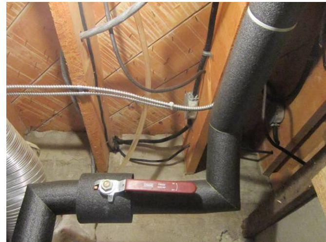
EL-008 – Various types of wiring with mechanical protection needed for wires penetrating floor and an inaccessible junction box.
