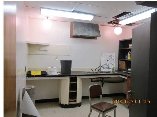
EL-022 – Lighting in Lab.
