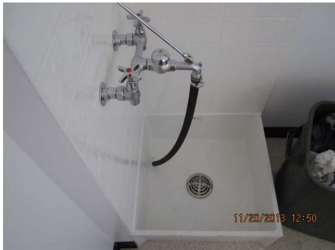
ME-011 – Slop sink - faucet with built-in vacuum breaker.
