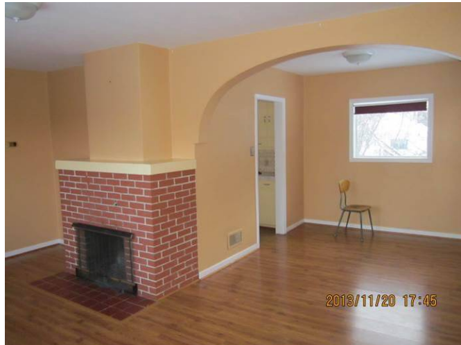
EL-013 – Interior lighting in living and dining area.
