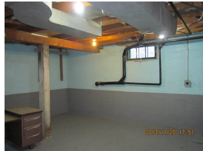
EL-016 – Incandescent lighting in basement.
