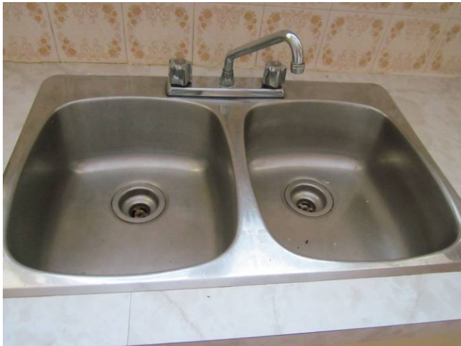
ME-007 – Kitchen sink and faucet.
