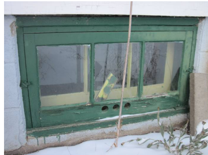
AR-008 – Deteriorated paint finish at window.
