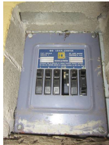
EL-004 – Frontal view of branch circuit breakers.
