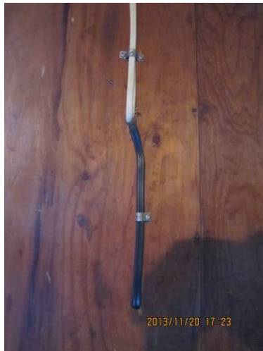
EL-007 – Cables used to wire outside light fixture without junction box.
