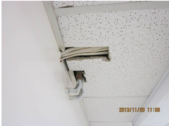
EL-009 – Cables run below ceiling without mechanical protection.
