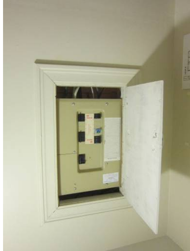
EL-003 – Branch circuit panel recessed in wall at main entrance.
