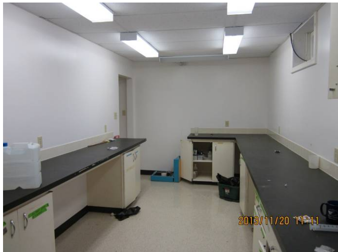
EL-019 – Two-lamp ceiling mounted, wrap-around fluorescent fixtures and cable run through window casing.
