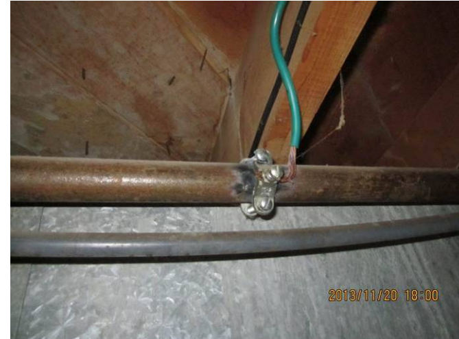
EL-010 – Ground conductor not effectively connected to ground; see area burnt due to short circuit, to be completed.
