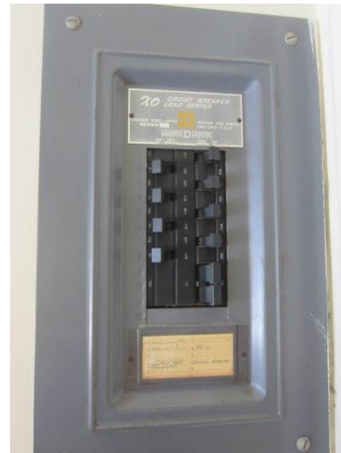
EL-004 – Recessed branch circuit panel in rear entrance hallway with incomplete panel directory and very old circuit breakers.
