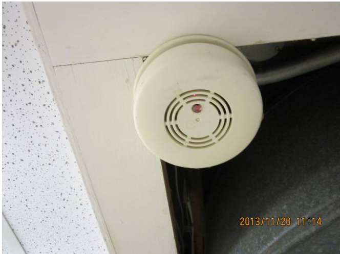
EL-025 – 120 volt smoke alarm to be replaced with combined smoke and carbon monoxide units and dual voltage.
