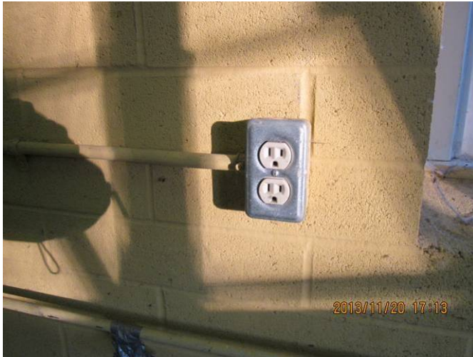
EL-005 – One of the many surface mounted receptacles.
