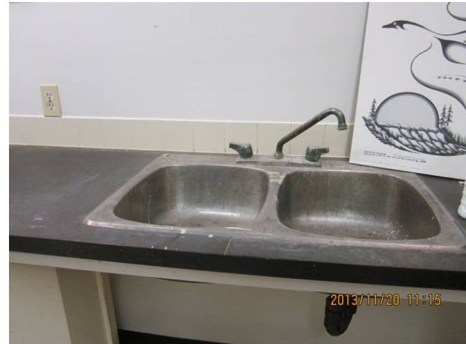
EL-010 – Receptacles within 1 m of sinks to be replaced with GFCI.
