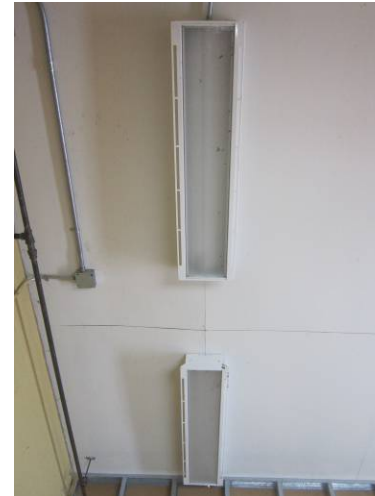
EL-010 – Interior lighting in the other half of the building.
