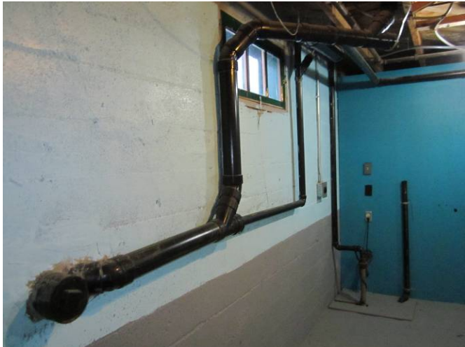
ME-013 – Sanitary sewer.
