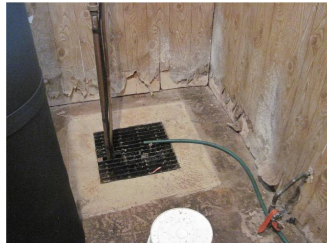
AR-008 – Deteriorated wall finish at basement service area.
