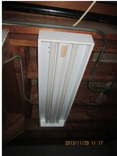
EL-017 – View of fluorescent fixture with T12 lamps and magnetic ballasts.
