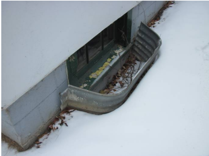
AR-005 – Shifted window well.
