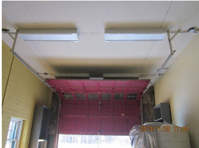
EL-009 – Interior lighting in one half of the building.
