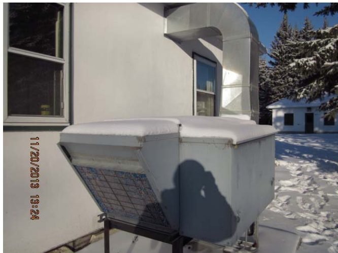
ME-027 – Make-up air handling unit.
