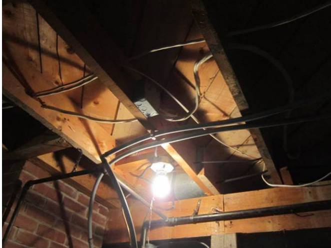
EL-019 – General wiring and lighting in basement.
