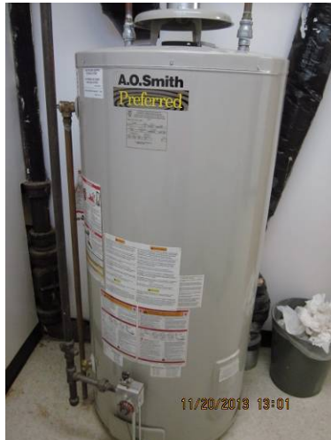
ME-009 – Hot water tank.
