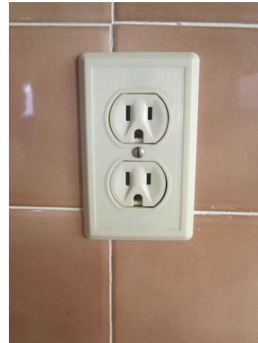
EL-014 – A three wire duplex receptacle with ground terminal.
