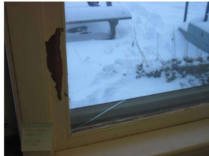
AR-012 – Damaged paint finish and broken glass at window.
