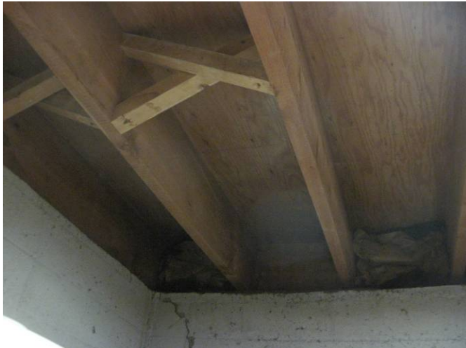
AR-005 – Uninsulated portions of rim joist.
