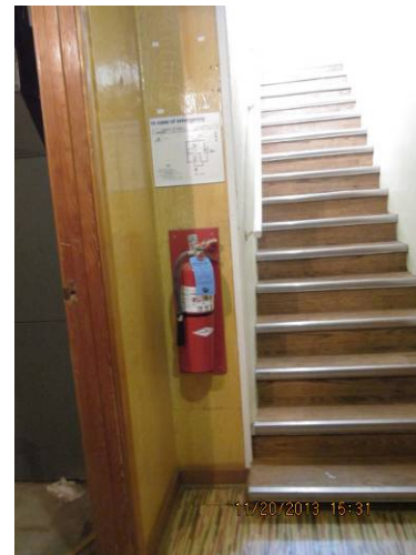
ME-028 – Fire extinguisher.
