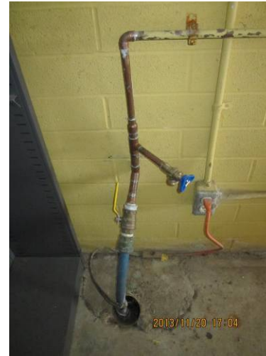
EL-006 – Outlet providing heat trace protection for water main.
