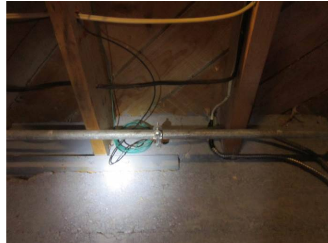
EL-006 – Electrical splice made without junction box between Romex and BX cable.
