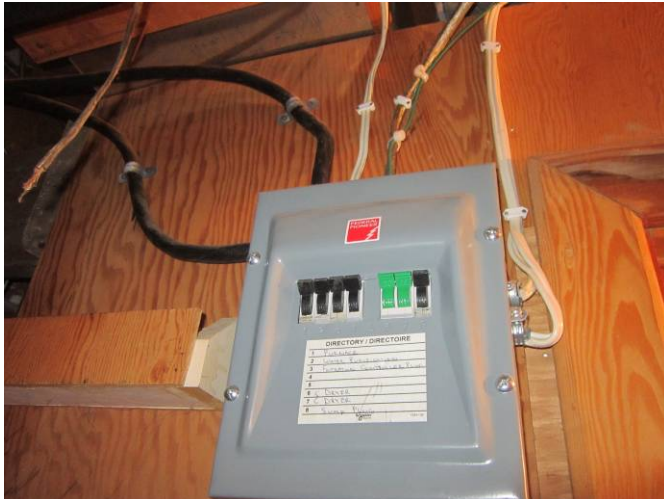
EL-005 – Additional sub-panel in basement mounted on wooden board and an abandoned cable.
