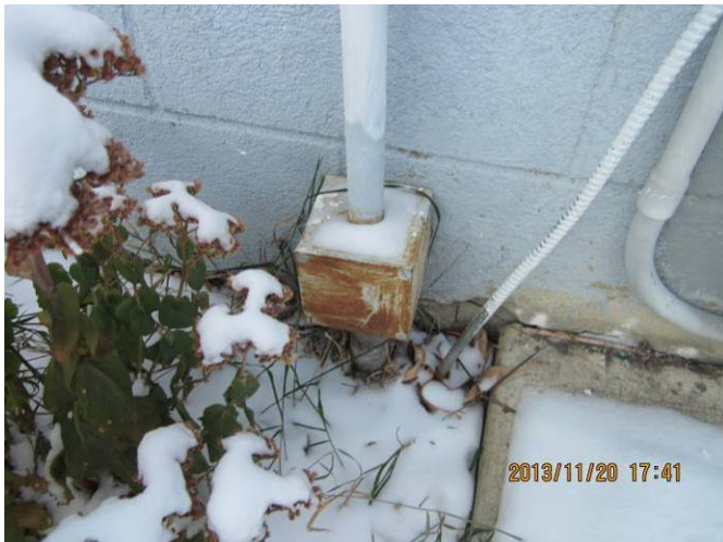
EL-003 – Main service junction box showing corrosion and metallic sheathed cable not design for outside use.
