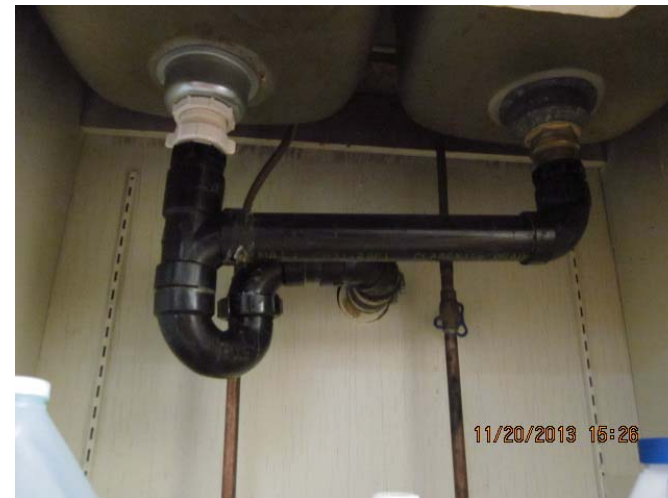
ME-008 – Piping and drainage.
