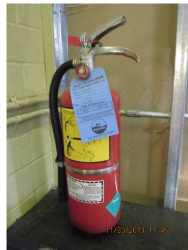
ME-008 – Portable fire extinguisher.
