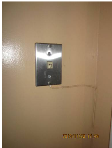
EL-023 – Wall mounted telephone outlet.
