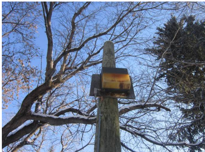
EL-027 – A close view and present condition of exterior pole mounted light with water penetration.
