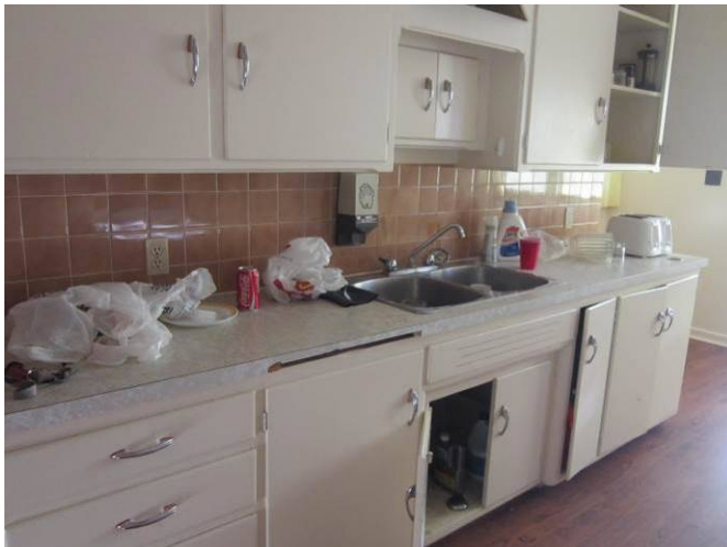
EL-015 – Receptacle within 1 M of kitchen sink to be replaced with GFCI.
