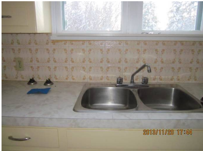
EL-011 – Receptacles within 1 m of sinks to be replaced with GFCI or install GFCI breakers in panel.
