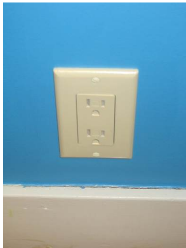
EL-011 – Type of receptacle used in building that are presently incorrectly wired.
