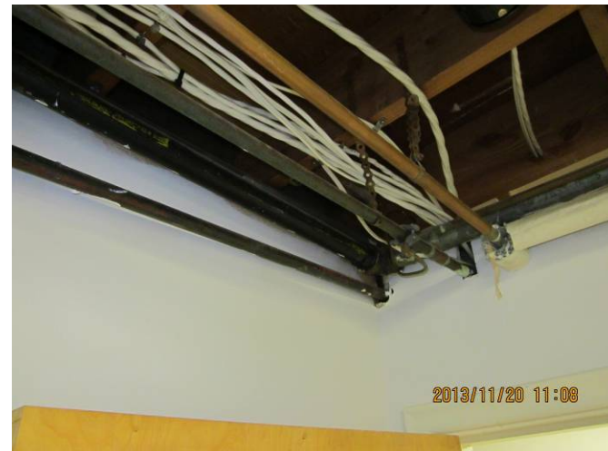
EL-008 – Cables bunched together and run through wall without mechanical protection and below ceiling joist.
