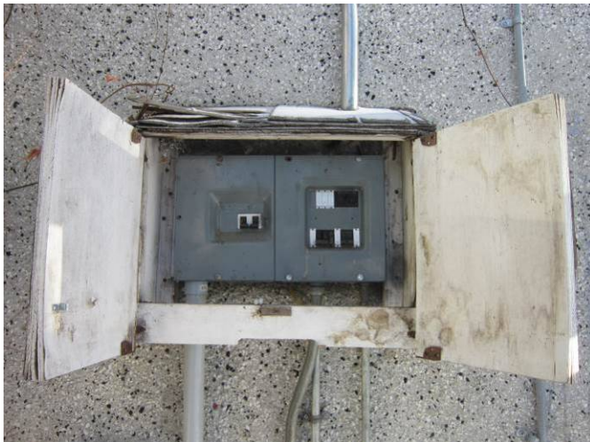
EL-003 – Frontal view and condition of exterior branch circuit panel without panel directory.
