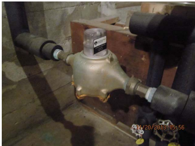
ME-023 – Water meter.
