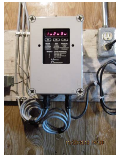
ME-020 – Water treatment control.
