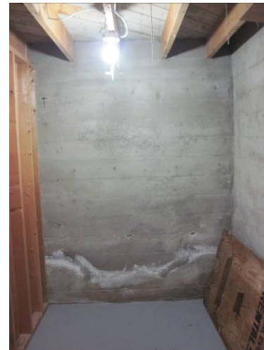
AR-004 – Localized efflorescence at interior surface of foundation wall.
