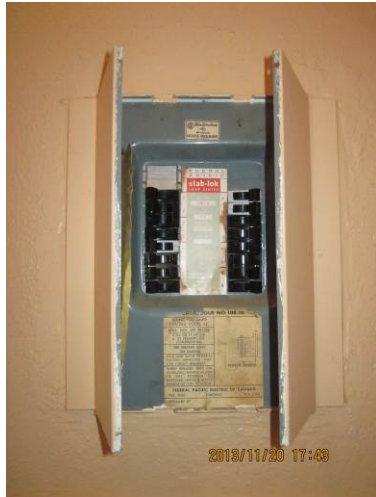
EL-005 – Branch circuit panel recessed in wall, with incomplete panel directory.
