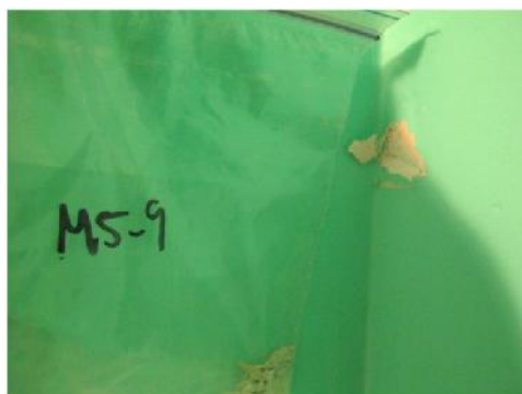
Photograph 77: Building M5- Sample #M5-9, Drywall Joint Compound None Detected
