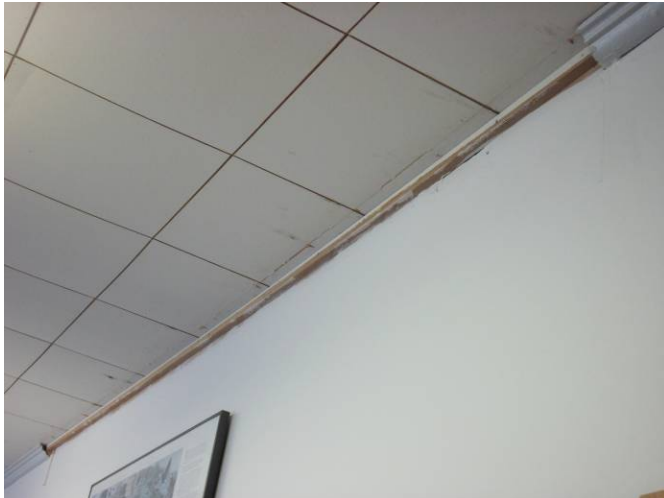
AR-013 – Missing fibreboard crown moulding in lounge.
