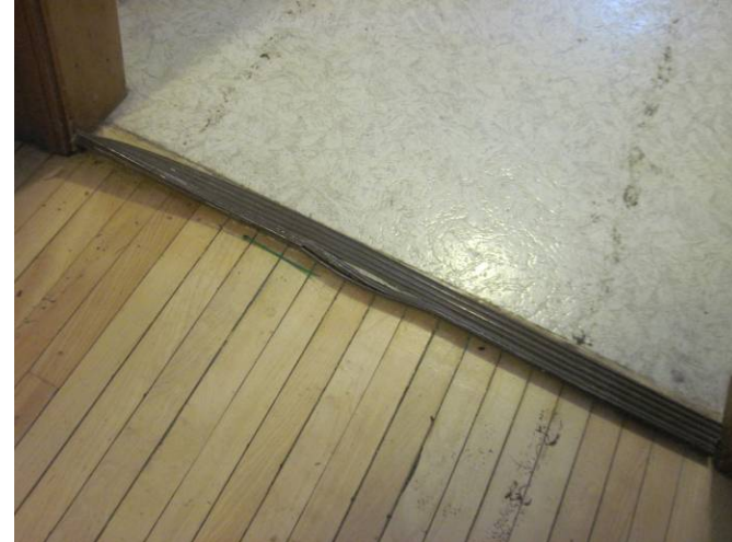
AR-008 – Damaged flooring termination strip.
