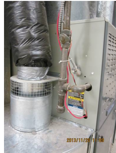
EL-018 – Missing rubber grommet for cables on furnace.
