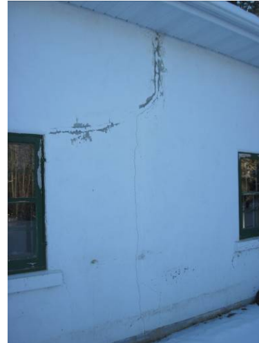
AR-006 – Cracks, including previous repairs, at stucco finish.
