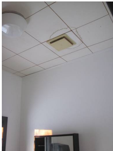
AR-011 – Water stained/damaged tile at ground floor washroom ceiling.
