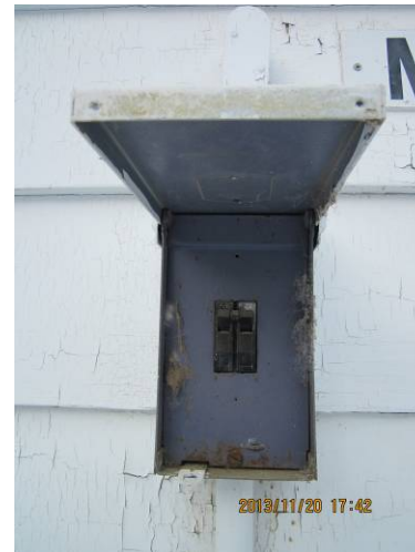
EL-004 – Main service disconnect on the exterior of building showing insect infestation.
