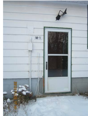
EL-002 – Incoming service, with BX and conduit installation outdoors in poor condition.
