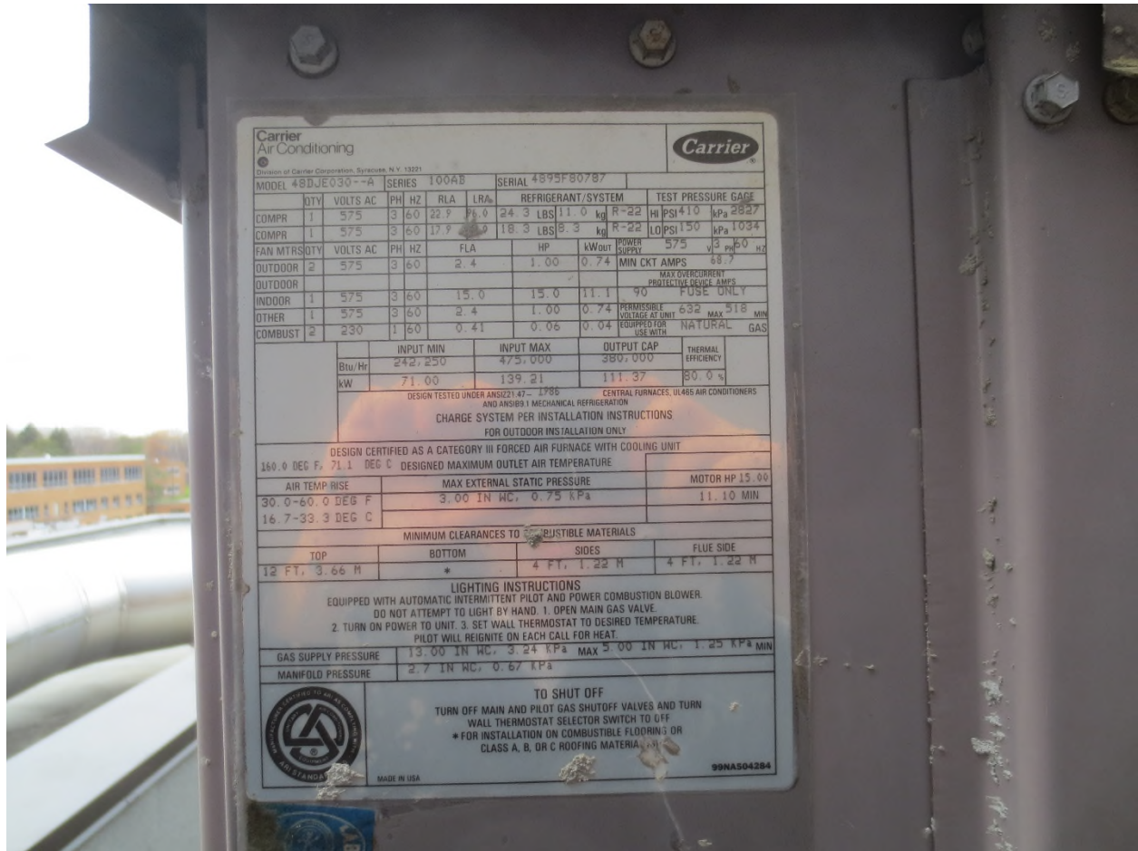
Existing RTU #3 nameplate
