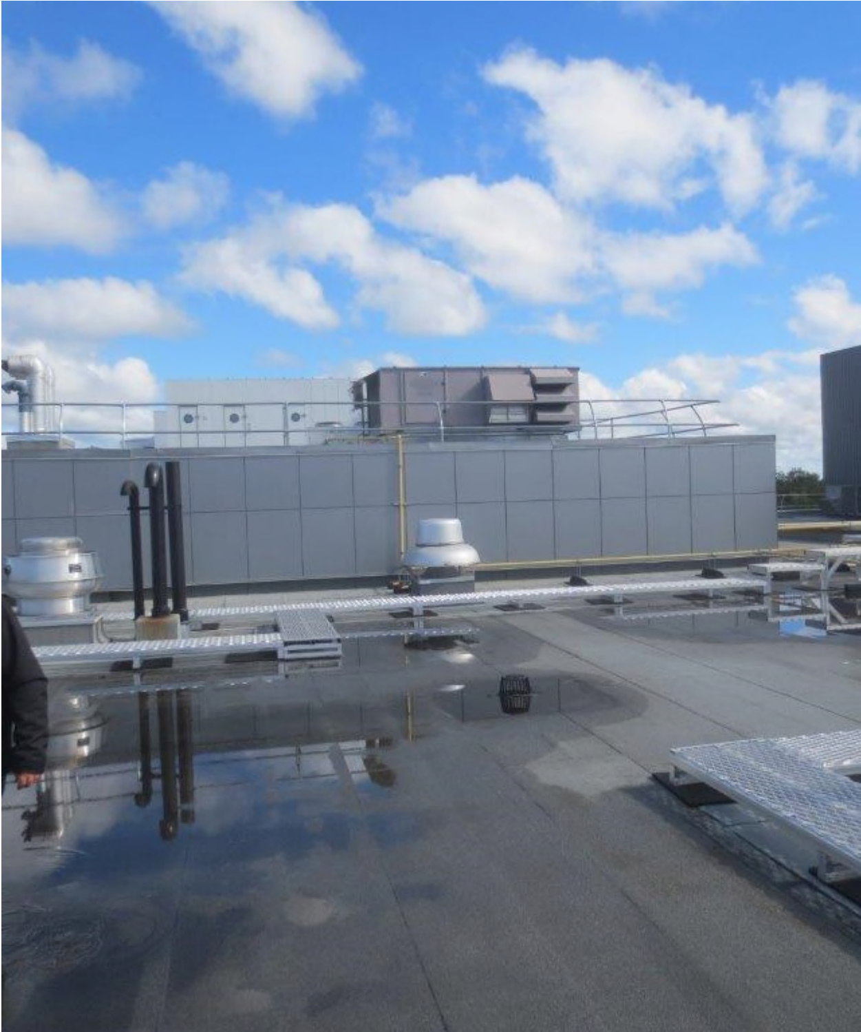
Existing RTU #1 Overview
