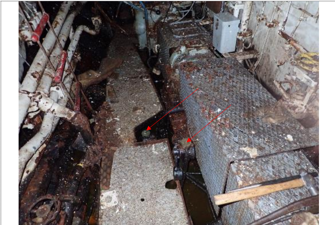
30. CPP and gear oil storage tank sounding pipes – tanks found full of clean lube oil
