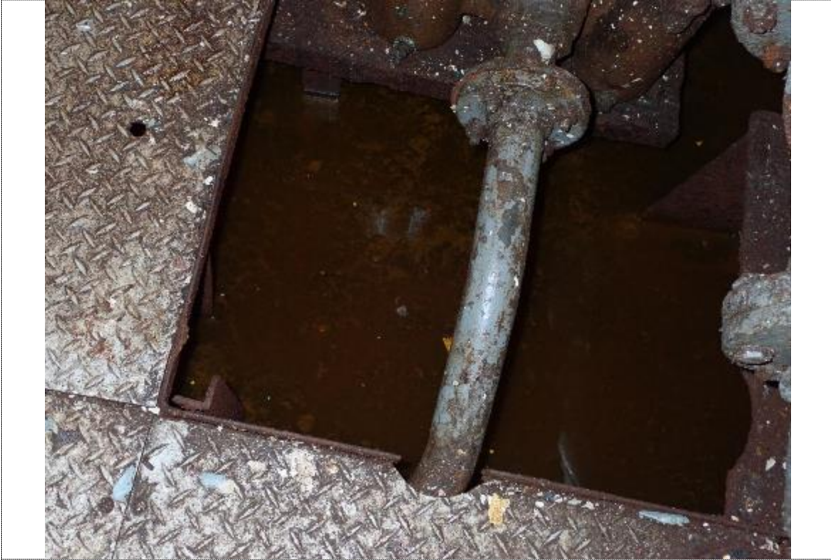
27. Main propulsion room bilges – approx. 50mm emulsified oil on top of water
