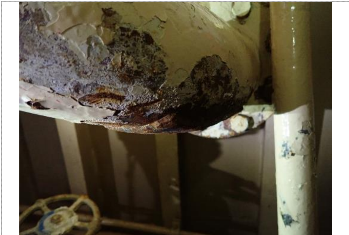
34. Patched overboard line starting to weep
