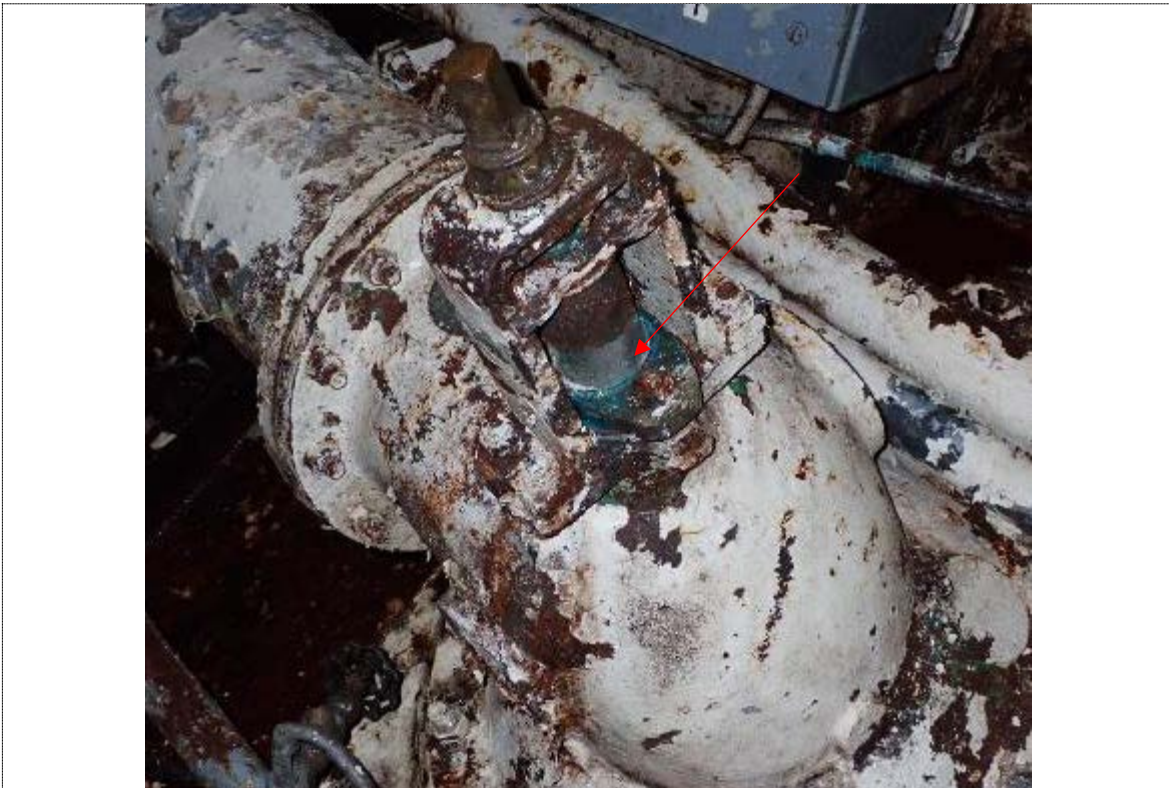
28. Stbd main sea valve in propulsion room in open position - port side same
