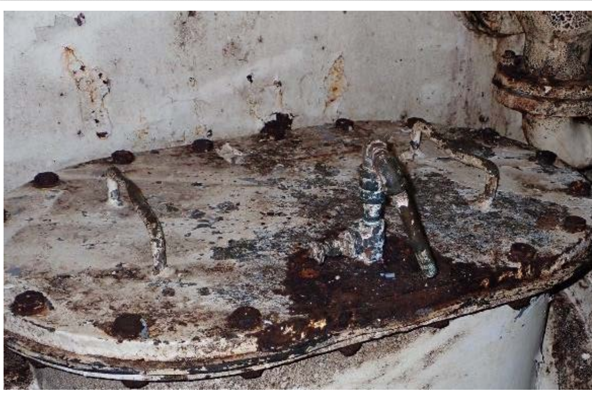
29. Sea strainer vent cock starting to corrode
