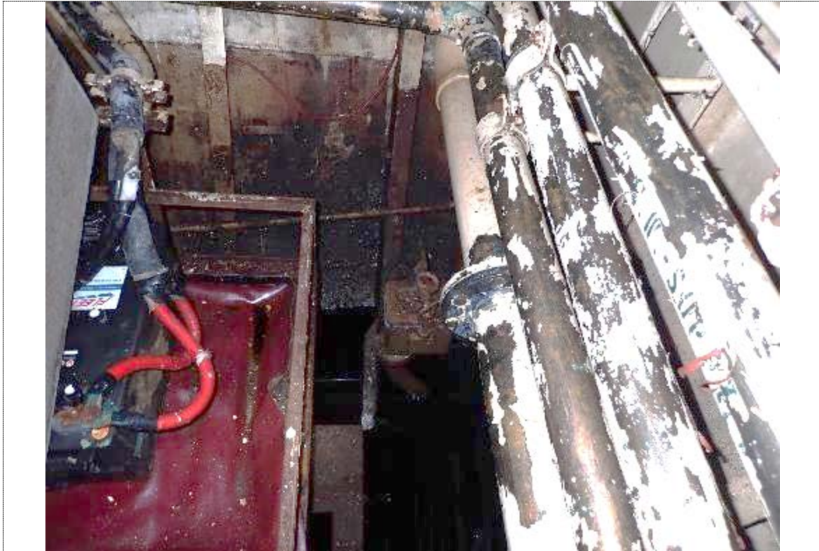
21. Diesel generator compartment bilge well – oil layer on top of water
