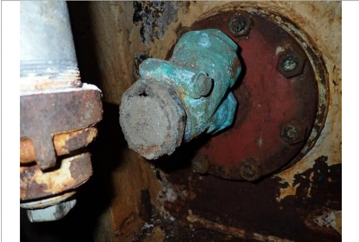
33. Overboard drain non-return fitted with cement plug
