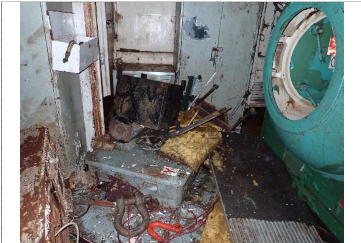
32. Decompression chamber compartment
