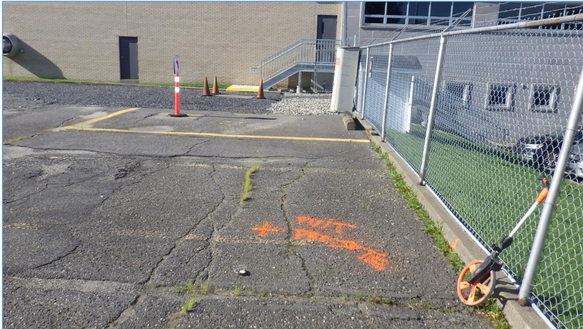
Photo 15: Localization of the new well projected at the Stanhope Border Crossing.
