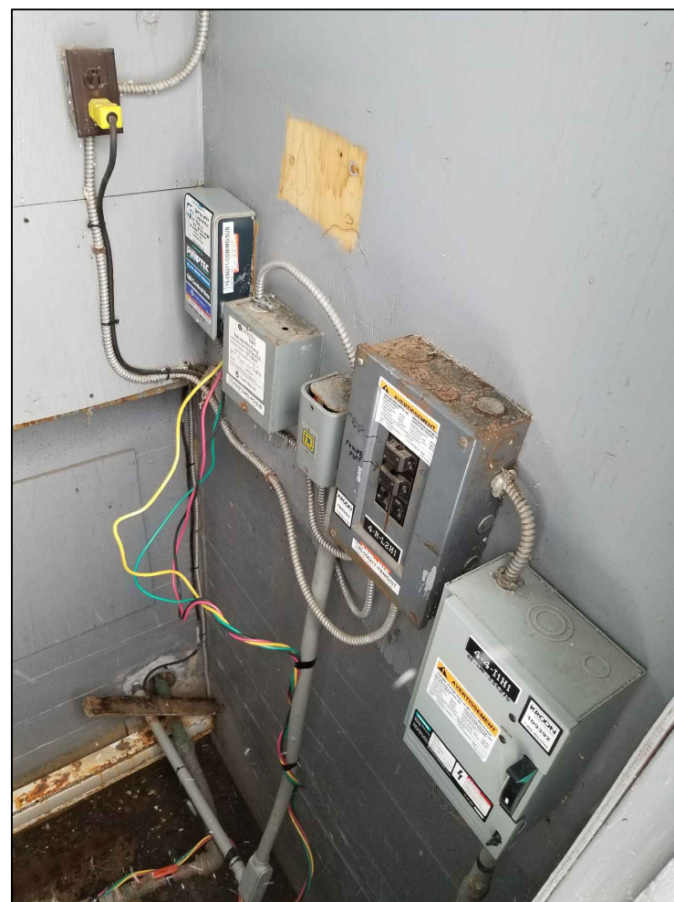
Electrical panels and components inside the shed
