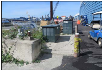
AUTHORIZED Sanitary Sewer Discharge point, Lift Station #11.
