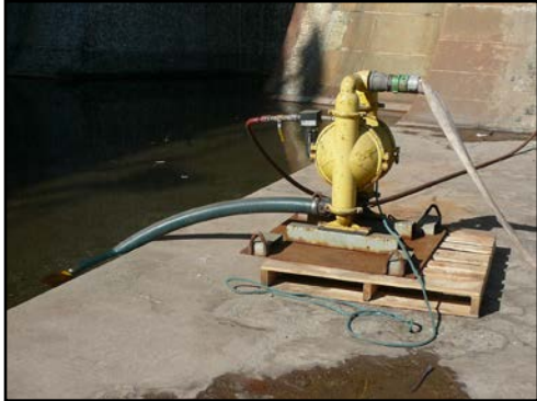
The sill diversion pump removes clean seawater from the pool at the front of Section 1 (moon pool) and discharges into the tunnel drains through a hard pipe on the graving dock wall.
