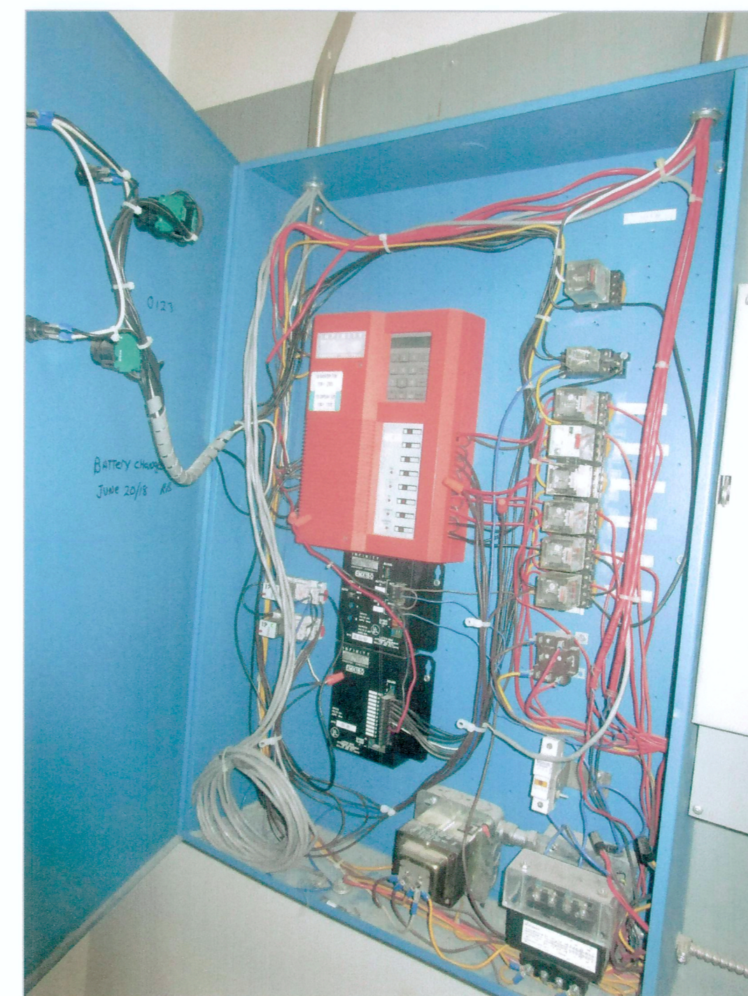
6 EXISTING CONTROL PANEL
