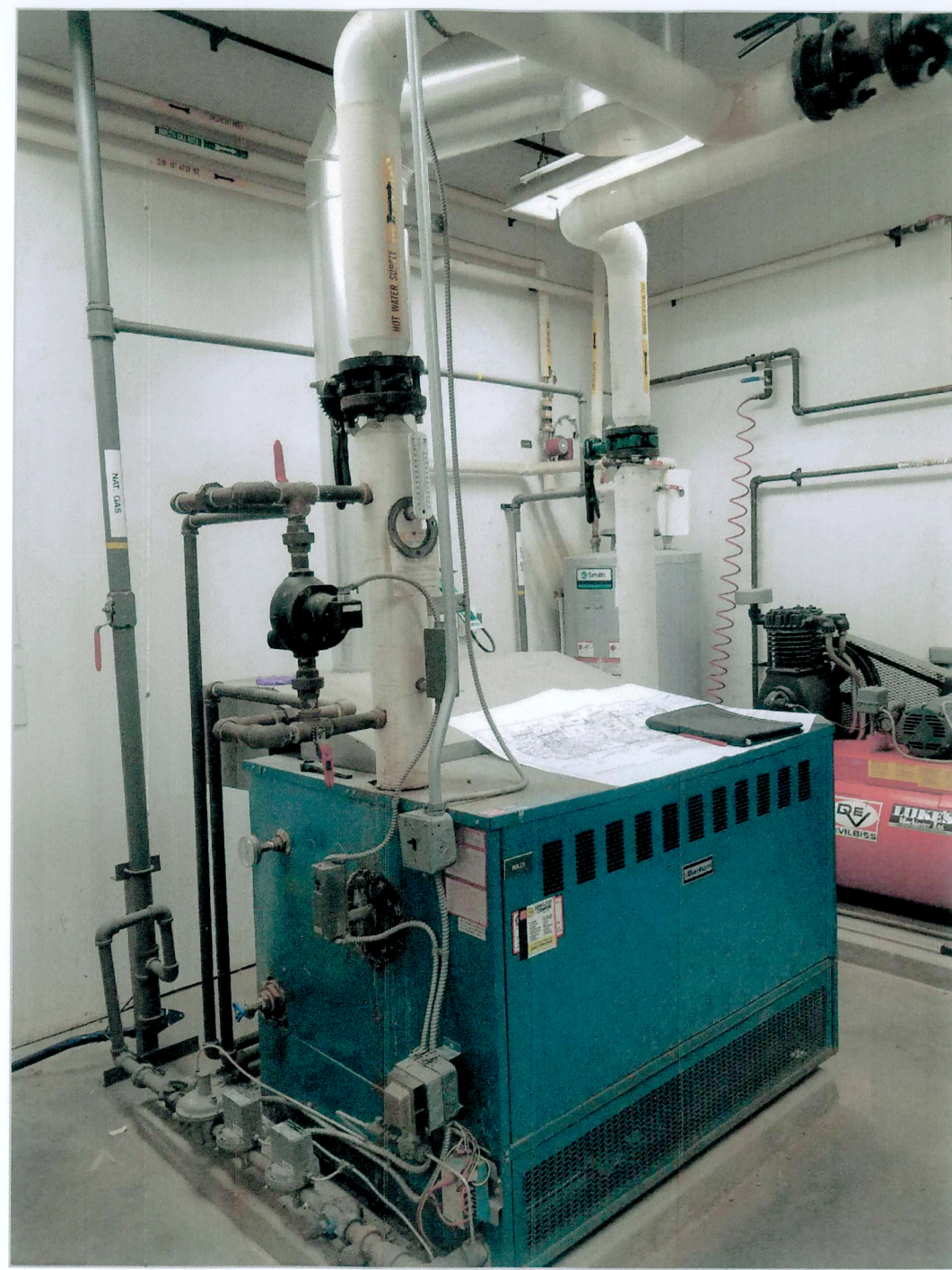
1 EXISTING BOILER (B-1)
