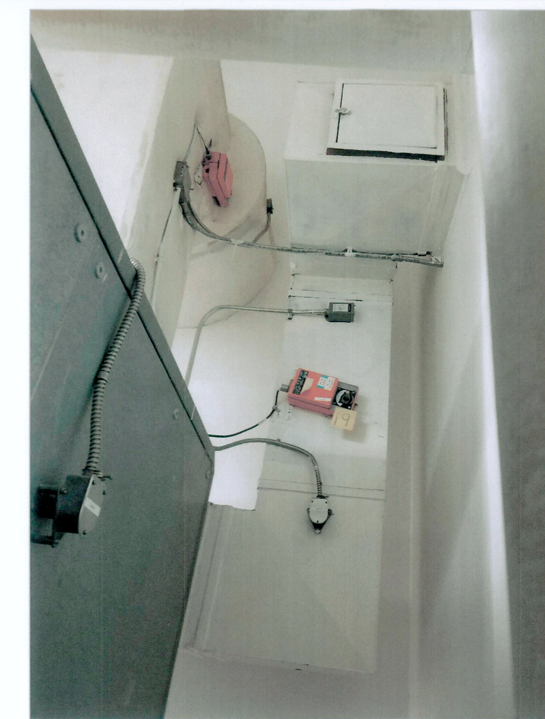
4 EXISTING AHU-1 O/A & R/A MOTORIZED DAMPERS
