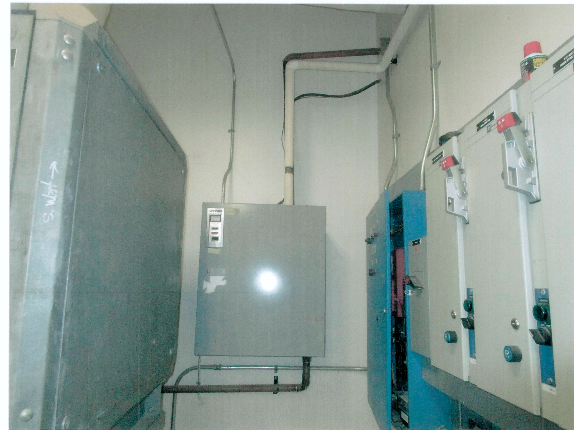
5 EXISTING HUMIDIFIER (HUM-1)
