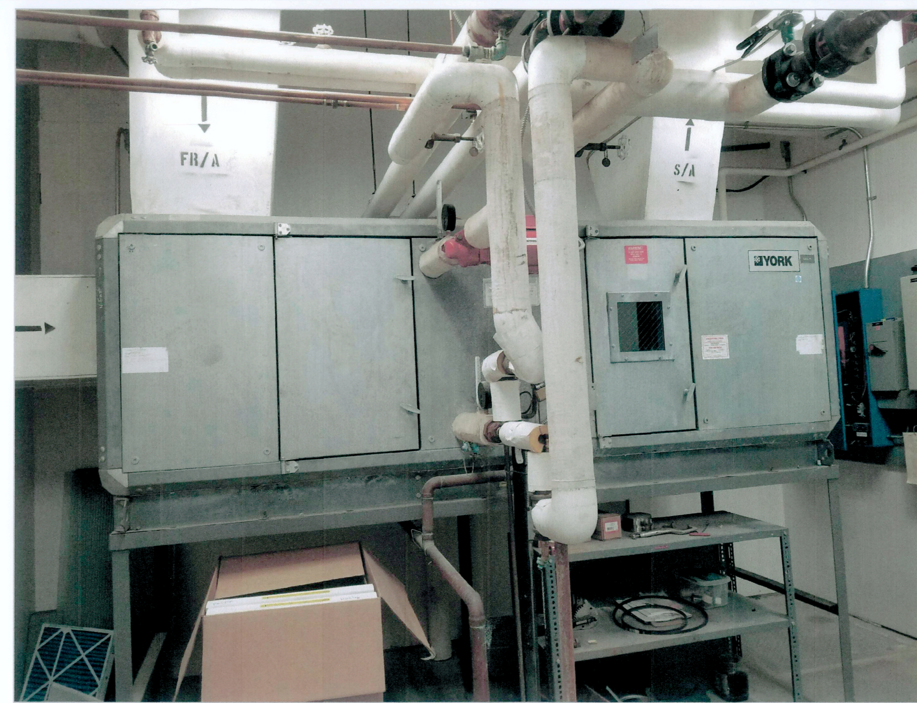
3 EXISTING AIR HANDLING UNIT (AHU-1)
