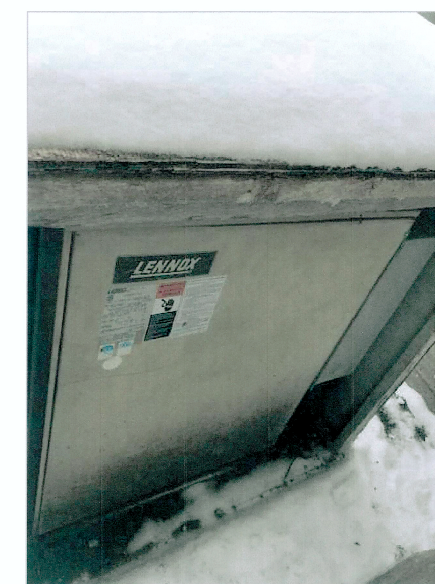
10 EXISTING OUTDOOR CONDENSING UNIT
