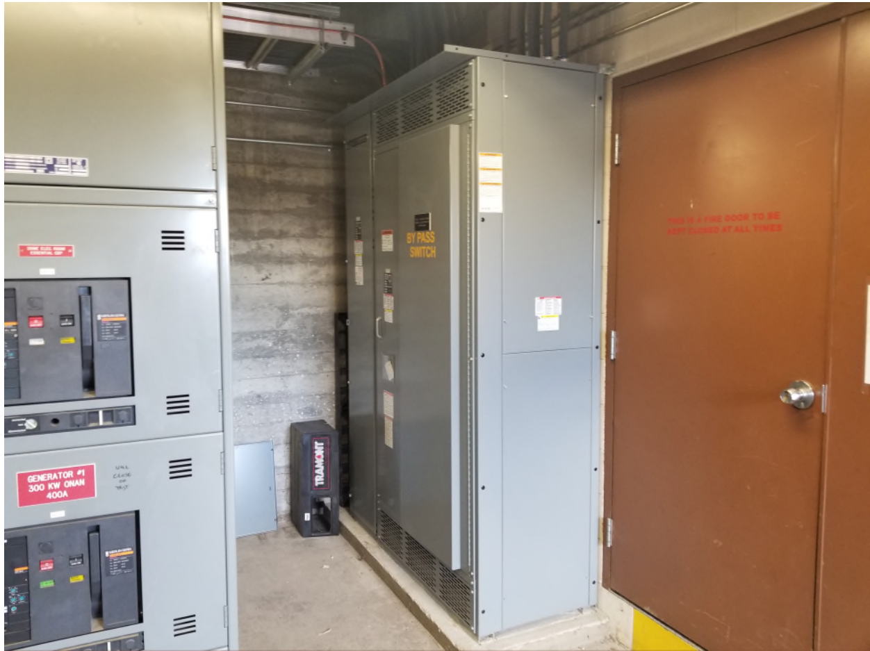
Picture 7 Showing Electrical Room, above Coal Vaults
