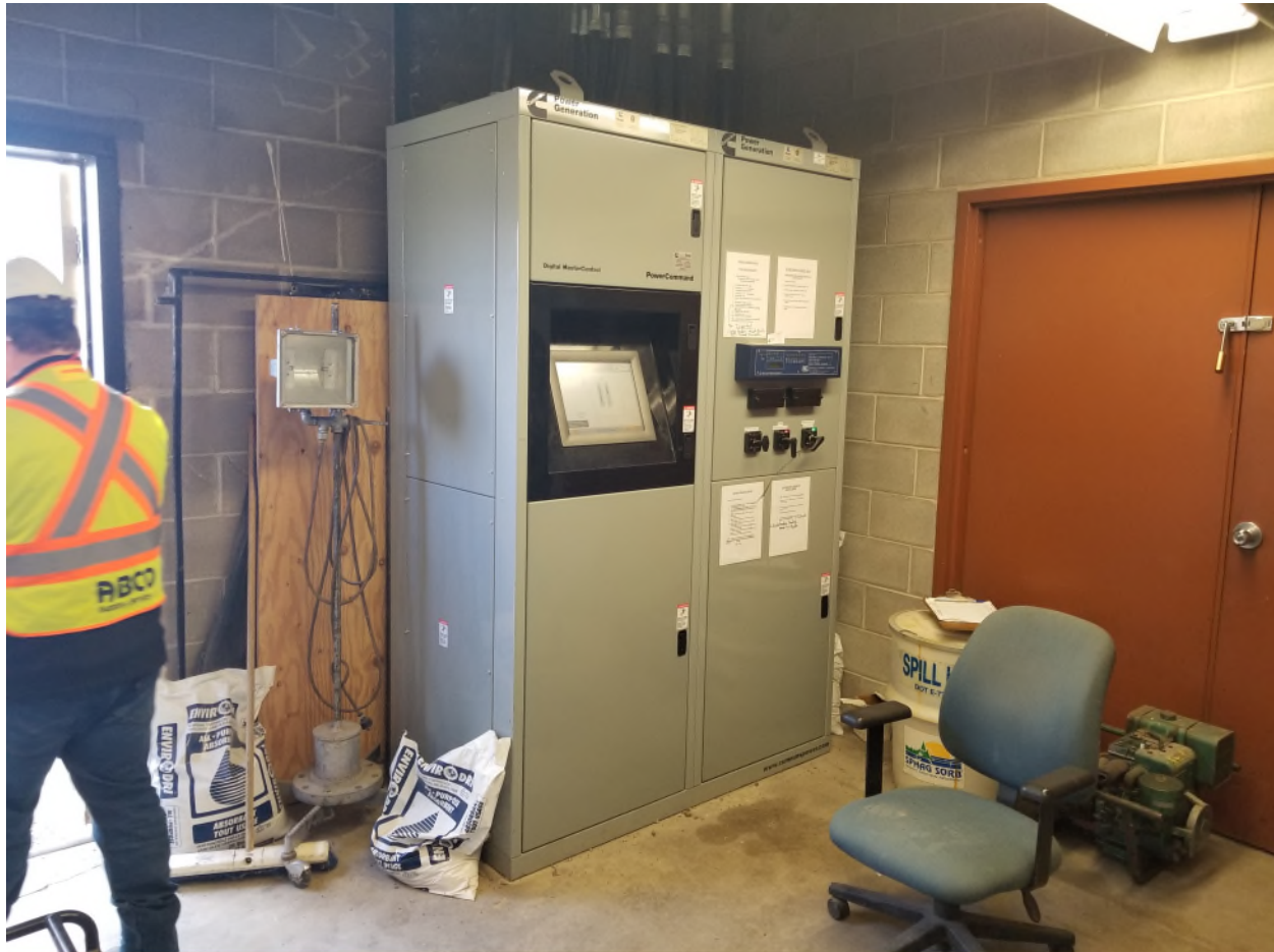
Picture 5 Showing Electrical Room, above Coal Vaults
