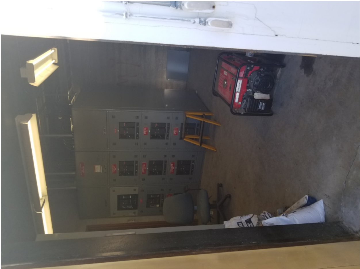
Picture 6 Showing Electrical Room, above Coal Vaults
