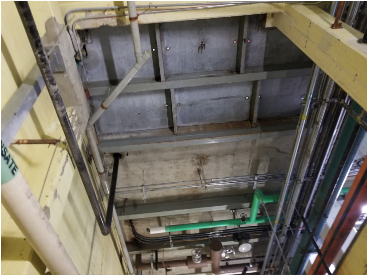
Picture 27 Showing main floor access panels, perspective looking up from sub basement
