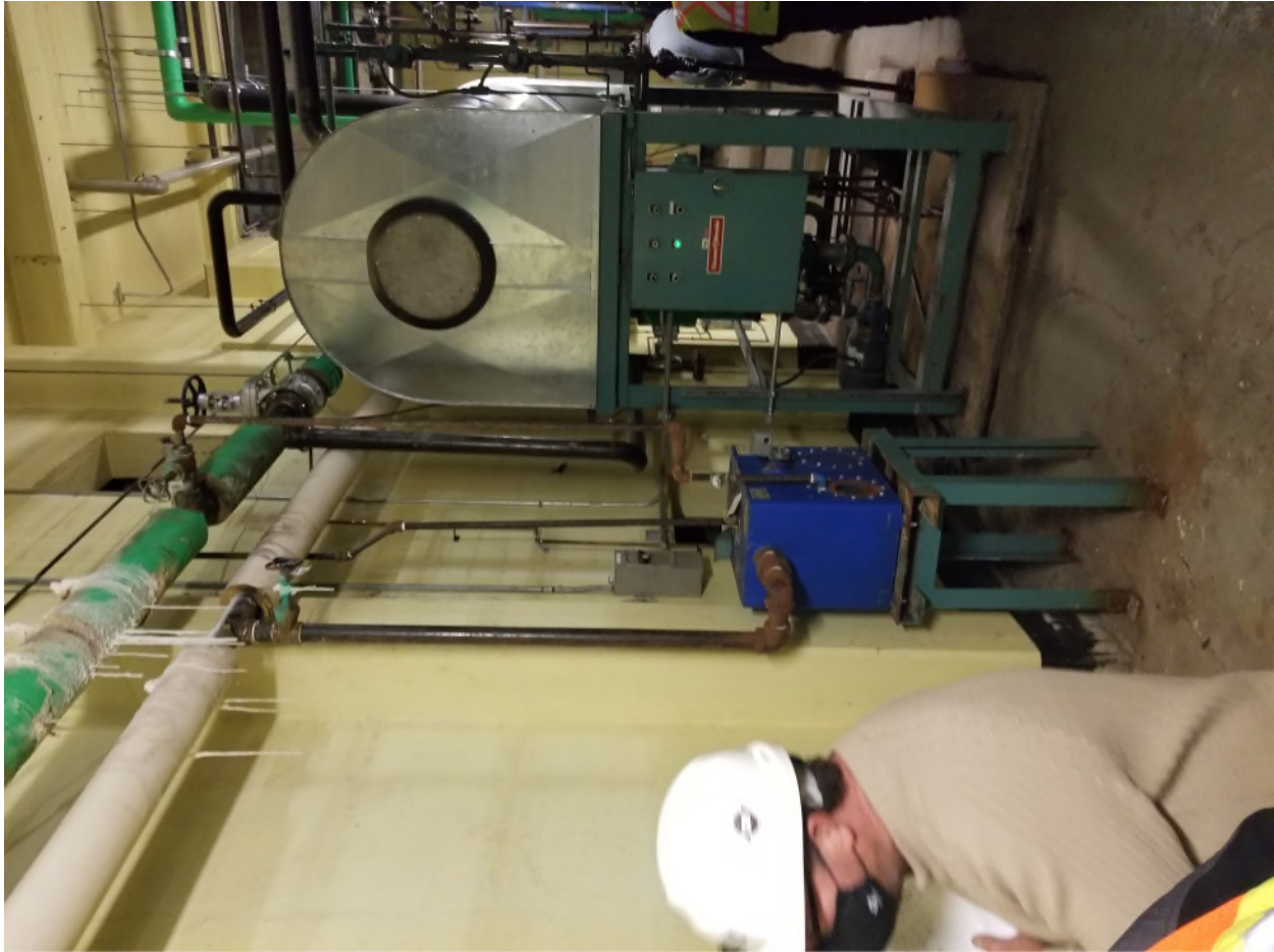
Picture 18 Showing sub basement walls and equipment
