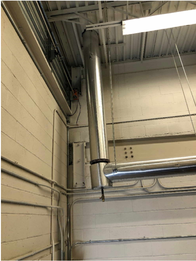
Photo #10– Existing surface conduit in plantroom
