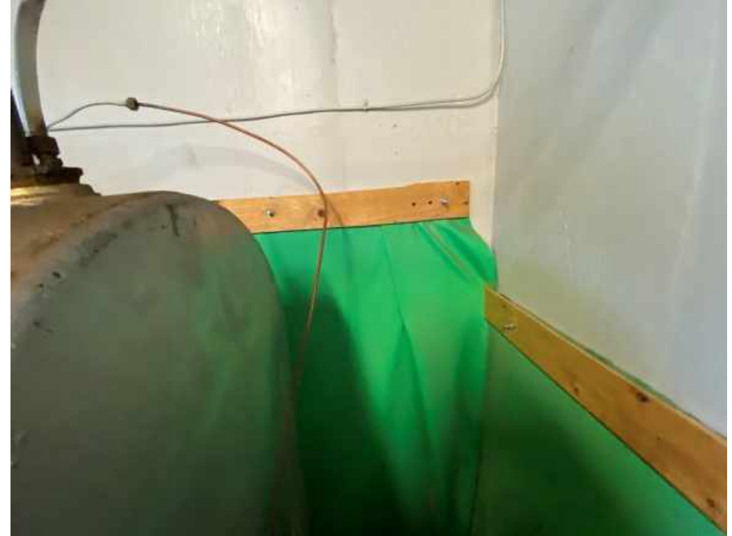
Photo #15 – Showing Spill Containment Seal
