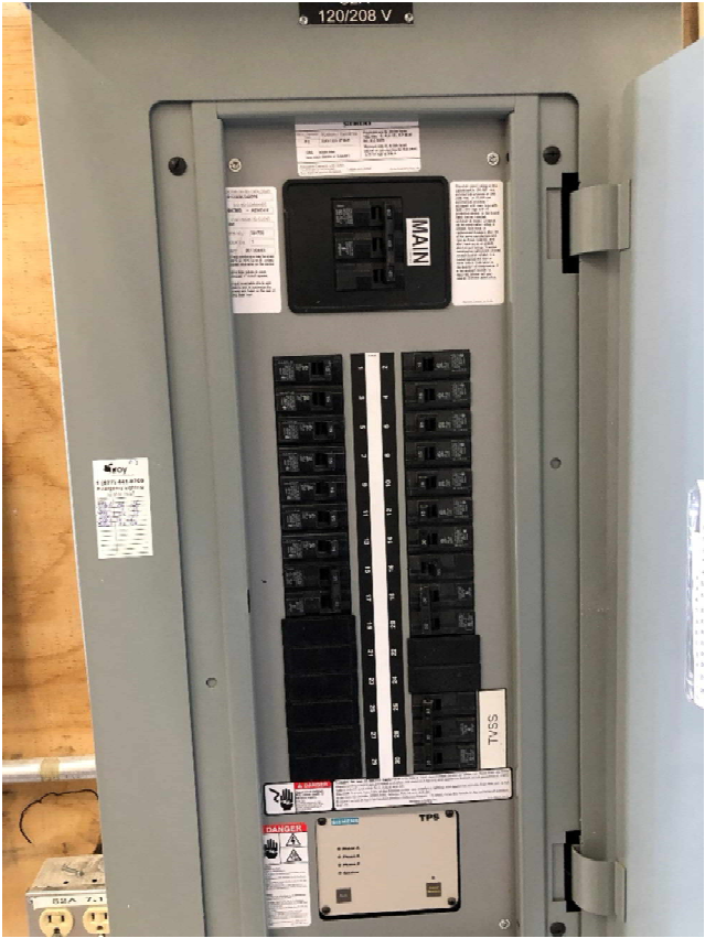
Photo #9 – Existing Electrical Panel in Plantroom
