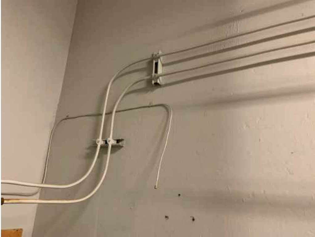
Photo #19 – Fuel oil lines to be re-run from new tank to generator
