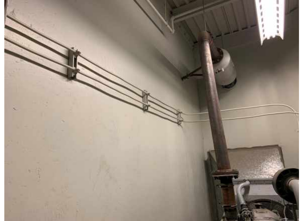
Photo #20 – Continuation of fuel lines
