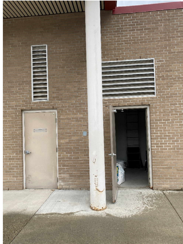
Photo #13 – Front Photo of the Generator and Electrical rooms
