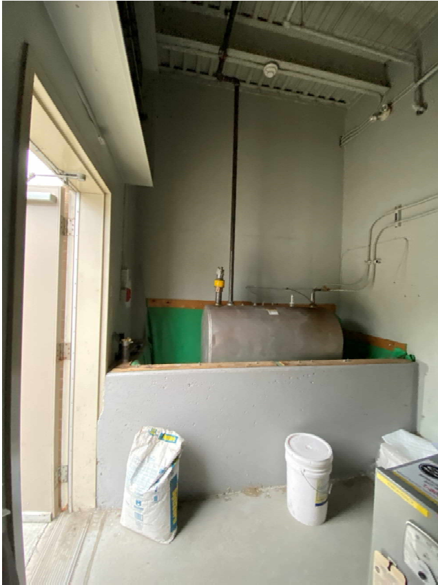
Photo #21 – Showing existing tank vent line
