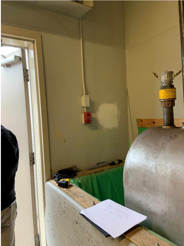
Photo #16 – Showing spill containment interface with wall and fill port wall opening
