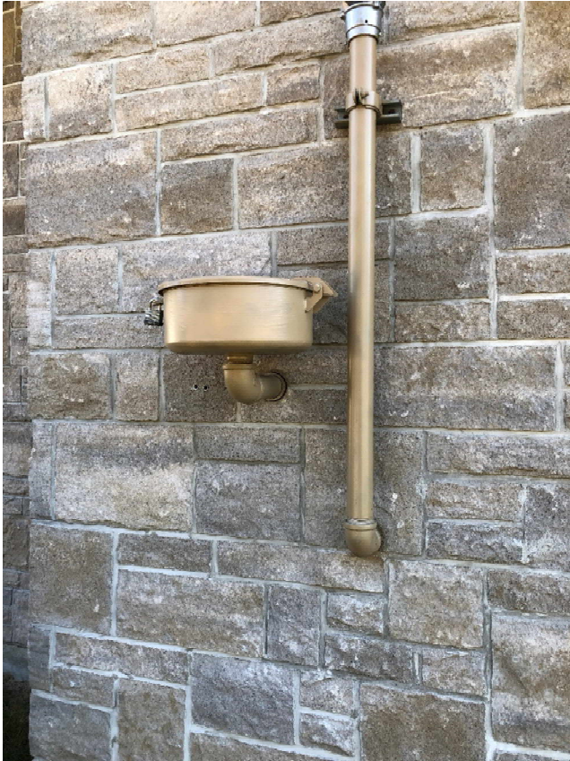
Photo #3 – Close up Photo of Fuel Fill Station
