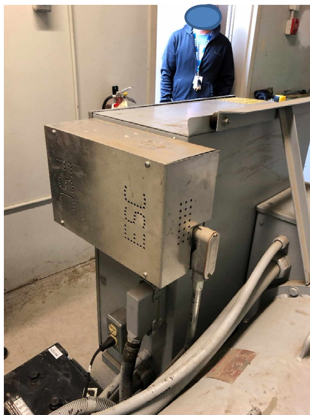
Photo #25 - ESC DDC Controller for fuel alarms
