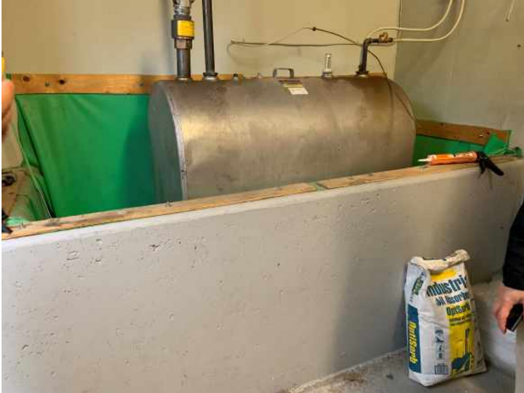
Photo #14 – Showing existing fuel tank and spill containment
