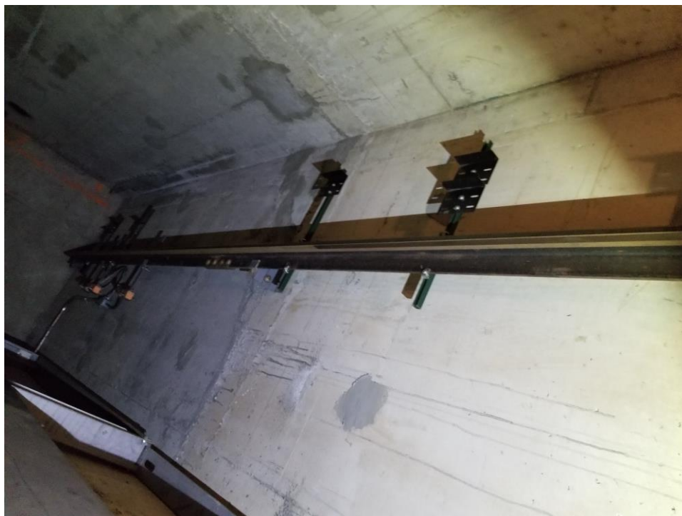
Photo 1: Cementitious patching patches in the elevator shaft do not contain asbestos .
