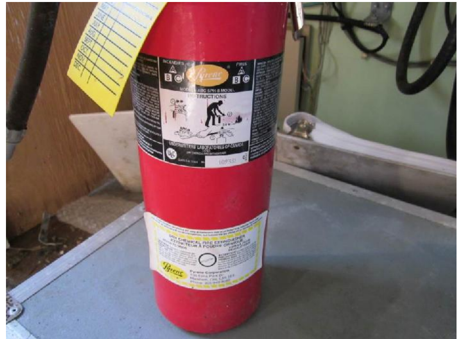
Photo 56: View of dry chemical fire extinguisher.
