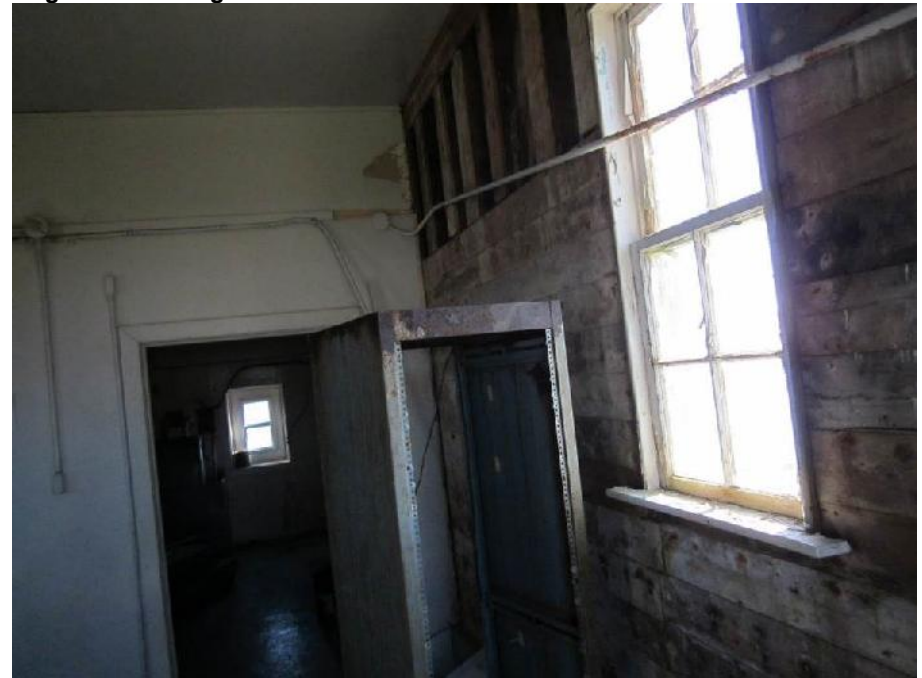
Photo 8: View of an exterior wall in the compressor room (Room 1) of the Former Fog Horn Building.
