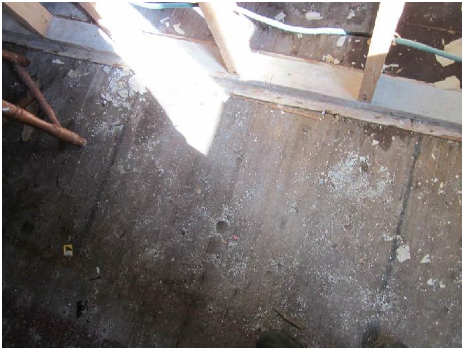
Photo 49: View of paint chips and debris on the floor in Room 3.
