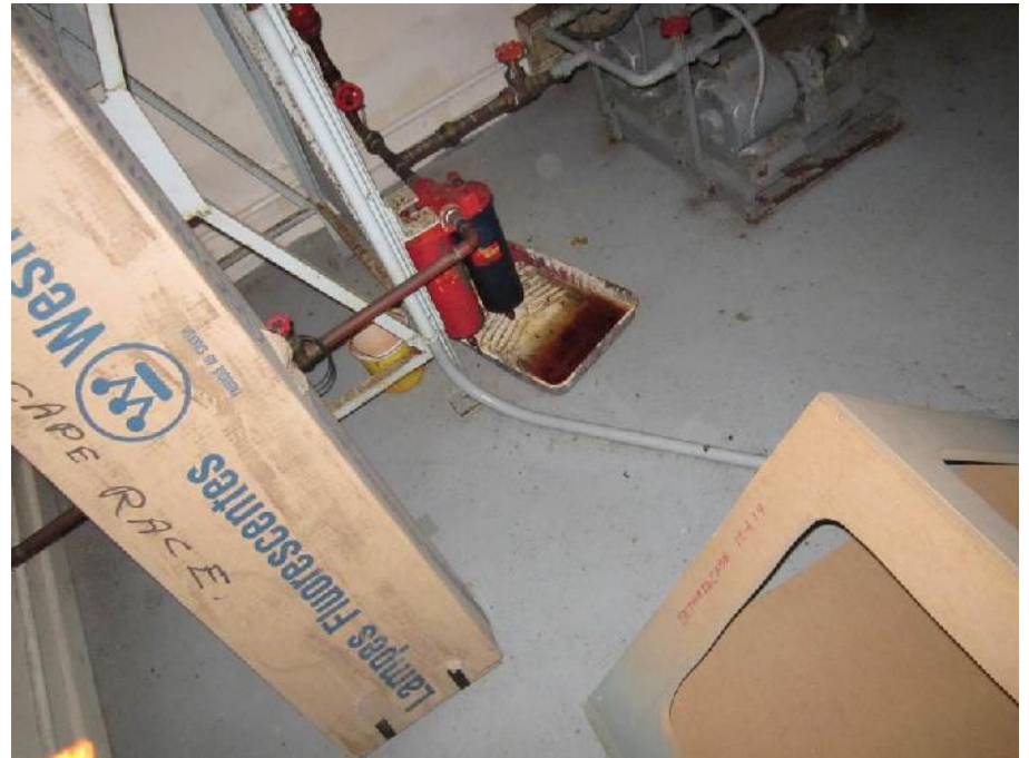
Photo 34: View of paint tray used to collect oil from fuel lines near the aboveground fuel storage tank on a metal frame in Room 2.
