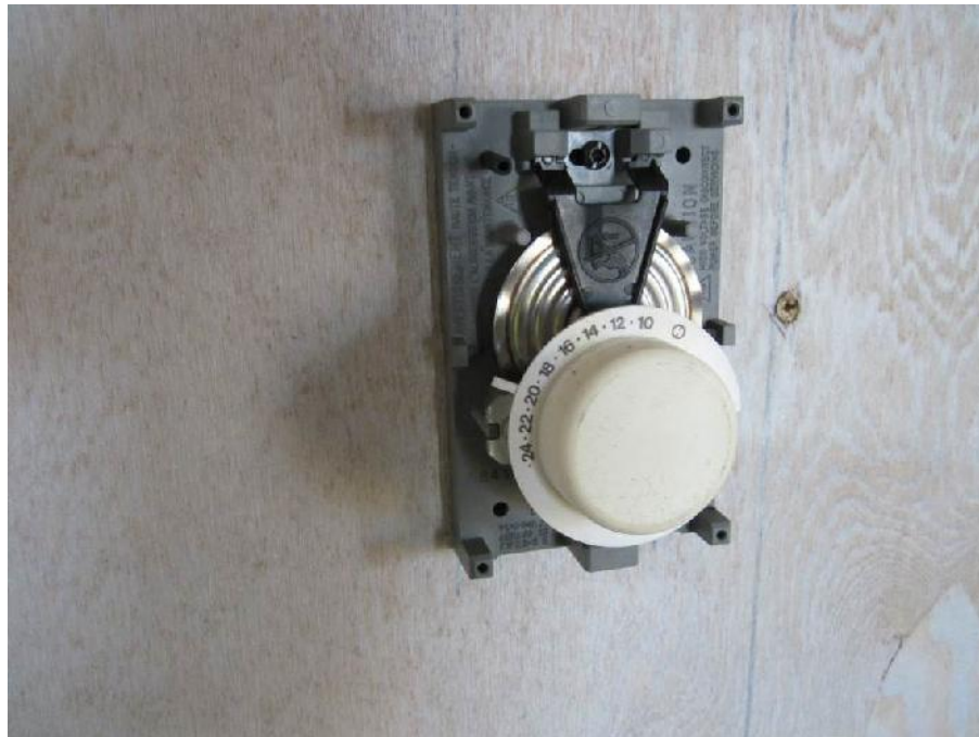
Photo 27: View of white Honeywell thermostat (casing removed).
