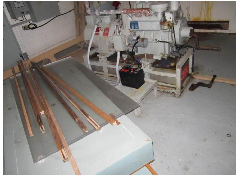
Photo 10: View of the generator in the generator room (Room 2) of the Former Fog Horn Building. Note: Potential lead-acid battery.
