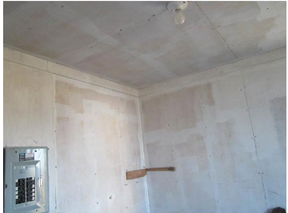
Photo 10: View of Room 2 in the Former Generator Building. Note: Electrical panel on wall.
