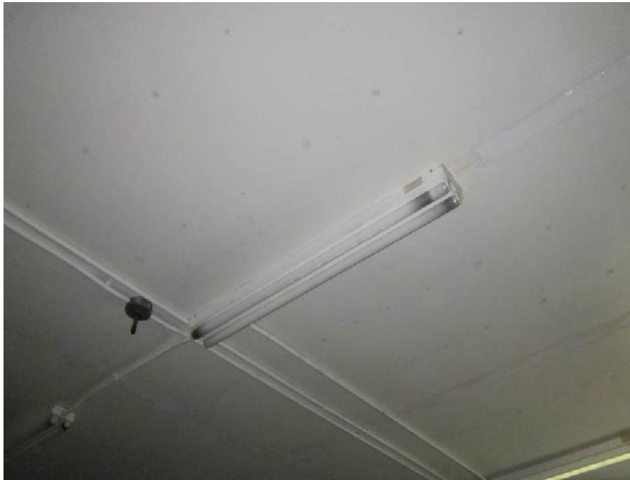
Photo 13: View of fluorescent lighting in the generator room (Room 2) of the Former Fog Horn Building.
