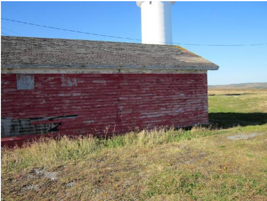
Photo 3: View of the southeast side of the Former Generator Building. Note: Missing roofing materials.
