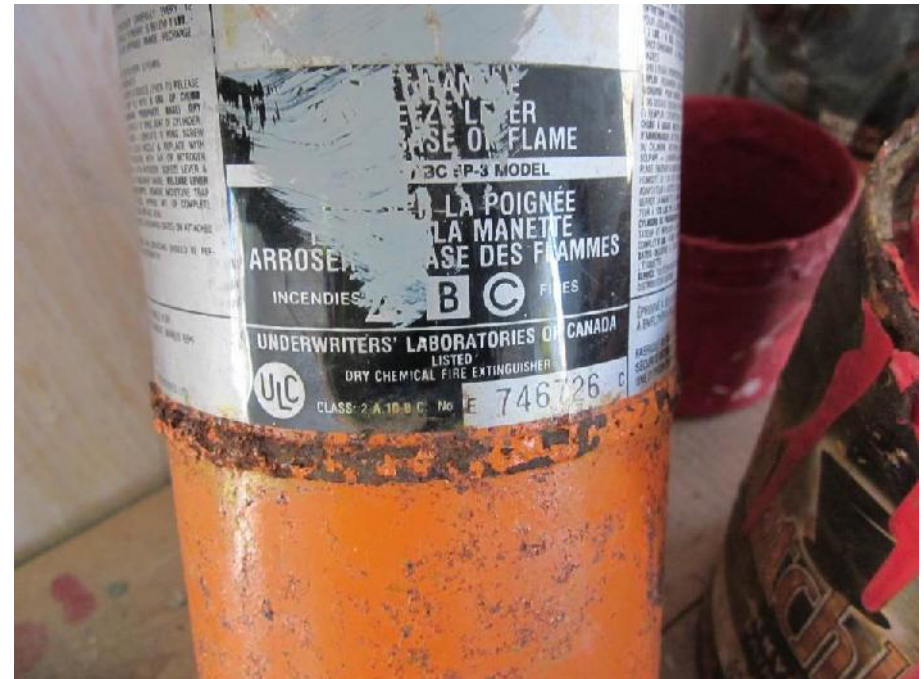
Photo 28: View of dry chemical fire extinguisher.
