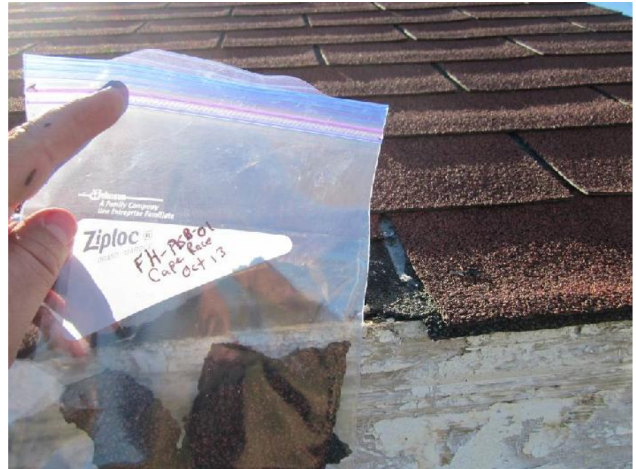
Photo 14: View of location of red shingle and black shingle sample FH-ASB-01 (roof).
