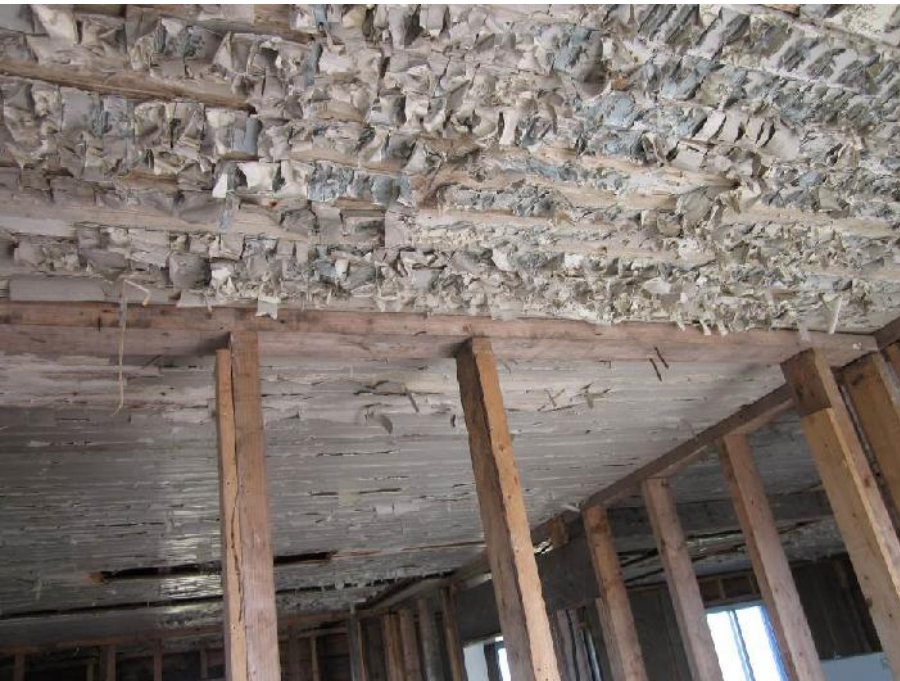
Photo 7: View of the ceiling in the porch (Room 1) of the Former Dwelling.
