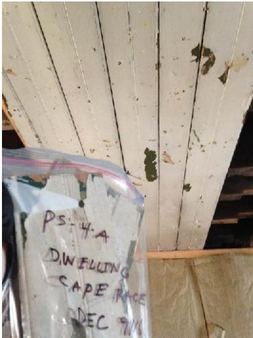
Photo 45: View of location of paint sample PS-4-A (including wood substrate) in Room 7 (ceiling).
