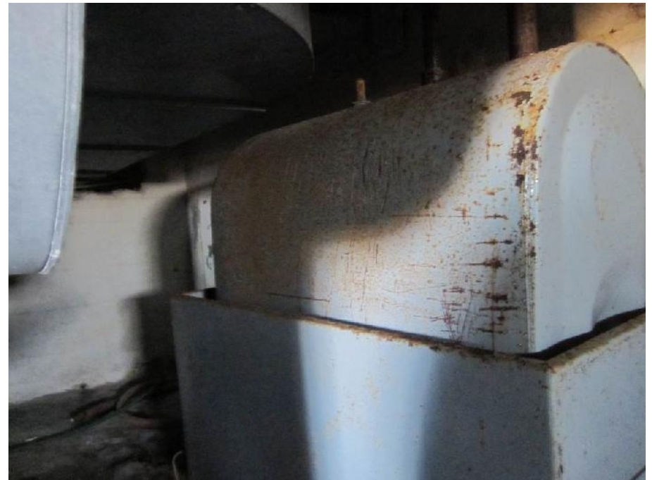
Photo 60: View of heating oil aboveground storage tank in the basement (Room 11).
