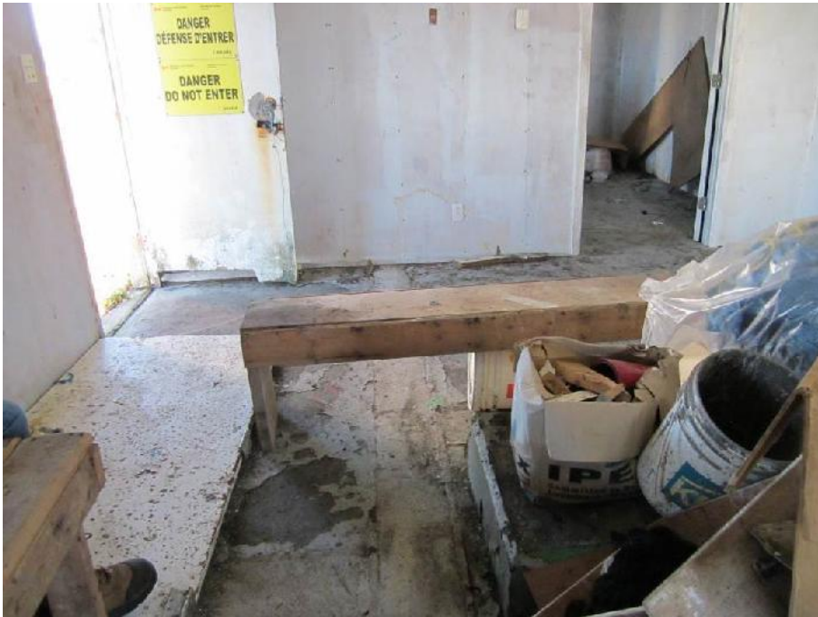
Photo 9: View of Room 1 in the Former Generator Building. Note: SVG on the surface of the painted metal door on the floor (possible fire-rated door).
