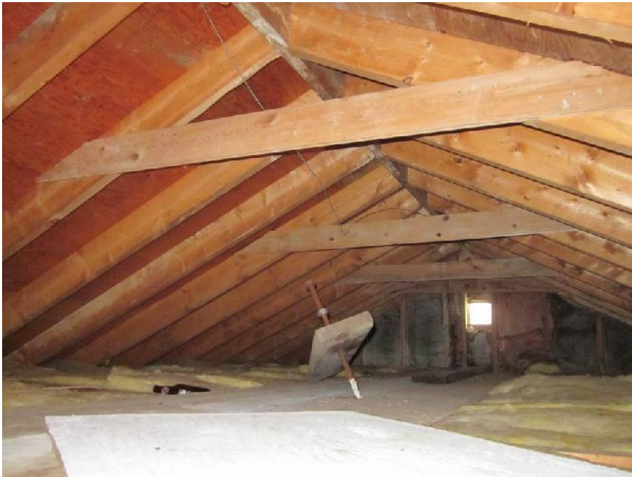
Photo 5: View of the attic in the Former Generator Building. Note: Pink fiberglass insulation on exterior wall in background (not sampled).
