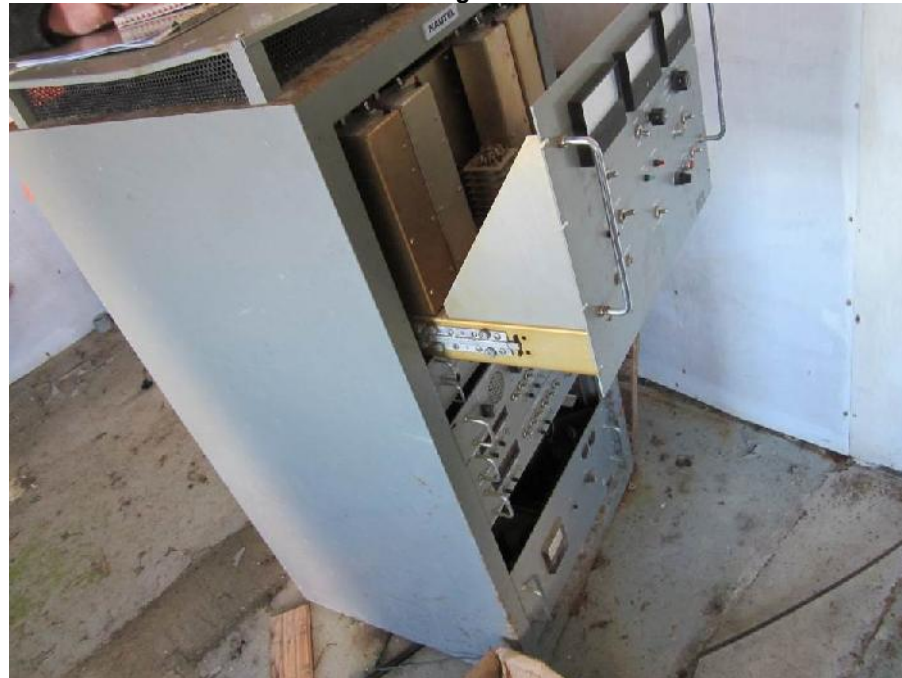
Photo 15: View of unknown equipment (possibly electrical equipment) in Room 2 of the Former Generator Building.
