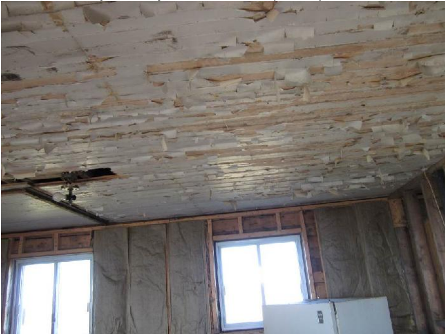
Photo 11: View of the ceiling in the dining room (Room 3) of the Former Dwelling.
