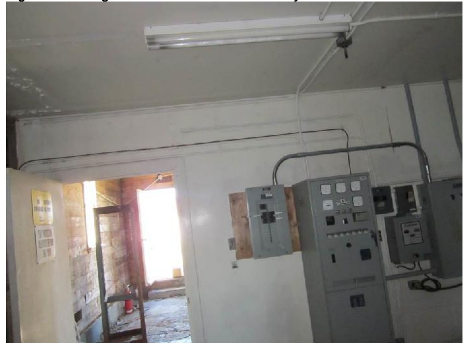
Photo 12: View of electrical boxes and panels in the generator room (Room 2) of the Former Fog Horn Building. Note: fire extinguisher in background.
