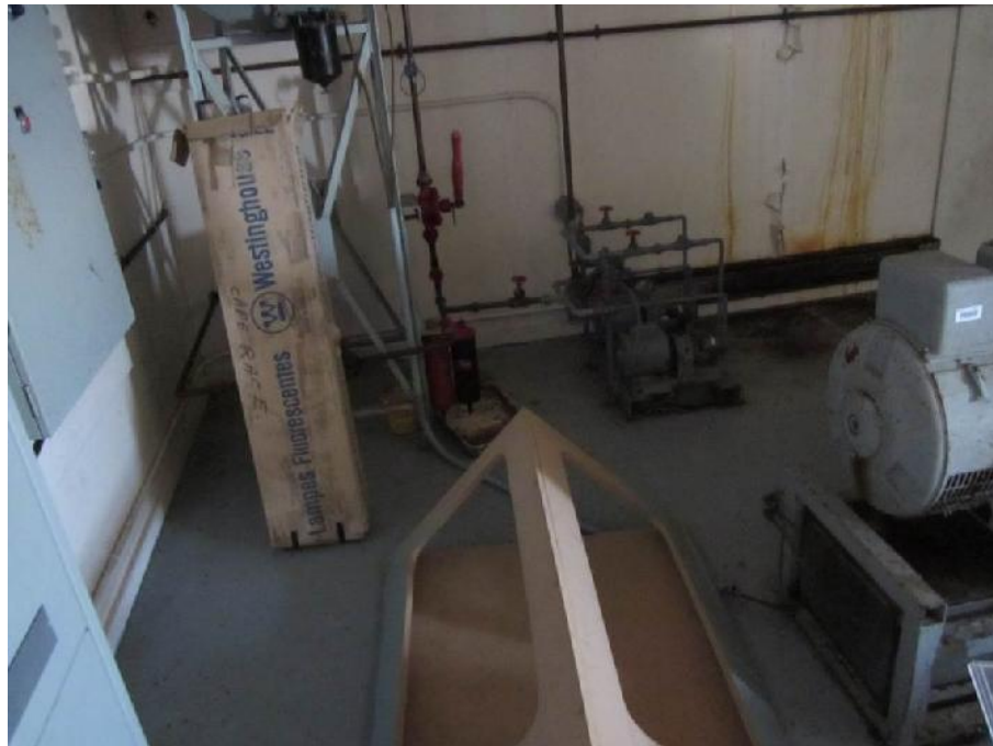
Photo 31: View of box of fluorescent light tubes in Room 2.
