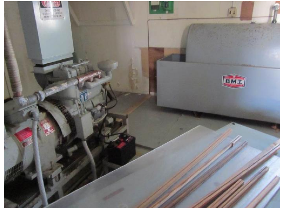
Photo 32: View of the generator and aboveground fuel storage tank in Room 2.
