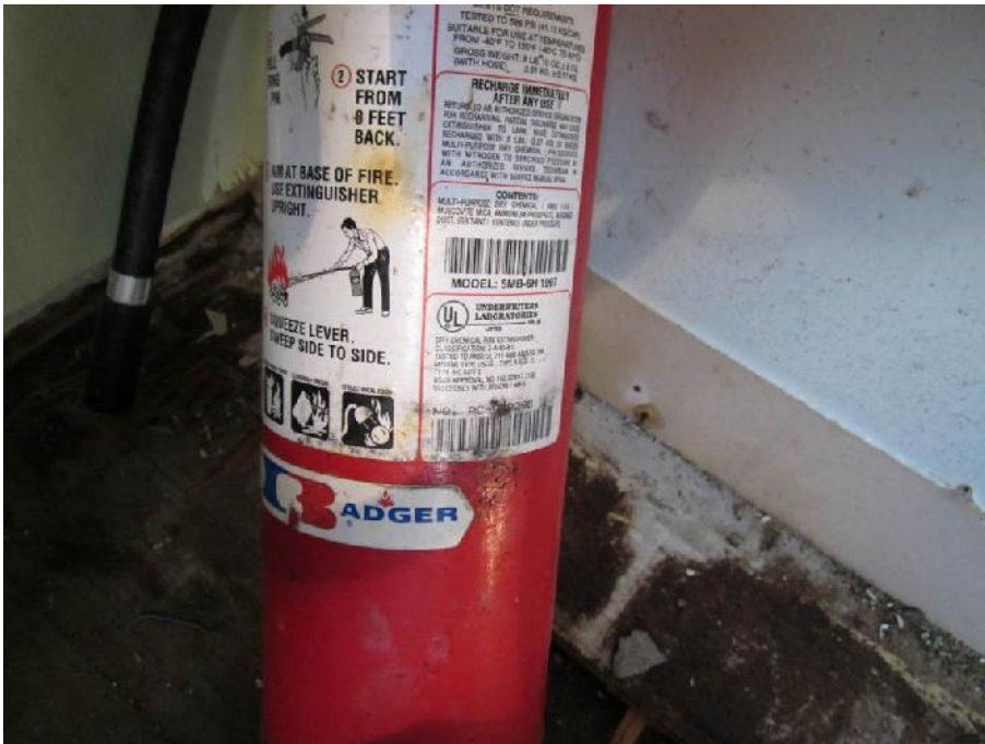
Photo 55: View of dry chemical fire extinguisher.
