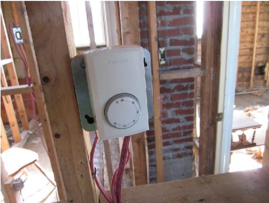
Photo 53: View of white Dimplex thermostat.
