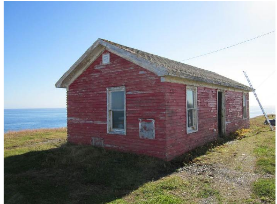
Photo 4: View of the northwest and northeast sides of the Former Generator Building.
