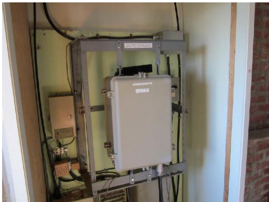
Photo 13: View of radio control equipment in the control room (Room 5) of the Former Dwelling.
