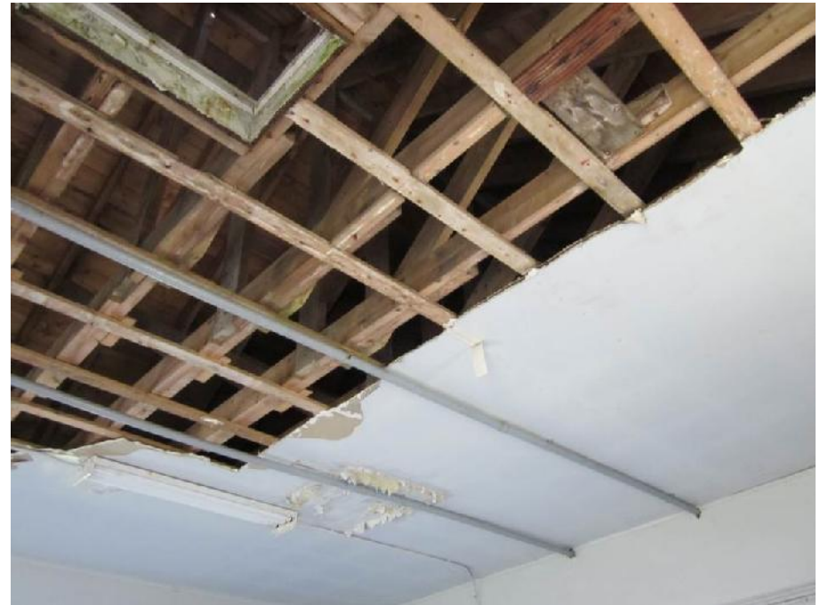
Photo 6: View of the ceiling in the compressor room (Room 1) of the Former Fog Horn Building.
