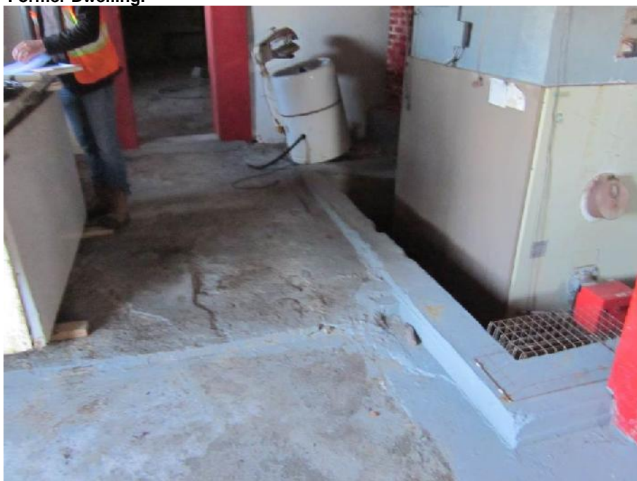
Photo 15: View of the oil fired warm air furnace (right) and freezer (left) in the basement (Room 11) of the Former Dwelling.
