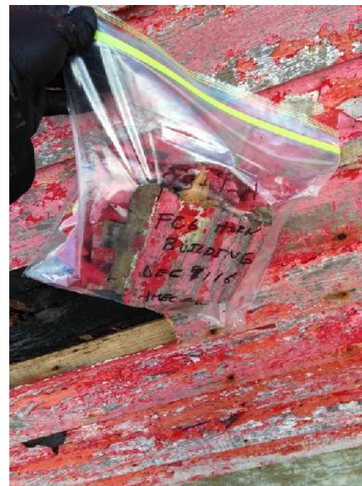
Photo 28: View of location of paint sample PS-1-A (exterior wall). Note: Sample mislabeled PS-1-A in the field; it should have been labeled PS-2-A.
