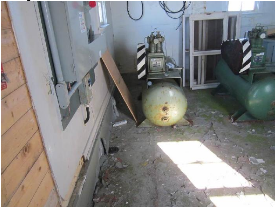
Photo 7: View of the air compressors in the compressor room (Room 1) of the Former Fog Horn Building.
