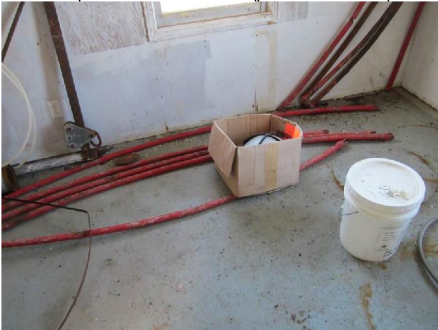
Photo 11: View of piping on the floor of Room 2 in the Former Generator Building.
