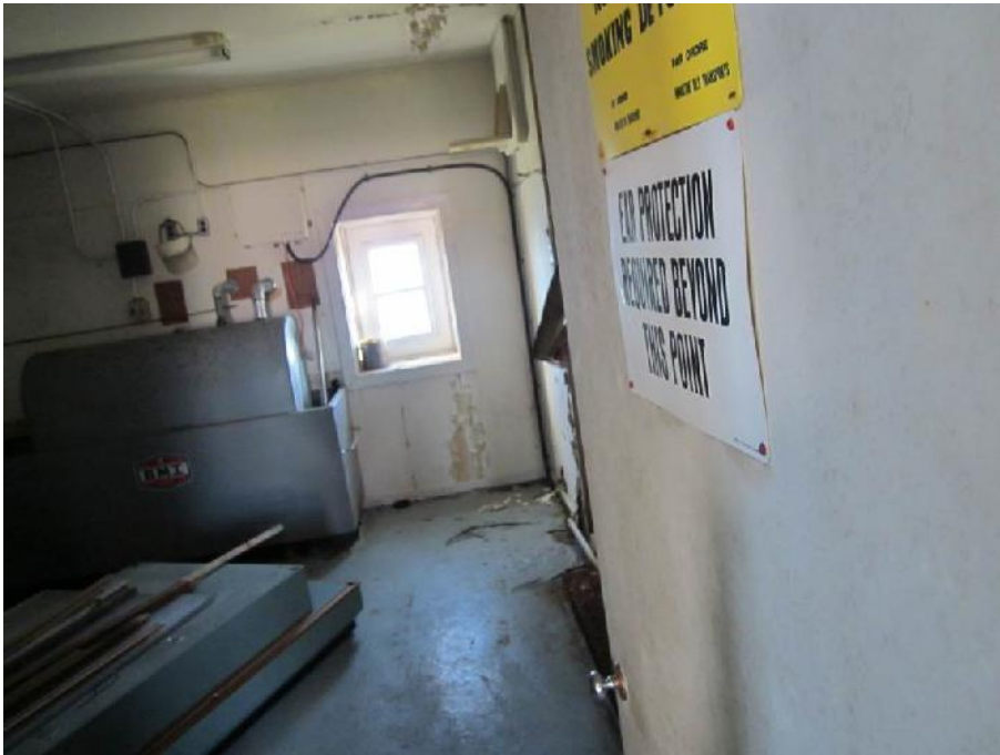
Photo 9: View of the aboveground fuel storage tank in the Generator Room (Room 2) of the Former Fog Horn Building.
