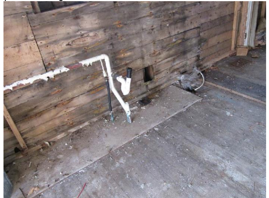
Photo 8: View of exposed piping in the kitchen (Room 2) of the Former Dwelling. Note dark-stained wood on exterior wall.
