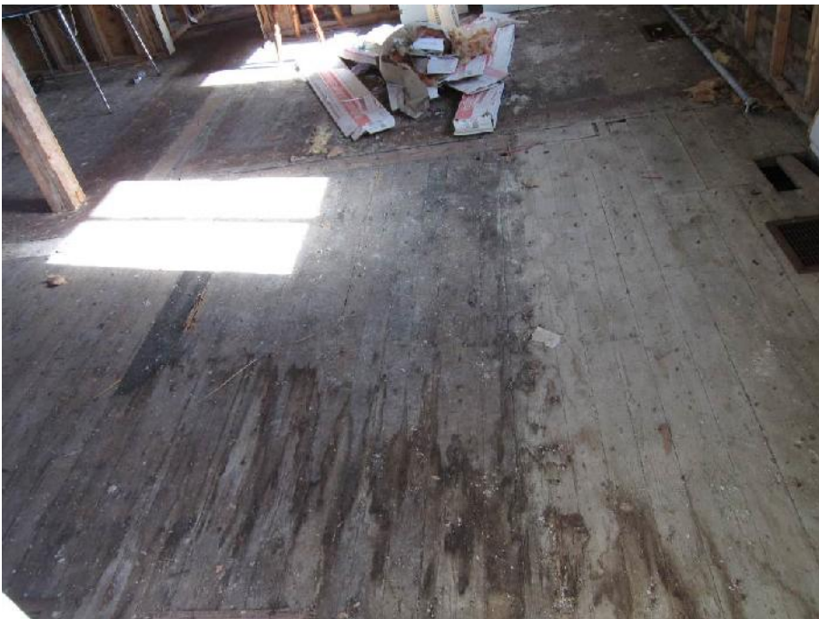
Photo 51: View of dark-coloured water staining on the surface of the wood floor in Room 3.
