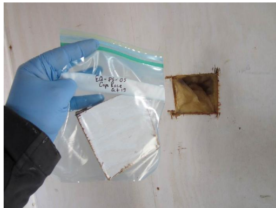
Photo 22: View of location of paint sample EQ-PS-5 (exterior wall). Note: Fibreglass insulation.
