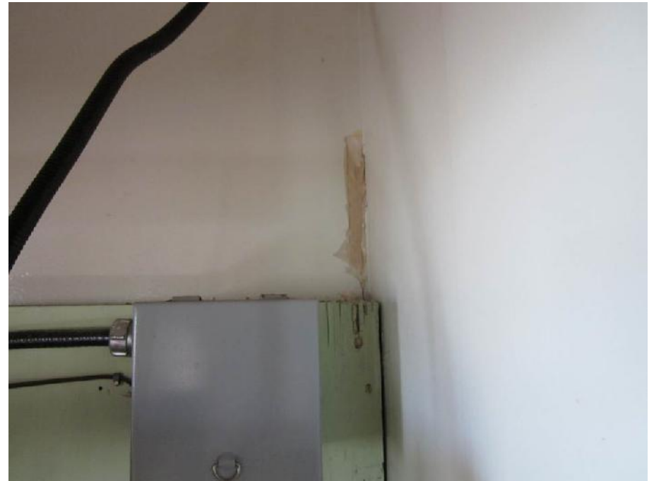
Photo 30: View of location of gypsum and drywall joint compound sample ASB-11 (Room 5).
