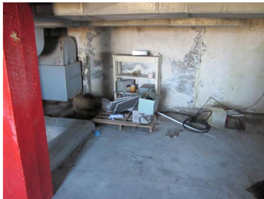
Photo 14: View of the heating oil aboveground storage tank (left) in the basement (Room 11) of the Former Dwelling.
