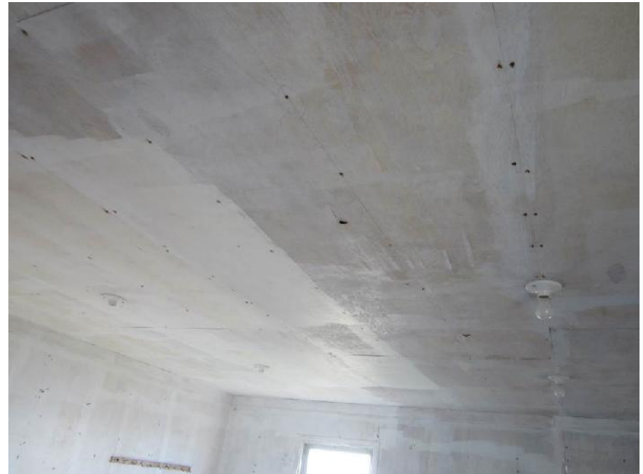
Photo 6: View of the ceiling and lighting (incandescent) in the Former Generator Building.
