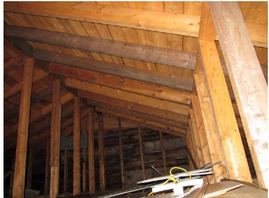
Photo 4: View of the attic in the Former Dwelling. Note dark-stained wood on exterior wall.
