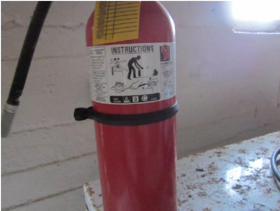
Photo 57: View of dry chemical fire extinguisher.
