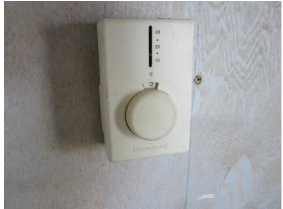
Photo 26: View of white Honeywell thermostat.
