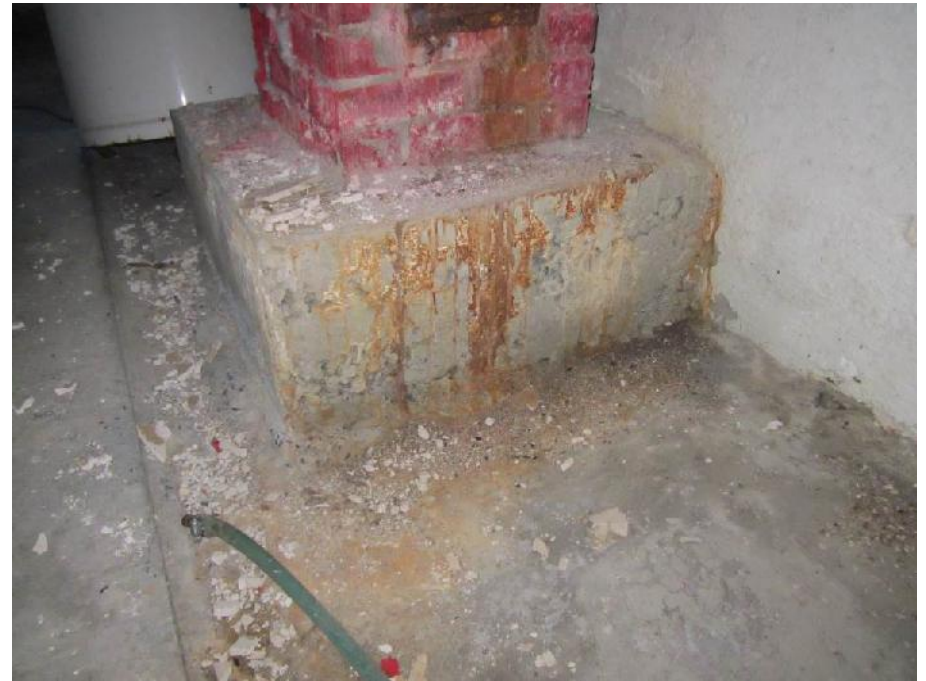
Photo 50: View of paint chips and debris on floor in Room 11 near the base of the brick chimney.
