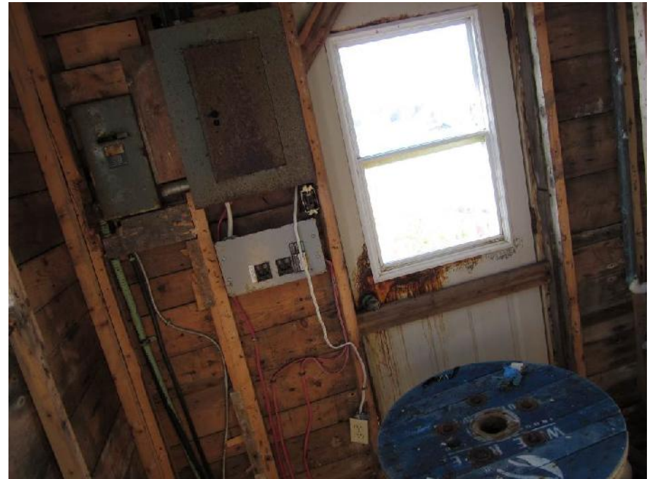
Photo 6: View of the porch (Room 1) in the Former Dwelling. Note electrical panels and wiring.
