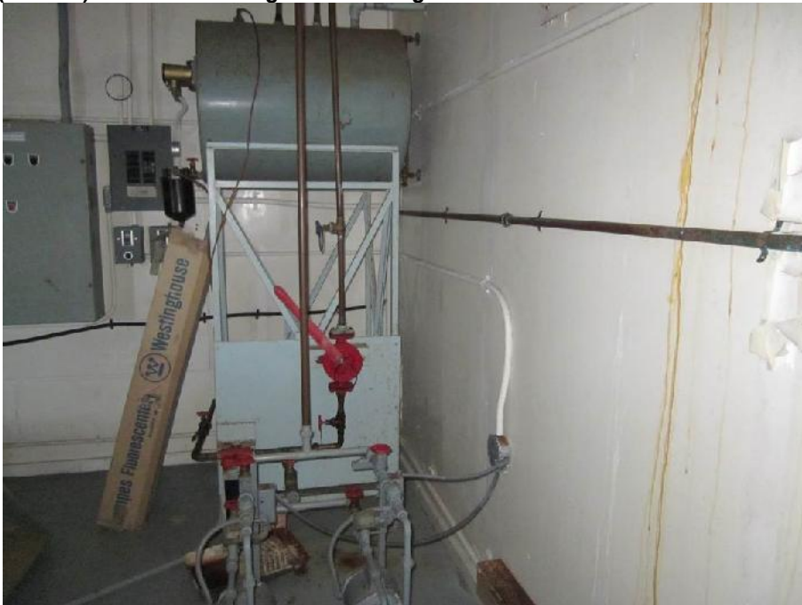
Photo 11: View of the raised fuel storage tank in the generator room (Room 2) of the Former Fog Horn Building. Note: Piping on wall.
