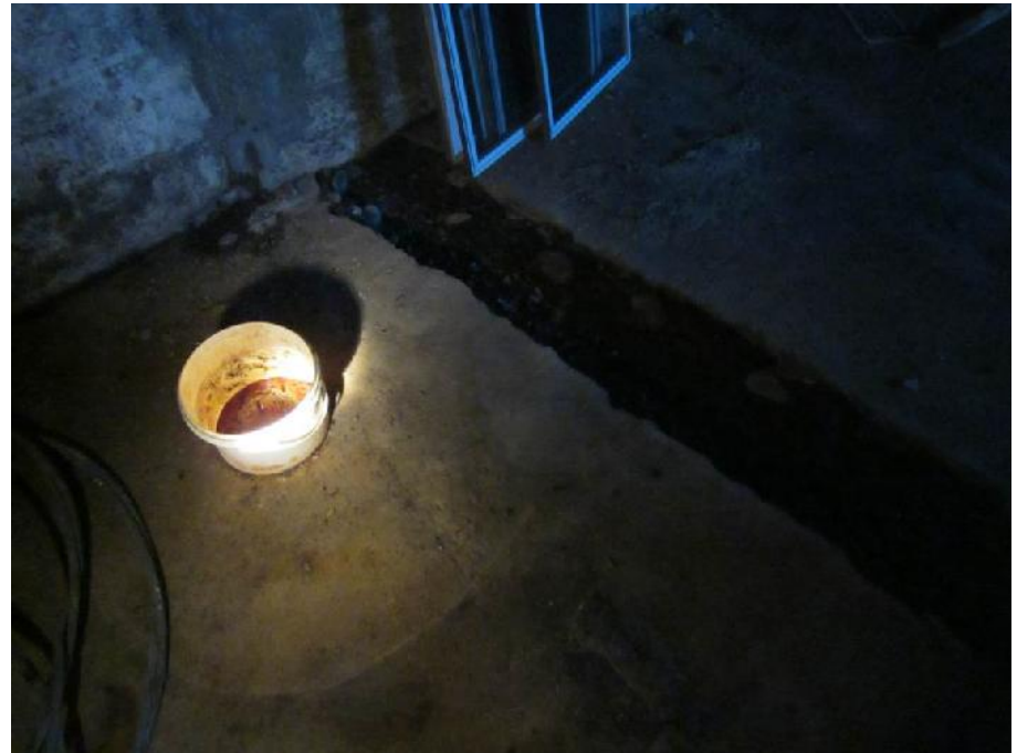
Photo 18: View of the trench in the basement (Room 12) of the Former Dwelling. Note suspected heating oil in pail.
