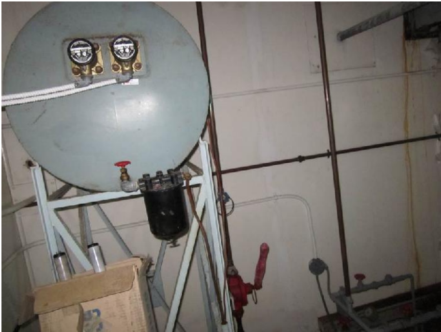
Photo 33: View of aboveground fuel storage tank on a metal frame in Room 2.
