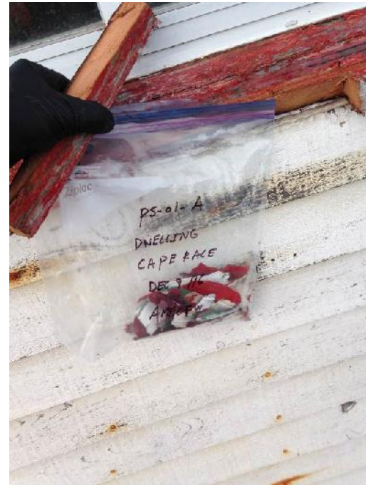
Photo 42: View of location of paint sample PS-1-A (including wood substrate) (exterior wall).
