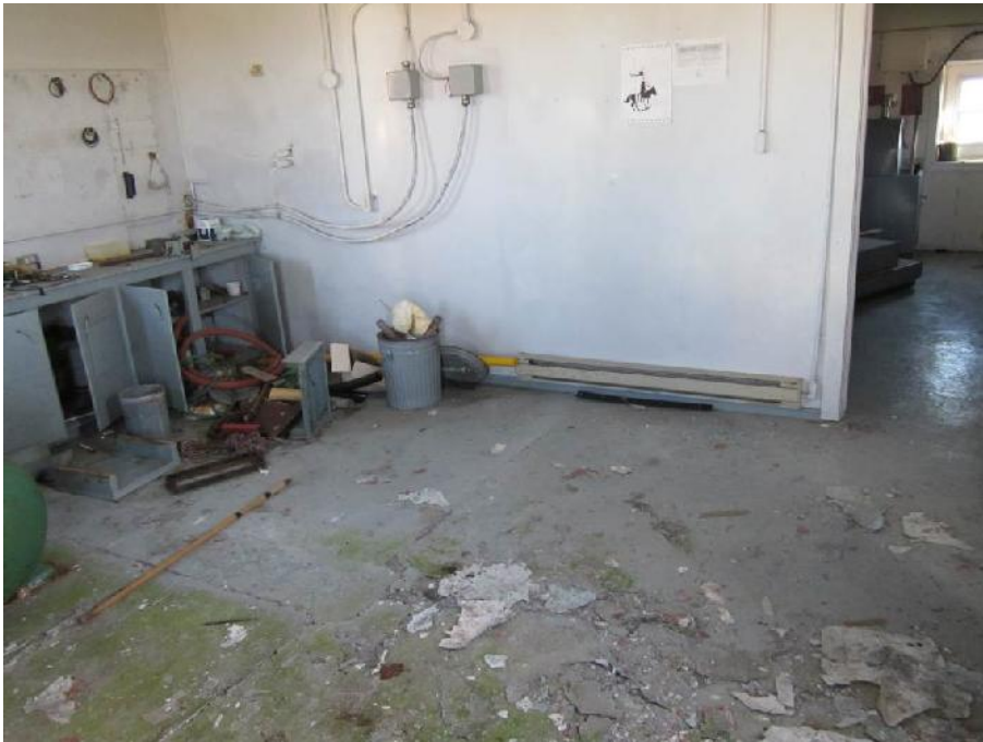
Photo 5: View of the compressor room (Room 1) of the Former Fog Horn Building.
