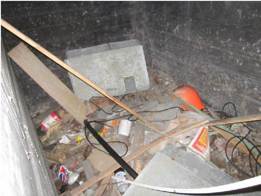
Photo 19: View inside the water cistern in the basement (Room 12) of the Former Dwelling.
