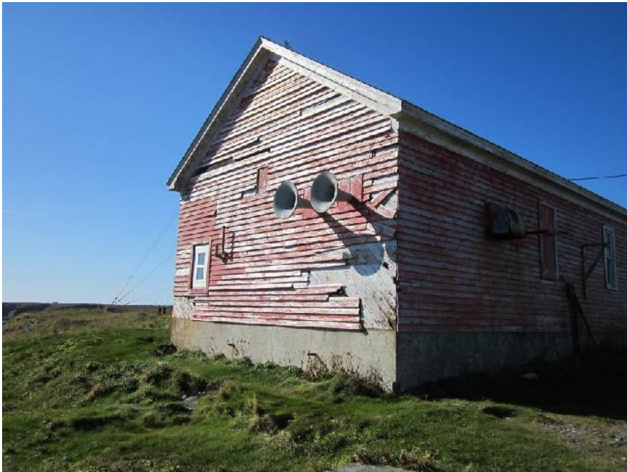
Photo 3: View of the southeast and northeast sides of the Former Fog Horn Building.
