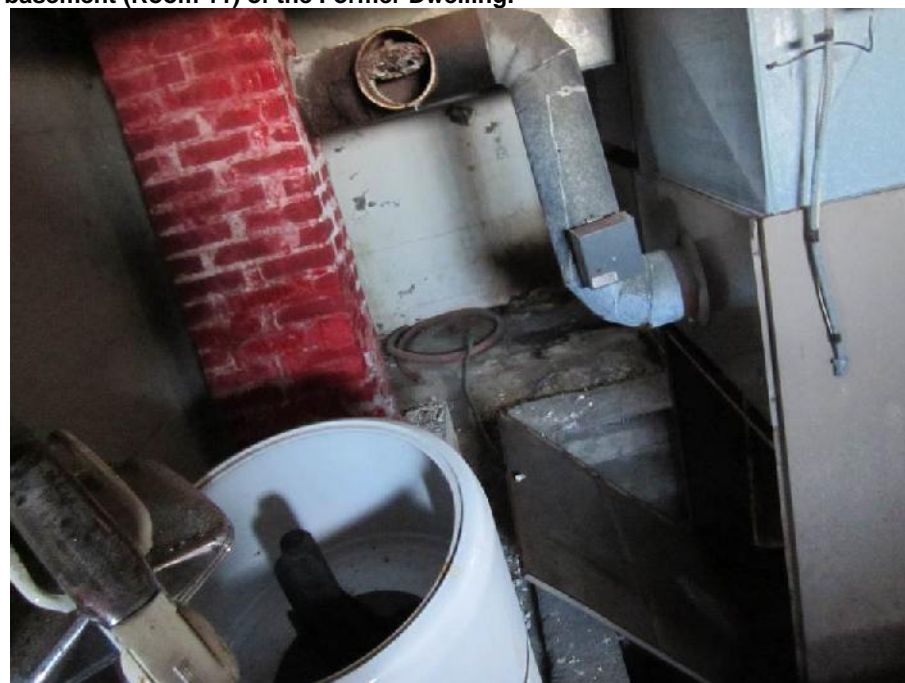
Photo 16: View of the brick chimney and furnace in the basement (Room 11) of the Former Dwelling.
