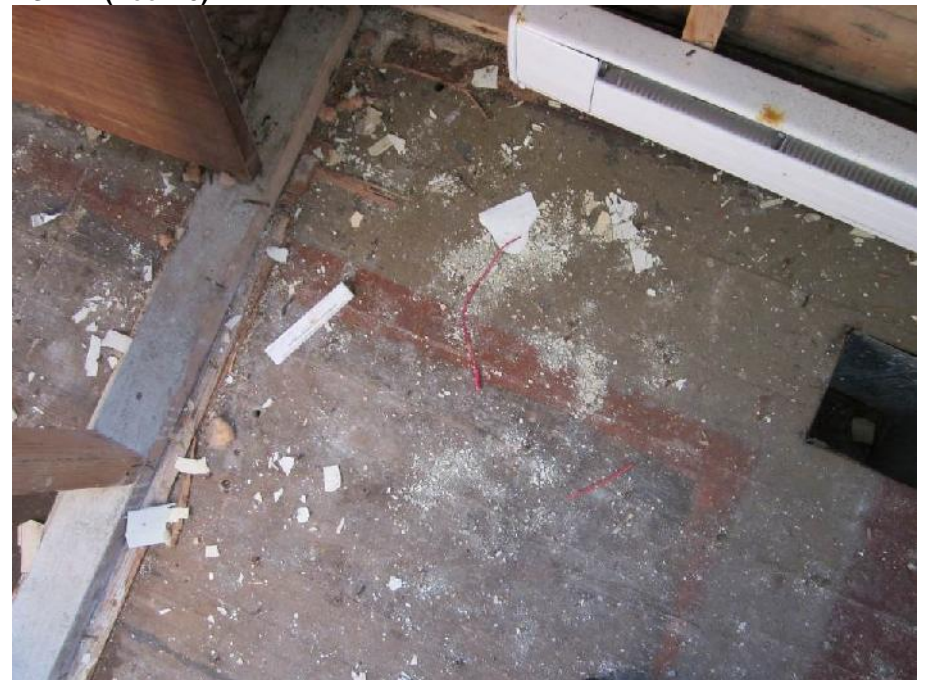
Photo 32: View of red paint on the floor in Room 5 (not sampled).
