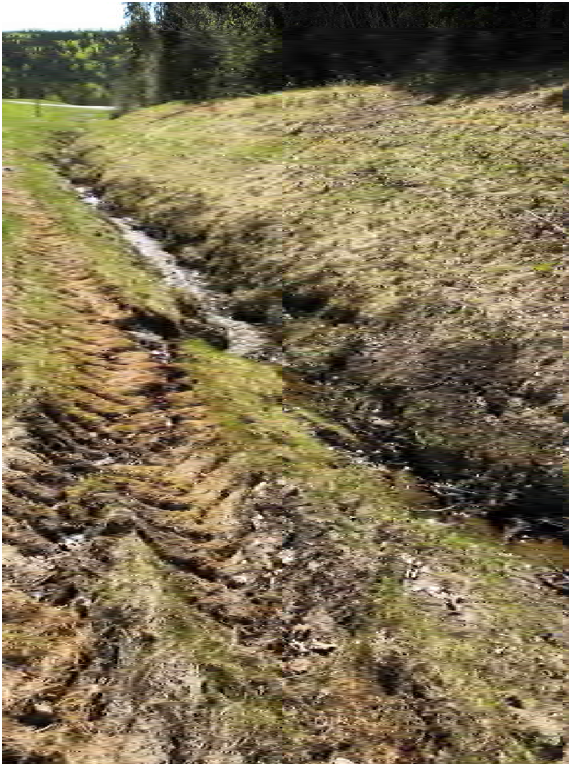
Photograph D-7: Ditch on the southwestern side of Alaska Highway (looking west)
