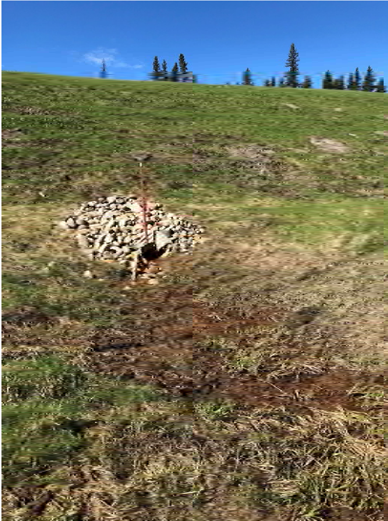
Photograph D-1: Damaged culvert outlet and swale running East on Highway fill
