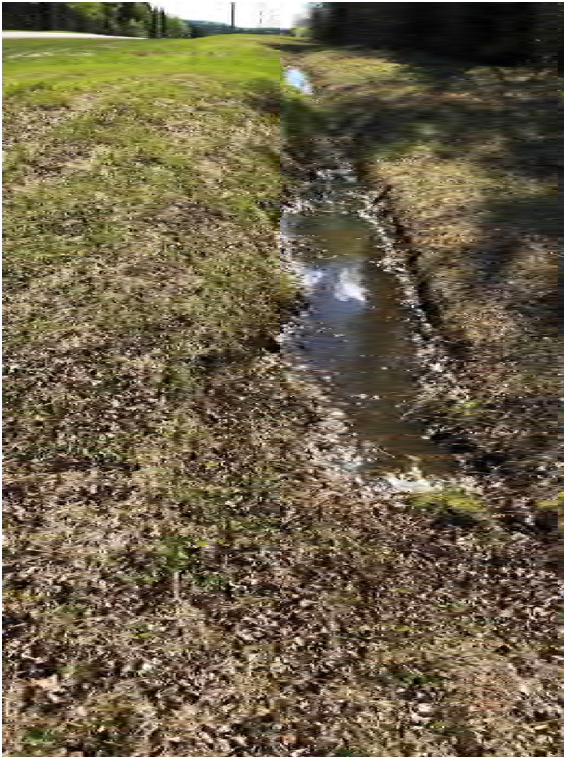
Photograph D-5: Ditch on the southwestern side of Alaska Highway (looking southeast)
