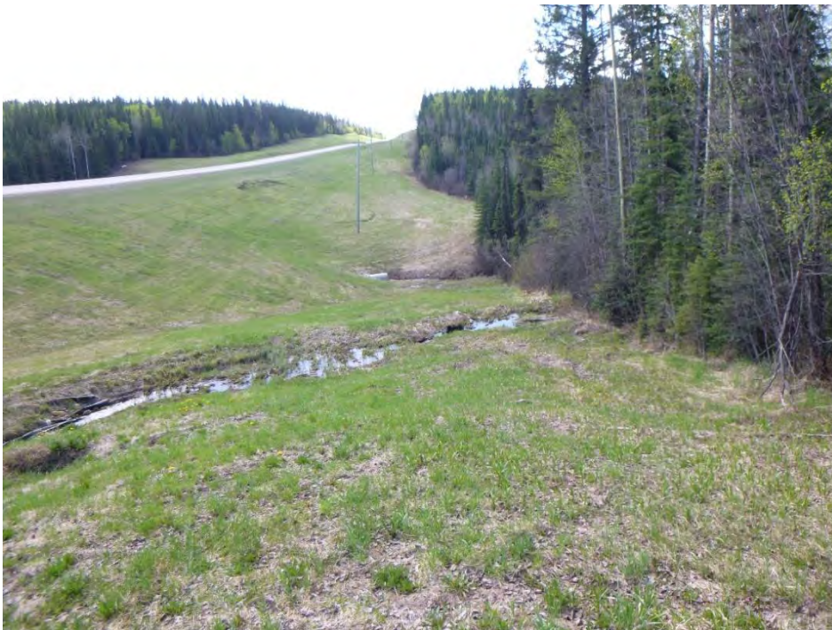
Photo 4: Surface runoff on the west side of the highway enters the unnamed stream at the culvert inlet in Reach 2.
