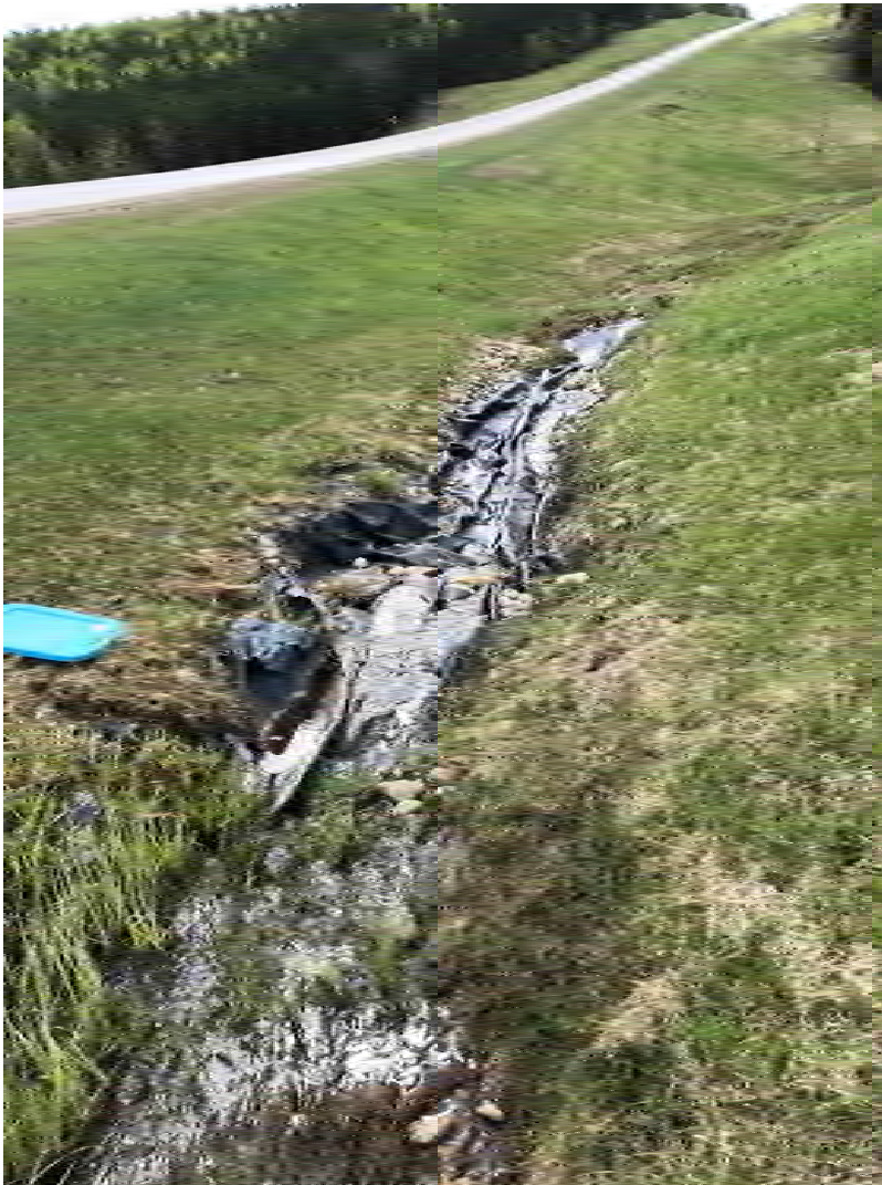
Photograph D-8: Ditch on the southwestern side of Alaska Highway (looking south)
