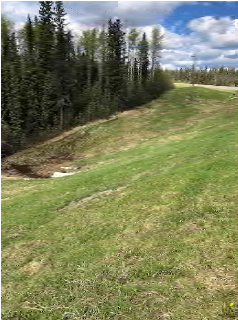
Photograph D-11: Southwestern side of Alaska Highway (looking north towards 1.2 m culvert)
