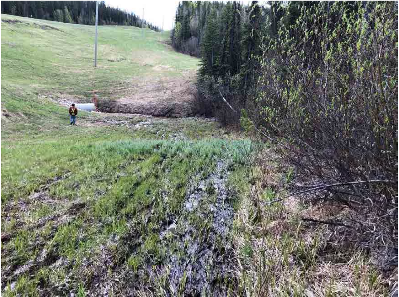
Photograph D-10: Southwestern side of Alaska Highway (looking south towards 1.2 m culvert)
