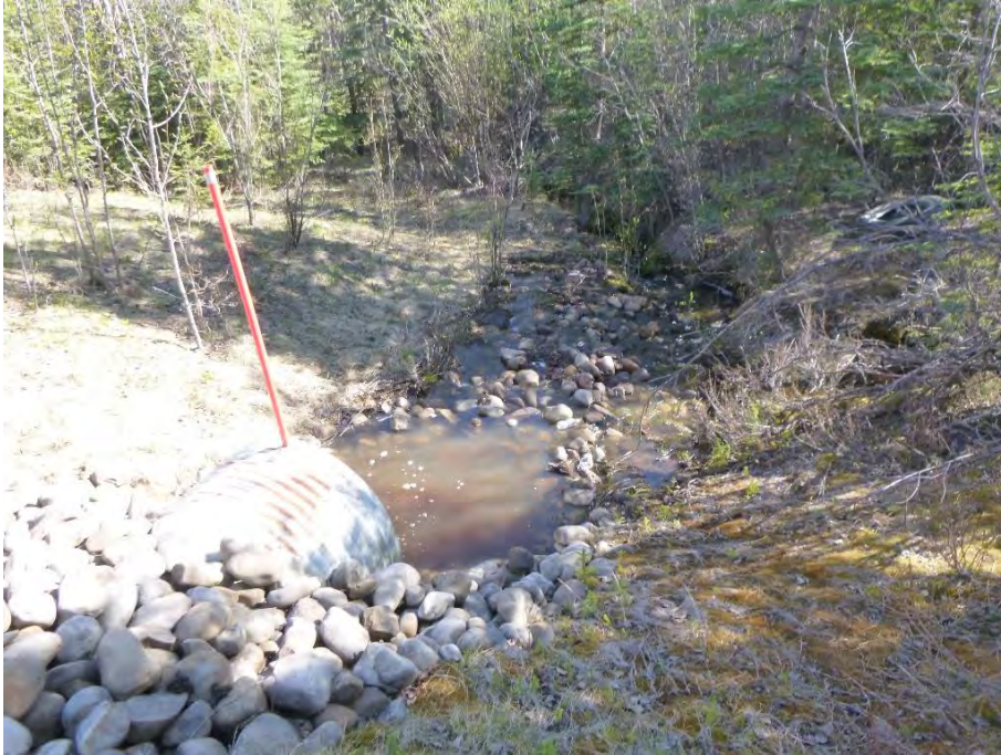
Photo 1: Upstream end of Reach 1 at culvert outlet, viewed downstream on 27 May 2020. Large cobble substrate placed as armouring during culvert installation and not the natural streambed substrate.
