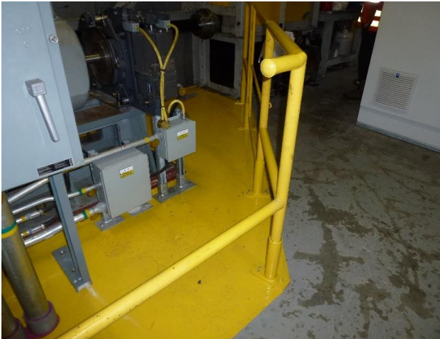
Photo 3: North tower 9peeling floor paint and bollards
