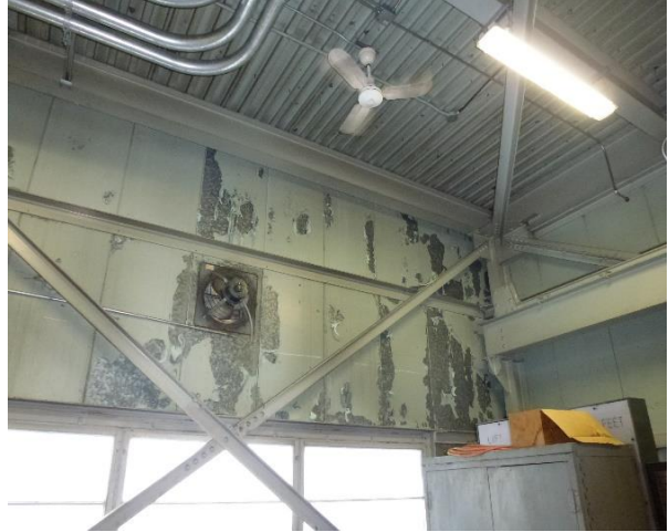
Photo 2: Peeling wall paint North Tower
