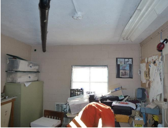
Photo 13: Ceiling Stucco old workshop
