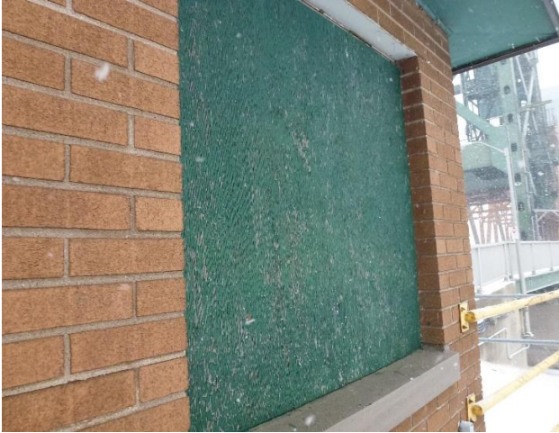
Photo 1 : Gatehouse peeling paint
