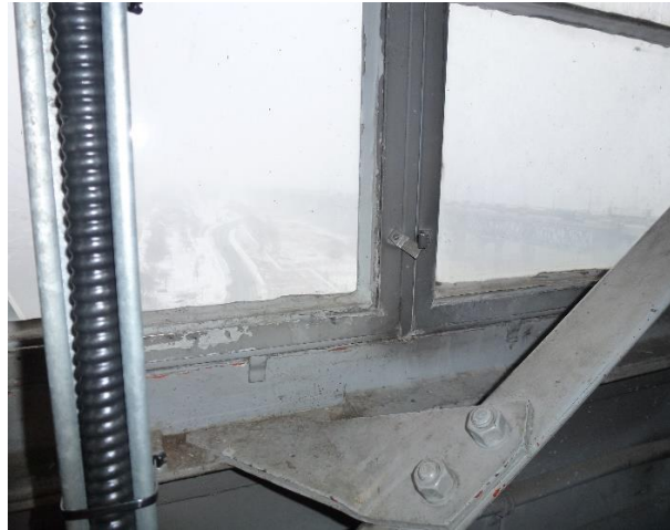
Photo 4: Window caulking South Tower
