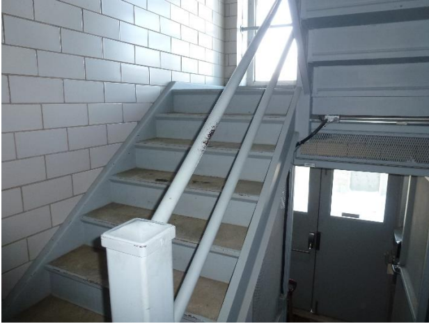
Photo 7: Control house stairwell wearing paint
