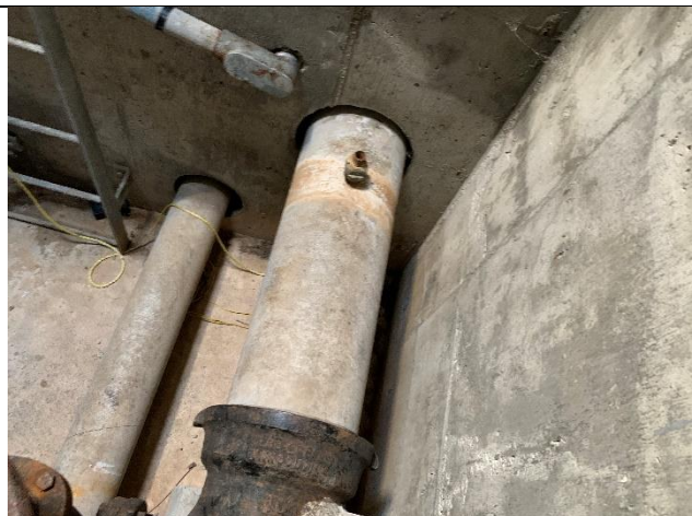
26: View of 10" inlet/outlet pipe along with 6" drainpipe
