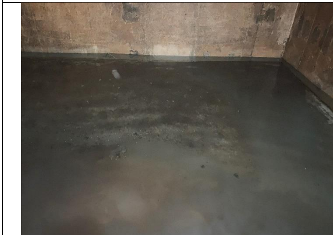
29: Up to 9" of accumulated silt near entrance to the tank
