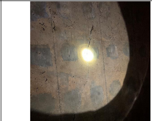
18: Diagonal concrete crack at dividing wall
