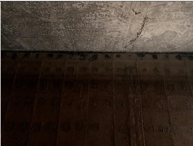
11: Concrete sealant material was noted on walls in cell 1
