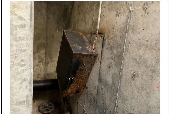
22: Loose electrical box inside control chamber
