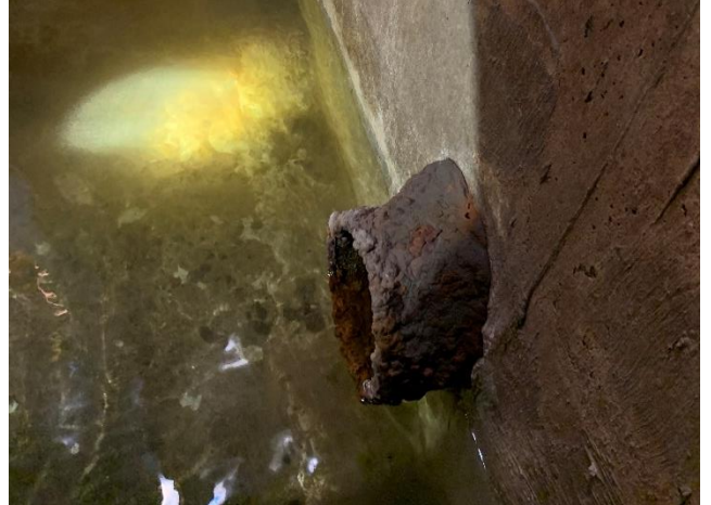
8: Corroded 8" inlet/outlet in south wall in cell 1
