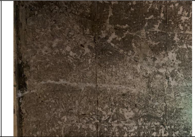
14: Minor concrete cracking on dividing wall
