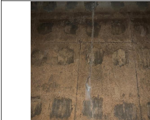
17: Noted more concrete crack on dividing wall
