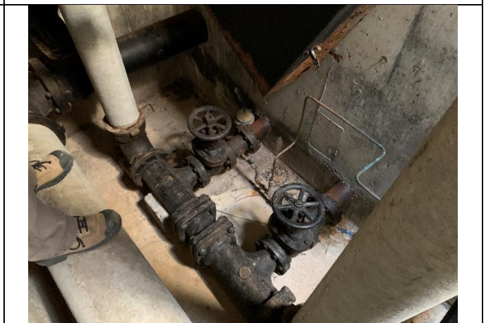
24: 4" drainpipes join 6" overflow pipe
