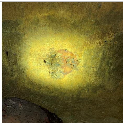
28: Minor concrete delamination is observed on south wall
