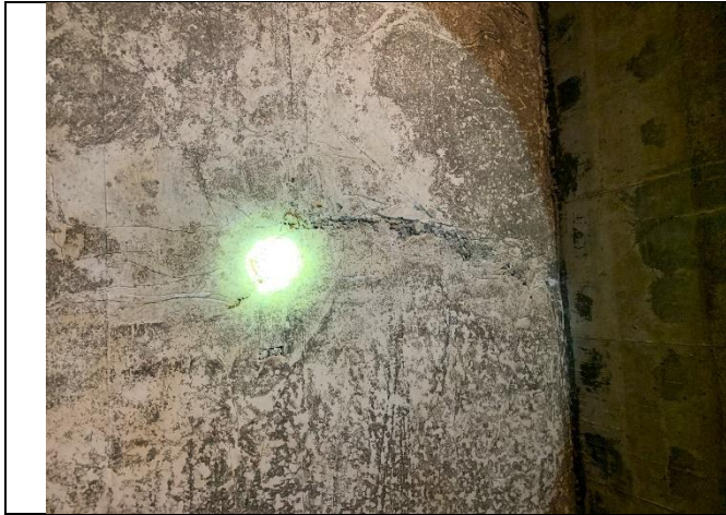
13: Minor cracking on top slab
