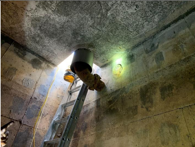
9: View of 6" overflow pipe along with sensor in cell 1
