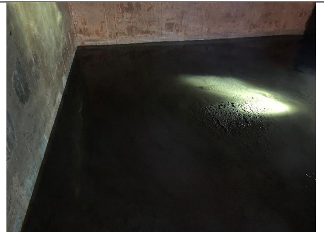
12: More accumulated silt at bottom of cell 1 up to 10"
