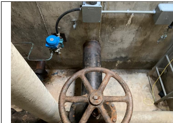
25: 8" inlet/outlet pipe to cell 2 located above 4" drainpipe
