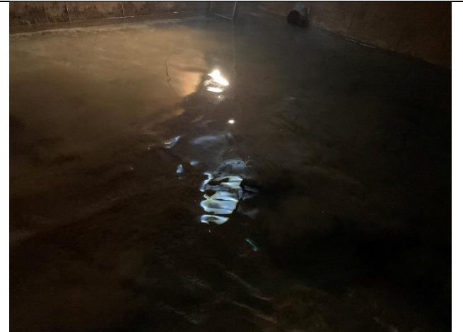
10: Up to 10" of ponding water and accumulated silt
