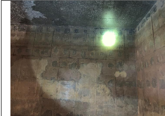
19: Moisture and leakage of water was observed on northern wall due to proximity of vegetation
