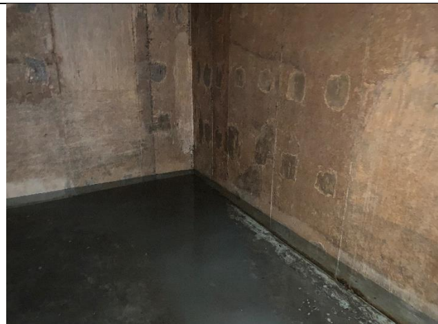
30: Concrete sealant patches were visible on cell 2 walls
