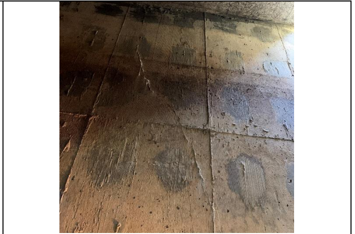
20: Minor crack on western wall of cell 1
