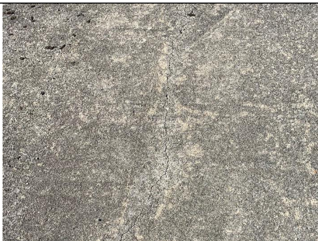
3: Visible hairline crack on top slab
