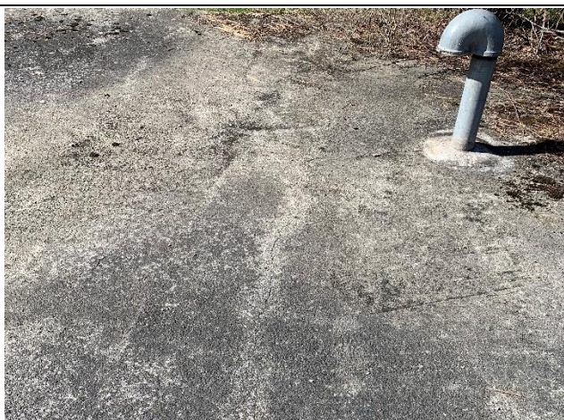
4: Extend of crack on top slab towards west
