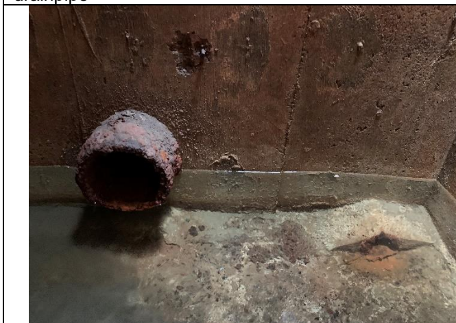
27: View of 8" inlet/outlet pipe along with 4" drainpipe in cell 2
