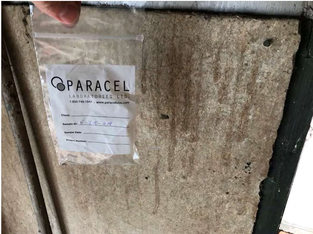
Photo 4: Asbestos-containing transite board. See sample F-TB-2A.
