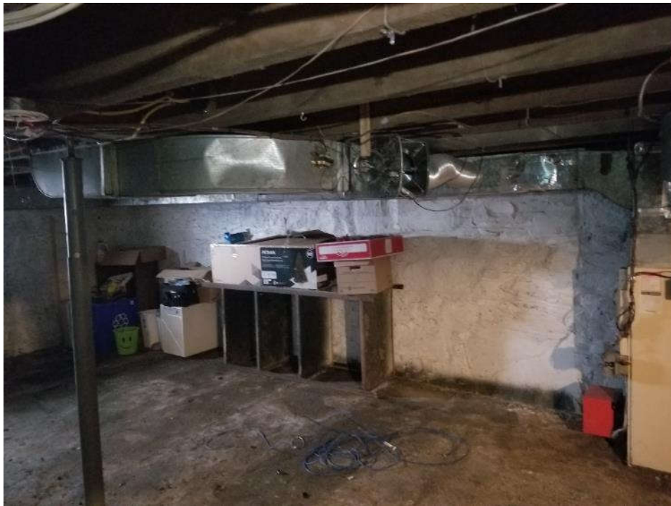
Photo 4: View of the white lead-based paint on the wall in the basement of the subject dwelling.
