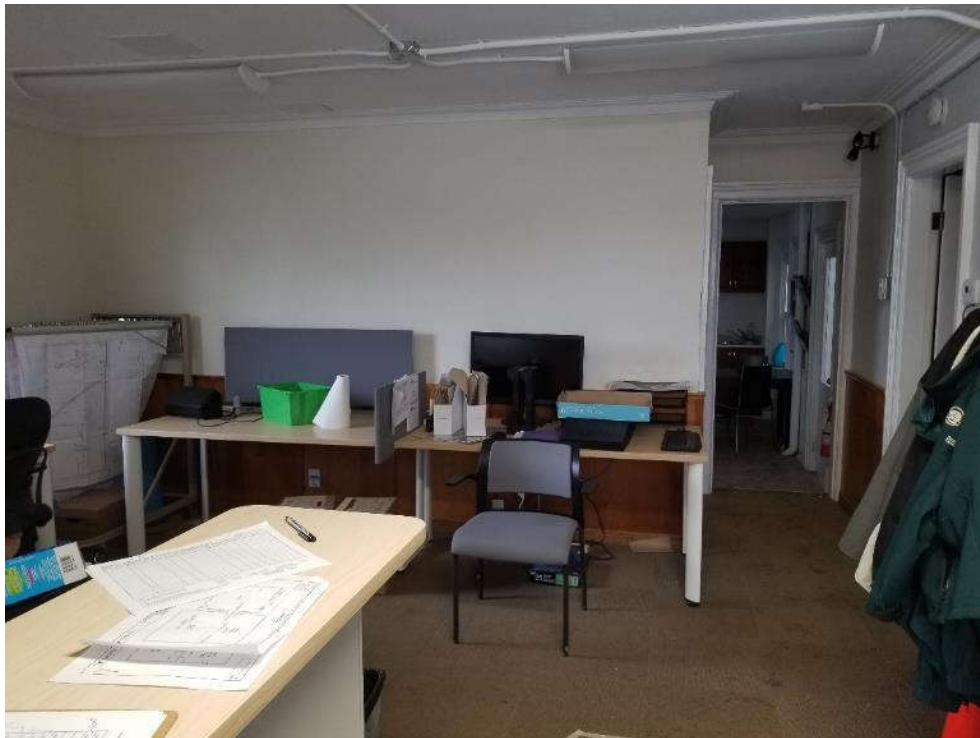
Photo 2: View of the asbestos-containing plaster walls and ceiling throughout the subject dwelling.
