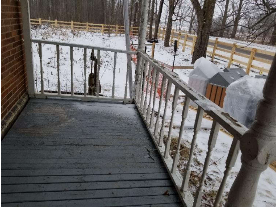
Photo 5: View of the white lead-based paint in the porch of the subject dwelling.
