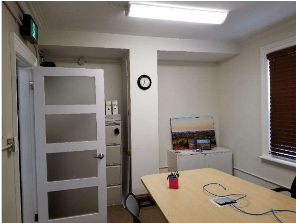
Photo 6: View of suspect mercury-containing fluorescent light tubes on the ceiling throughout the subject dwelling.
