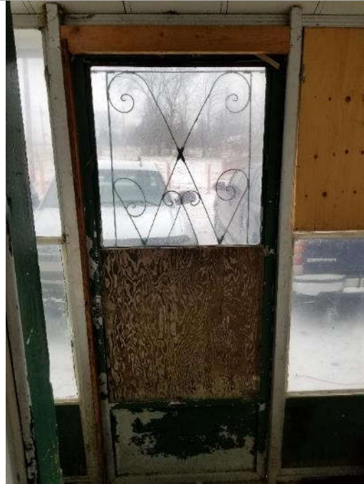
Photo 3: View of the green lead-based paint on the west door frame of the subject dwelling.
