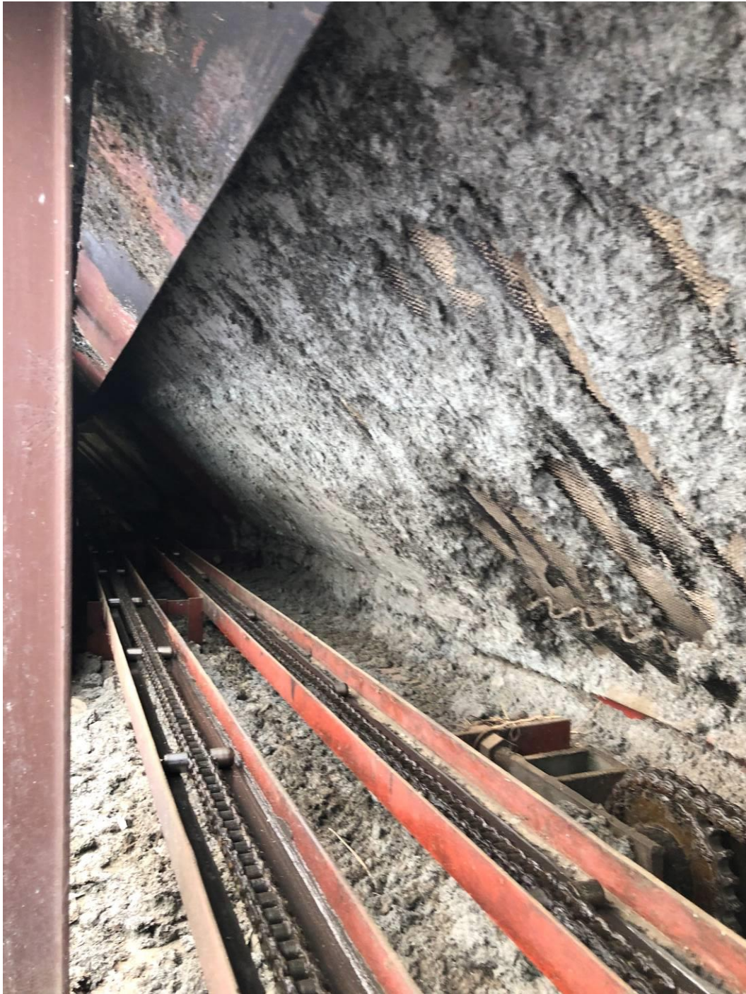
Photograph 1: Door track and chain system as viewed from opening created at roof level (reference Drawing A1-011227-20, Sheet 5). Photograph taken at west roof level, between dome and concrete door pocket area, looking east. Note spray-applied fireproofing on sloped transite siding (at right of image) and spray-on fireproofing debris among door chain and track system.
