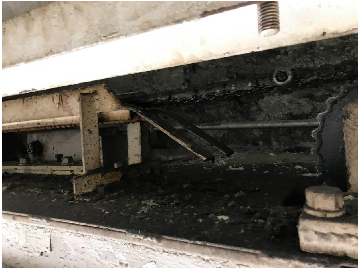
Photograph 3: Door track and chain system above hanger doors and beneath dome (west of gridline 4 as per Drawings A1-011227-20). Note the spray-applied fireproofing debris. Chain, mechanical tracks, and associated mechanical equipment considered contaminated with asbestos and require decontamination under asbestos precautions.
