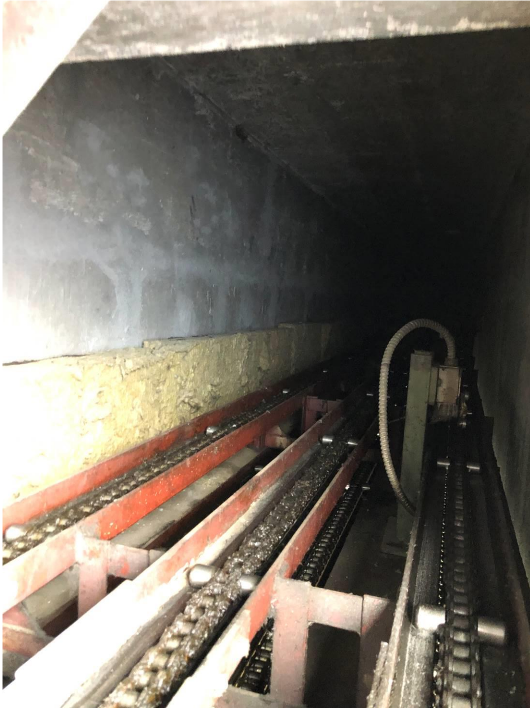
Photograph 2: Door track and chain system as viewed from opening created at roof level (reference drawing A1-011227-20). Photograph taken at west roof level, between dome and concrete door pocket area, looking west into door pocket void. Note the lack of spray-applied fireproofing on concrete walls and the non-asbestos insulation applied to the wall. Chain, mechanical tracks, and associated mechanical equipment considered contaminated with asbestos and require decontamination under asbestos precautions. Also note, solid “floor” ends shortly beyond support post, with majority of track system open to the door pocket area beneath.
