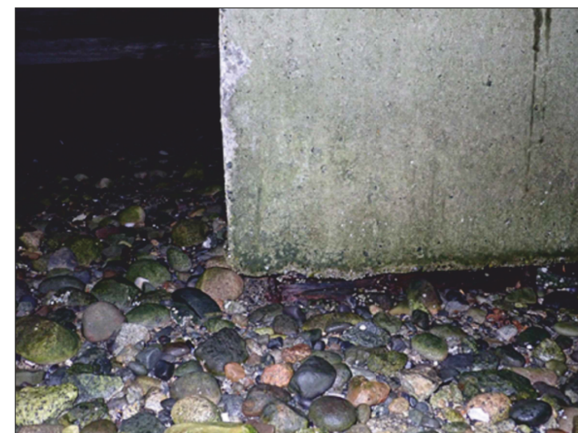
E CONCRETE FOUNDATION WITH SPALLING (PILE 11-D) S-101 NTS
