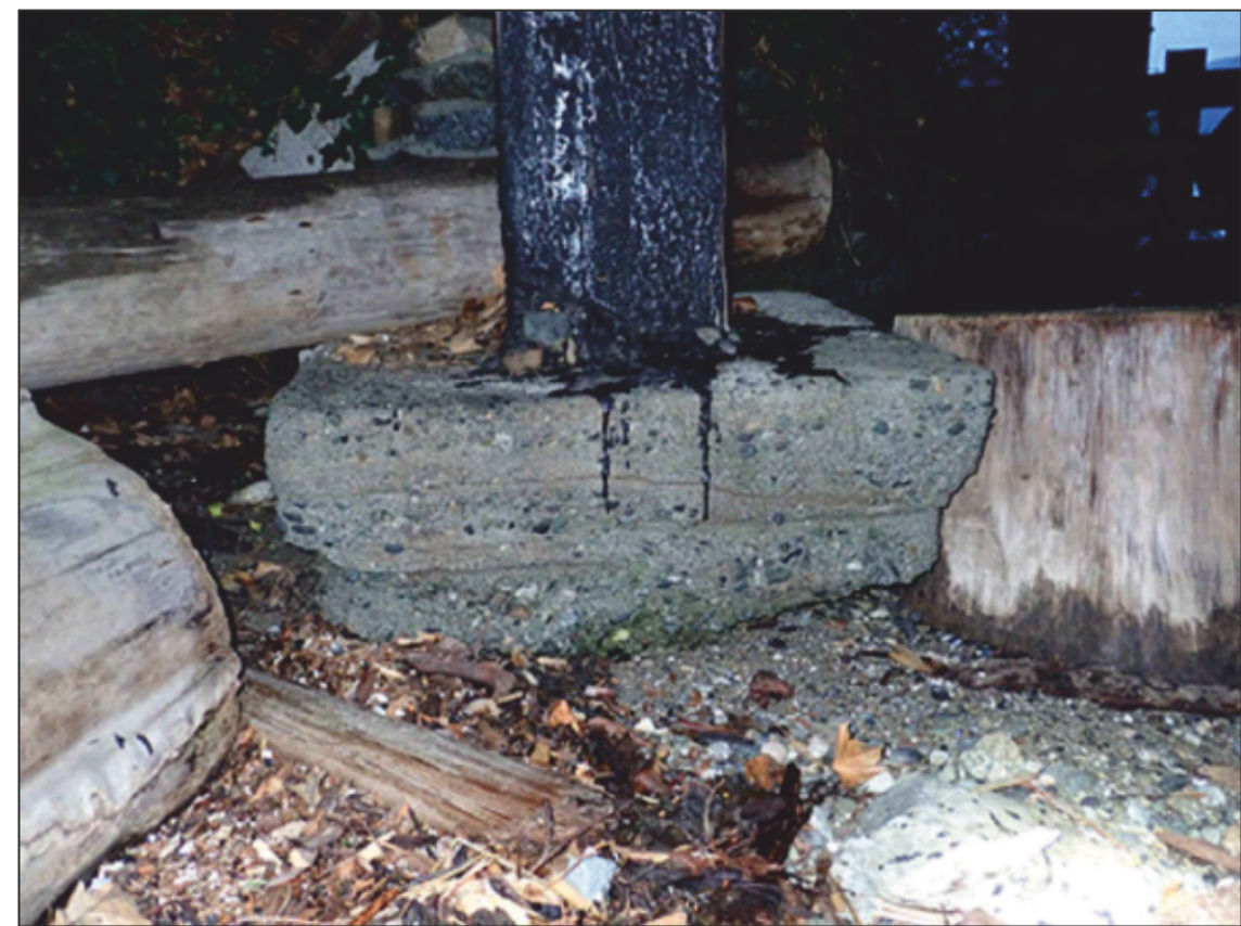
B CONCRETE FOUNDATION WITH SPALLING (PILE 9-C) S-101 NTS
