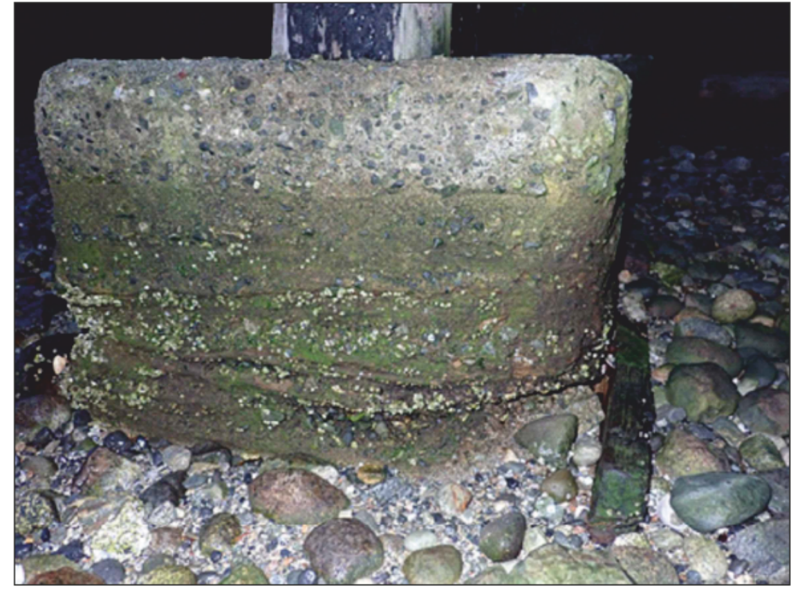
D CONCRETE FOUNDATION WITH SPALLING (PILE 11-A) S-101 NTS
