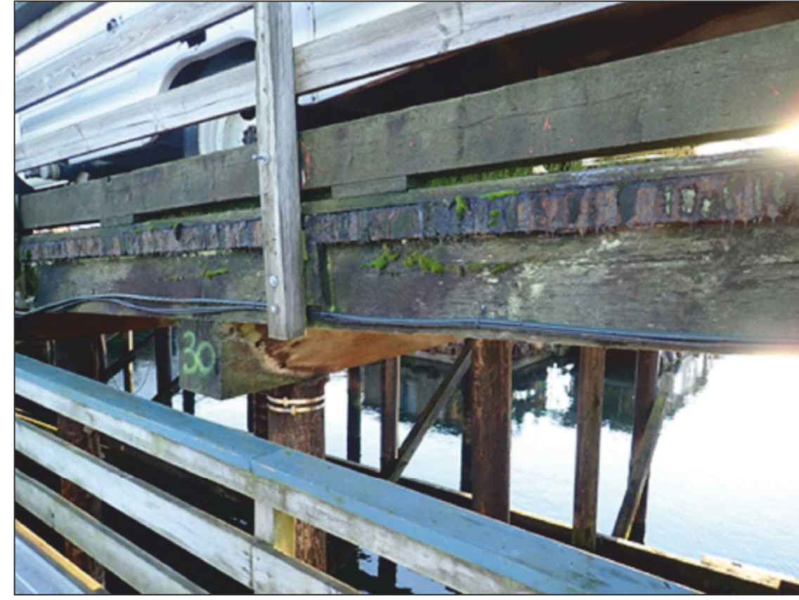
I DAMAGED STRINGER - PILE CAP 28 TO 38 SCALE: NTS
