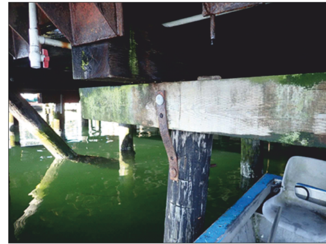
H RECENTRE PILE CAP ONTO PILE AT BENT 49 PILE L S-102 NTS
