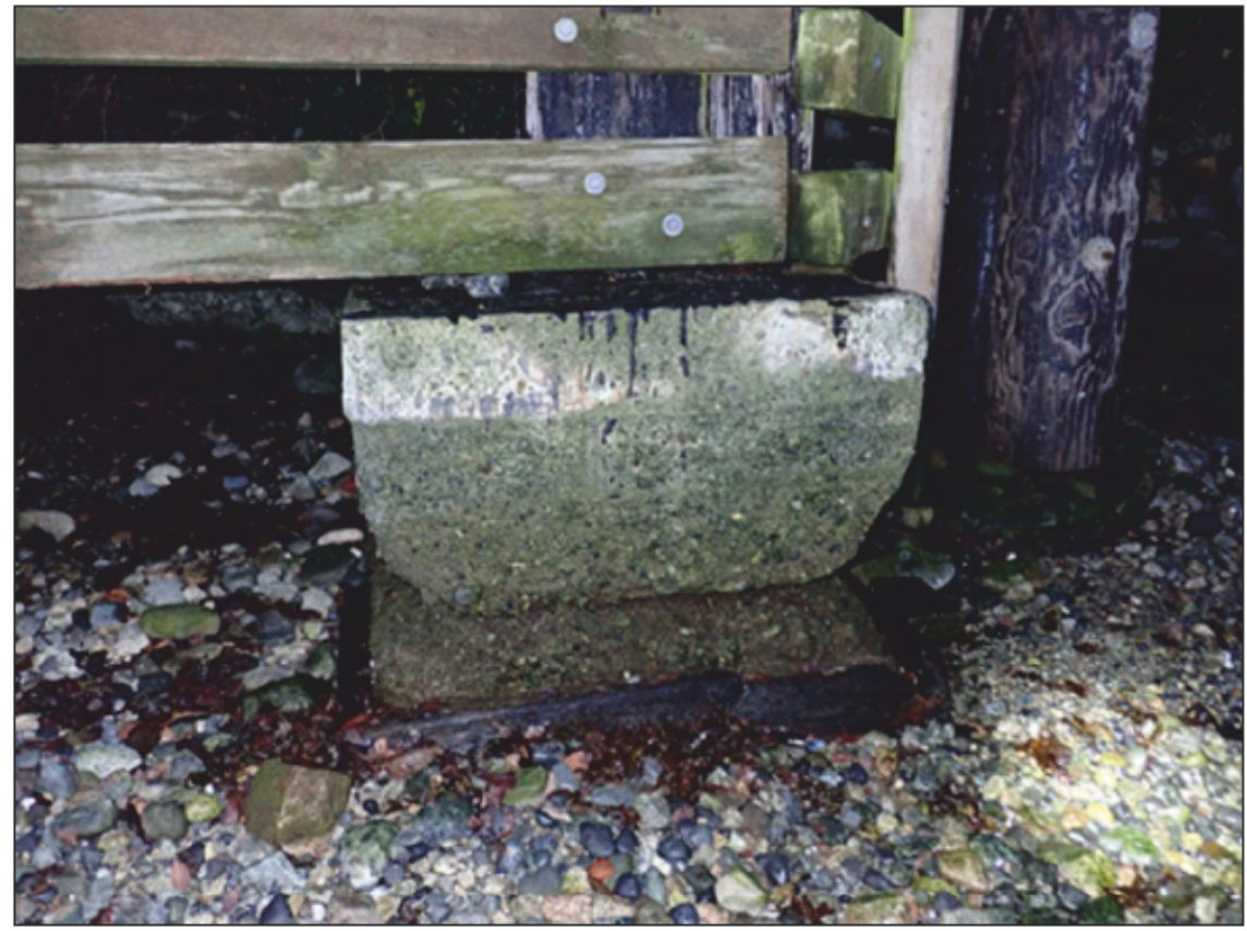
C CONCRETE FOUNDATION WITH SPALLING (PILE 10-D) S-101 NTS
