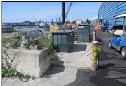
AUTHORIZED Sanitary Sewer Discharge point, Lift Station #11.
