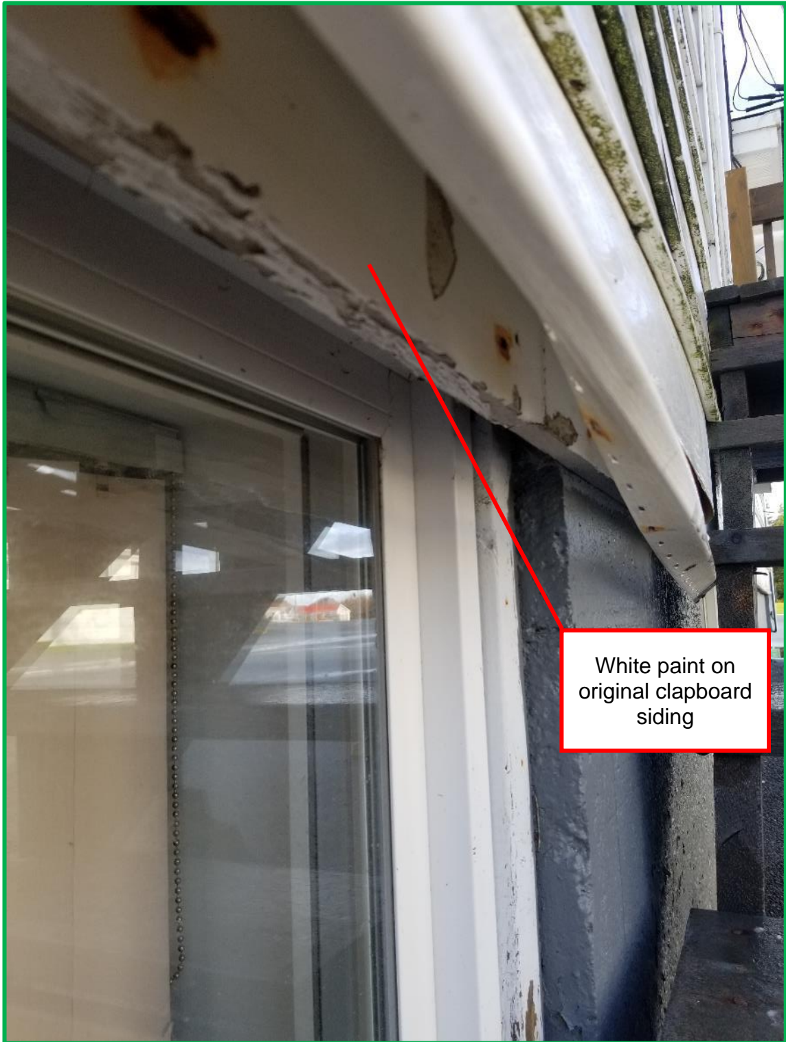
Photograph #5: Sample NL7689-L07 sample location. White paint on original clapboard siding (beneath existing vinyl siding). Photo taken on November 16, 2020.
