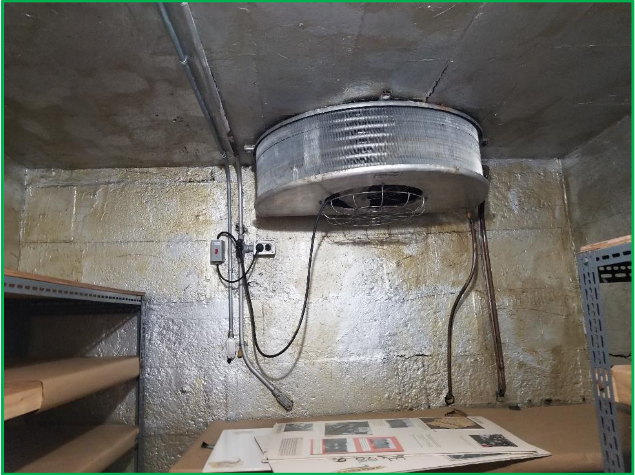
Photograph #6: Example of cooler unit potentially containing ODS within the Basement Cellar. Photo taken on November 16, 2020.
