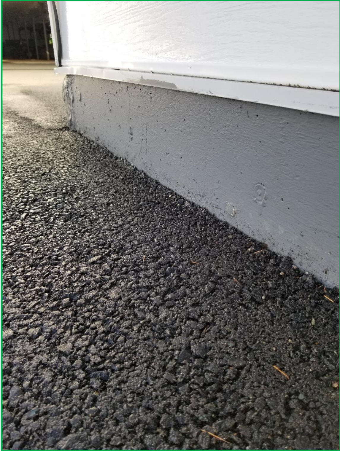
Photograph #4: Sample NL7689-L06 sample location. Grey paint on building foundation. Photo taken on November 16, 2020.
