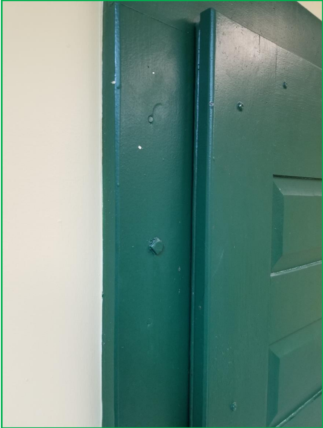
Photograph #2: Sample NL7689-L03 sample location. Green paint on Basement Cellar door. Photo taken on November 16, 2020.
