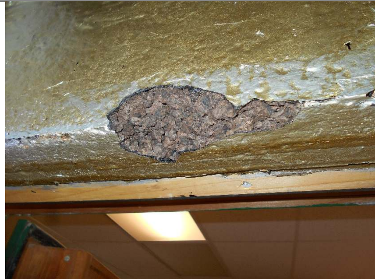
Photo 7-34: view of damaged wall in Room 13
