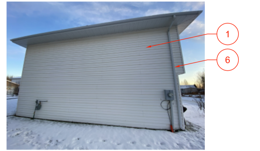
4. SIDE VIEW WITH GAS AND HYDRO METERS
