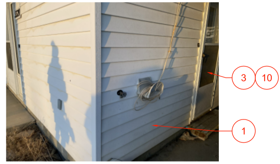
7. SERVICE PENETRATIONS AROUND CARPORT
