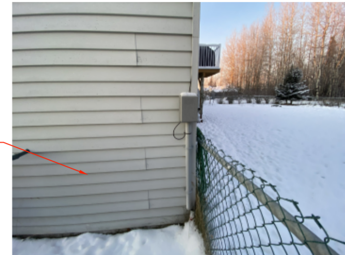
6. CABLE BOX AT SIDE
