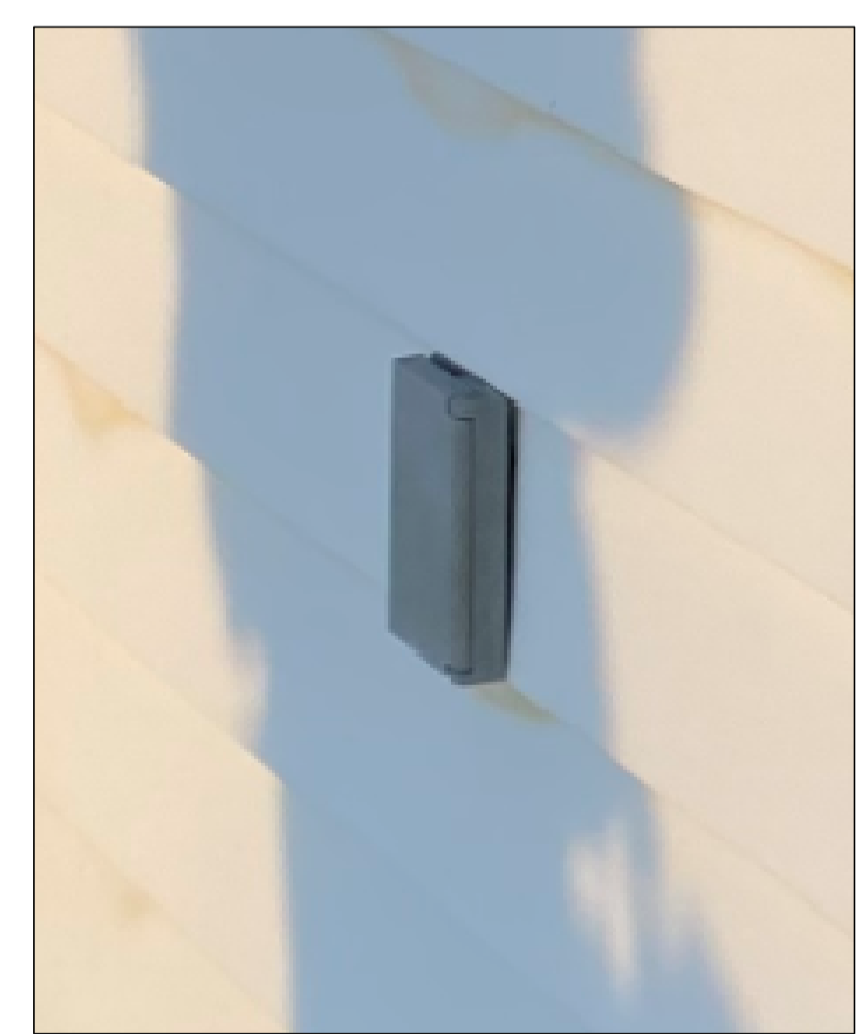
TYPICAL ELECTRICAL BOX
