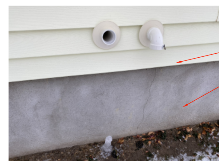
8. EXHAUST PIPES AT SIDE
