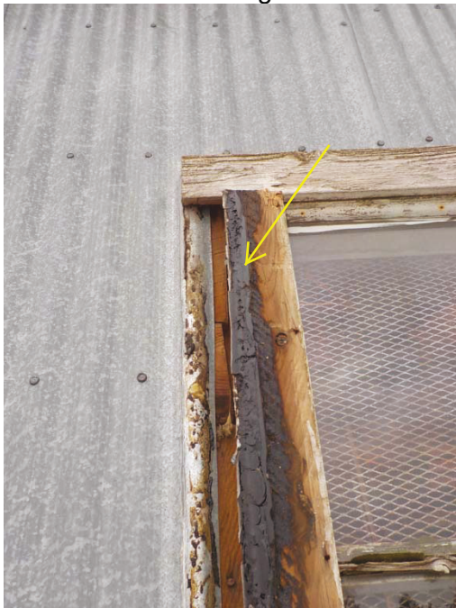
Photograph 3: Asbestos-containing black mastic beneath the window casing on the west side of the Building at sample location A1. The photograph was taken following removal of the casing for analysis of lead in paint via TCLP methodology.
