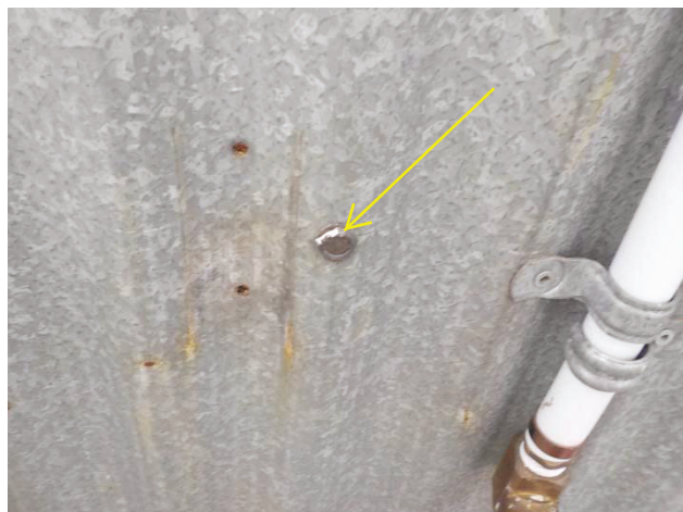
Photograph 8: Suspect lead grommets were identified on the exterior of the Building.
