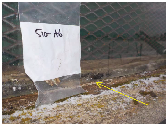
Photograph 4: Asbestos-containing tan mastic (window putty) on the window between the frame and the pane. The photograph of sample location A6 is used to represent sample A4 as it best depicts the position of the ACM in relation to window construction.
