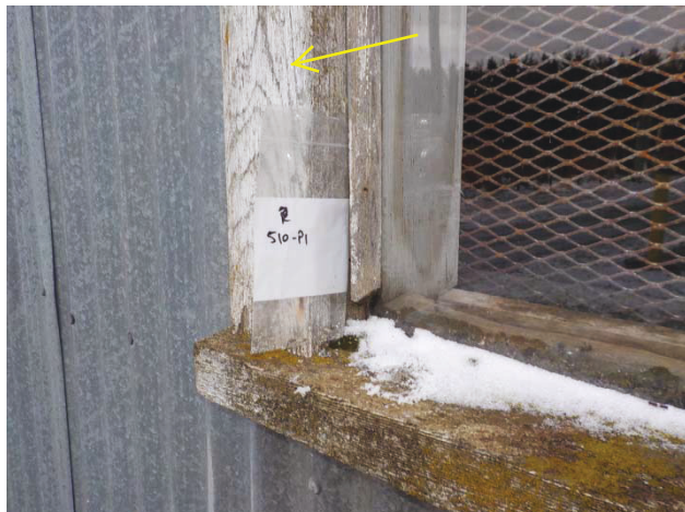
Photograph 5: Lead-containing white paint collected from the window frame on the west side of the Building.
