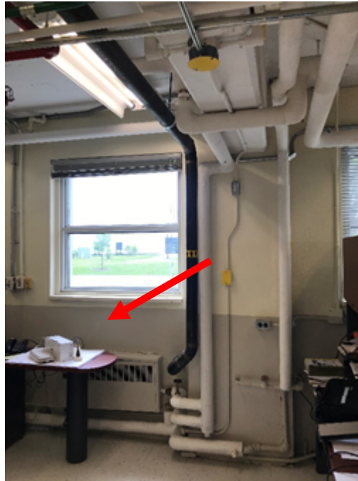
Photo 1: Friable (when destructively disturbed) smooth white over grey plaster applied to the walls throughout the building were confirmed to contain 0.5%- 1% Chrysotile asbestos (DST Sample ID 02002246.000-06A-E).
