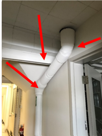
Photo 4: Friable Aircell pipe insulation containing >75% Chrysotile asbestos (historical Oakhill Sample ID U62-03A) and pipe fitting insulation containing 30-50%, >75% Chrysotile asbestos and 5-15% Amosite asbestos (historical Oakhill Sample ID U62-04A and 05A) were identified on the drain pipe located on the second floor hallway outside room 212.
