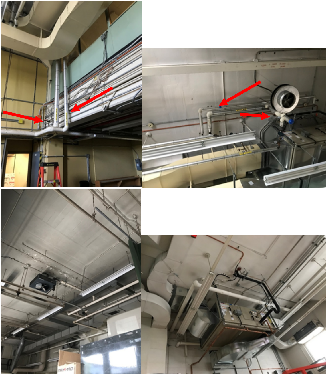
Photo 5-8: Insulated pipe fittings were observed throughout the building on the LPC and LPS lines. Aircell pipe insulation is assumed to be present beneath the metal jacking on each line.
