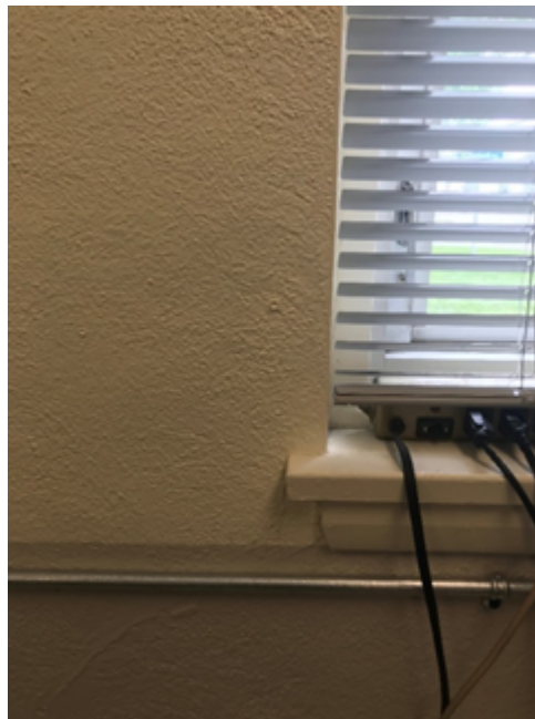
Photo 2: Friable (when destructively disturbed) grey textured plaster applied to the walls and perimeter columns throughout the building were confirmed to contain 0.5% Chrysotile asbestos (DST Sample ID 02002246.000-05C-E).
