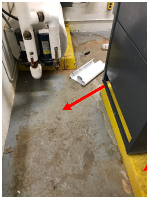
Photo 11: Grey paint applied to the floor and yellow paint applied to the concrete pads of the boiler room contain 348 and 1020 ppm lead (DST Sample 02002246-LP01 & 02002246-LP02).
