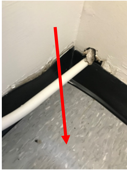
Photo 3: Non-friable black mastic concealed beneath 12" x 12" vinyl floor tiles with grey and white streaks observed throughout the 2 nd floor hallway, room 203, 203A and 204, was confirmed to contain 3% Chrysotile asbestos (DST Sample ID 02002246-08A-C). Black mastic was also observed beneath the carpet in room 212 and was confirmed to contain 3% Chrysotile asbestos (DST Sample ID 02002246.000-10A-C).
