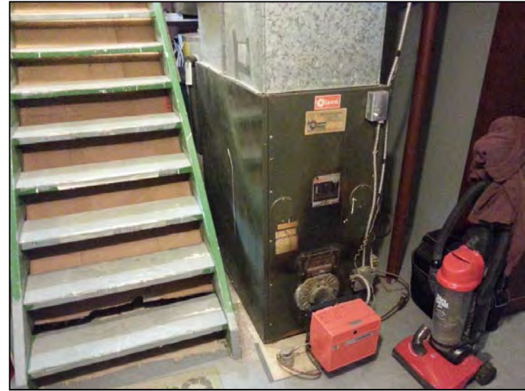
Photo 18: View of the heating oil-fueled furnace in the basement.
