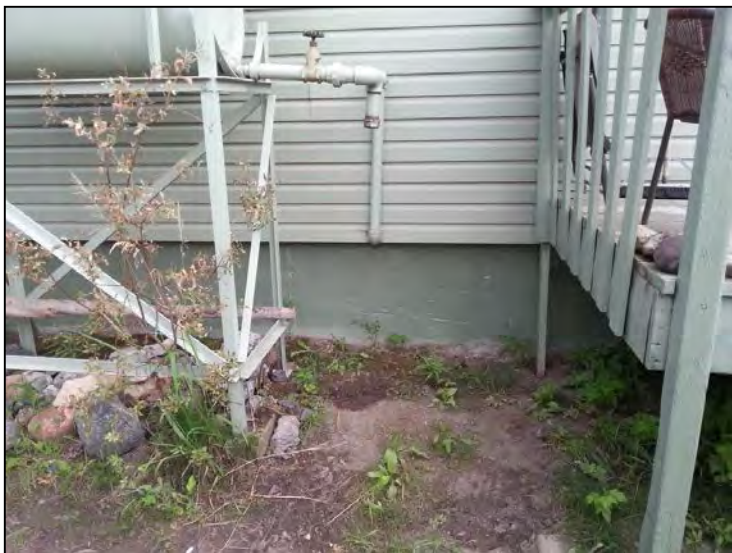
Photo 25: View of the western side of the heating oil AST, piping, and area underneath.
