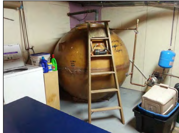
Photo 16: View of the potable water tank in the basement.
