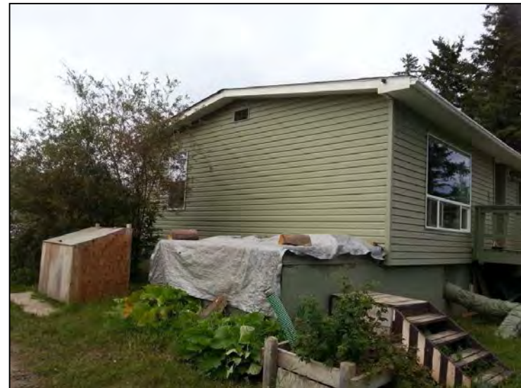
Photo 4: View of the western side of the residence and location of septic tank.
