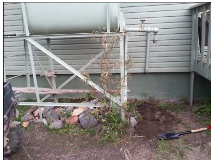
Photo 26: View of the location of the test pit dug underneath the valve of the heating oil AST.
