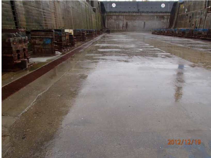
Photo 7: Poor drainage (no positive sloping towards drains)
