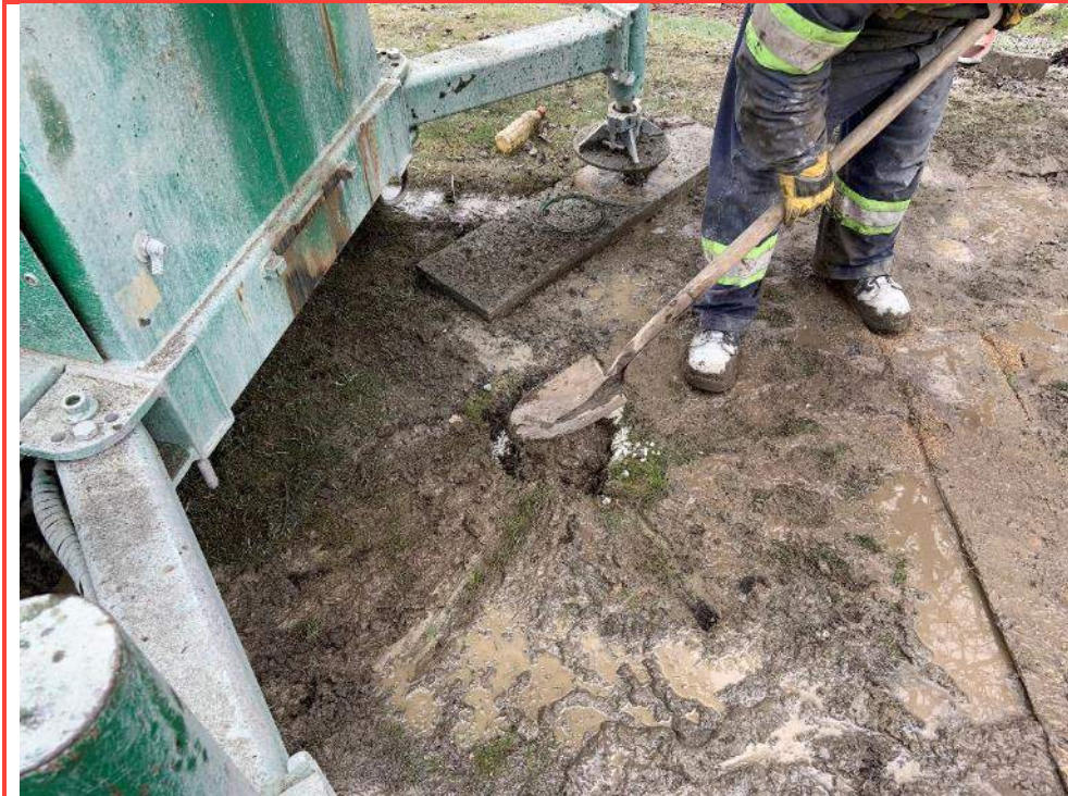
Photo 49: BH20-01A backfilled using bentonite chips and thin lift of native soil at surface.
