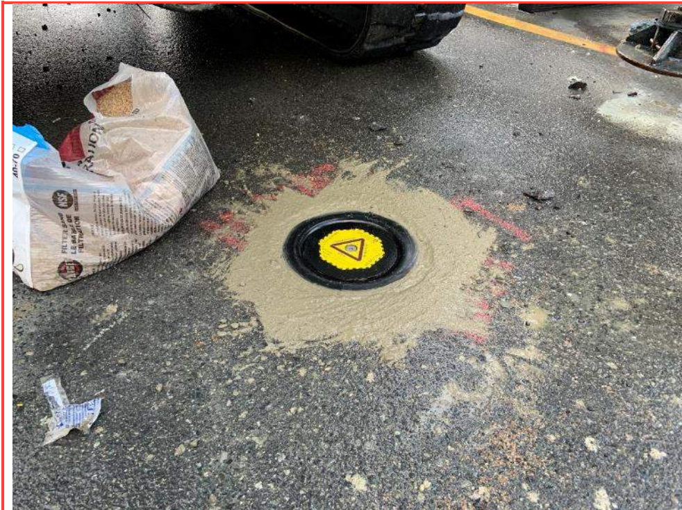
Photo 39: Monitoring well flush mounted to pavement at BH20-07.
