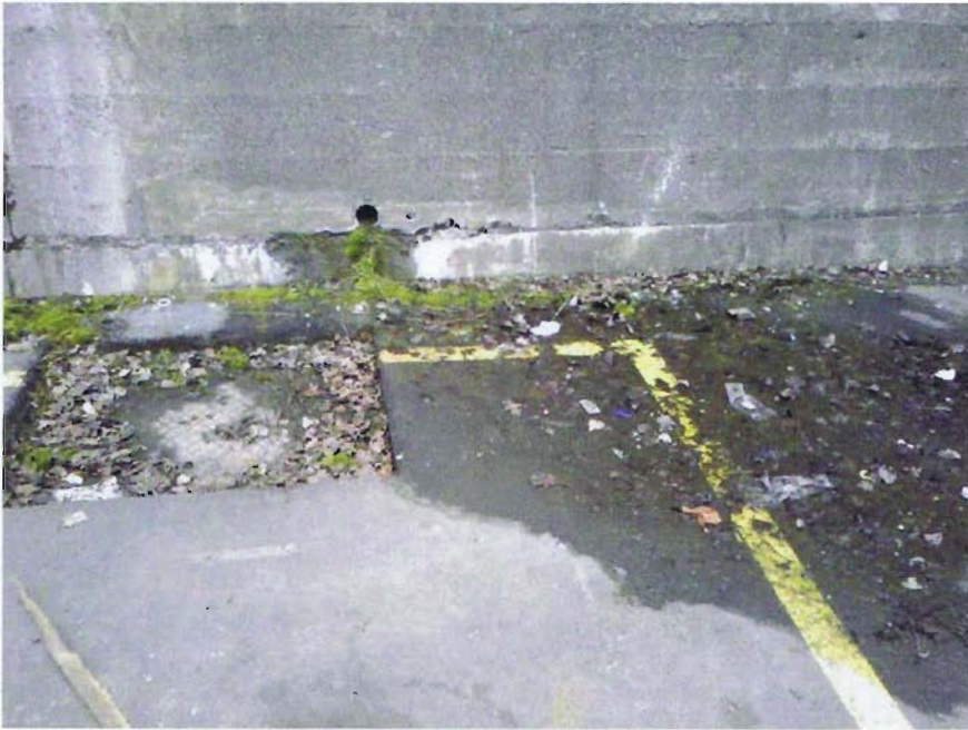
Photograph 5: Seepage through retaining wall along north side of dock craneway.
