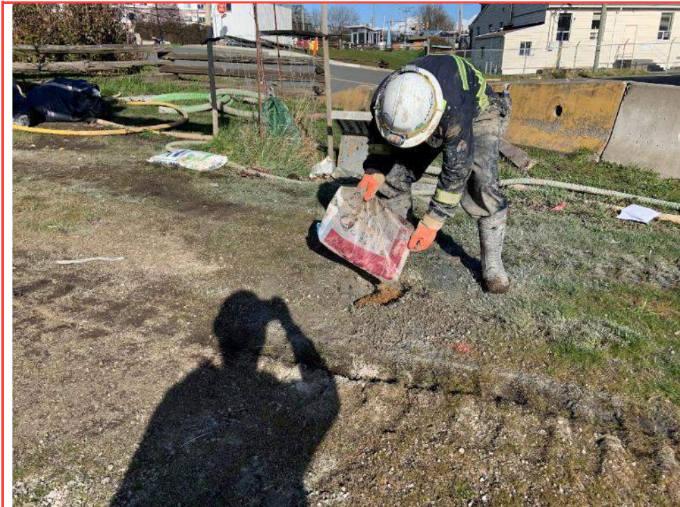
Photo 57: Contractor backfilling BH20-03 up to existing grade using bentonite chips and a thin lift of filter sand.
