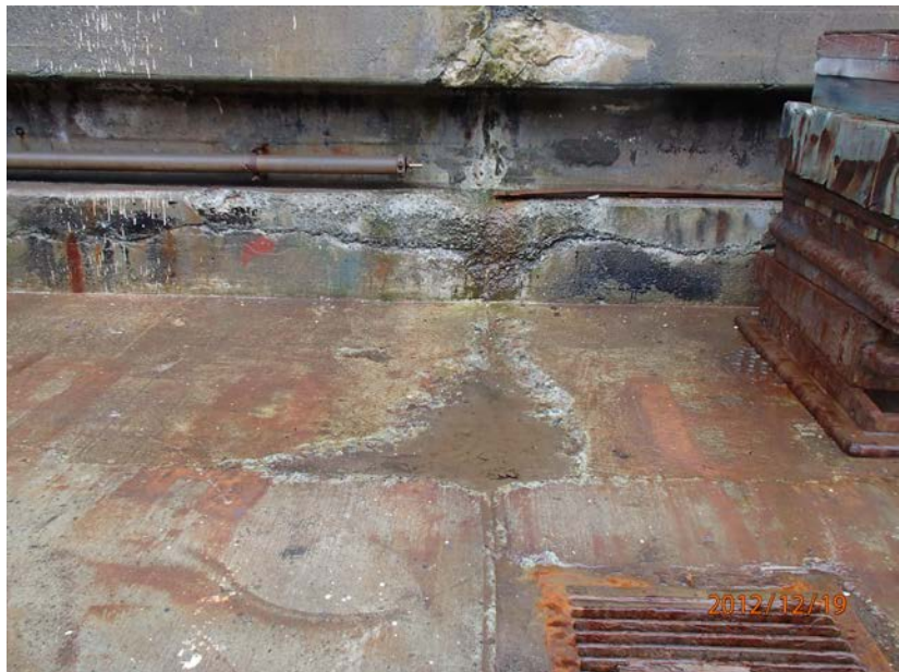
Photo 4: Deterioration of slab surface
