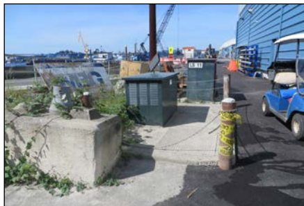
AUTHORIZED Sanitary Sewer Discharge point, Lift Station #11.
