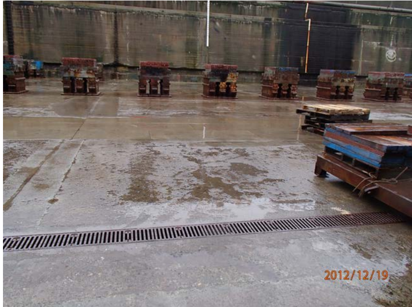
Photo 3: Typical slab surface with localized damage
