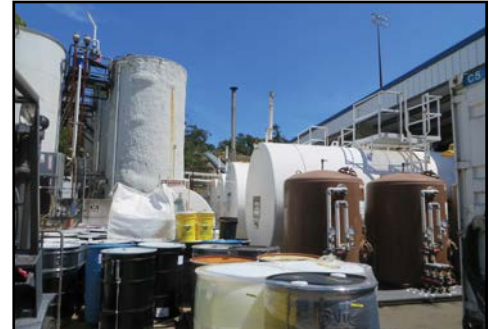
ADEQUATE containment of odorous waste.
