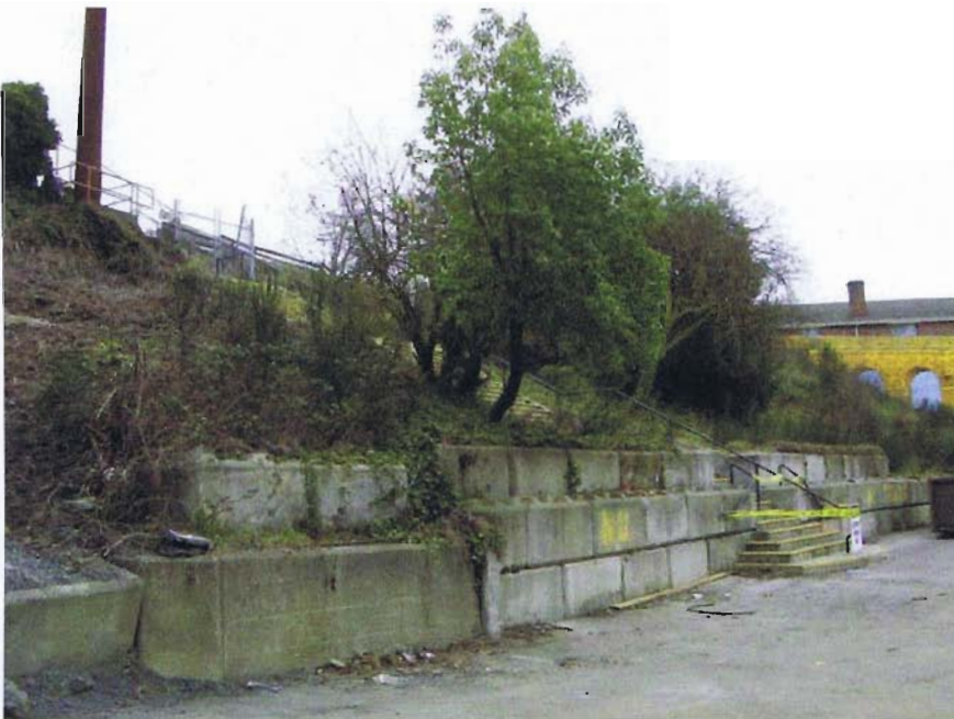
Photograph 4: Storm drain cover at toe of slope.
