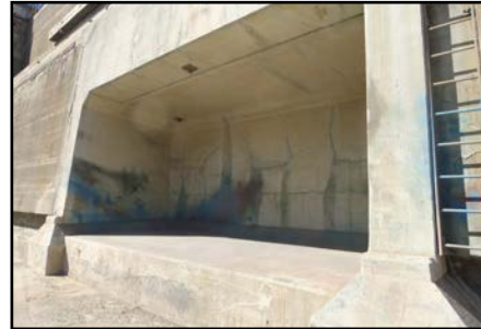
Paint overspray due to INADEQUATE containment stabilizer pocket doors.
