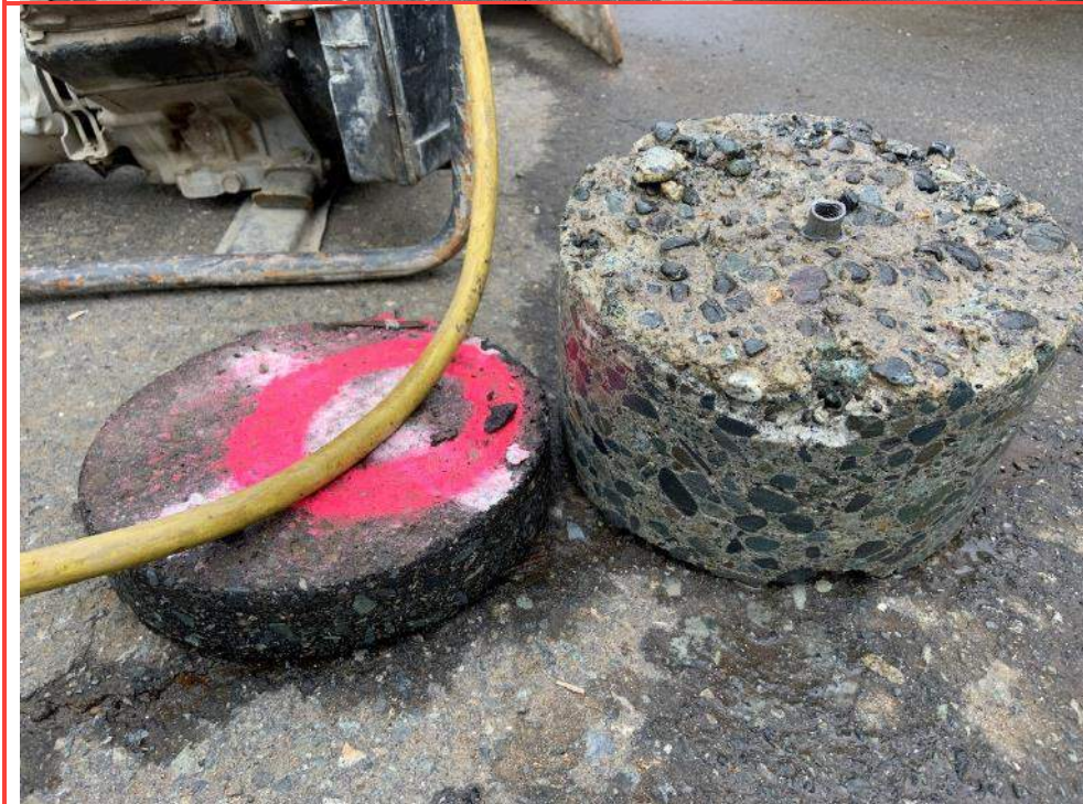
Photo 4: Typical pavement structure at east end of graving dock (i.e. 25-75 mm asphalt over 100-200 mm concrete)
