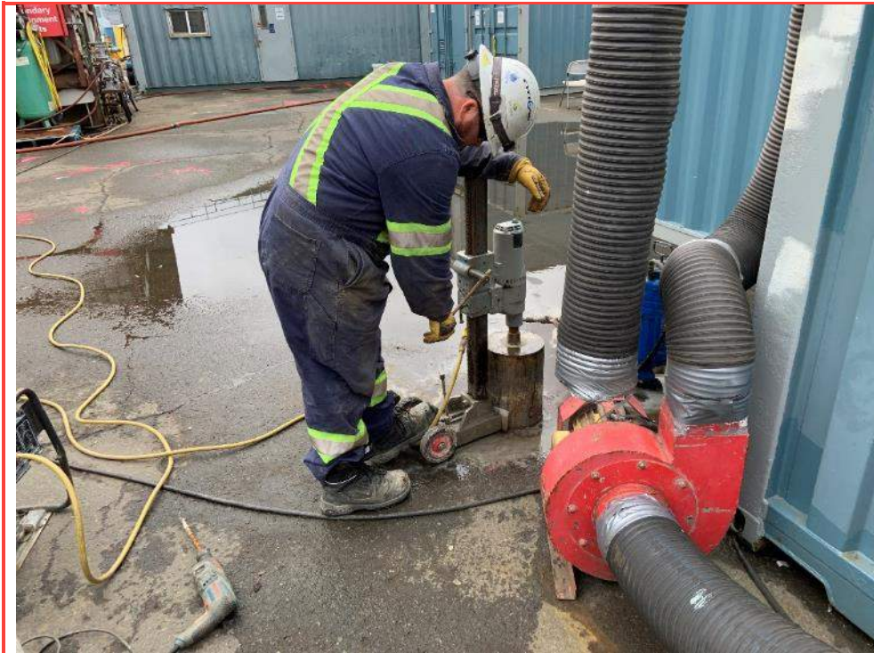
Photo 3: Typical coring of asphalt/concrete for lower boreholes located at east end of graving dock.
