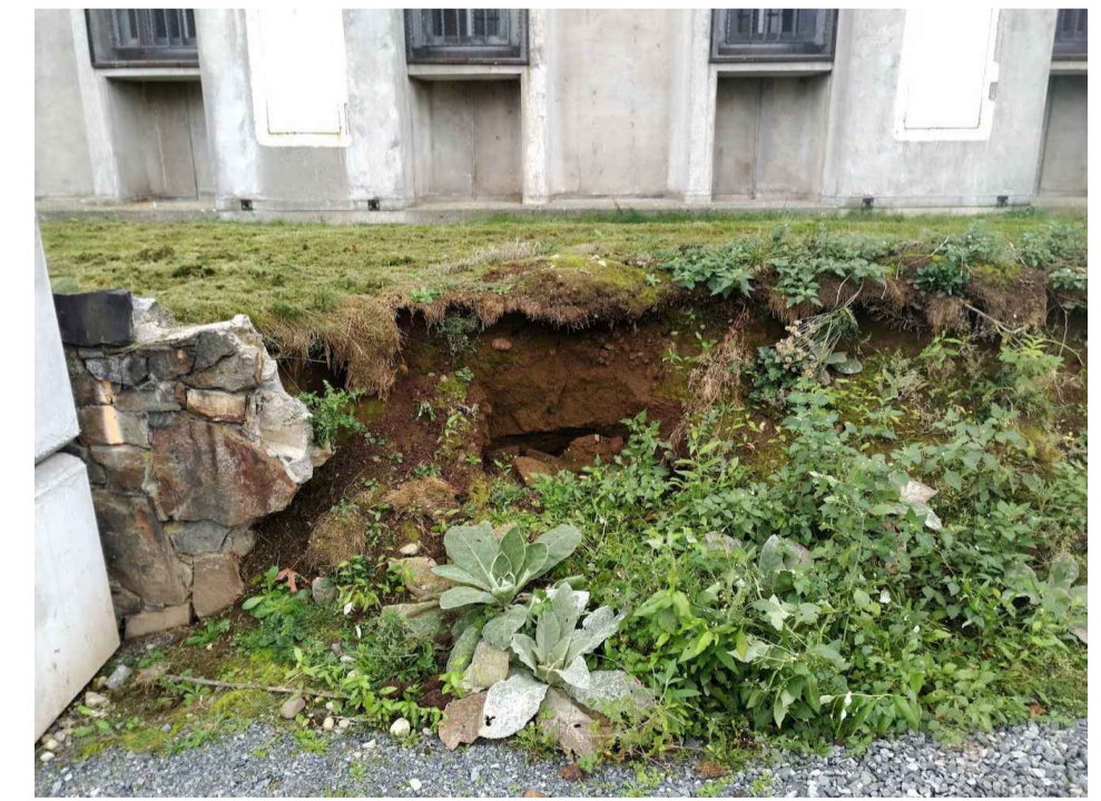
SITE PHOTO #2 DAMAGED SECTION OF ROCK WALL
