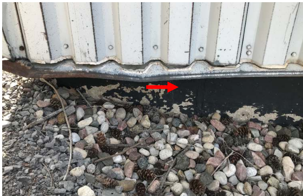
Photo 2. Exterior, Foundation: Black tar was confirmed to be non-asbestos containing (DST Sample ID 2759-ACM1-3). This material was confirmed to contain <5 ppm PCBs (DST Sample ID 2759-PCB1).
