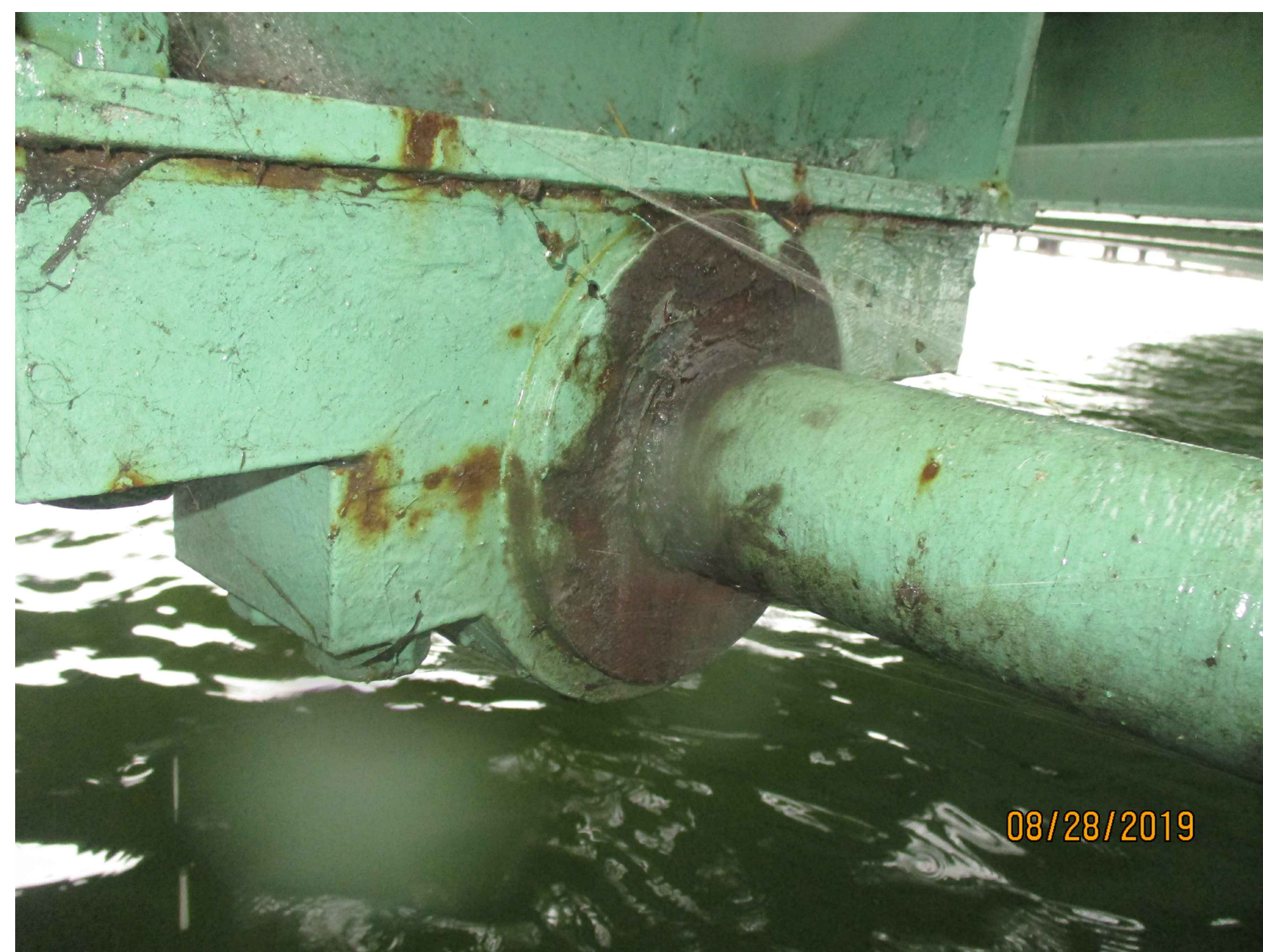
PHOTO OF CORRODED SPAN LOCK CROSS SHAFT BEARING
