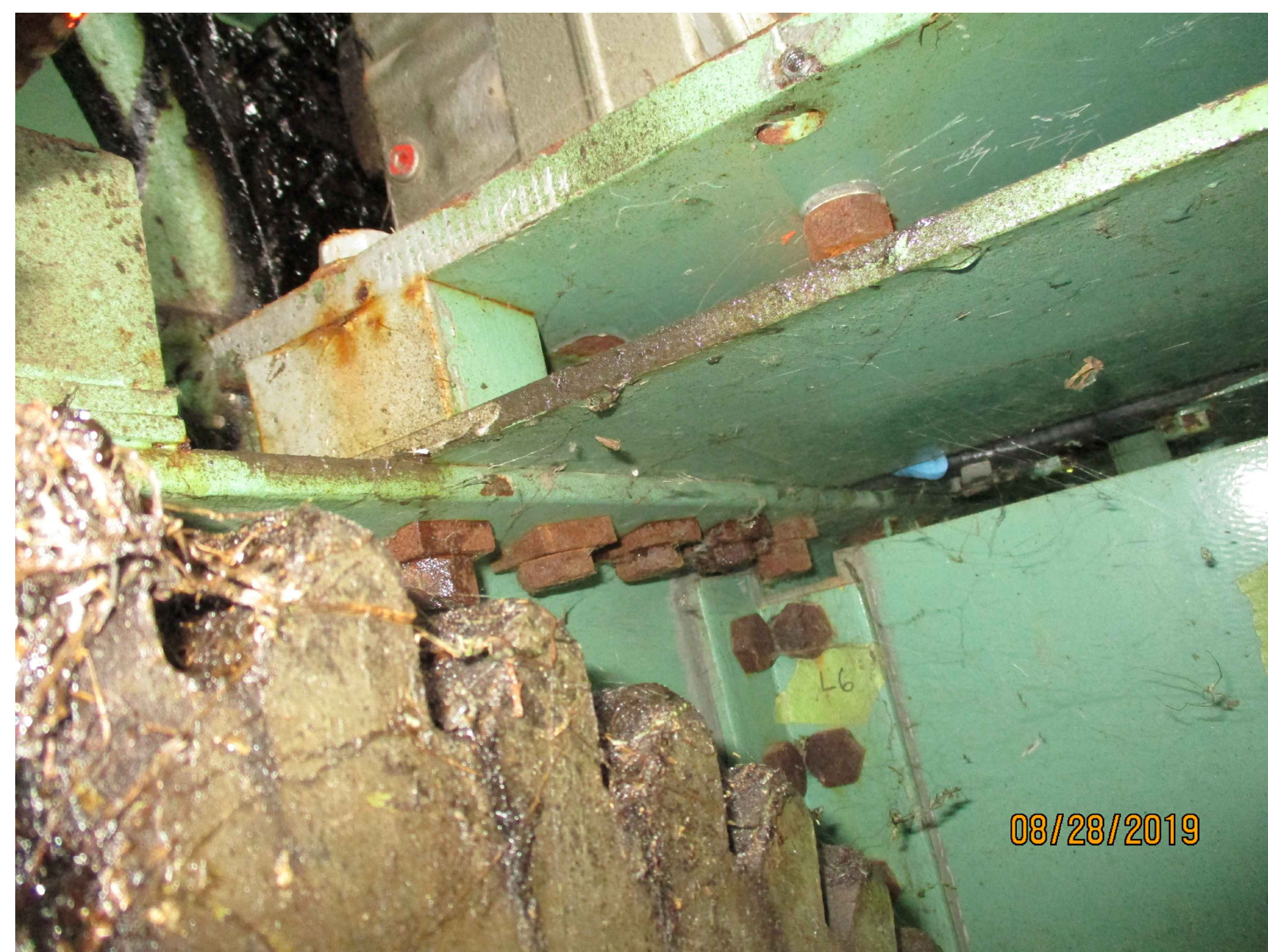
PHOTO OF CORRODED SPAN LOCK MOTOR/REDUCER SUPPORT MOUNTING BOLTS
