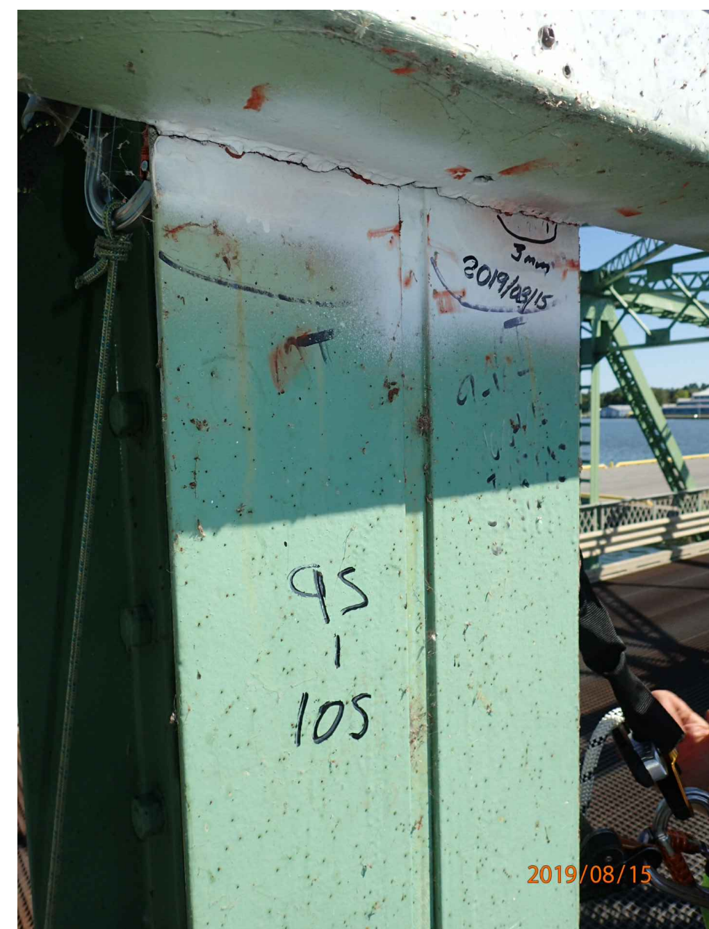
9S-10S VERTICAL - CRACK BEHIND SIGN SUPPORT ANGLE
