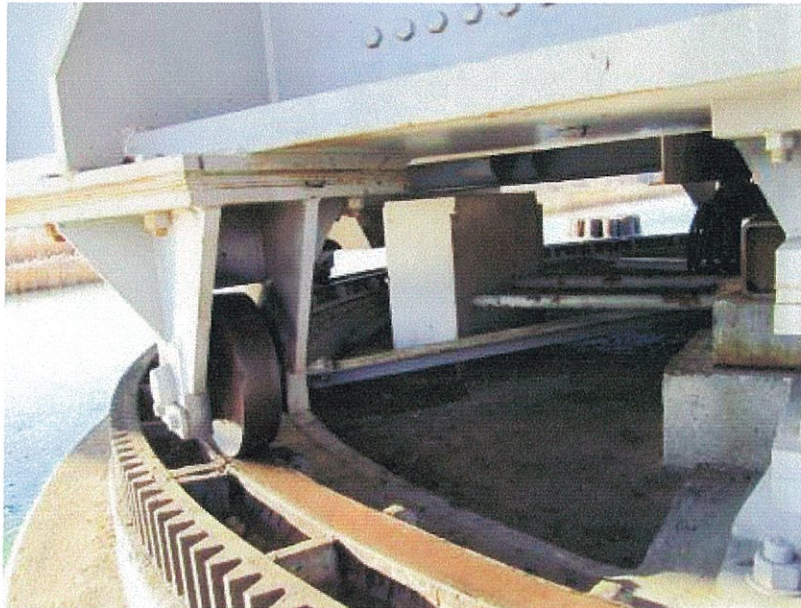
PHOTOGRAPH 13: CENTRE PIER BALANCE WHEELS ON TRACK WITH SPUR GEAR
