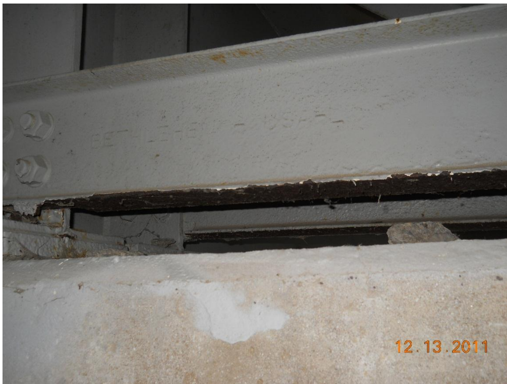
Photograph 92 - Bracing, east shore pier, note coating failure on bottom of bottom flange - typical of most bracing
