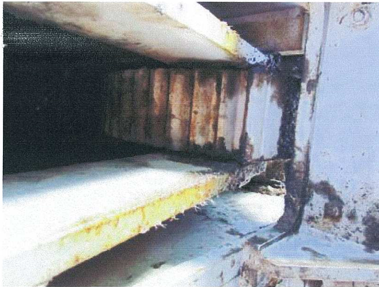
PHOTOGRAPH 7: WEDGE MECHANISM GEAR SECTOR ON THE REST PIER SHOWING LACK OF LUBRICATION AND CORROSION
