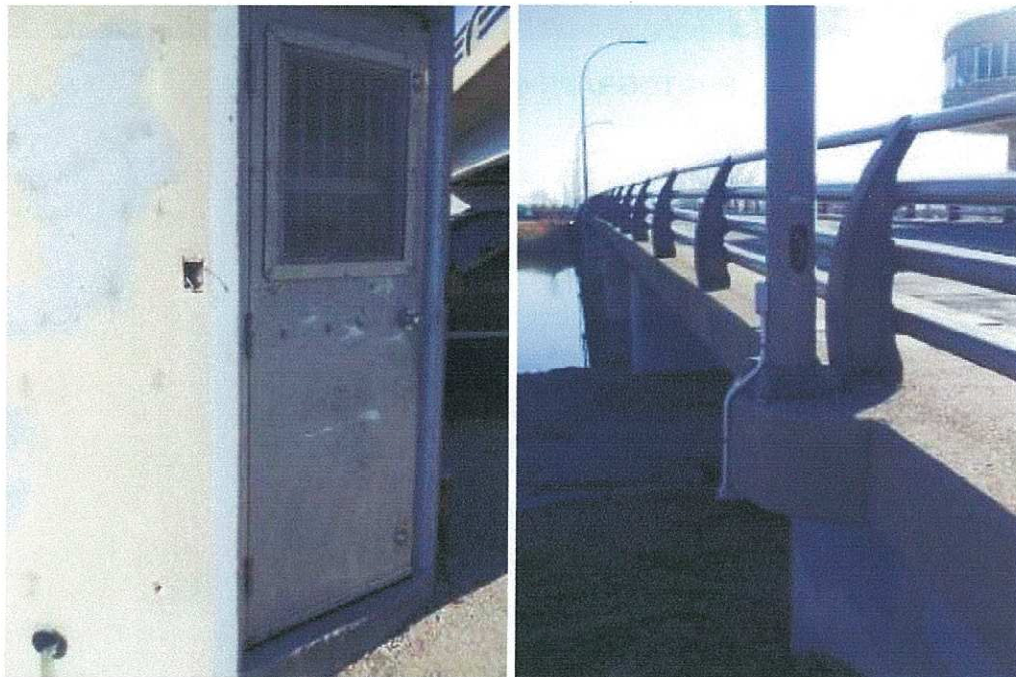
PHOTOGRAPH 42: JUNCTION BOX COVERS
