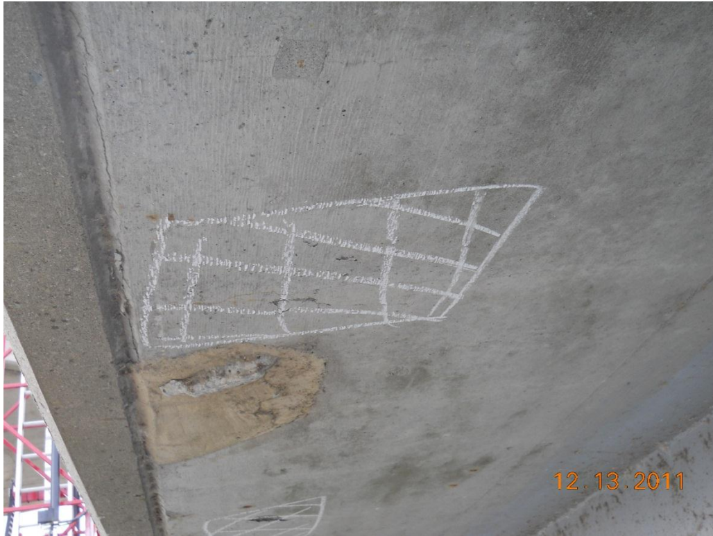
Photograph 87 - Soffit, span 2 south exterior, note delamination and previous patching
