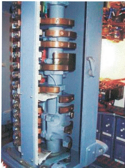
PHOTOGRAPH 41: SPAN ROTATE DRUM CONTROLLER
