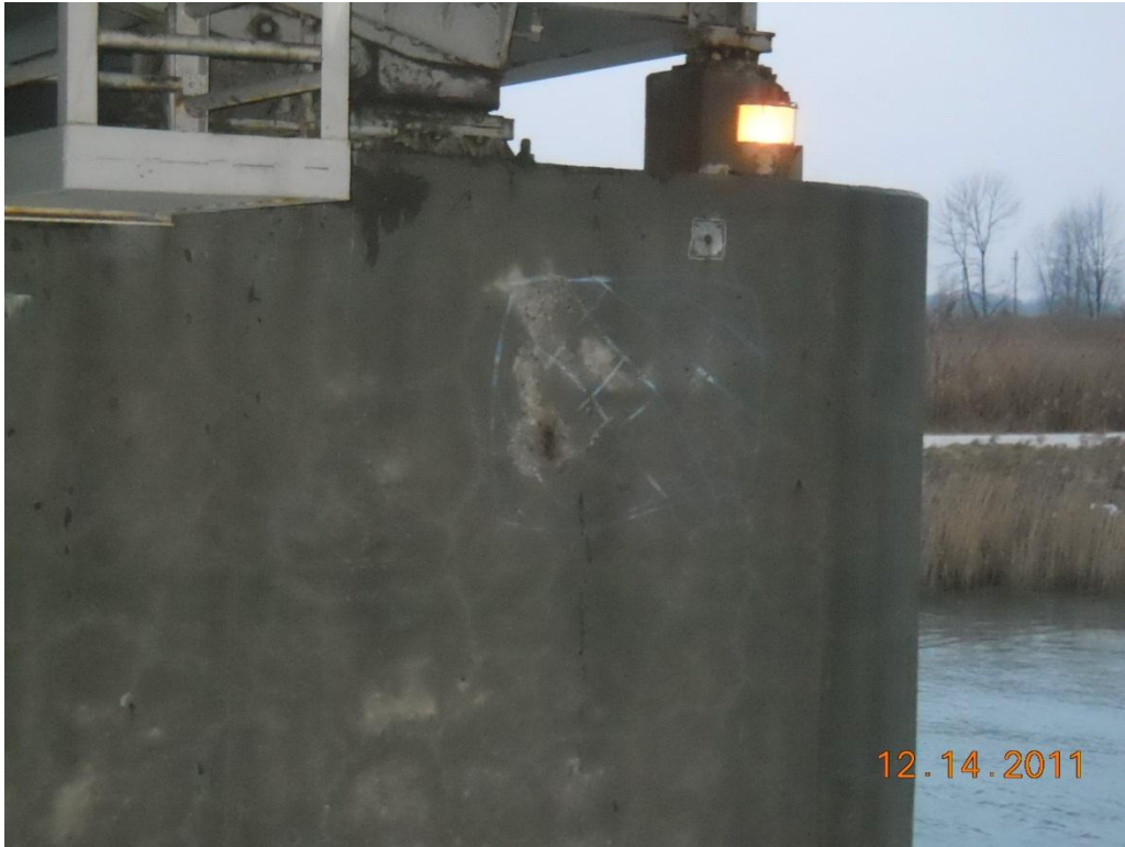
Photograph 63 - North end of east face of west rest pier, note delamination
