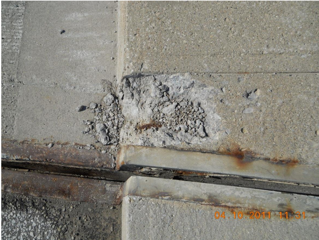
Photograph 25 - Spall on north curb at west rest pier
