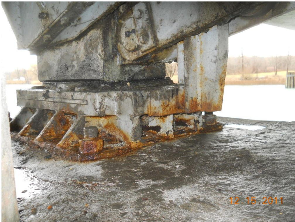
Photograph 76 - Span 4 east rest pier, south bearing, typical to other
