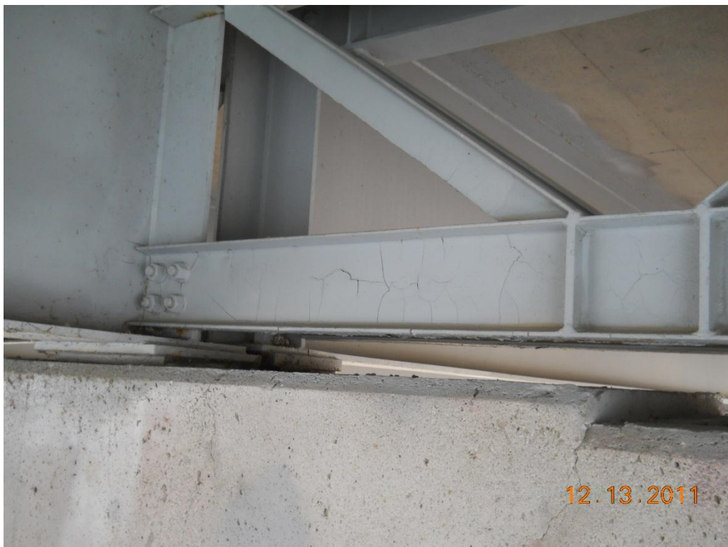
Photograph 120 - Bracing, west shore pier, note coating failure on bottom member
