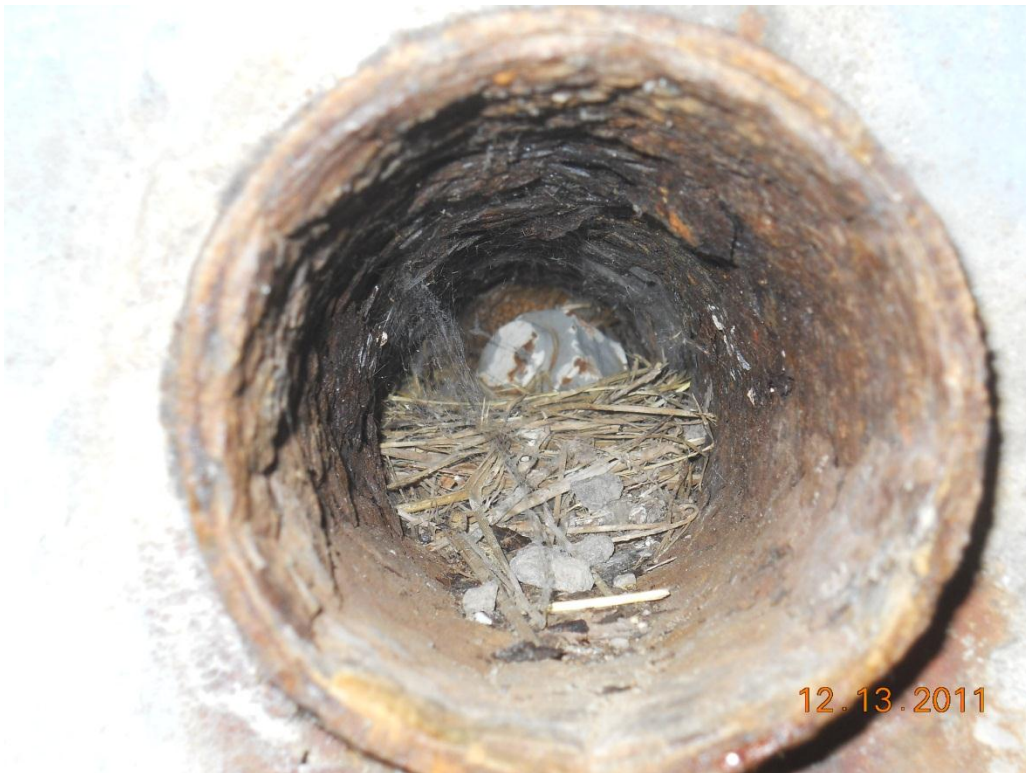
Photograph 44 - Typical west abutment drain, note debris clogging drain
