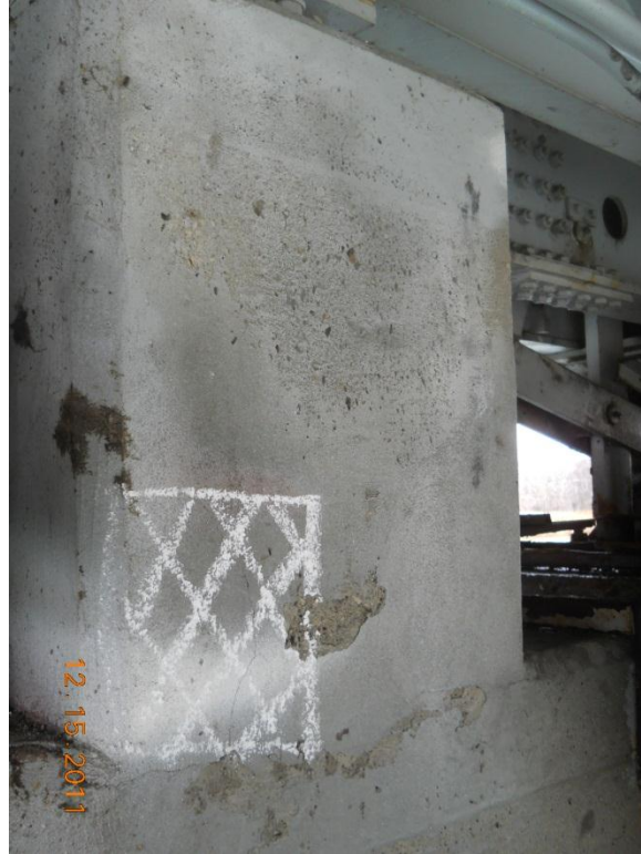
Photograph 59 - Span 5 girder 3 bearing pedestal, note delamination
