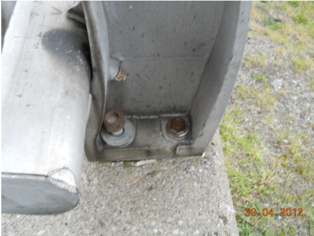
Photograph 141- North railing post, first from east abutment - Note loose bolt at base
