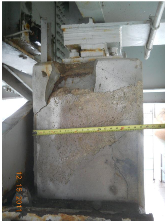
Photograph 68 - West rest pier, third bearing pedestal from north, note spalling
