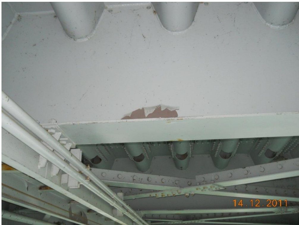
Photograph 116 - Span 3, note coating failure on cross beam web
