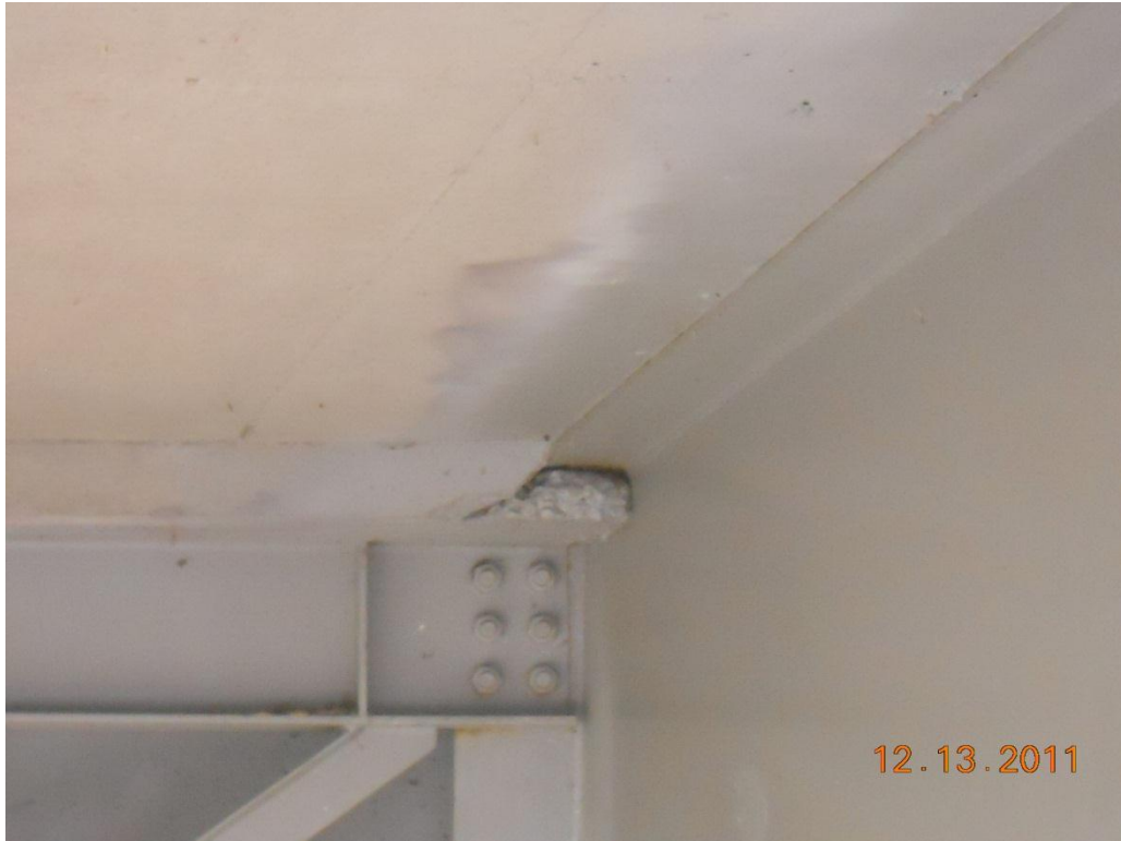
Photograph 89 - Soffit, span 1, note spall near haunch at girder 4
