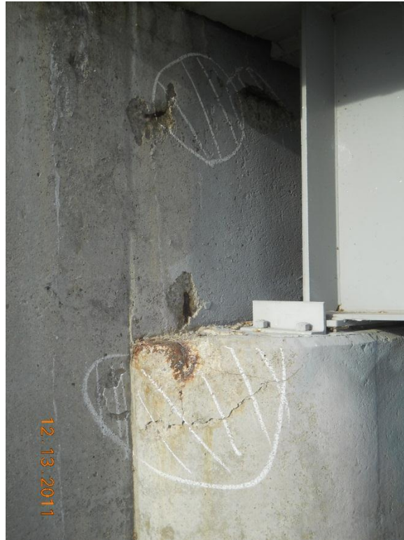
Photograph 49 - South end of west abutment, note spalling and delamination
