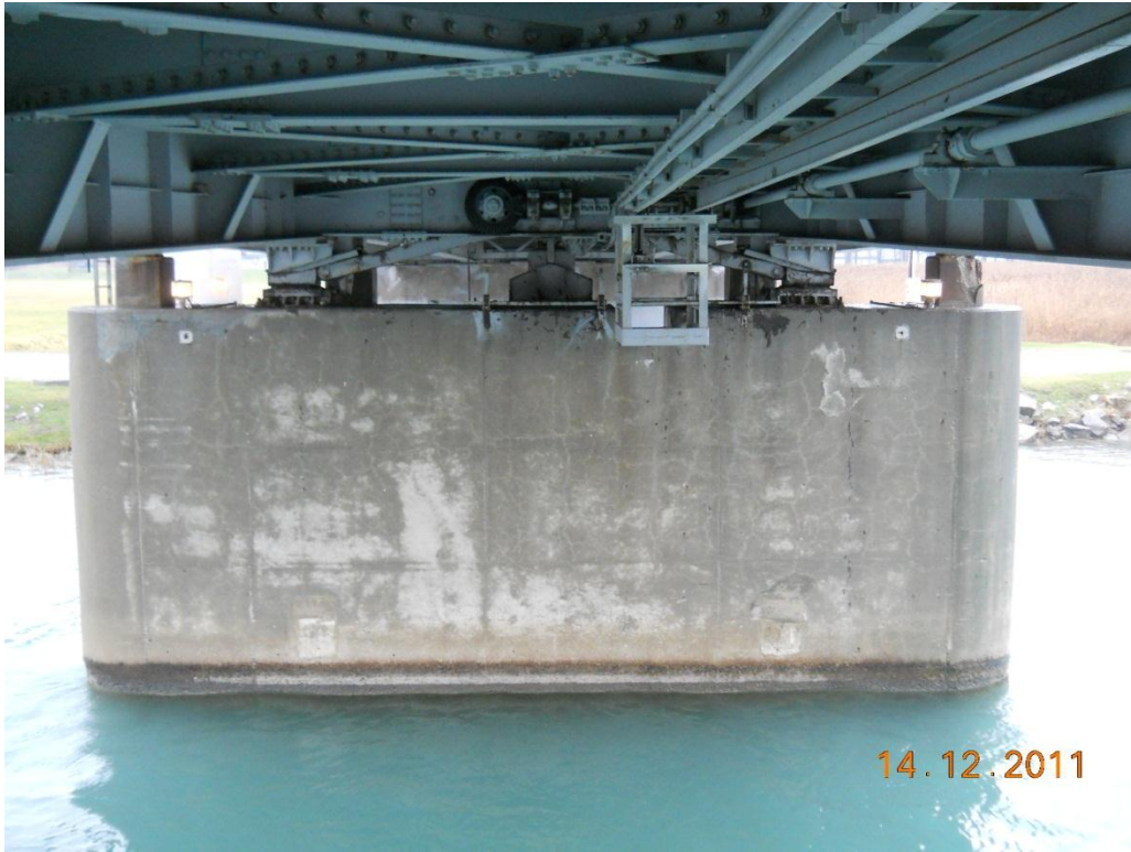
Photograph 61 - East face of west rest pier, note random cracking
