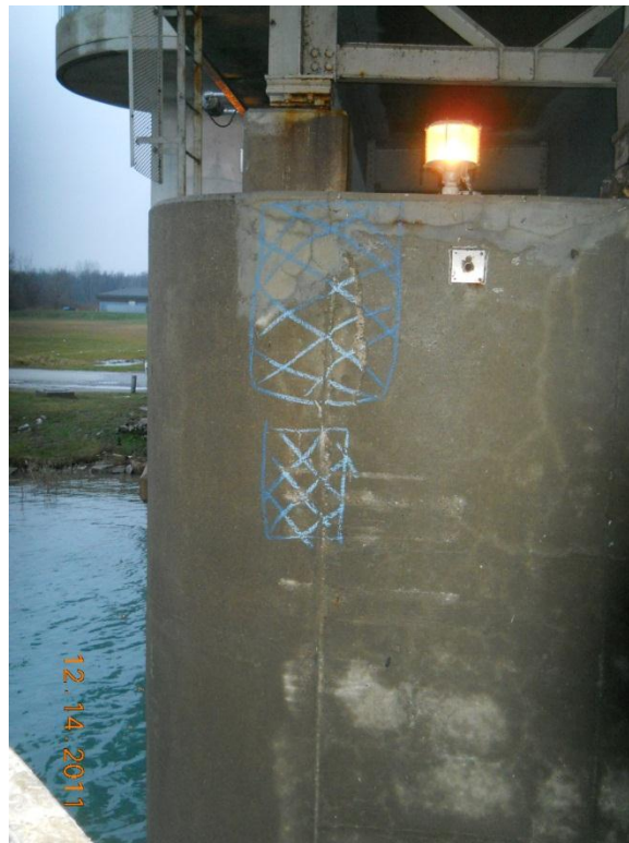
Photograph 64 - South end of east face of west rest pier, note delamination
