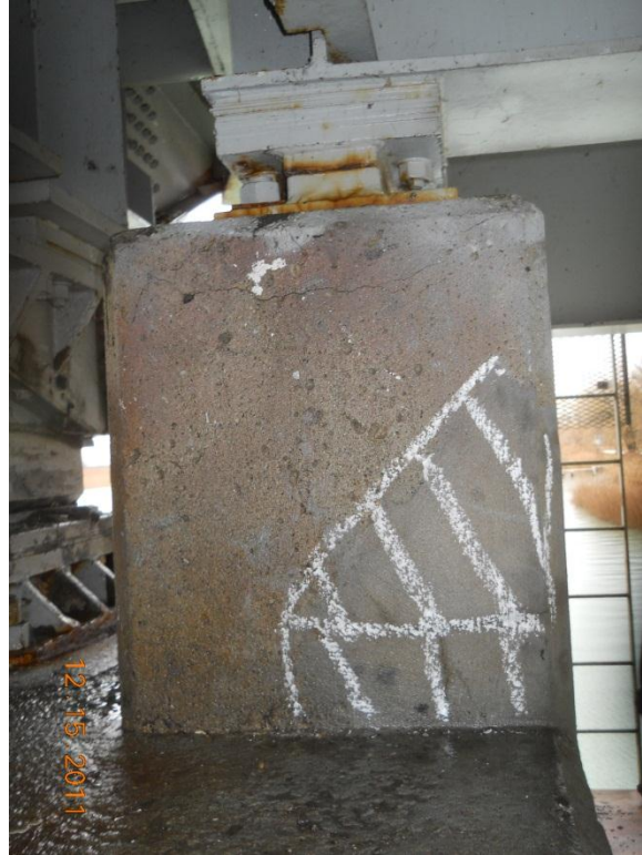
Photograph 69 - West rest pier, fourth bearing pedestal from north, note delamination and cracks
