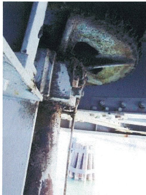
PHOTOGRAPH 30: CENTRE PIER WEST SIDE SWING DRIVE GEAR SHOWING LACK OF LUBRICATION AND CORROSION
