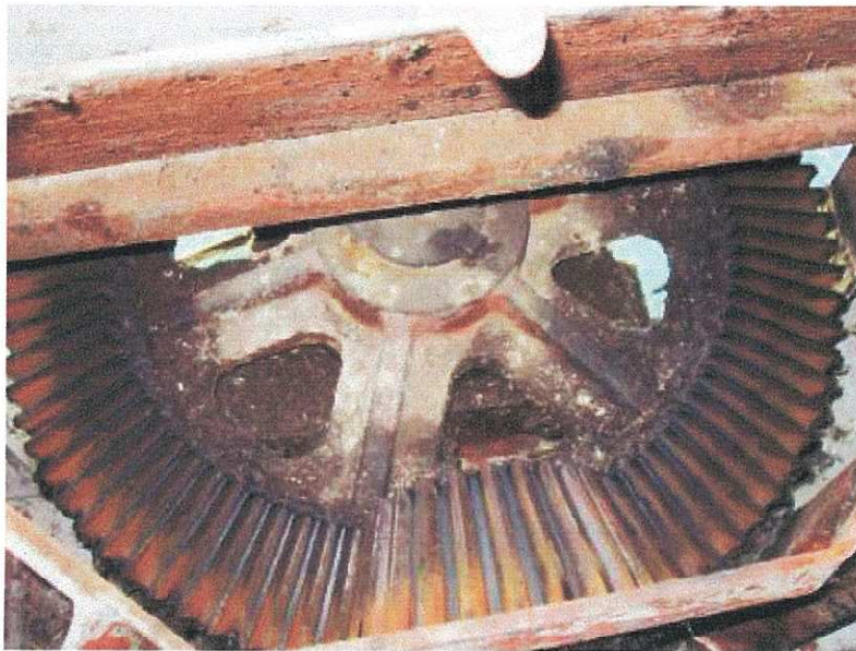
PHOTOGRAPH 28: CENTRE PIER WEST SIDE SWING DRIVE BEVEL GEARS SHOWING LACK OF LUBRICATION AND CORROSION
