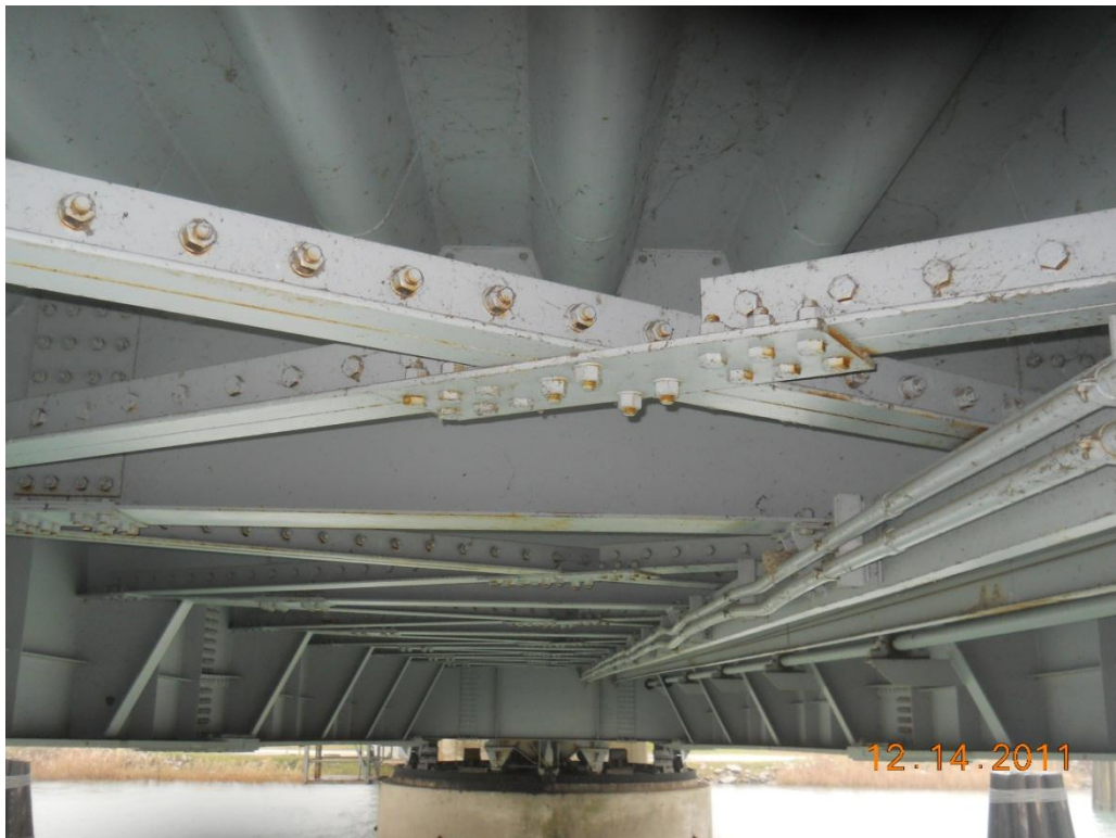
Photograph 106 - Soffit, span 4 looking west
