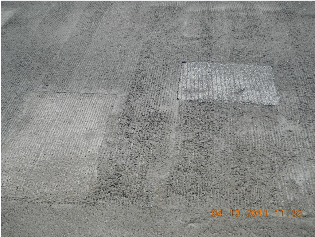
Photograph 23 - Span 1 concrete patches
