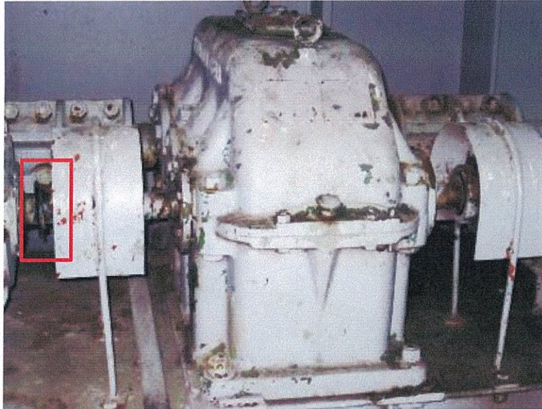
PHOTOGRAPH 25: SEAL PUSHED OUT OF ITS HOUSING AT THE CENTRE PIER WEDGE DRIVE MOTOR
