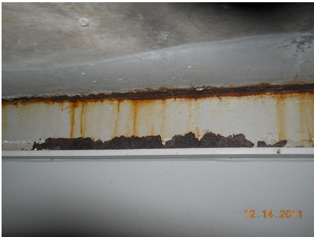
Photograph 104 - Span 4, coating failure and rusting on north side of north exterior longitudinal trough
