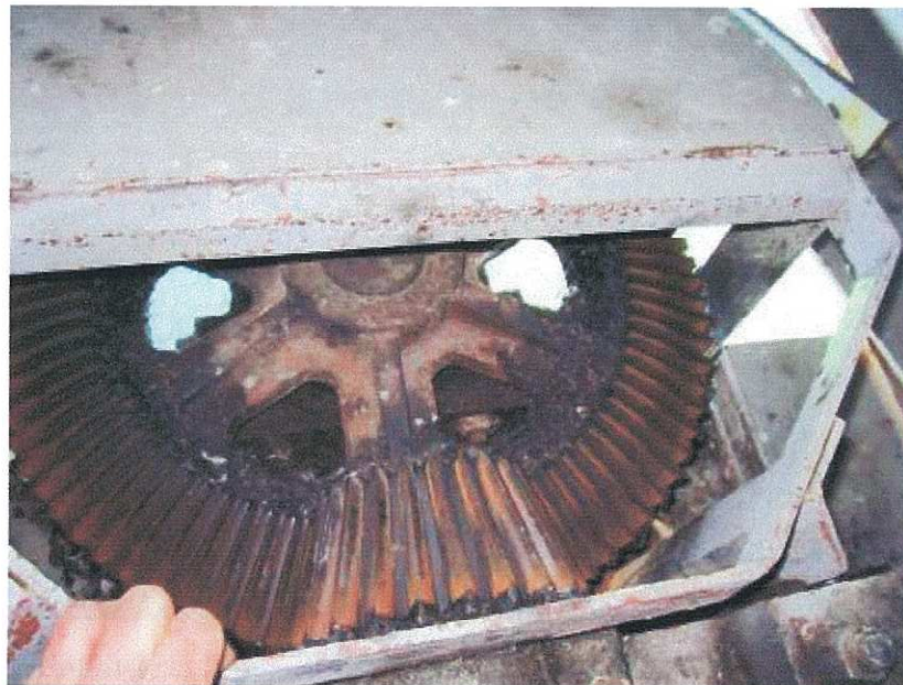
PHOTOGRAPH 20: CENTRE PIER EAST SIDE SWING DRIVE BEVEL GEARS SHOWING LACK OF LUBRICATION AND CORROSION
