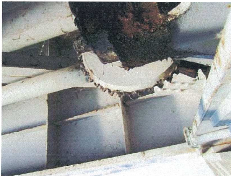
PHOTOGRAPH 8: WEDGE DRIVE SHAFT AND BEVEL GEARS ON THE EAST REST PIER SHOWING LACK OF LUBRICATION AND CORROSION
