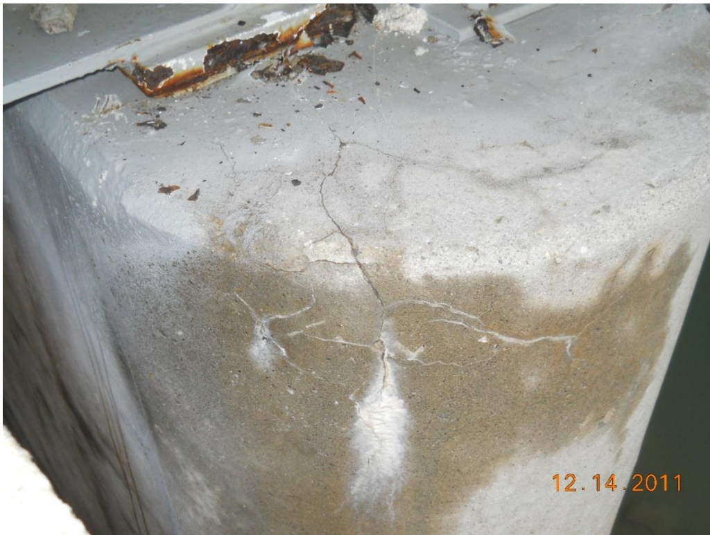
Photograph 52 - North end of bearing seat of east shore pier, note cracking and efflorescence
