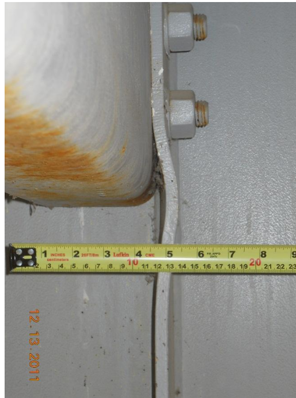
Photograph 127 - Span 1, diaphragm 2 connection to girder 5, note deformation of stiffener
