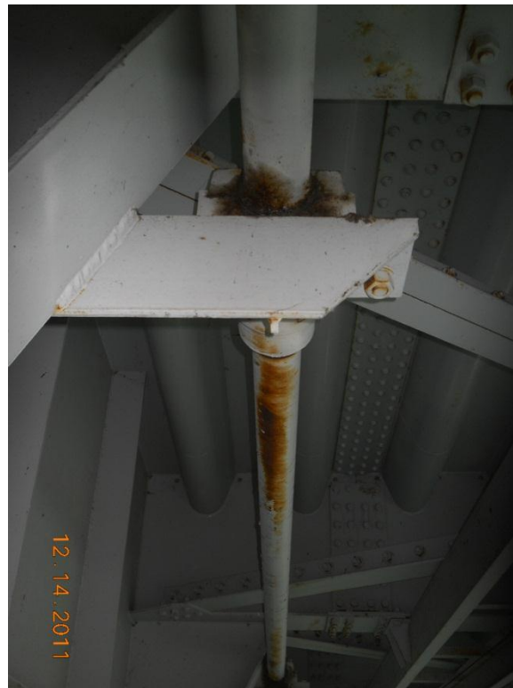
Photograph 110 - Span 3, note rusting on bottom of rest pier wedge driveshaft
