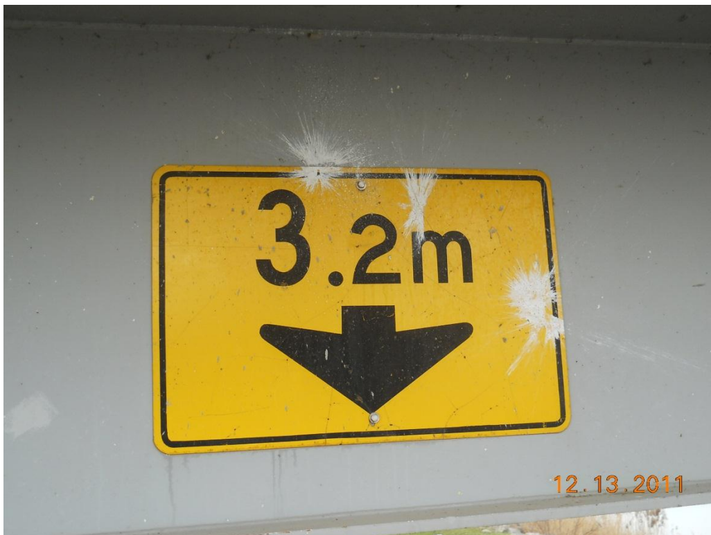
Photograph 132 - Low clearance sign, south side of span 1, north side similar
