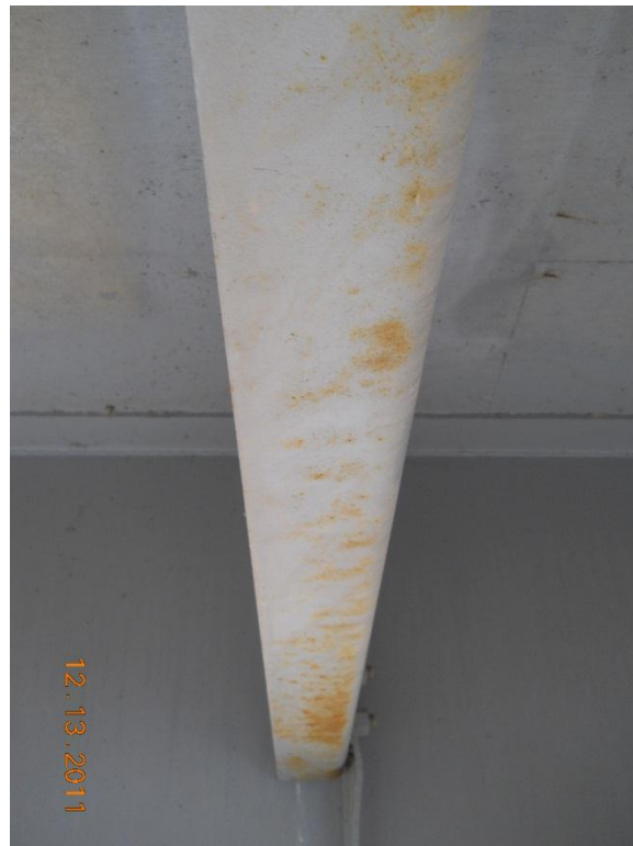
Photograph 128 - Span 1, diaphragm 2, note rusting on bottom of member
