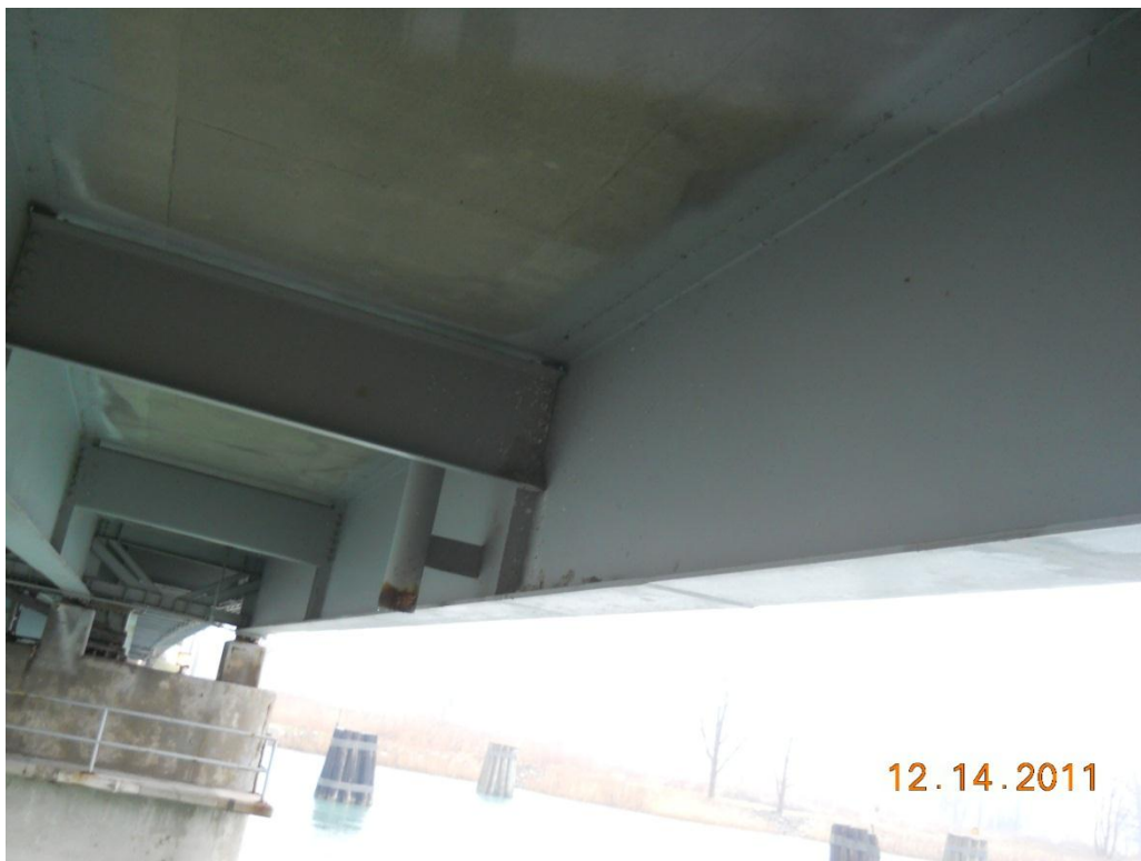
Photograph 94 - Soffit and girder 1, span 5 looking west, note coating failure on bottom of web
