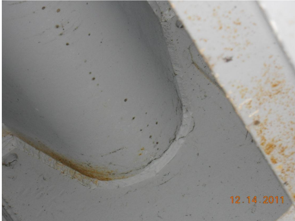
Photograph 99 - Longitudinal trough, span 4, third trough south of girder 1 east of transverse splice, note potential crack near weld
