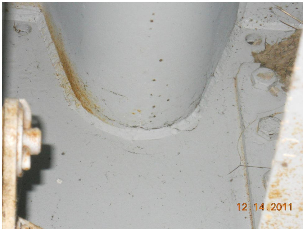
Photograph 98 - Longitudinal trough, span 4, third trough south of girder 1 east of transverse splice, note potential crack near weld
