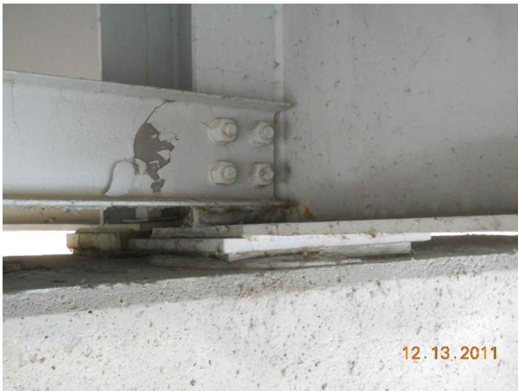
Photograph 80 - Span 2 west shore pier bearing second from north end, note coating failure on bracing, typical to others
