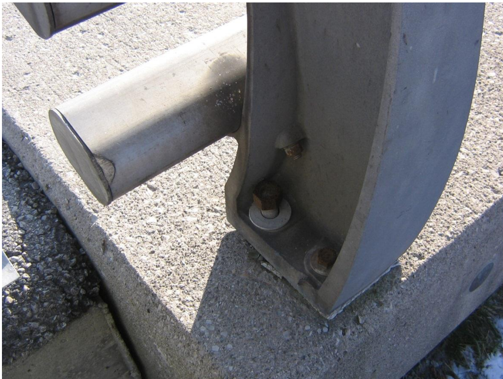
Photograph 30 - Note loose bolt on railing post at northeast corner
