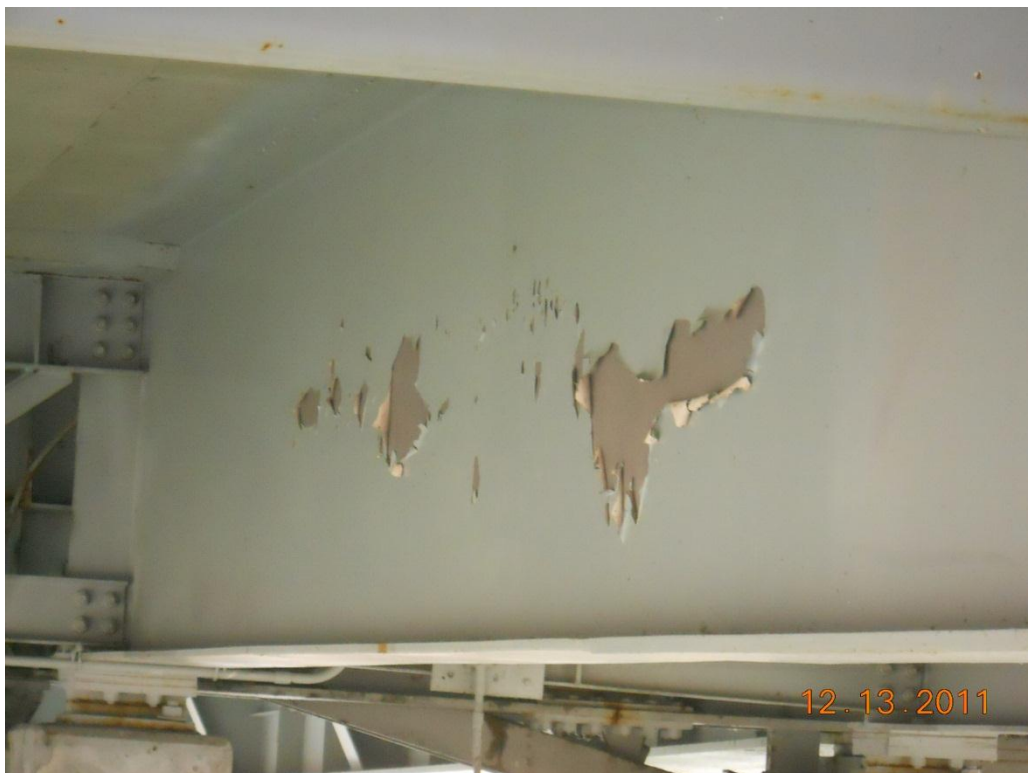
Photograph 118 - Span 2, girder 3, note coating failure on web
