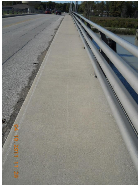
Photograph 24 - North sidewalk looking west, typical condition
