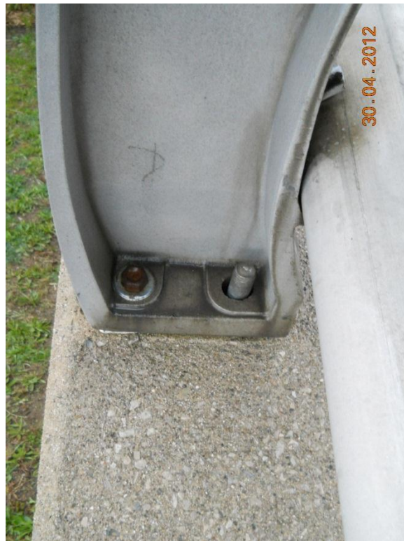
Photograph 140 – South railing post, second from east abutment - Note missing bolt at base.
