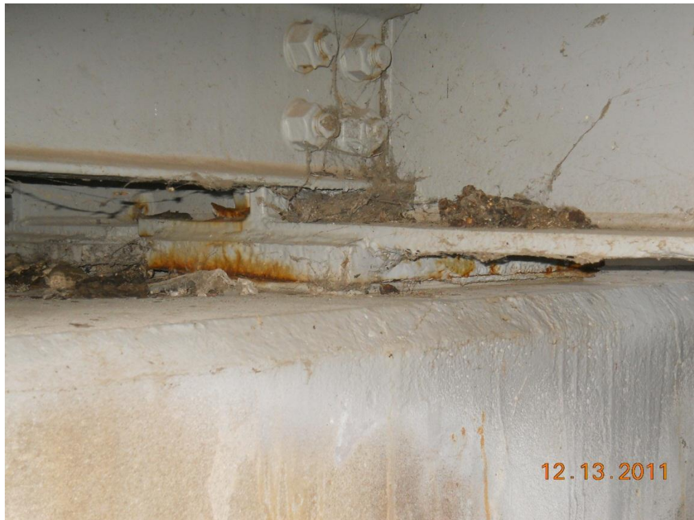
Photograph 74 - Span 6 east shore pier bearings, first from north end, typical to others
