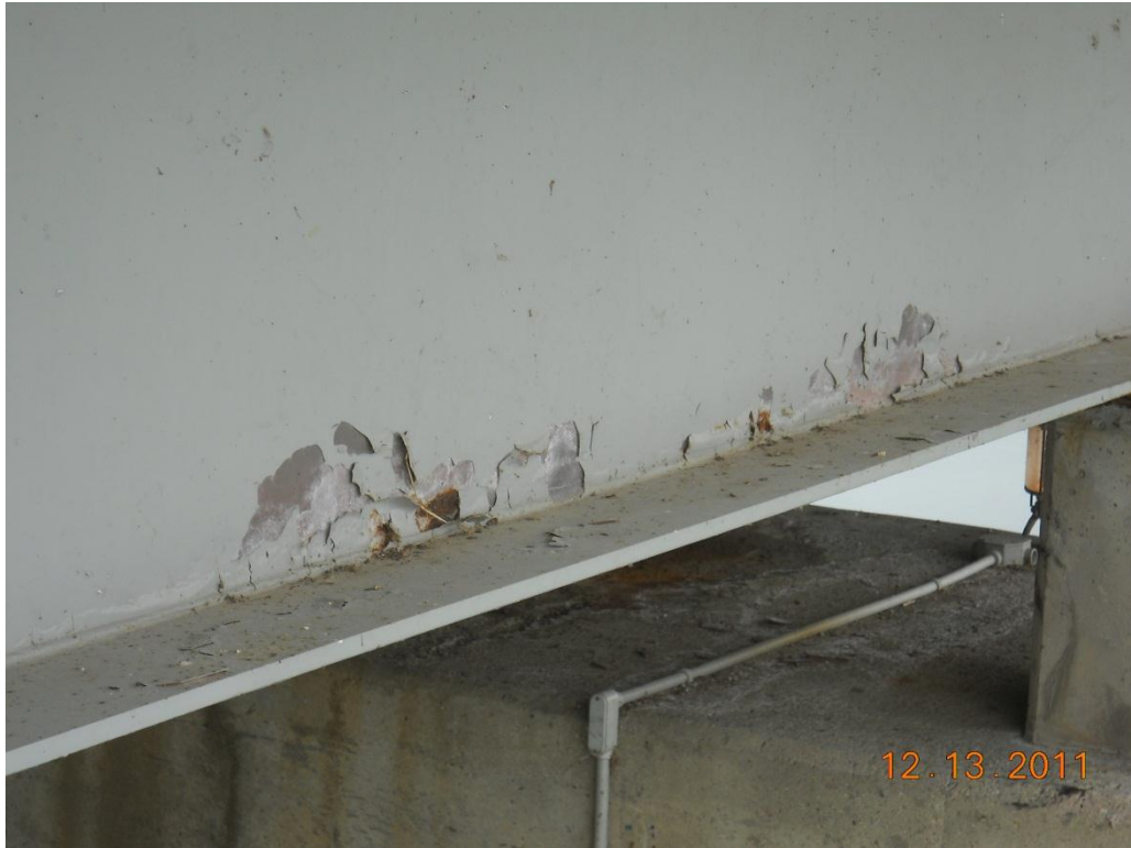
Photograph 129 - Span 1, girder 5 exterior, note coating failure
