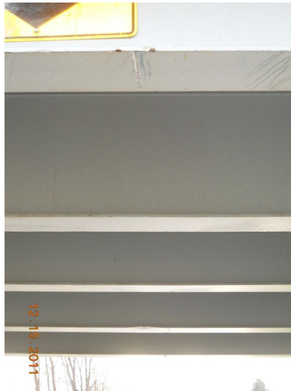
Photograph 122 - Span 1 girders looking south, note impact damage
