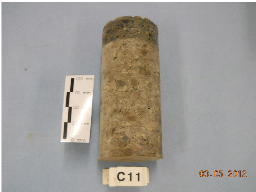
Core C11 - Note air voids noted
