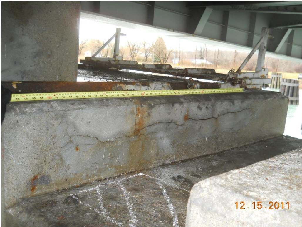
Photograph 58 - Top of east rest pier, note crack
