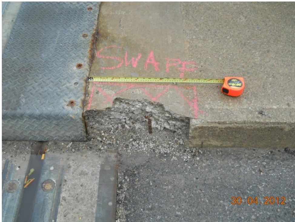
Photograph 144 - South sidewalk, east end of span 1 - Note spall with exposed corroded reinforcing steel bar.
