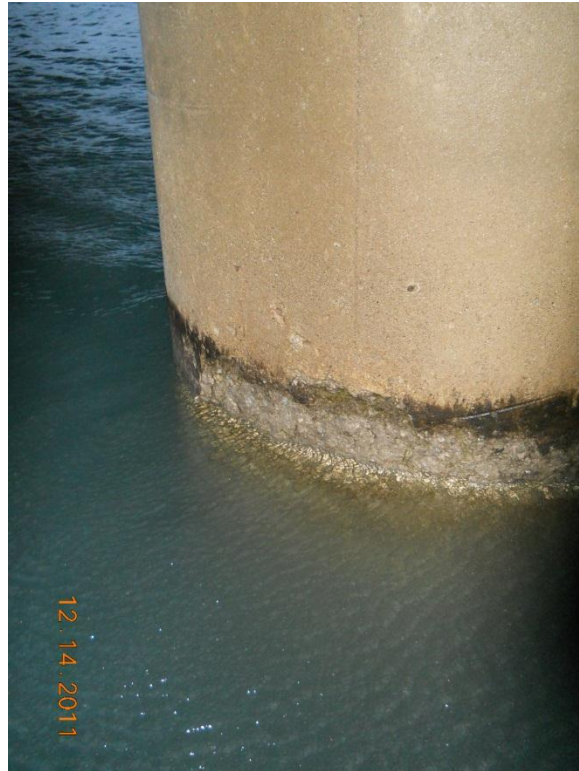
Photograph 65 - South face of west rest pier, note concrete erosion at waterline
