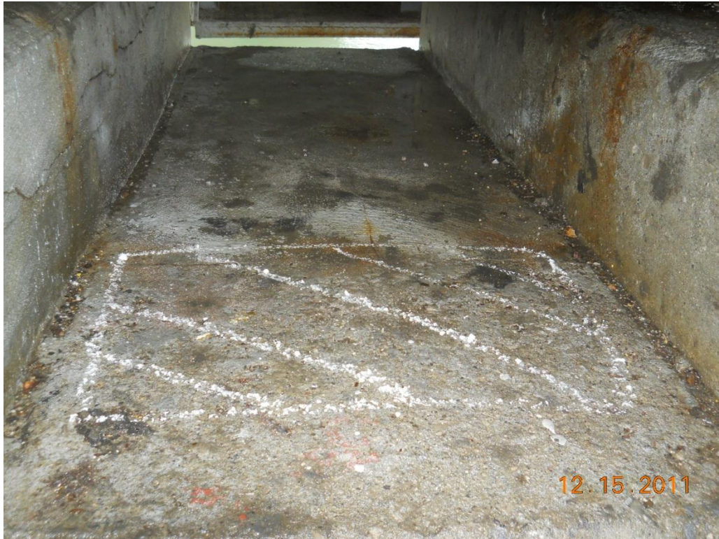
Photograph 57 - Top of east rest pier, note delamination
