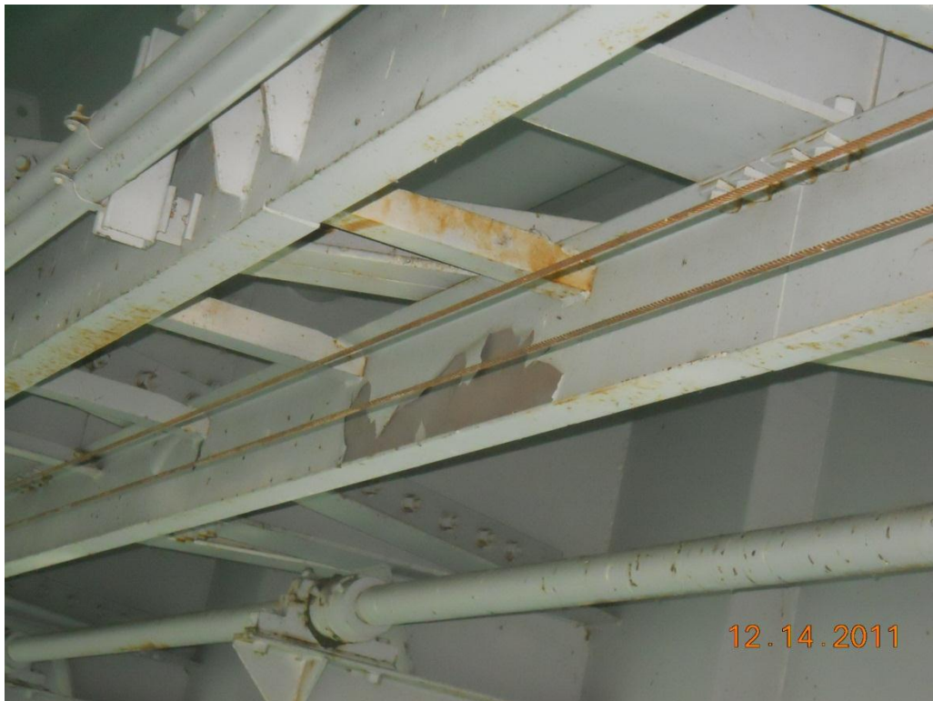
Photograph 108 - Span 3, note coating failure on machinery beam
