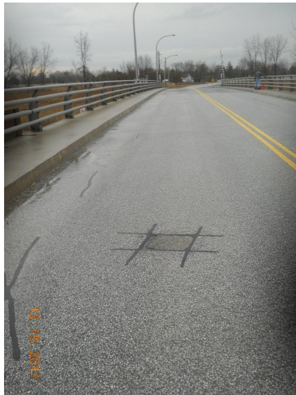
Photograph 16 - Span 4 asphalt wearing surface looking east, westbound lane, note patch
