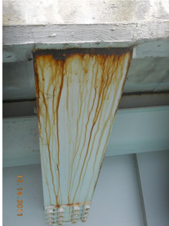
Photograph 103 - Span 4, exterior end of cross beam, typical condition
