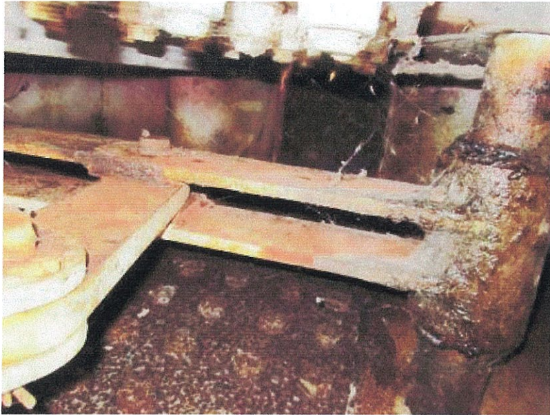
PHOTOGRAPH 9: WEDGE MECHANISM ON THE EAST REST PIER, NORTH SIDE SHOWING LACK OF LUBRICATION AND CORROSION
