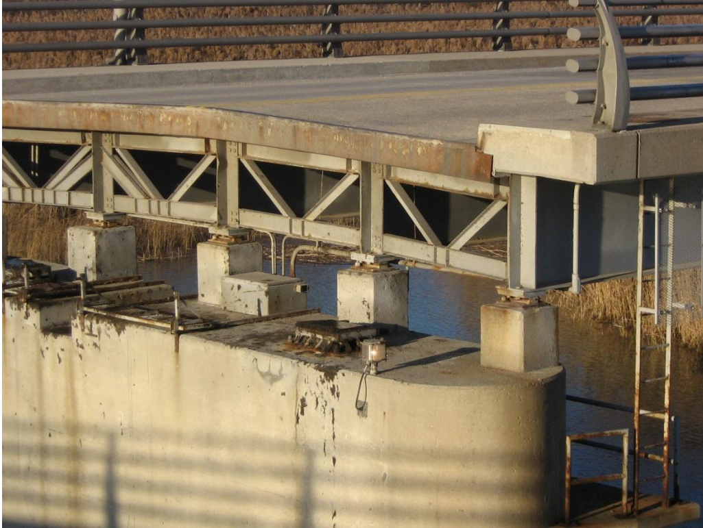
Photograph 55 - Top of east rest pier looking north with swing span in open position
