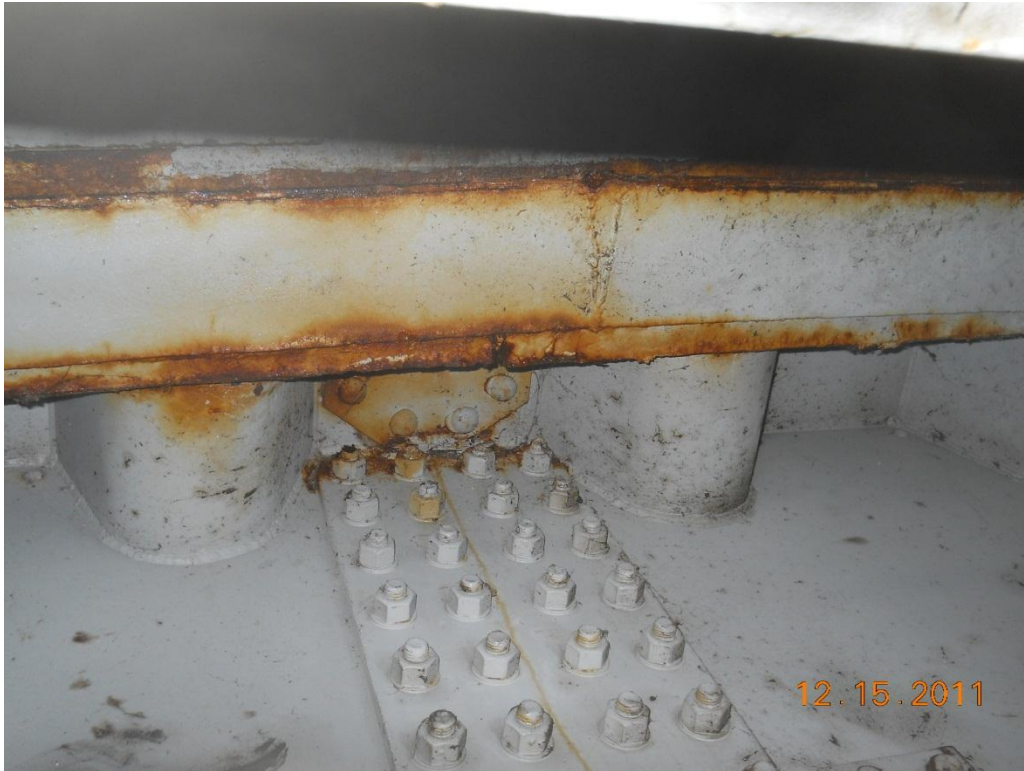
Photograph 35 - East rest pier underside of joint looking up from centre, note corrosion
