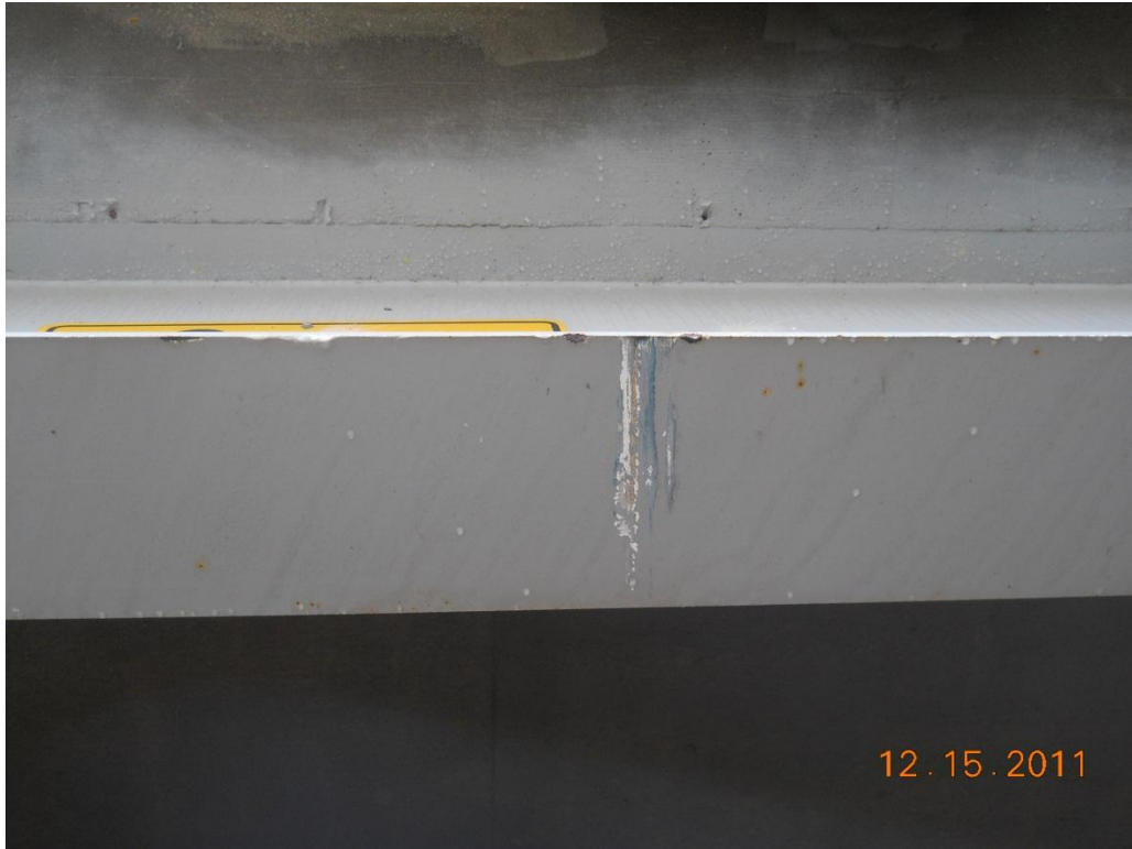
Photograph 123 - Span 1, girder 1, note impact damage
