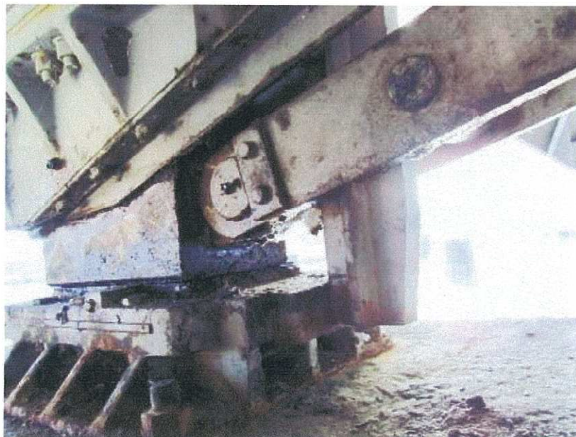
PHOTOGRAPH 12: SPAN WEDGE WITH CORRODED BASE PLATE ON THE NORTH SIDE OF THE EAST REST PIER
