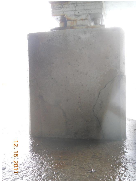
Photograph 70 - West rest pier, fifth bearing pedestal from north, note delamination and cracks
