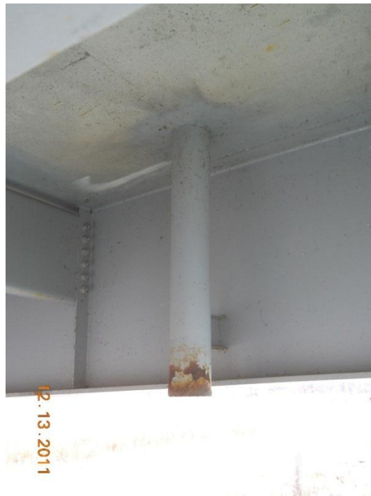
Photograph 130 - Deck drain, typical for spans 1, 2, 5, 6, note corrosion at bottom. Deck drain does not extend far enough beyond girder bottom flange.
