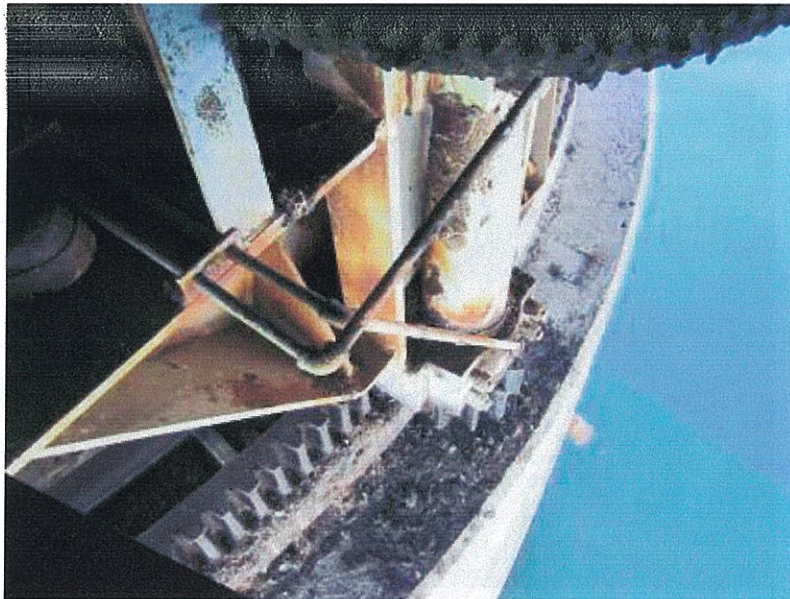
PHOTOGRAPH 21: CENTRE PIER EAST SIDE SWING DRIVE GEAR SHOWING LACK OF LUBRICATION AND CORROSION
