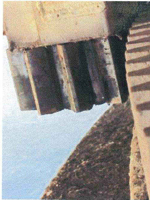
PHOTOGRAPH 31: CENTRE PIER EAST SIDE SWING DRIVE FINAL GEAR AND CIRCULAR RACK SHOWING LACK OF LUBRICATION AND CORROSION
