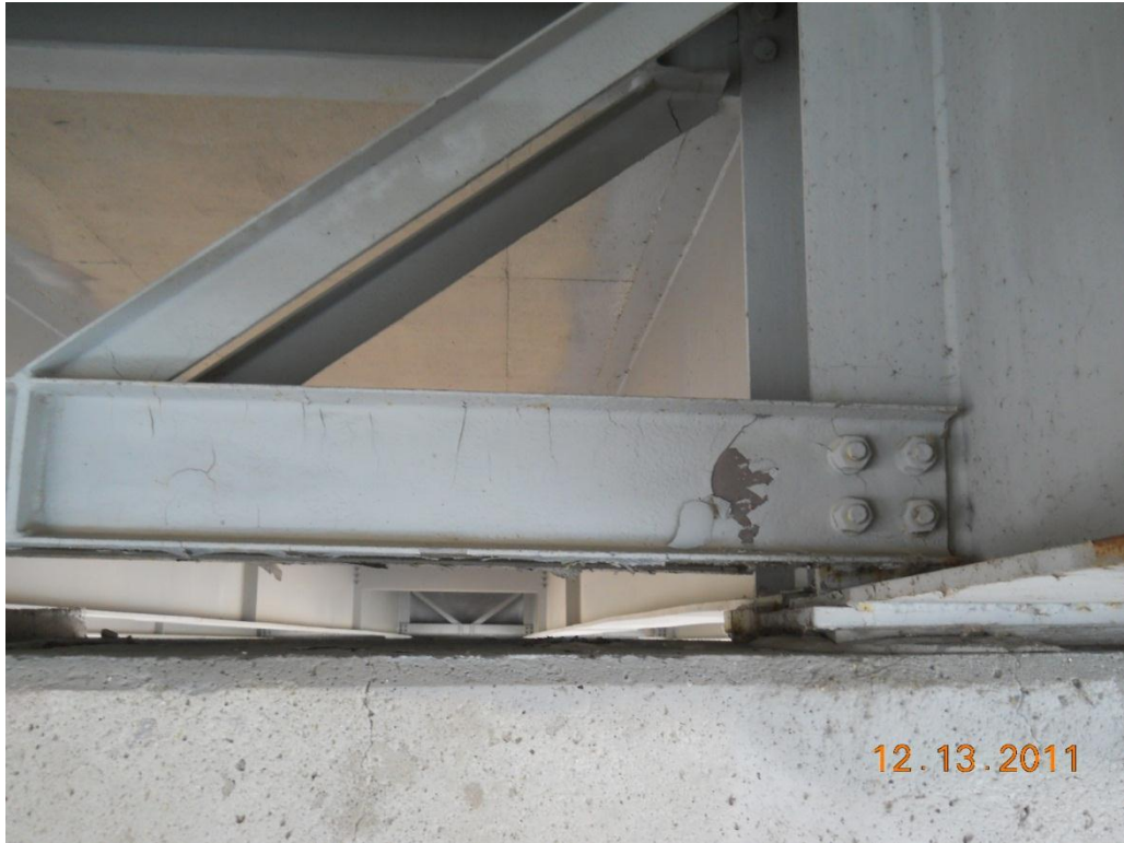
Photograph 119 - Bracing, west shore pier, note coating failure on bottom member
