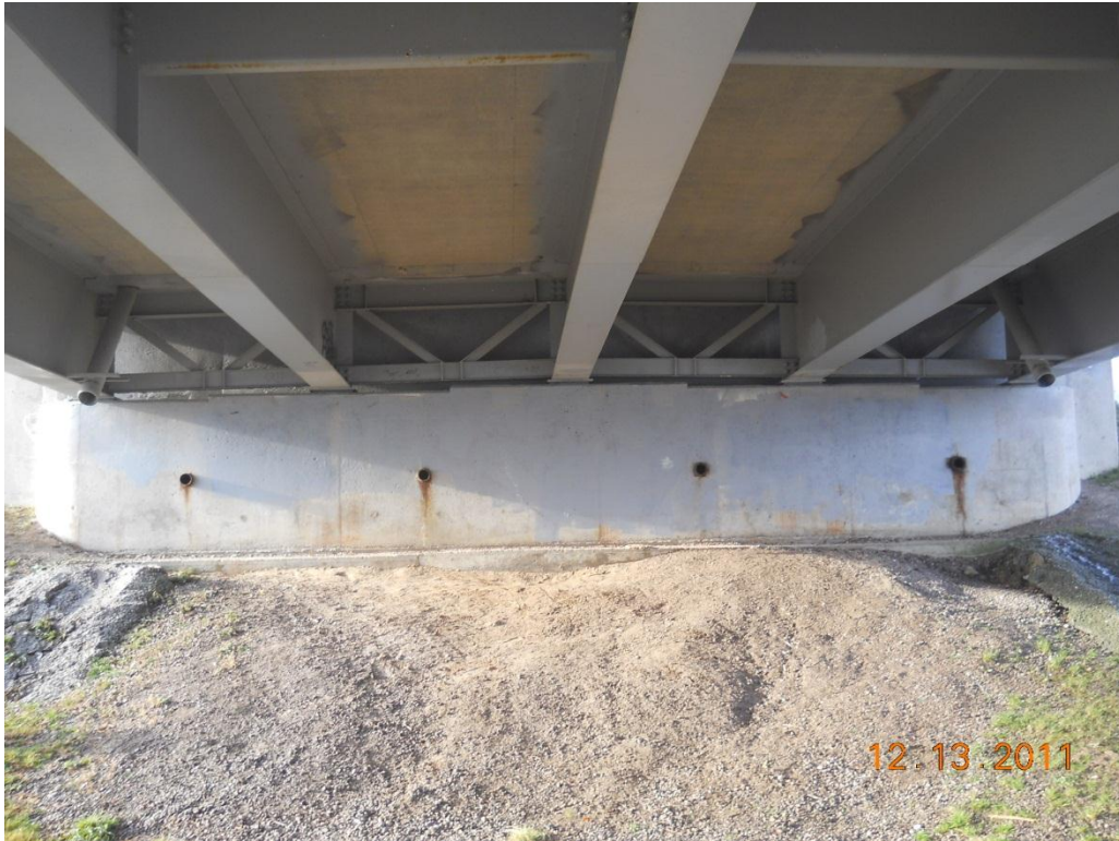
Photograph 43 - West abutment, note gullies and exposed concrete footing
