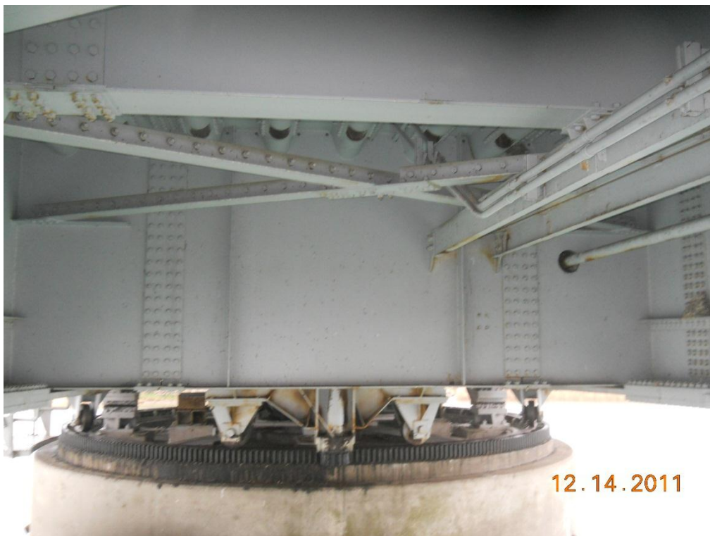
Photograph 96 - Diaphragm, span 4 near pivot pier, note localized areas of rusting
