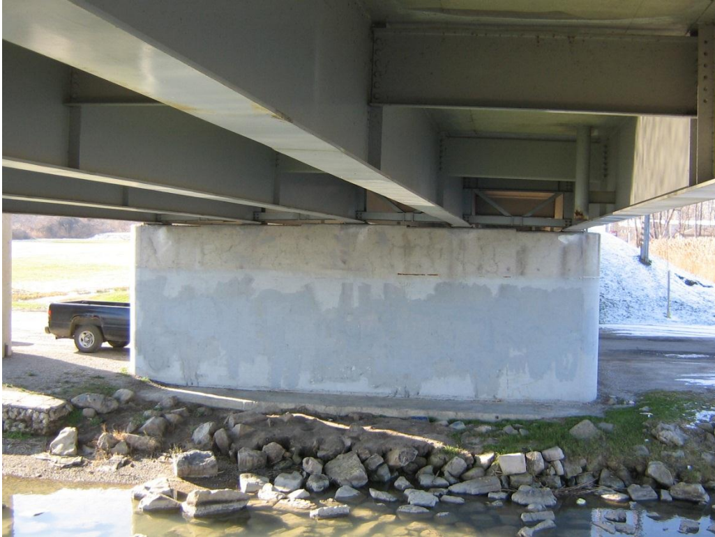
Photograph 71 - East face of west shore pier, note exposed footing
