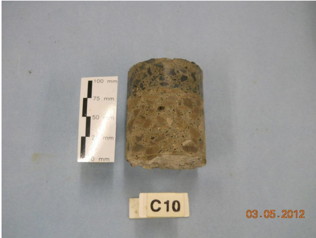
Core C10 - Note air voids noted
