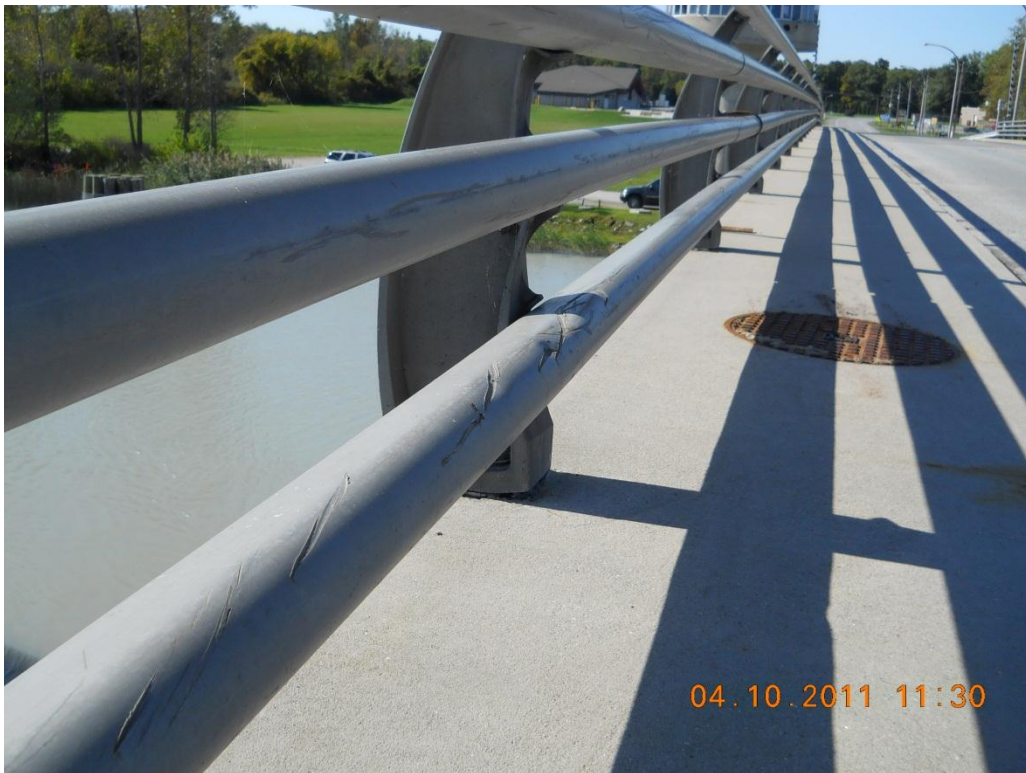
Photograph 28 - South railing, note impact damage above west rest pier
