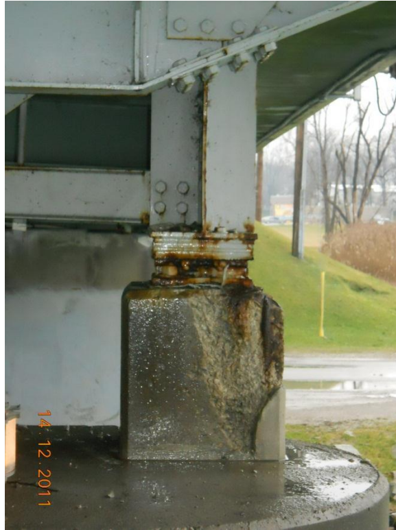
Photograph 67 - West rest pier, span 2 girder 1 bearing pedestal, note spalling and delamination
