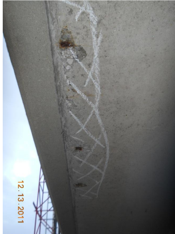
Photograph 83 - Soffit, span 6 south exterior, note delamination and exposed reinforcement
