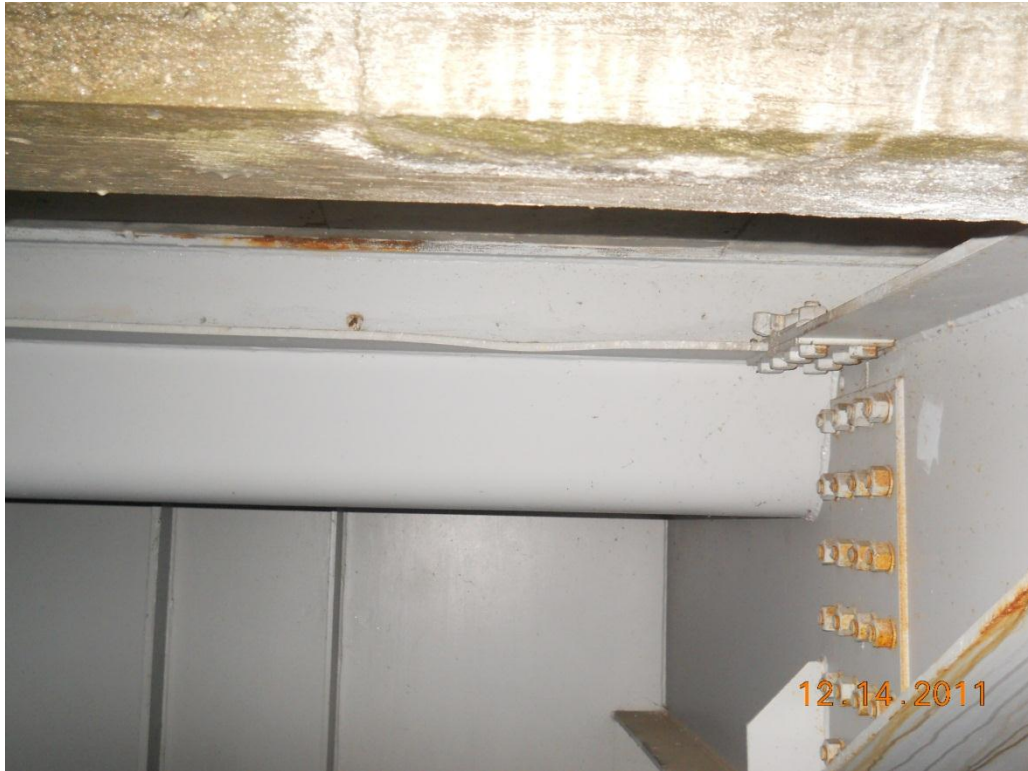
Photograph 117 - Span 3, note deformation in south exterior deck plate
