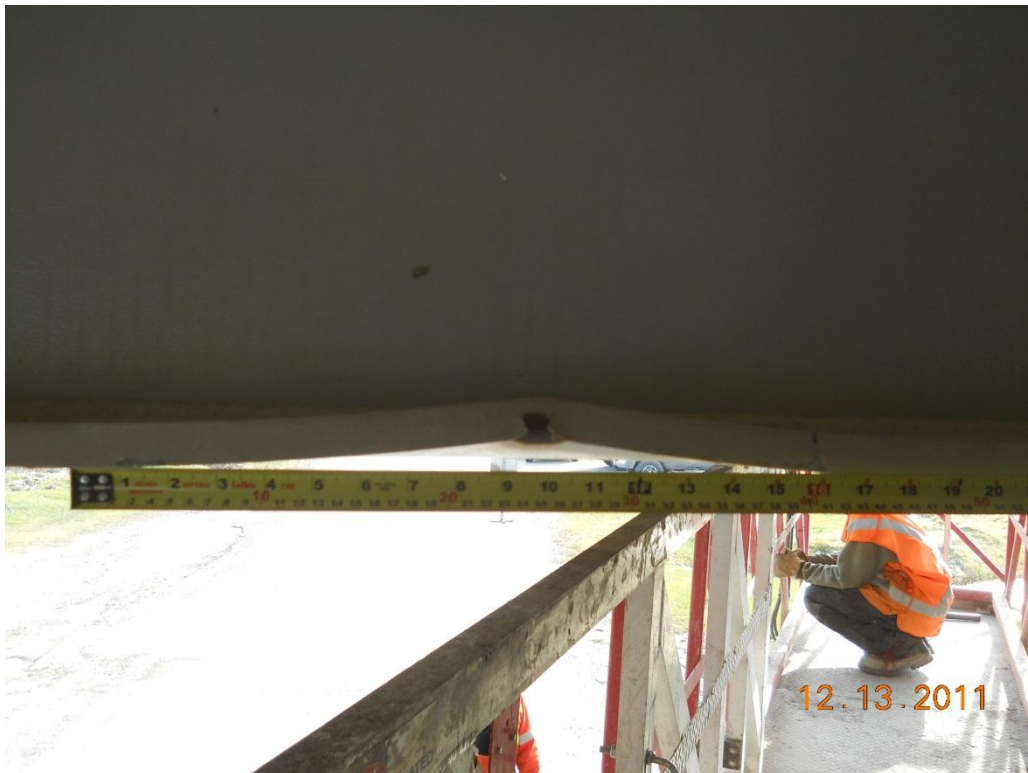
Photograph 124 - Span 1, girder 4, note impact damage
