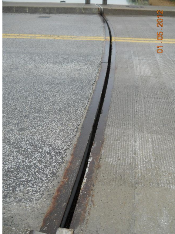
Photograph 149 - Joint over west rest pier looking south - Note corrosion of armoring angles.
