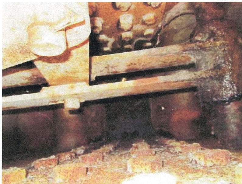
PHOTOGRAPH 6: WEDGE MECHANISM ON THE EAST REST PIER, SOUTH SIDE SHOWING LACK OF LUBRICATION AND CORROSION
