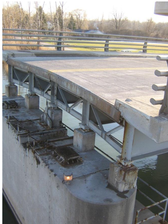
Photograph 62 - Top of west rest pier looking south with swing span in open position
