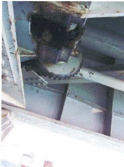
PHOTOGRAPH 4: WEDGE DRIVE SHAFT AND BEVEL GEARS ON THE WEST REST PIER SHOWING LACK OF LUBRICATION AND CORROSION
