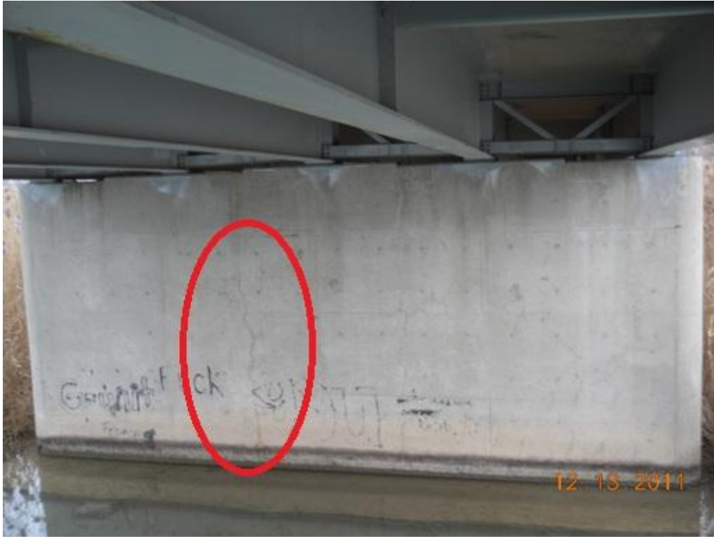
Photograph 51 - West face of east shore pier, note vertical crack near centre
