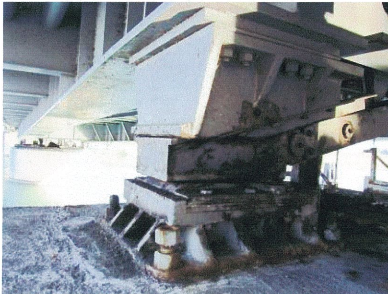
PHOTOGRAPH 2: SPAN WEDGE WITH CORRODED BASE PLATE ON THE NORTH SIDE OF THE WEST REST PIER
