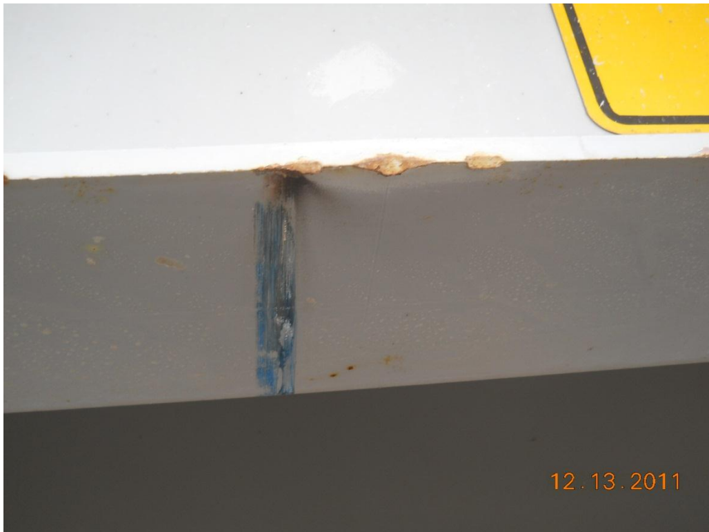
Photograph 126 - Span 1, girder 5, note impact damage
