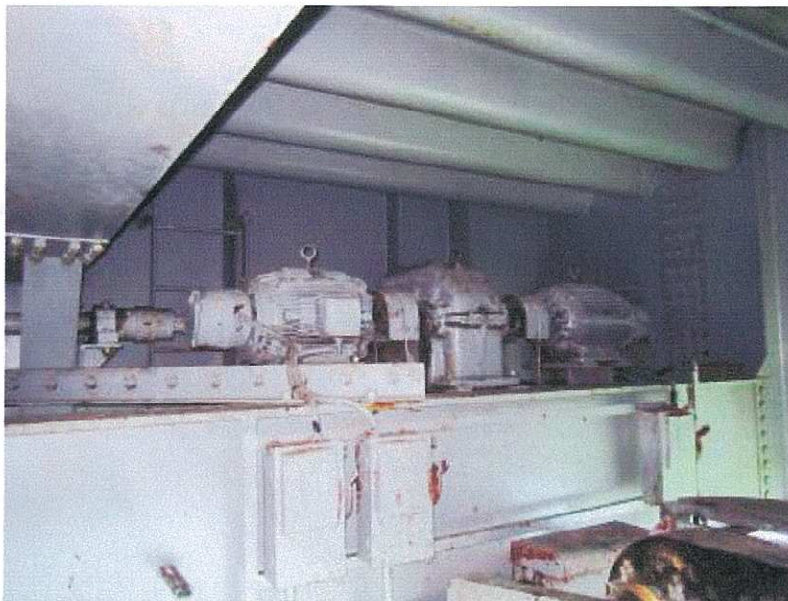
PHOTOGRAPH 24: CENTRE PIER WEDGES DRIVE MOTORS AND REDUCER
