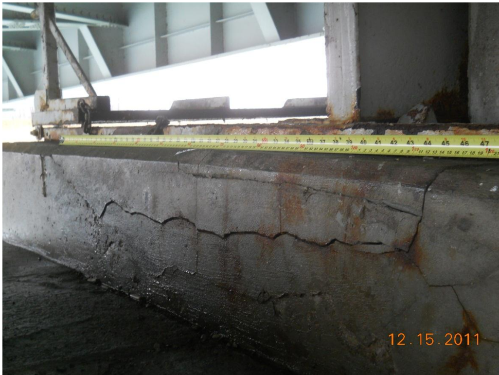
Photograph 66 - Top of west rest pier, note cracking and delamination
