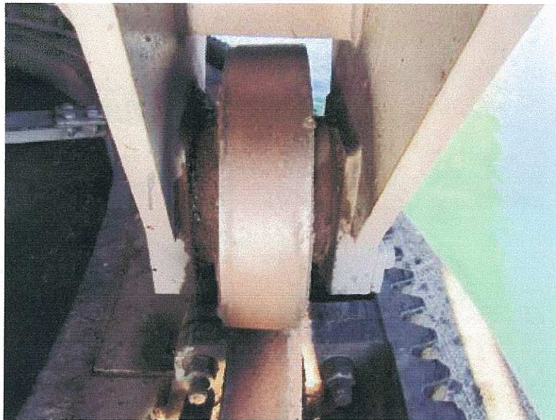
PHOTOGRAPH 15: CENTRE PIER BALANCE WHEELS ON TRACK WITH SPUR GEAR SHOWING LACK OF LUBRICATION
