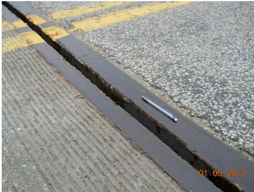
Photograph 147 - Joint over east rest pier - Note abrasion damage to armouring angles.
