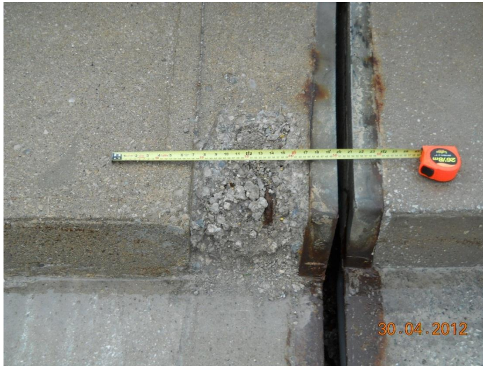
Photograph 143 - North sidewalk, east end of span 2 - Note spall with exposed corroded reinforcing steel bar.
