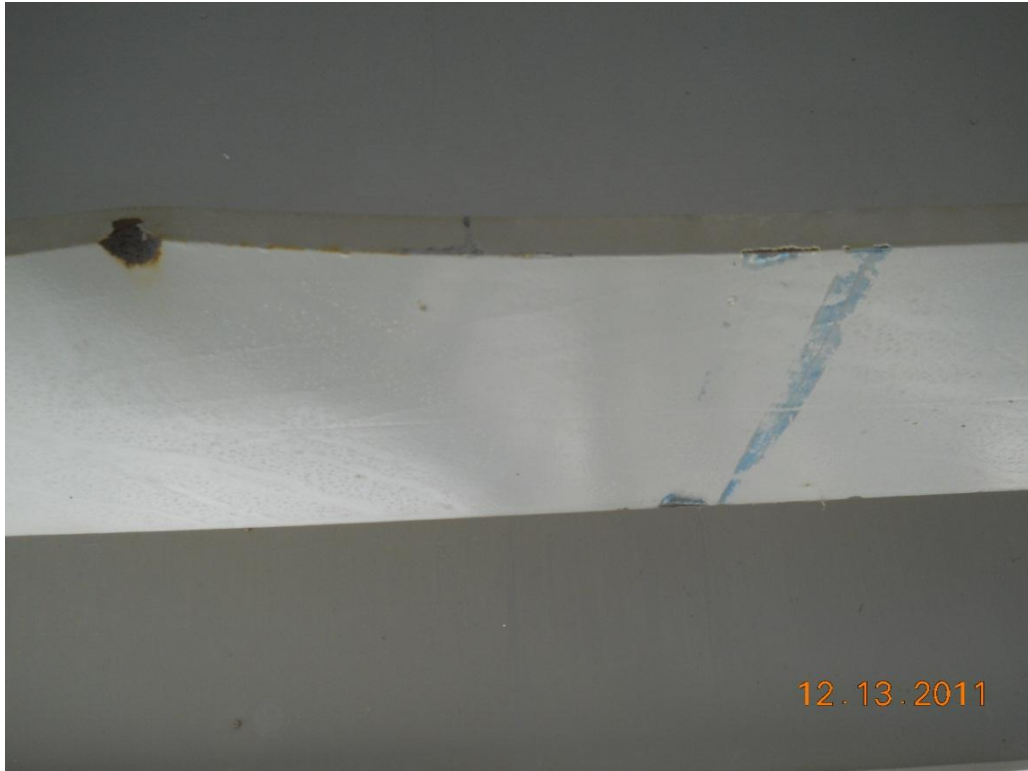
Photograph 125 - Span 1, girder 4, note impact damage
