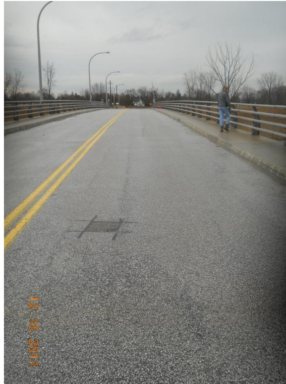
Photograph 17 - Span 3 asphalt wearing surface looking east, eastbound lane, note patch
