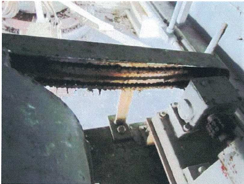
PHOTOGRAPH 23: CENTRE PIER SWING DRIVE POSITION CONTROLLER TRANSMISSION SHOWING LACK OF LUBRICATION AND CORROSION
