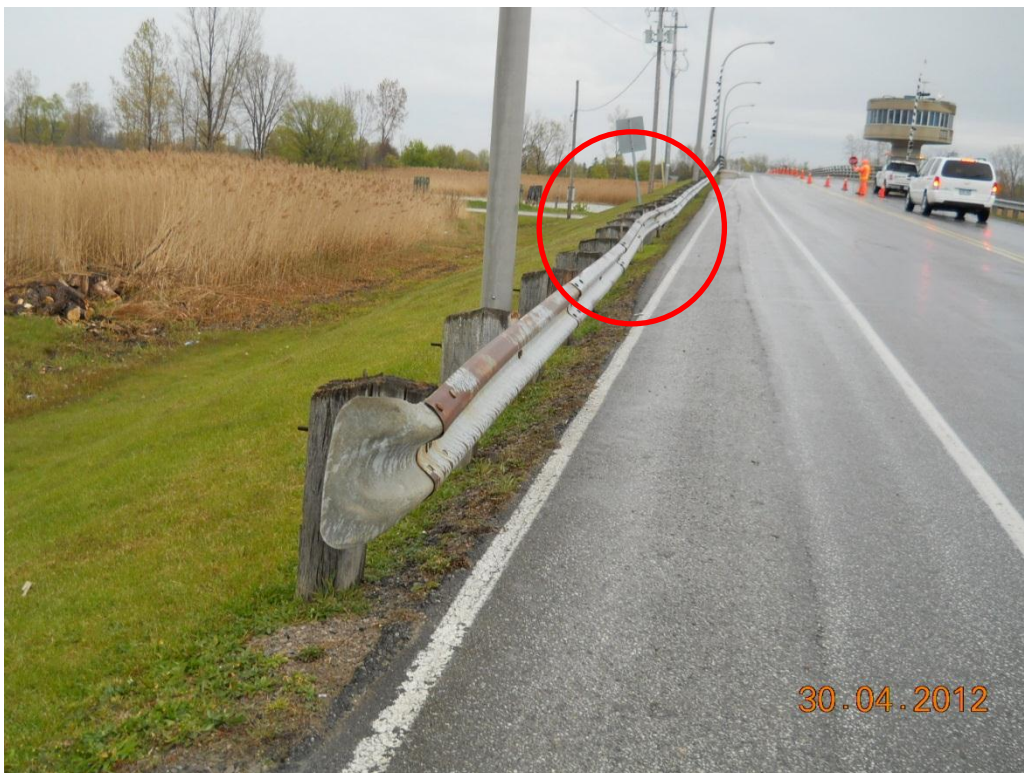
Photograph 142 - Northwest approach SBGR - Note deformation near mid length.
