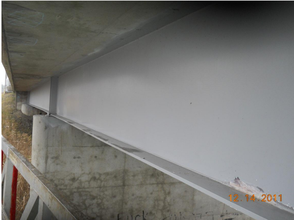
Photograph 93 - Span 5, north exterior soffit and girder 1, note coating failure on bottom of web
