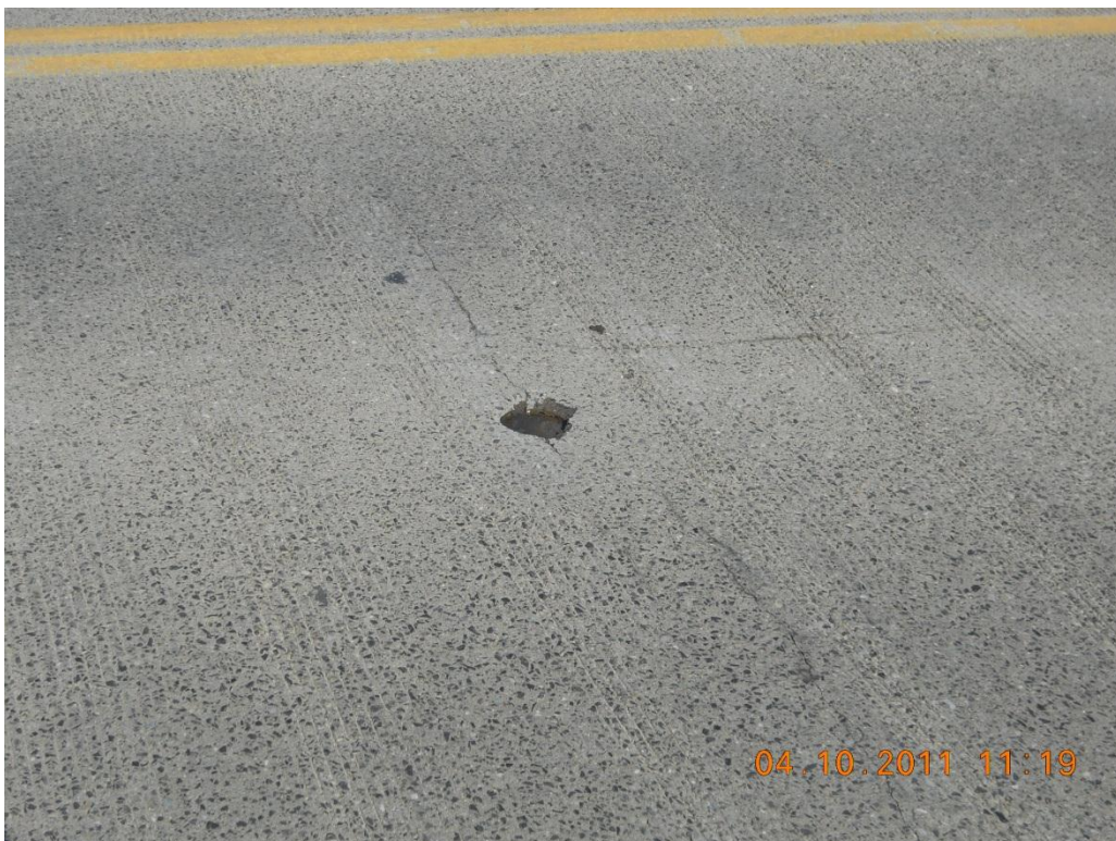
Photograph 22 - Span 2, note core hole and cracking
