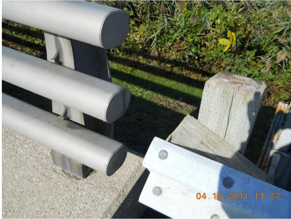
Photograph 139 – Typical guide rail at structure, note lack of connection between the guide rail and bridge barrier
