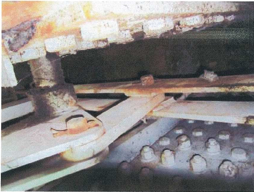
PHOTOGRAPH 3: WEDGE MECHANISM ON THE WEST REST PIER SHOWING LACK OF LUBRICATION AND CORROSION
