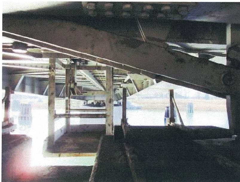
PHOTOGRAPH 32: WEST REST PIER MAINTENANCE PLATFORM SHOWING CORROSION
