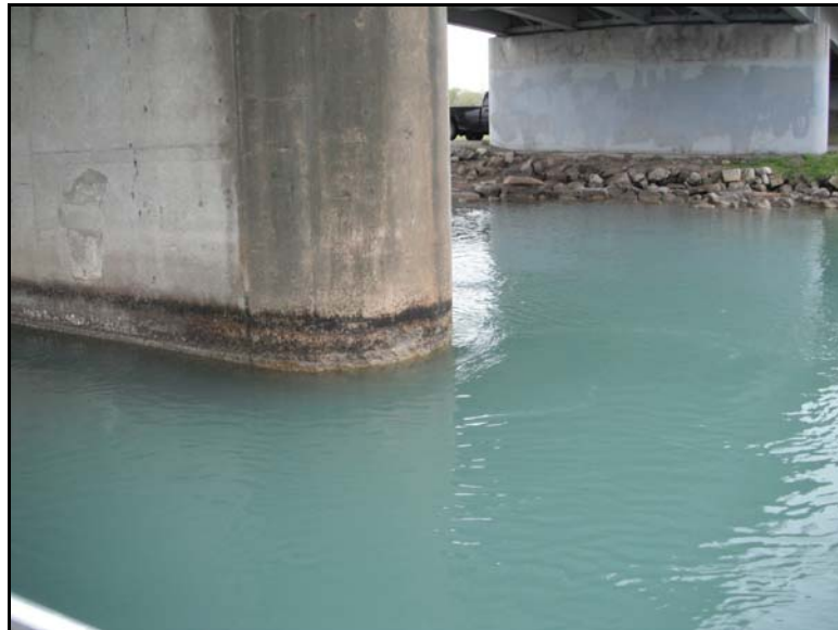
Figure 3: West Rest Pier, North Nose showing Spall at Water Line
