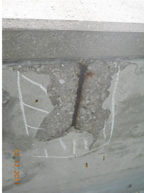
Photograph 91 - Soffit, span 1 south exterior, note delamination and exposed reinforcing steel
