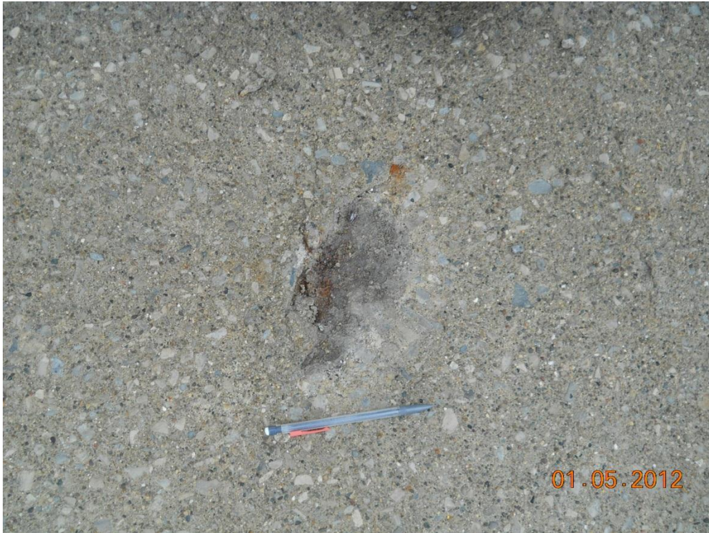
Photograph 145 - North sidewalk near west end of span 1 - Note spall
