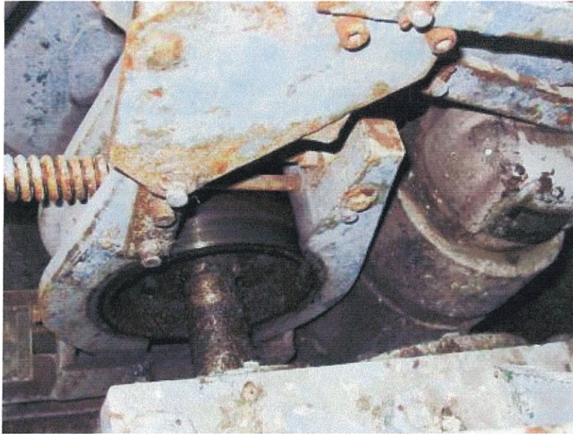
PHOTOGRAPH 29: EAST SIDE SWING DRIVE BRAKE HUB SHOWING CONTAMINATION WITH LUBRICANT
