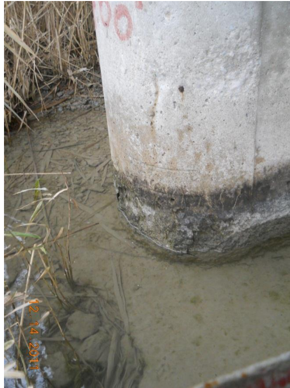
Photograph 53 - North end of east shore pier, note light concrete erosion at waterline
