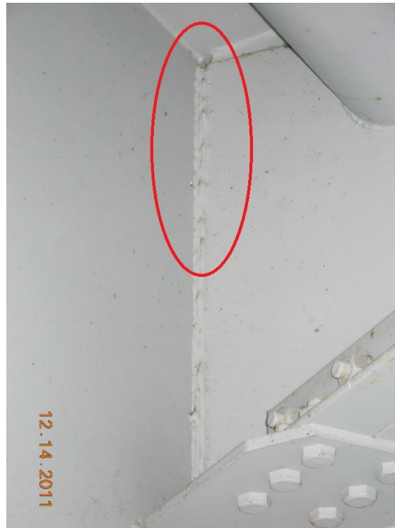
Photograph 115 - Span 3, girder 2 at fifth cross beam from pivot pier, note potential crack in vertical weld (limited access during inspection prevented confirmation of crack)
