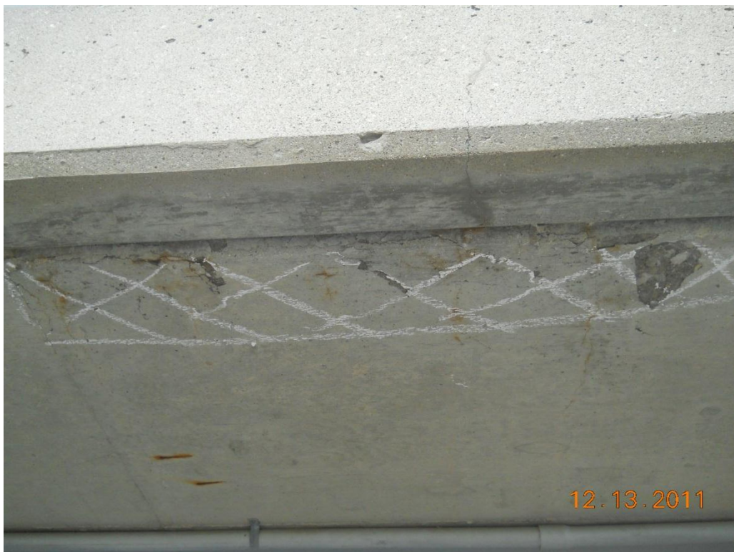
Photograph 90 - Soffit, span 1 south exterior, note delamination and spalling
