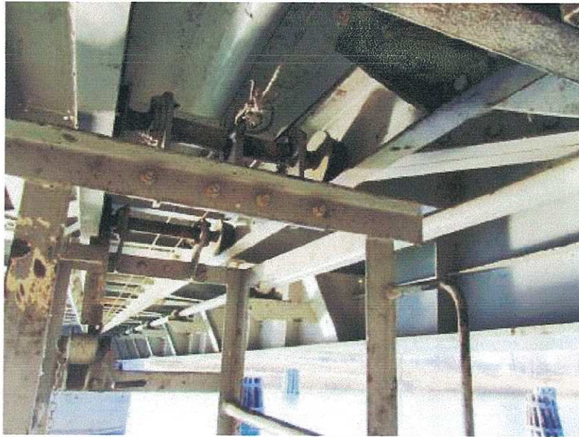
PHOTOGRAPH 11: INSPECTION CRADLE AND TRACK SHOWING LACK OF LUBRICATION AND CORROSION
