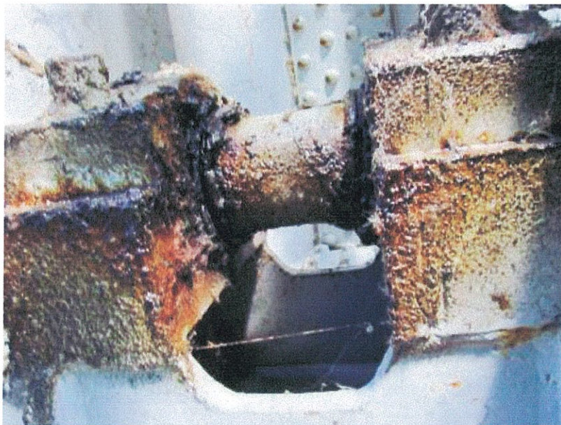
PHOTOGRAPH 10: SLEEVE BEARINGS SHOWING LACK OF LUBRICATION
