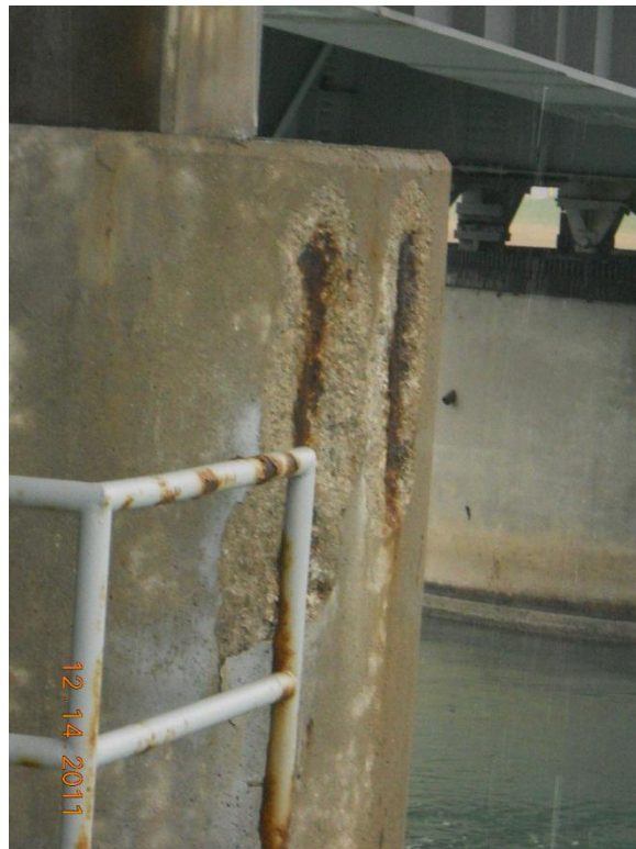
Photograph 56 - North face of east rest pier, note exposed corroded reinforcing steel bars
