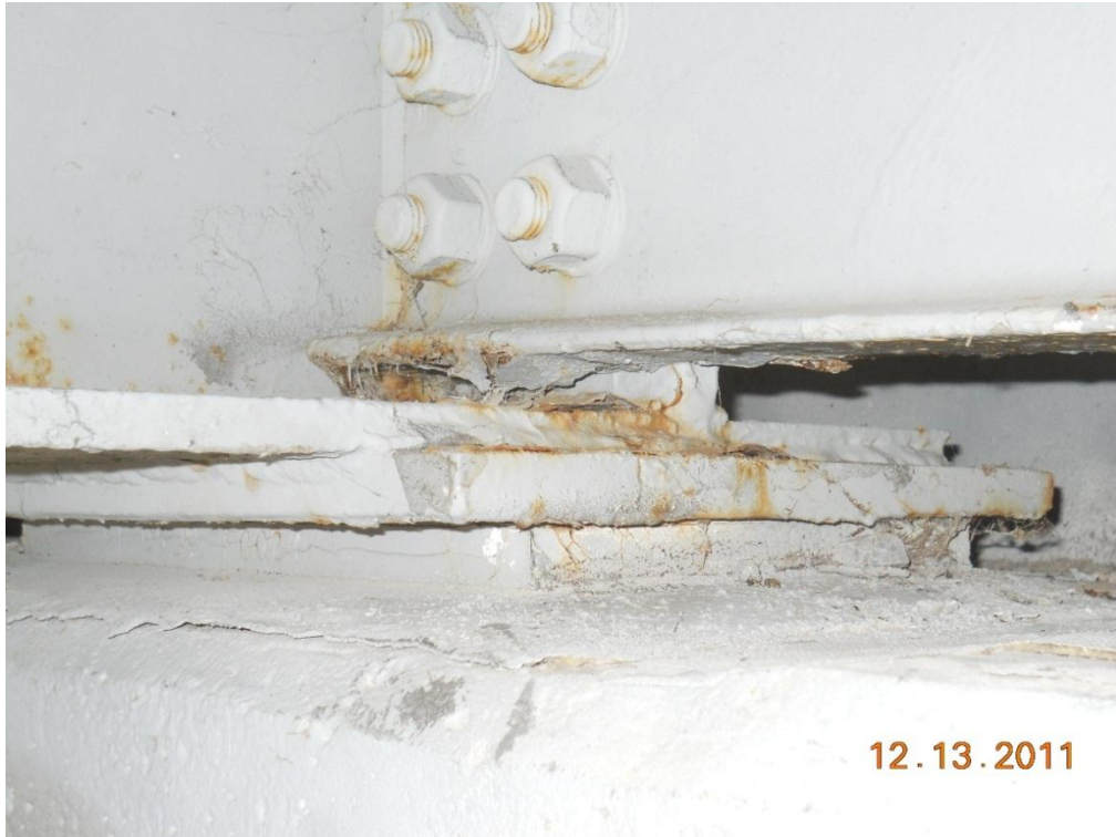
Photograph 81 - West abutment bearing second from north end, note typical coating breakdown
