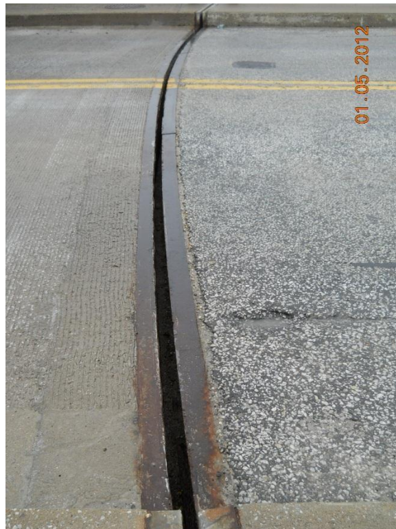
Photograph 148 - Joint over east rest pier looking south - Note corrosion of armouring angles.
