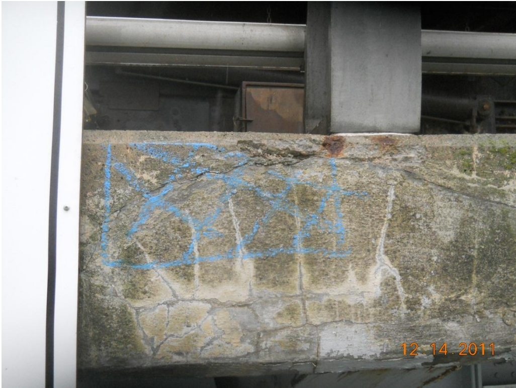
Photograph 85 - Fascia, span 4 north side, note delamination and cracking
