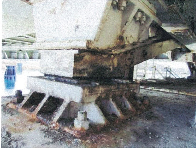
PHOTOGRAPH 5: SPAN WEDGE WITH CORRODED BASE PLATE ON THE SOUTH SIDE OF THE EAST REST PIER
