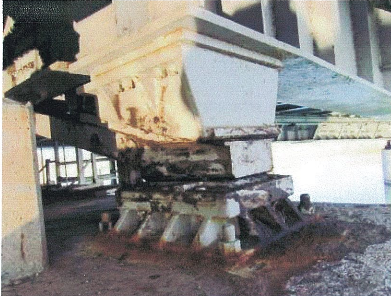
PHOTOGRAPH 1: SPAN WEDGE WITH CORRODED BASE PLATE ON THE SOUTH SIDE OF THE WEST REST PIER
