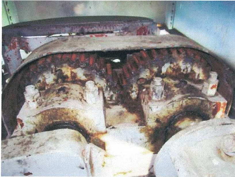
PHOTOGRAPH 19: CENTRE PIER SWING DRIVE SPUR GEARS SHOWING LACK OF LUBRICATION AND CORROSION
