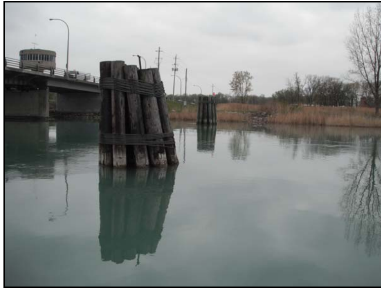
Figure 8: North Dolphin showing lean toward the bridge. Dolphin in the background shows only one band at the top and missing band above the waterline
