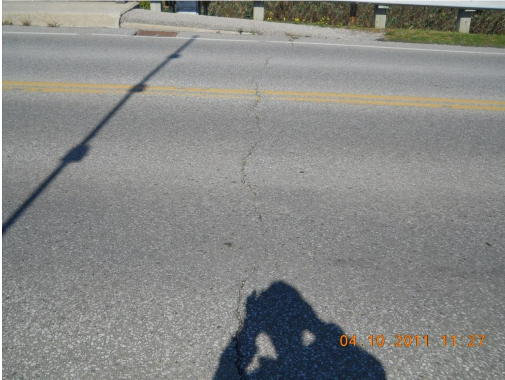
Photograph 11 - East approach slab wearing surface, note transverse crack
