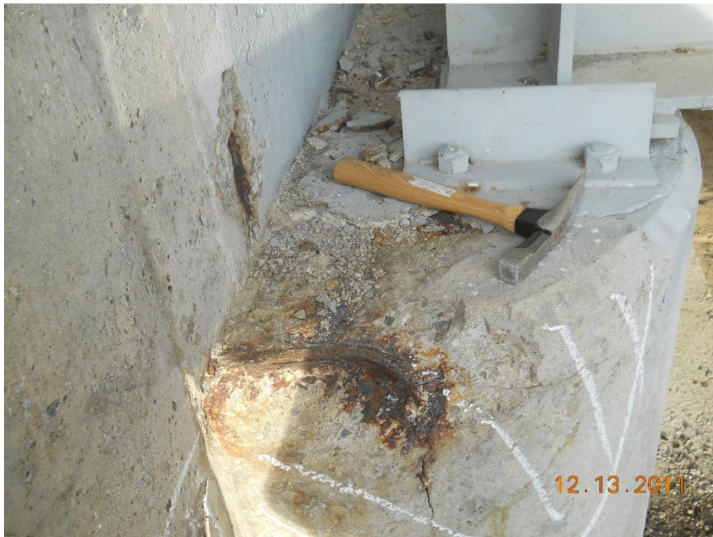
Photograph 50 - South end of west abutment bearing seat, note spalling and delamination
