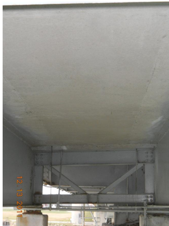
Photograph 84 - Soffit, span 5 looking west, typical condition
