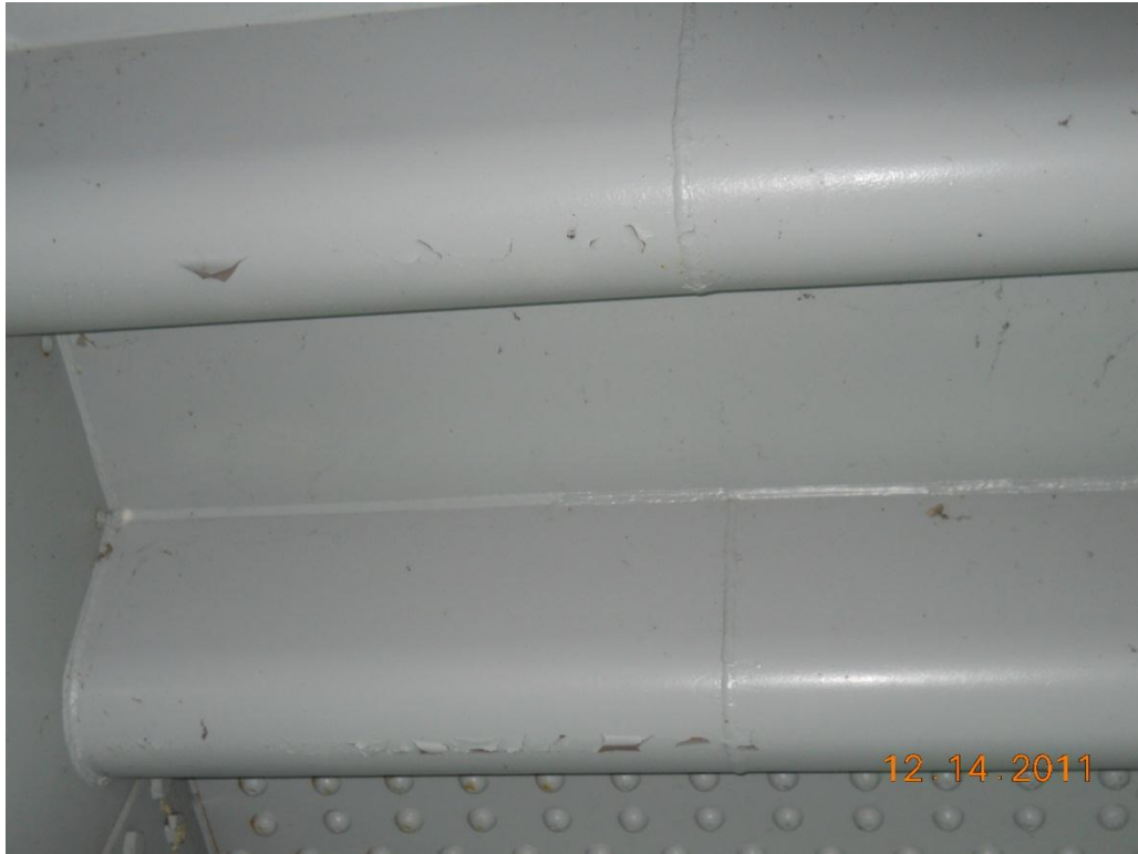
Photograph 109 - Soffit, span 3, note coating failure on bottom of troughs
