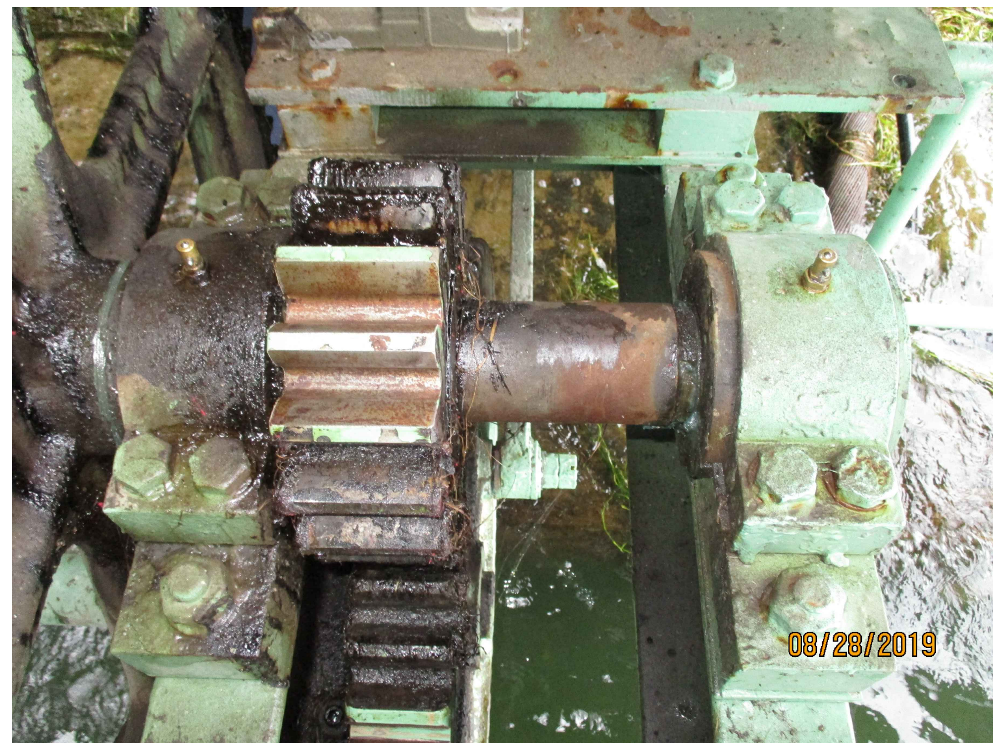
PHOTO OF CORRODED SPAN LOCK SHAFT
