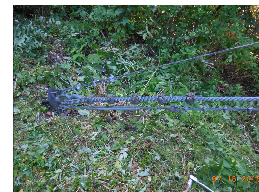
PHOTO 3: EXISTING CABLE TERMINATIONS, HARDWARE AND FITTINGS
