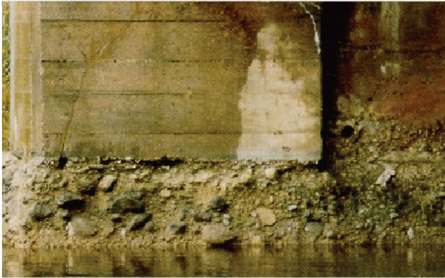
Figure 2.2.3 Very Severe Erosion of a Concrete Footing
