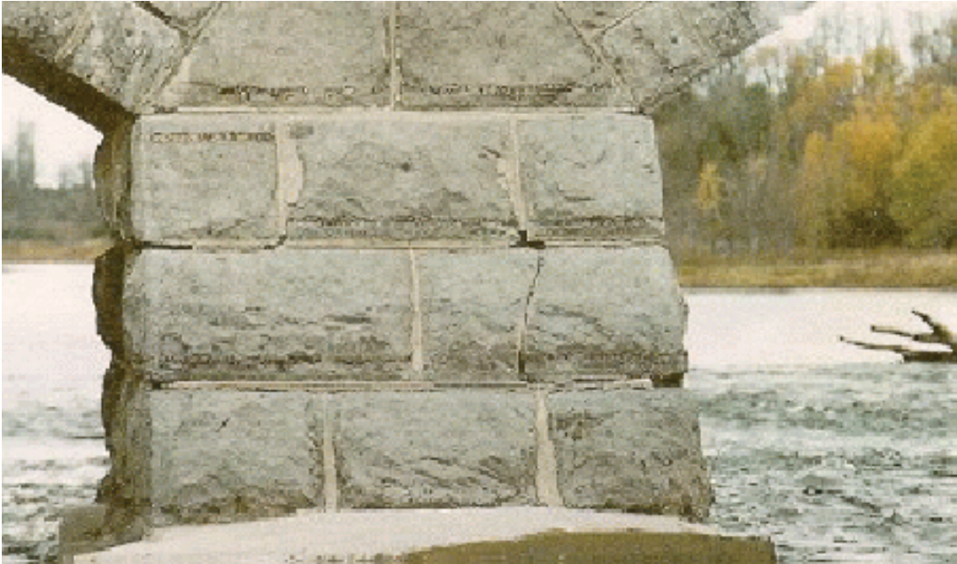
Figure 2.5.1 Wide Crack Through a Stone in a Masonry Pier
