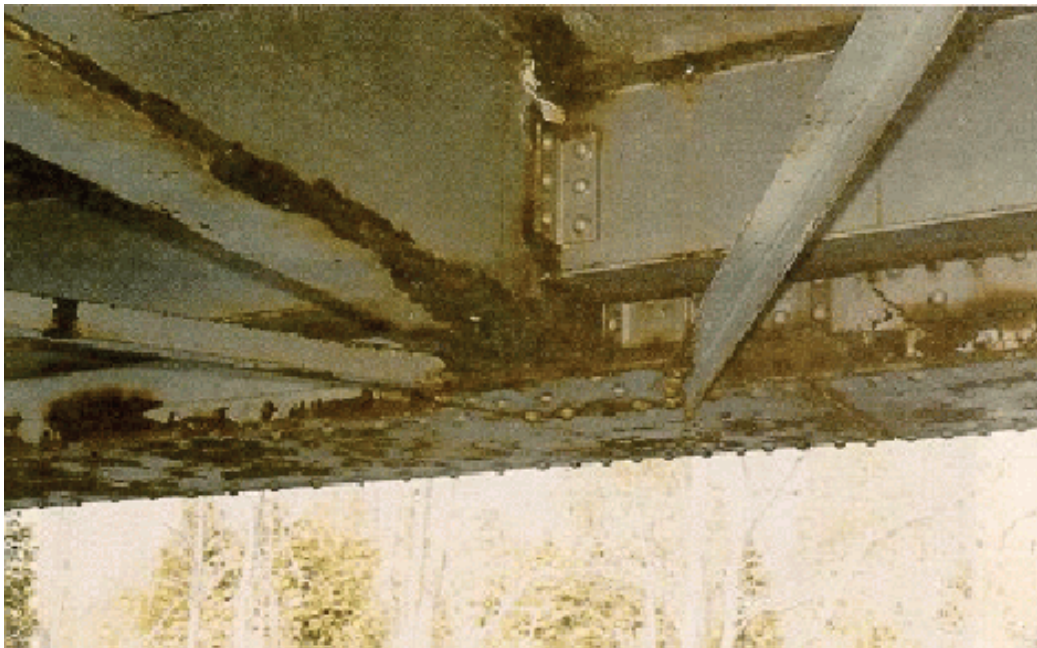
Figure 2.3.1 Medium Corrosion of Steel Beams
