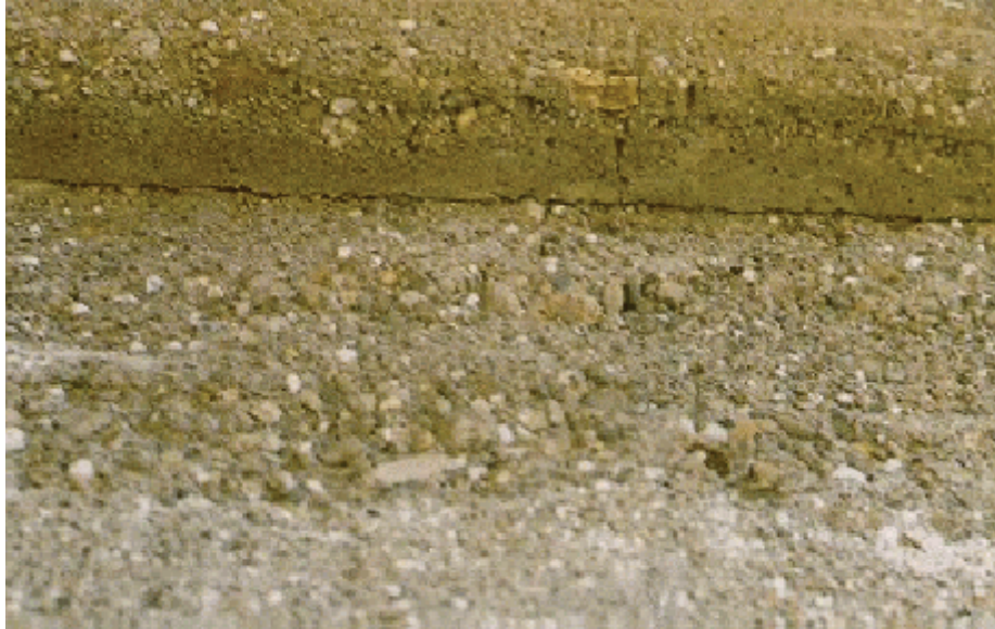
Figure 2.2.1 Severe Scaling in a Concrete Deck and Curb
