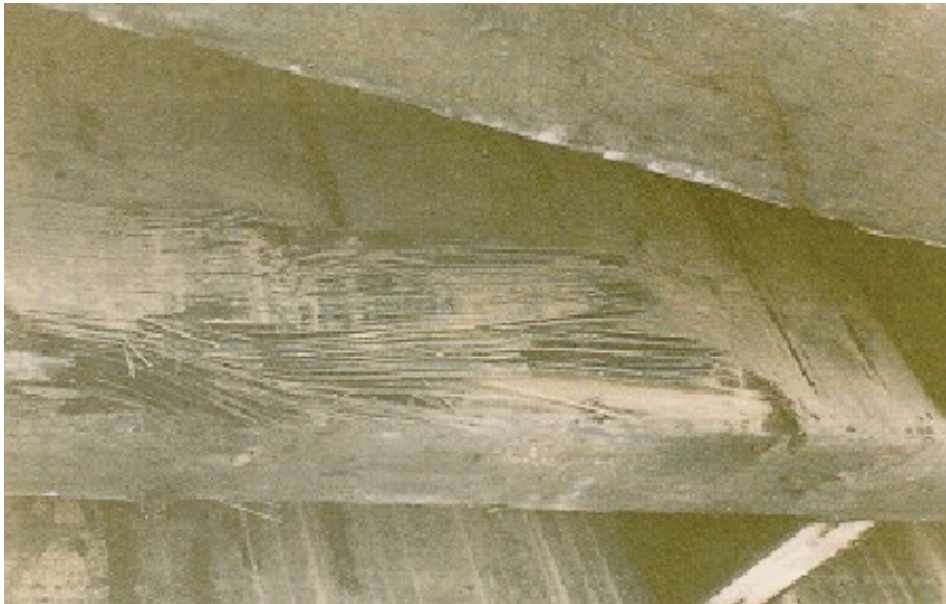
Figure 2.4.5 Very Severe Crushing and Splintering of Wood Due to Vehicular Impact
