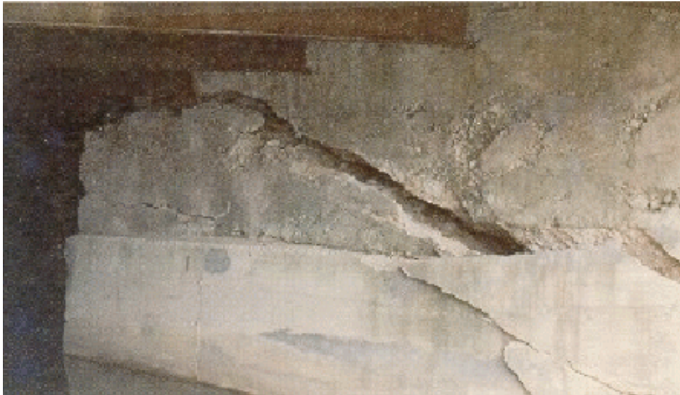
Figure 2.2.7(d) Very Wide Movement Crack in an Abutment
