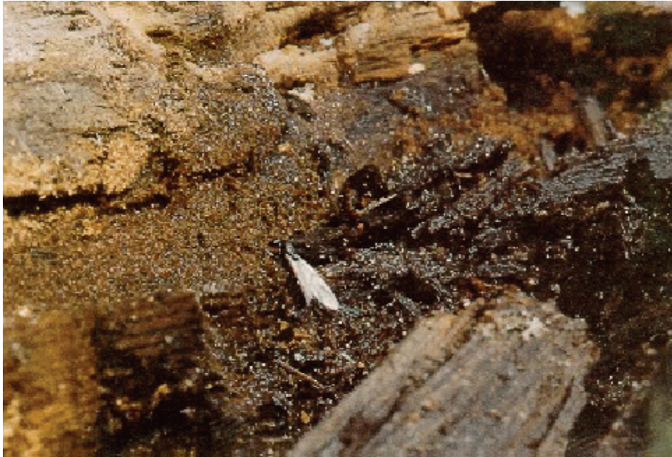
Figure 2.4.3(b) Very Severe Insect Damage in Wood
