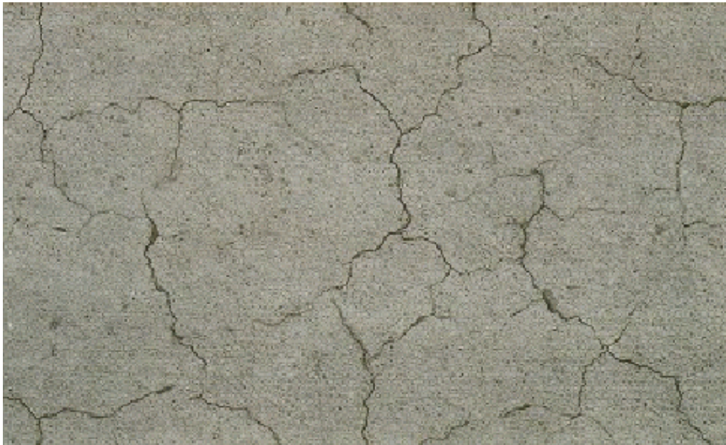
Figure 2.2.8 Severe Alkali-Aggregate Reaction
