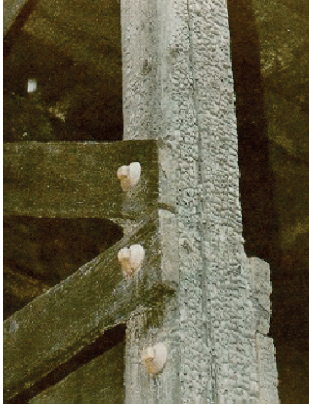
Figure 2.4.6(a) Medium Fire Damage on Wood
