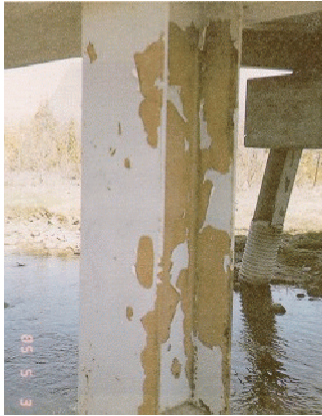
Figure 2.8.2(c) Intercoat Delamination
