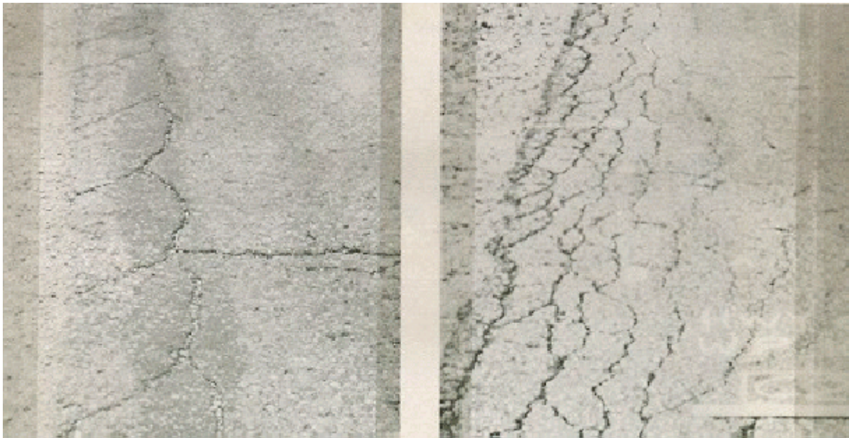
Figure 2.7.1(e) Medium Progressive Edge Cracks
