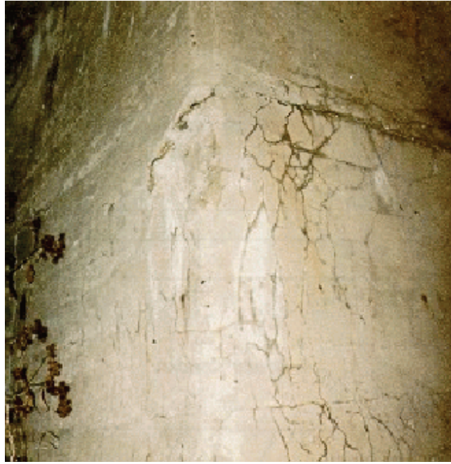
Figure 2.2.7(c) Medium Pattern Cracks in an Abutment
