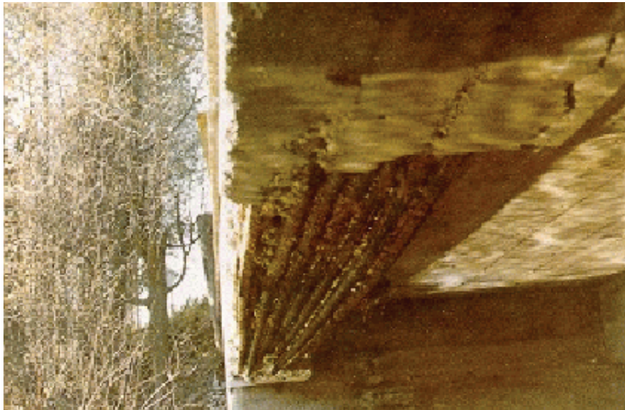
Figure 2.2.5 Very Severe Spalling and Delamination in Concrete Beams
