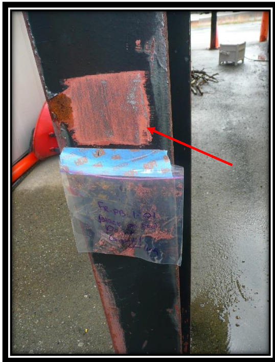
Photograph 1: Black paint with red primer caulking observed on the posts and frames of the carport on the north side of the Custom's Building with a lead content of 6,400 ppm.
