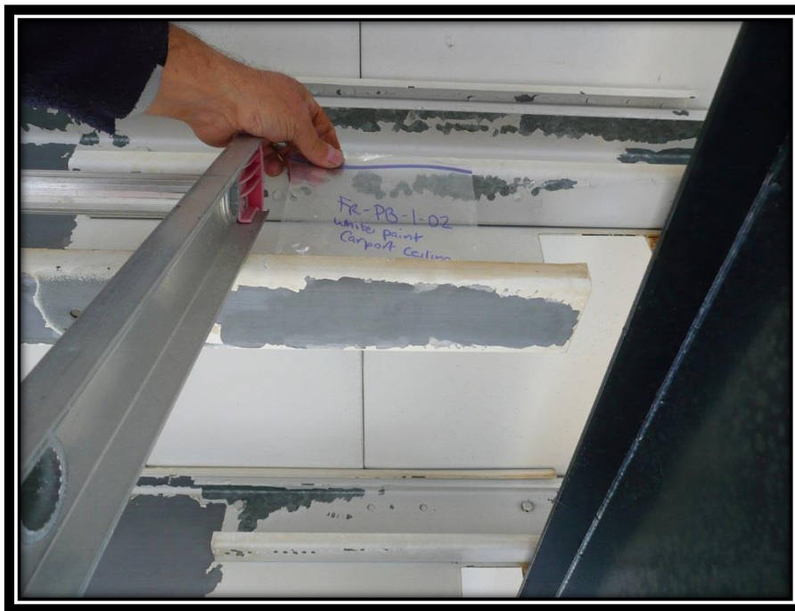
Photograph 2: White and cream paint observed on the frames and ceiling of the carport on the north side of the Custom's Building with a lead content of 1,800 ppm.
