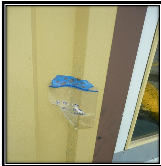
Photograph 4: Yellow paint observed on the metal panels on the south exterior of the Custom's Building with a lead content of 10,000 ppm.
