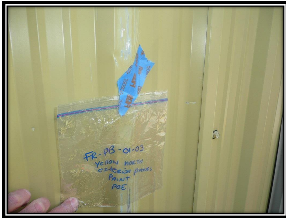
Photograph 3: Yellow paint observed on the metal panels on the north exterior of the Custom's Building with a lead content of 13,000 ppm.
