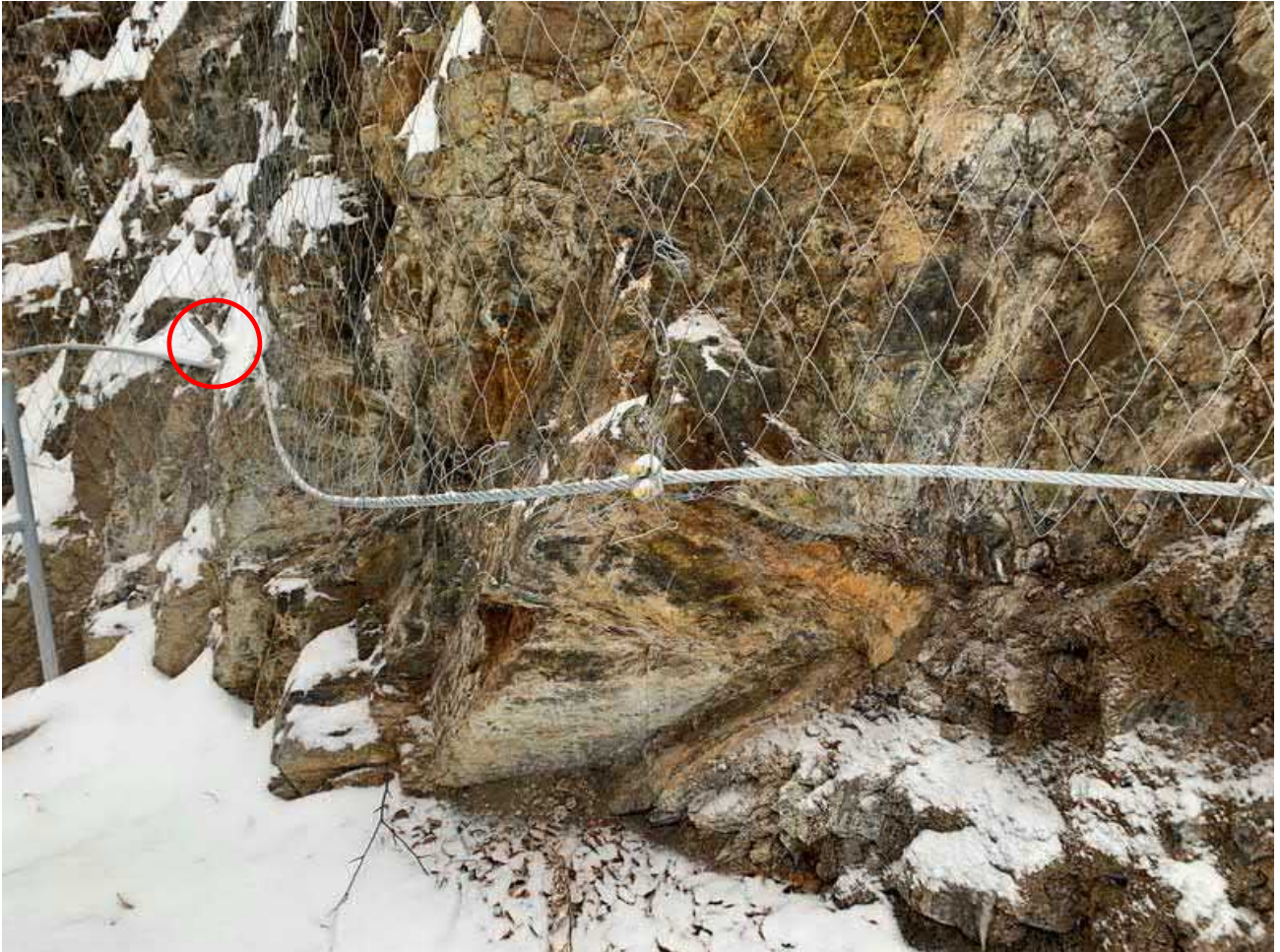
Photograph 7: View looking along base of mesh where it is above the top of the valve house. Red circle indicates a rock anchor used to pin the mesh to the slope.
