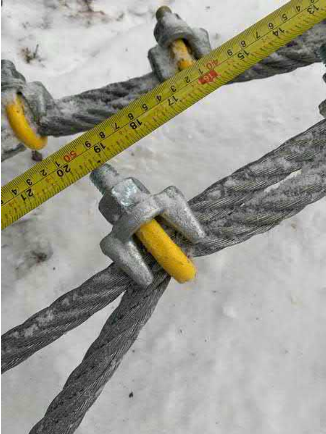
Photograph 2: Close view of clamp on an End Cable.
