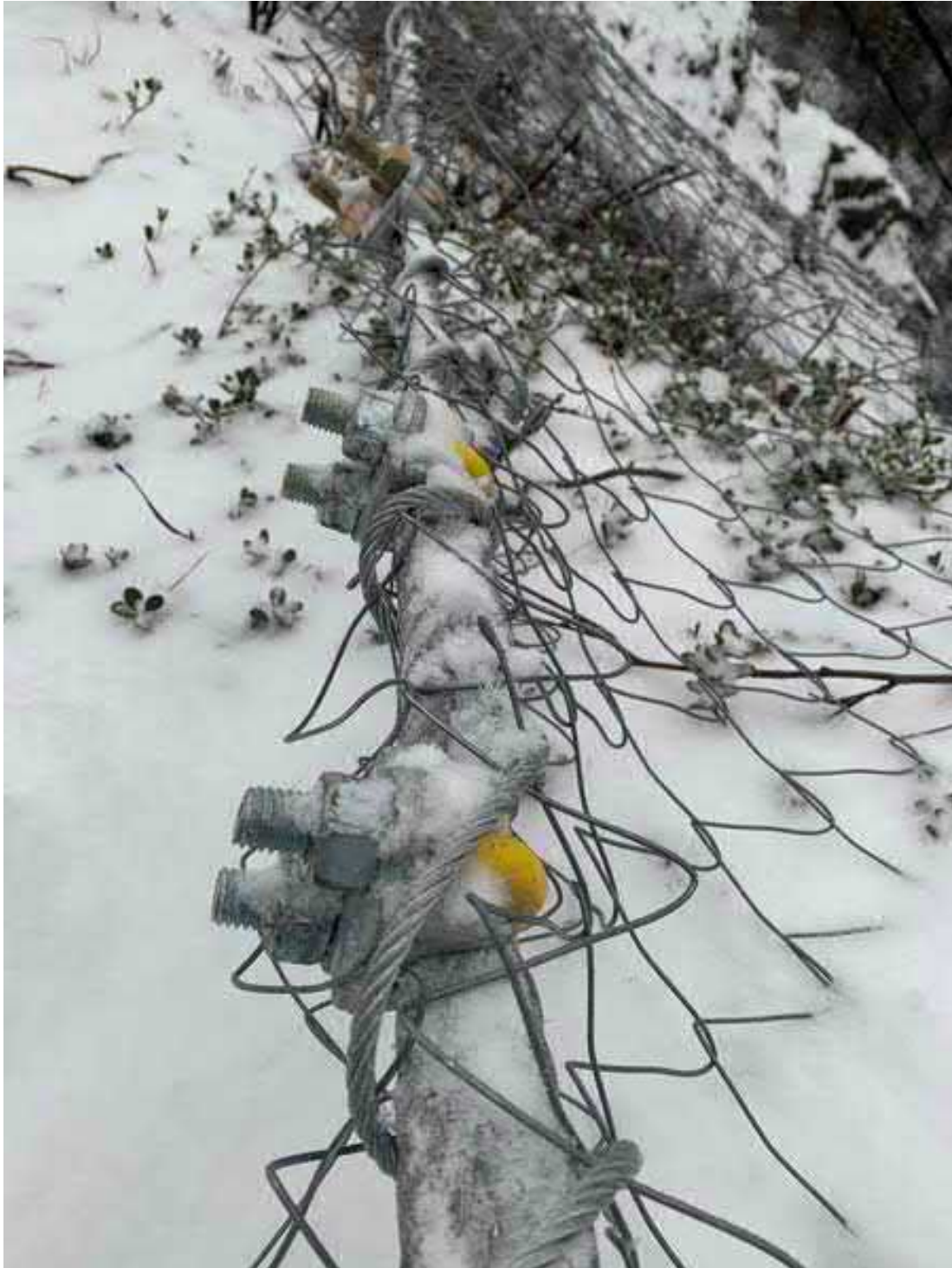
Photograph 3: View looking along Suspension Cable showing arrangement of wire mesh, Lacing Cable, and Cable Clamps.
